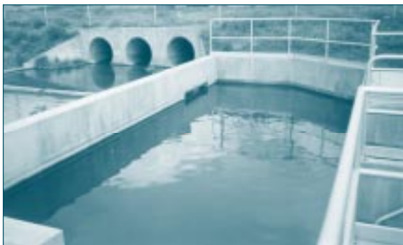
The concrete diversion channel diverts low flows from the drainage channel. The trash collection chamber traps large debris.
