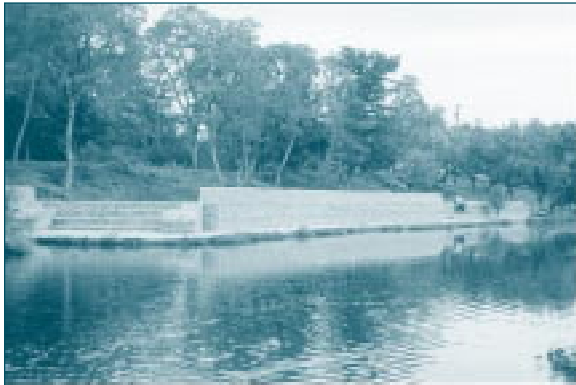
The gabion structure between the wet pond and the river, near completion.
