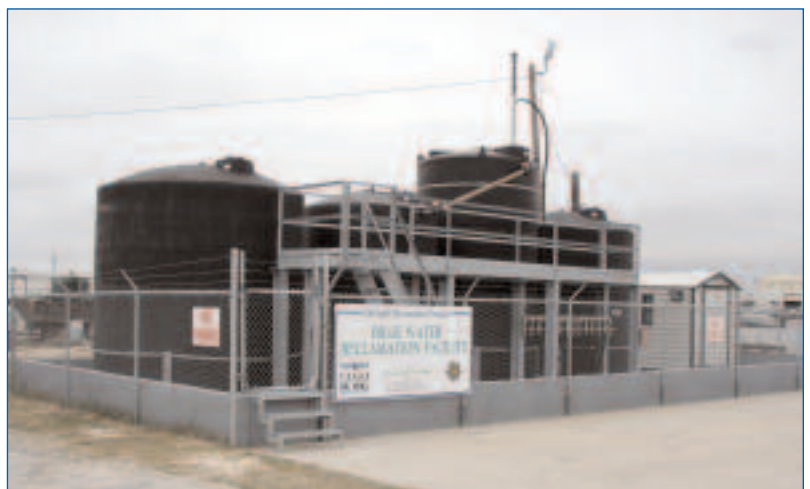
This new bilge water reclamation facility at Rockport is the fourth built since Land Commissioner Jerry Patterson took office in 2003. Oil collected at the facility will be recycled, and bilge water will either be cleaned or hauled away for proper disposal.
