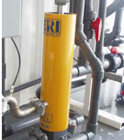
Figure 4-3.2.4-4 Pressure Exchanger Installation (MacHarg)
