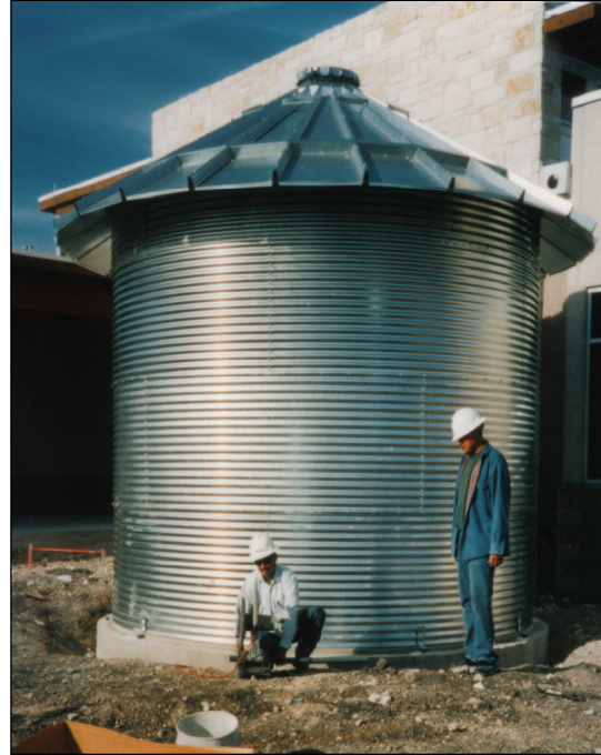
Four lined, galvanized steel tanks will capture water for irrigation of native and adapted plants.
