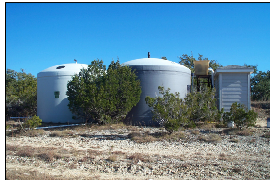
Figure 2-5. Two 10,000-gallon fiberglass tanks
