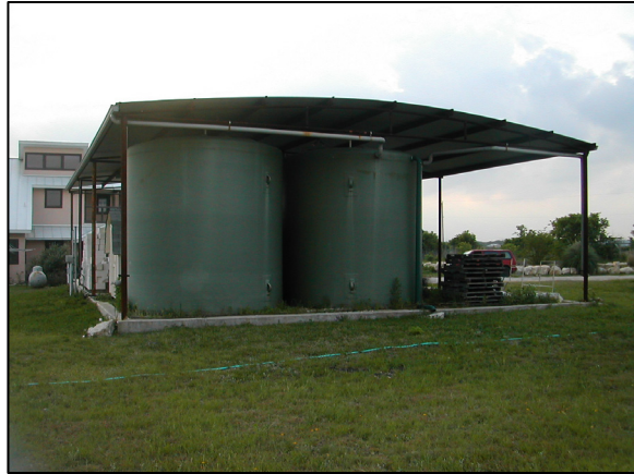
Two 10,000-gallon cisterns collect rainwater at the Pomerening/Dunford residence in Bexar County.
