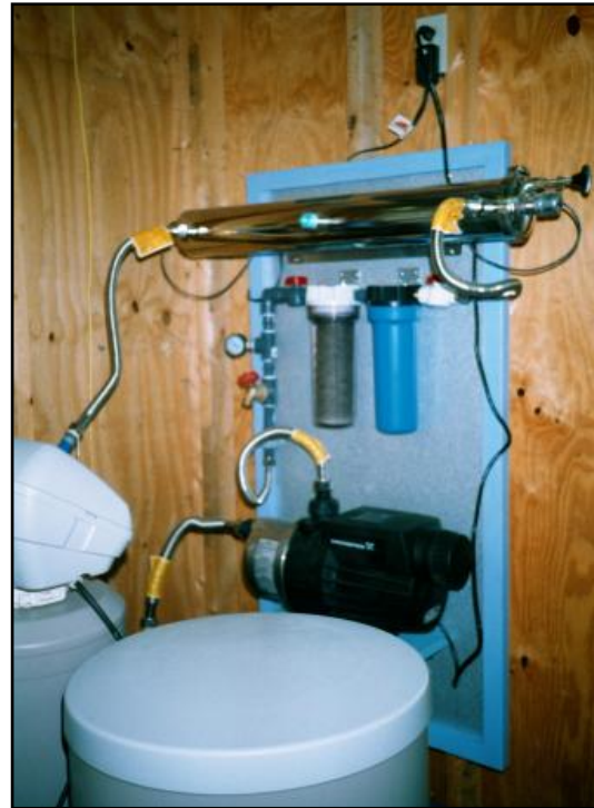
Figure 2-12. Typical treatment installation of an on-demand pump, 5-micron fiber filter, 3-micron activated charcoal filter, and an ultraviolet lamp (top).
