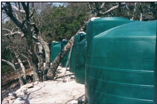
Figure 2-6. Low-profile 5,000-gallon polypropylene tanks
