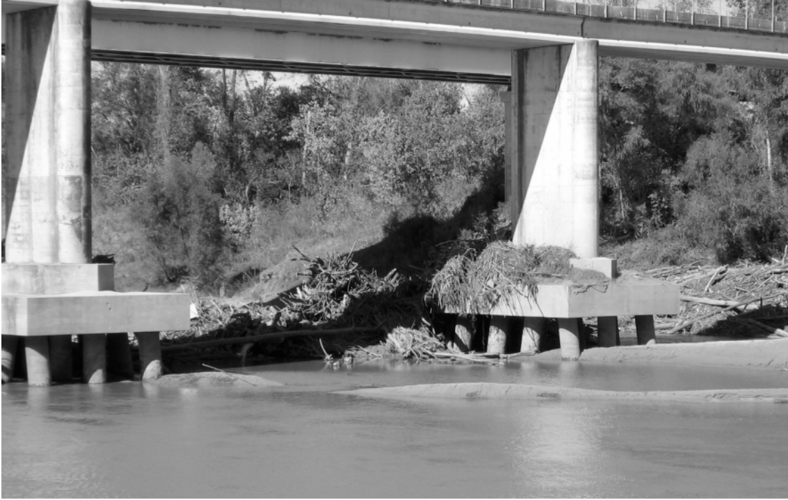
Figure 14. Concrete pads originally flush with the channel bed now exposed at FM1093 near Simonton.
