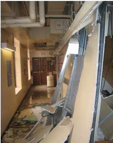
Figure 2 - Hallway Outside Laboratory Showing Explosion Damage
