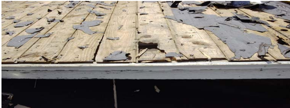
Older Deteriorated and Damaged Deck (Board Decking)
