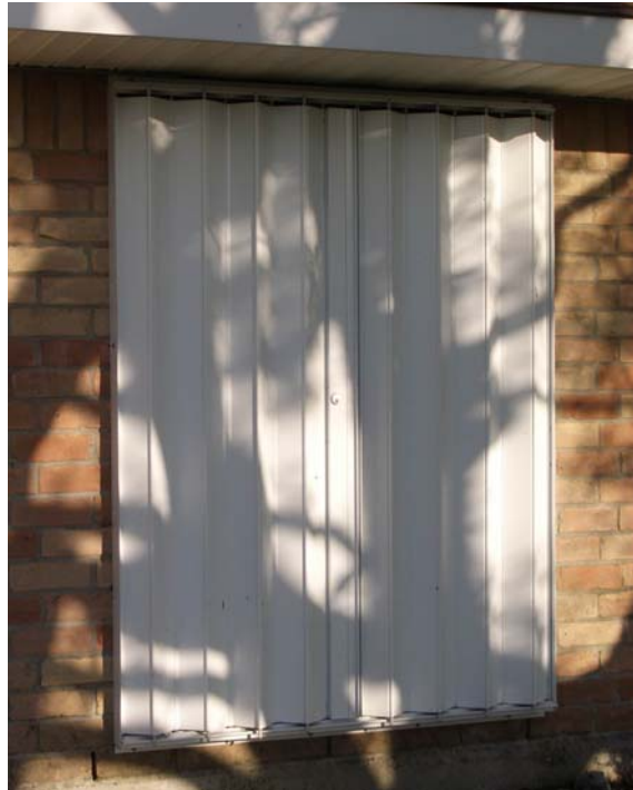
Impact Resistant Shutter System Installed Over a Window Opening
