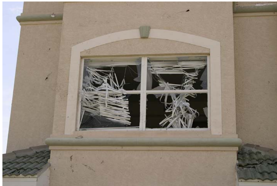
Window Glass Broken from Windborne Debris
