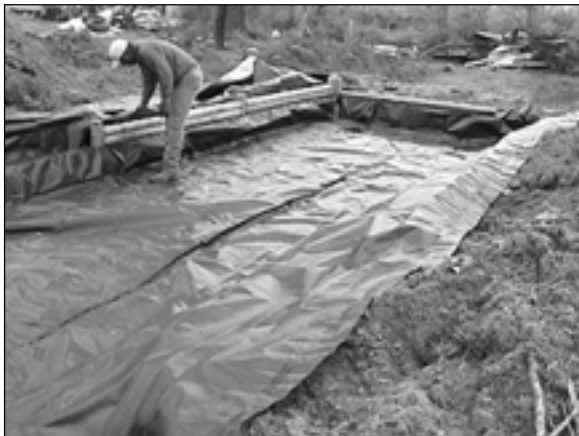
Construction of a lined, single-cell wetland at one of the project sites.
