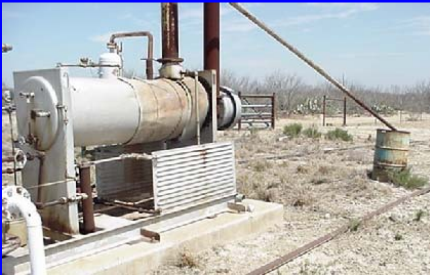
Glycol Dehydrator at a Compressor Station
