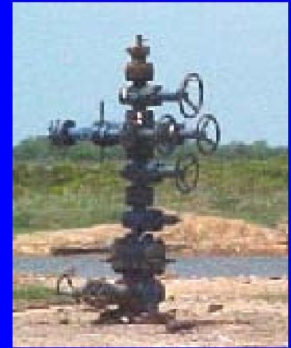
Gas Well Head
