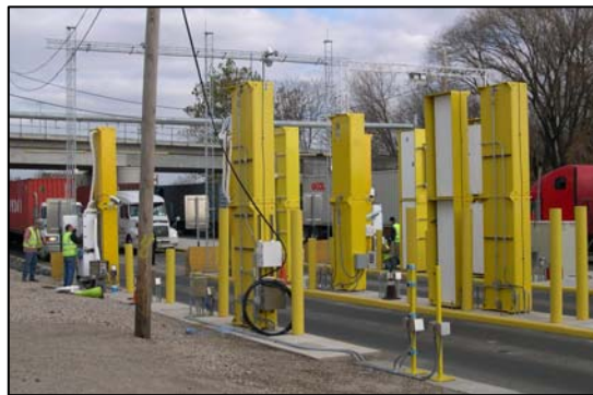
Advanced Spectroscopic Portals are installed at the New York Container Terminal for initial operational testing.
