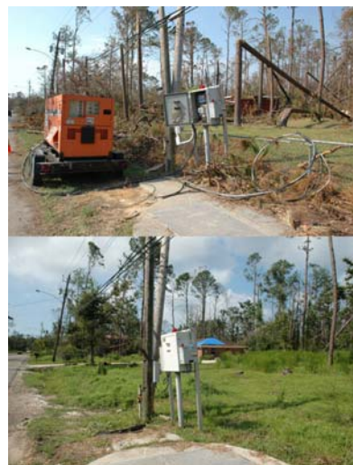
Waveland, Miss., September 9, 2005 and August 10, 2006 -- Before (top) power was restored it was necessary to use portable generators to create electricity in Waveland. Work to restore electricity after Hurricane Katrina was a top priority.
