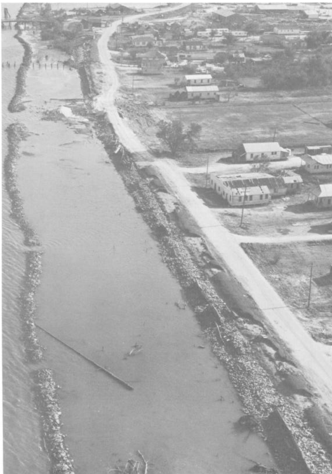
Figure 52. Erosion of Mississippi River levee at Venice, La.
