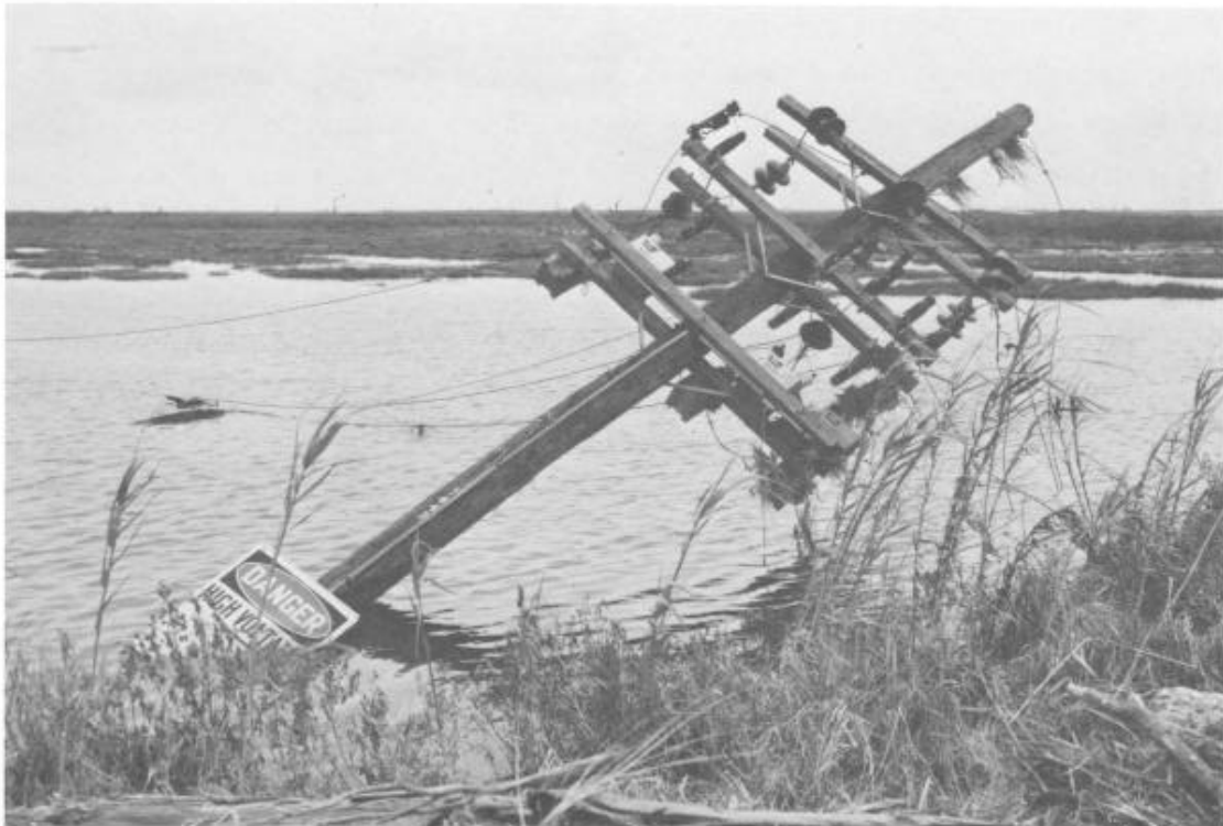
Figure 44. Power lines in some 20 parishes were blown down by the hurricane winds
