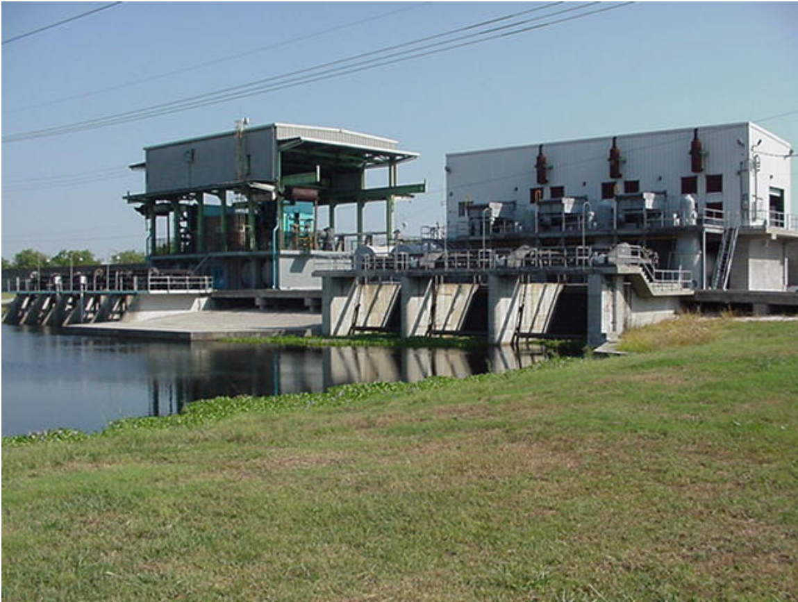
FORTIFICATION PUMPING STATION #1 On Left JEAN LAFITTE PUMPING STATION #6 On Right
