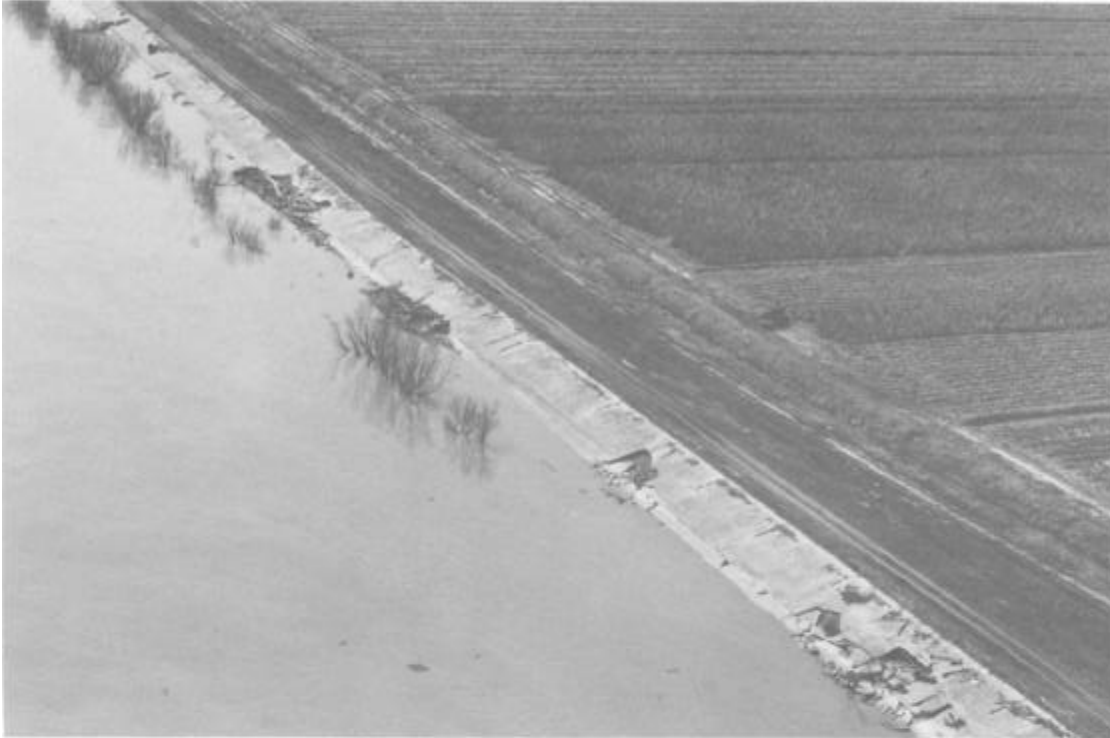
Figure 56. Damage to Mississippi River levee upper bank paving
