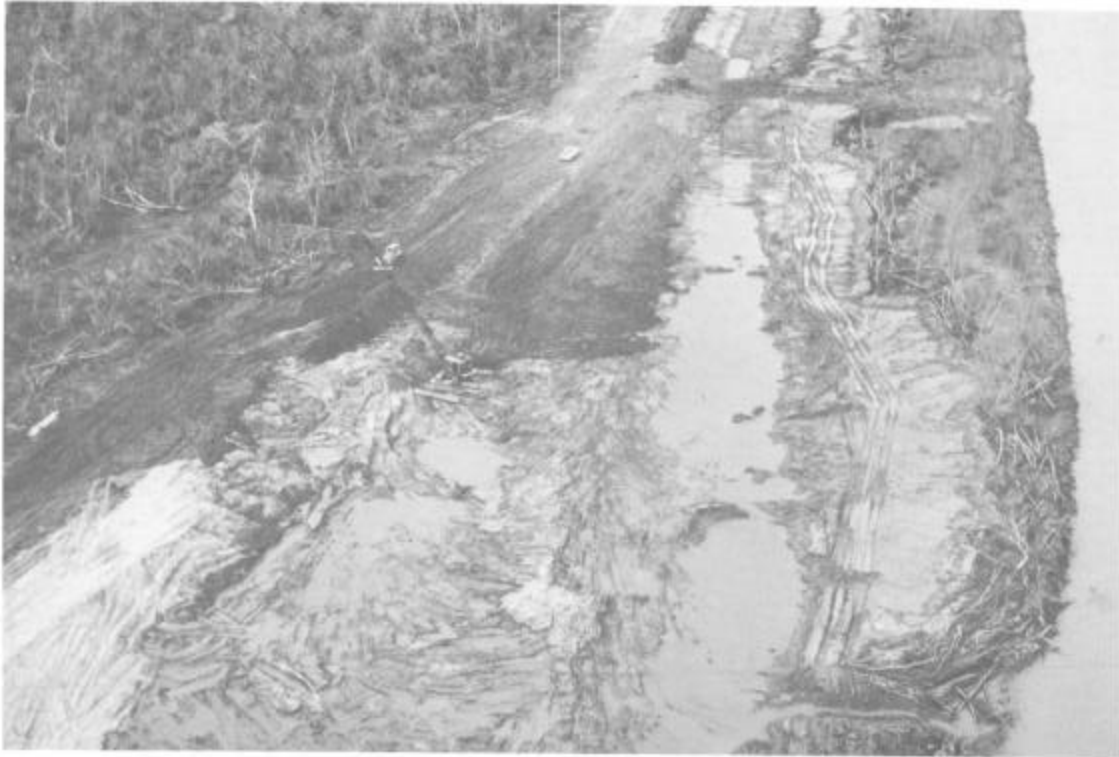
Figure 53. Repair of main line Mississippi River levee on the west bank in Plaquemines Parish
