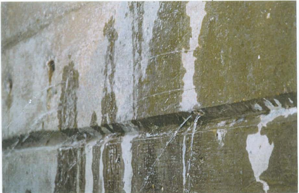
PHOTO NO. 4 – PROTECTED SIDE (NORTH FACE) OF EAST GATE BAY WALL OPPOSITE COUNTERWEIGHT RECESS WITH WATER SQUIRTING OUT.
