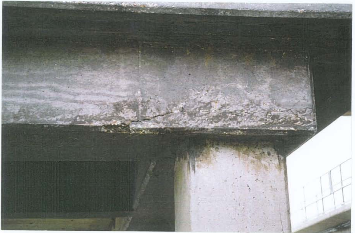
PHOTO NO. 15 – CRACK IN WEST FACE OF UPPER DECK PERIMETER SUPPORT BEAM AT SOUTH WEST CORNER OF PUMP PLATFORM.
