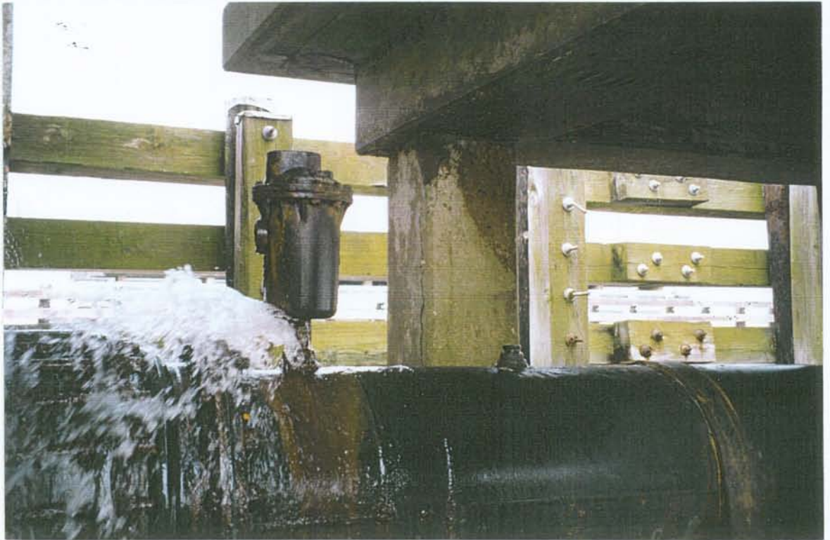
PHOTO NO. 8 – LOOKING WNW AT CRACKS IN SOUTH AND EAST FACES OF PUMP PLATFORM PILE NO. 3.
