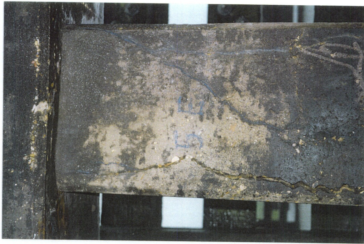
PHOTO NO. 28 - PILE NO. 5, EAST FACE, UPPER PORTION OF PILE. CRACK AT SOUTHEAST CORNER OPEN 1/4 INCH ±.
