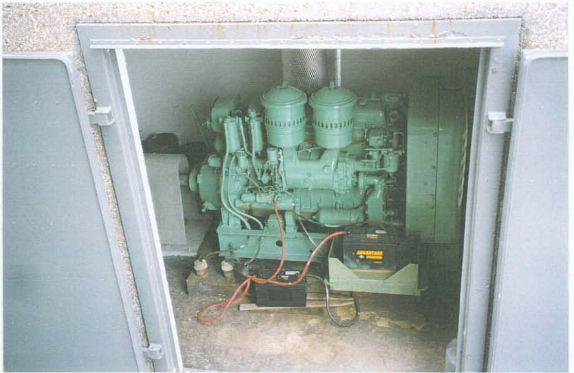
PHOTO NO. 28 – ENGINE FOR GATE RECESS FLUSHING SYSTEM PUMP.
