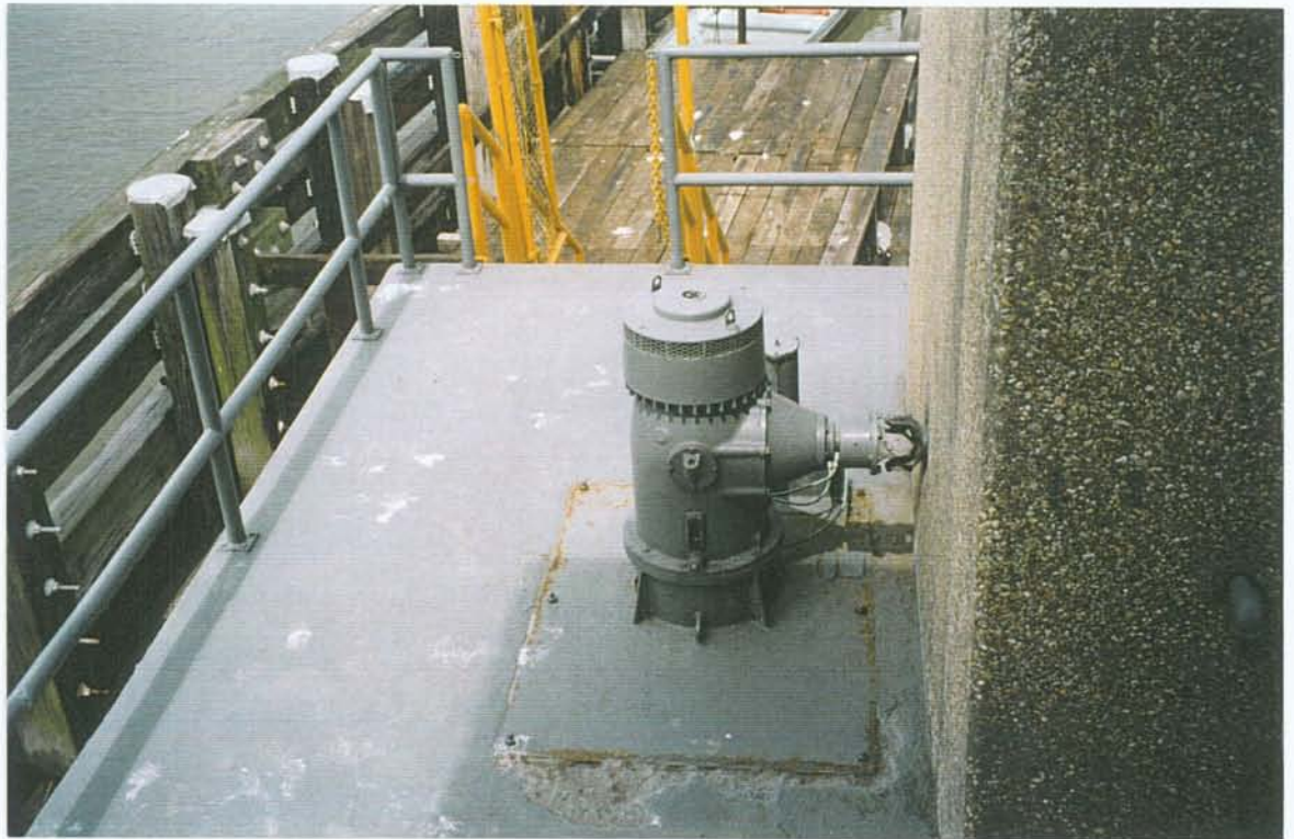
PHOTO NO. 6 – RIGHT ANGLE PUMP DRIVE.
