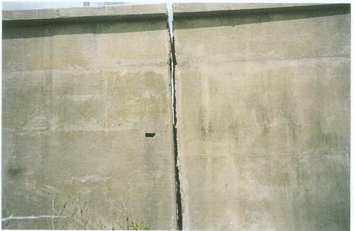
PHOTO NO. 2 – FLOODSIDE VIEW OF WEST "T" WALL AT JOINT BETWEEN MONOLITHS T-3L AND T-4L. NOTE OPEN JOINT AND TORN WATER STOP.
