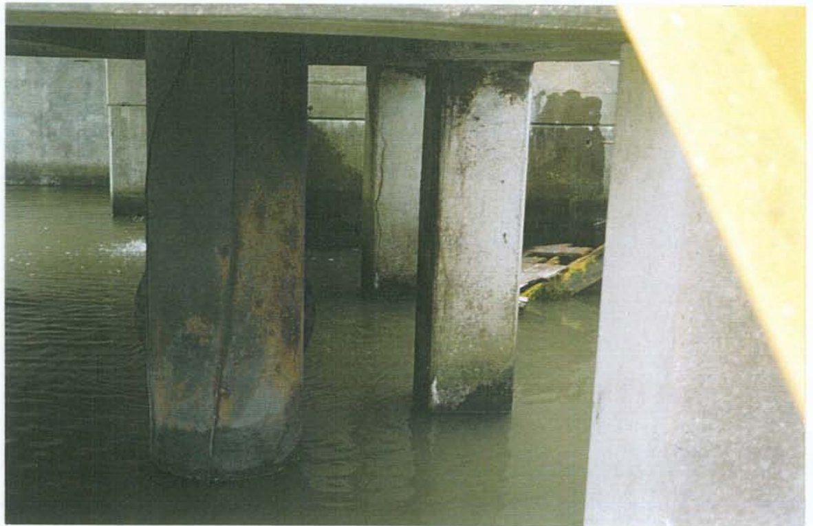
PHOTO NO. 9 – LOOKING SOUTH AT CRACKS IN NORTH FACES OF PUMP PLATFORM PILE NOS. 3 (BACKGROUND) AND 5 (FOREGROUND)
