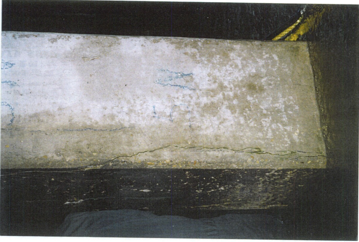
PHOTO NO. 22 - PILE NO. 5 NORTH FACE, LOWER PORTION OF PILE. CONTINUATION OF CRACK SHOWN IN PHOTO NO. 21 AND CRACK AT NORTHEAST CORNER OF PILE.
