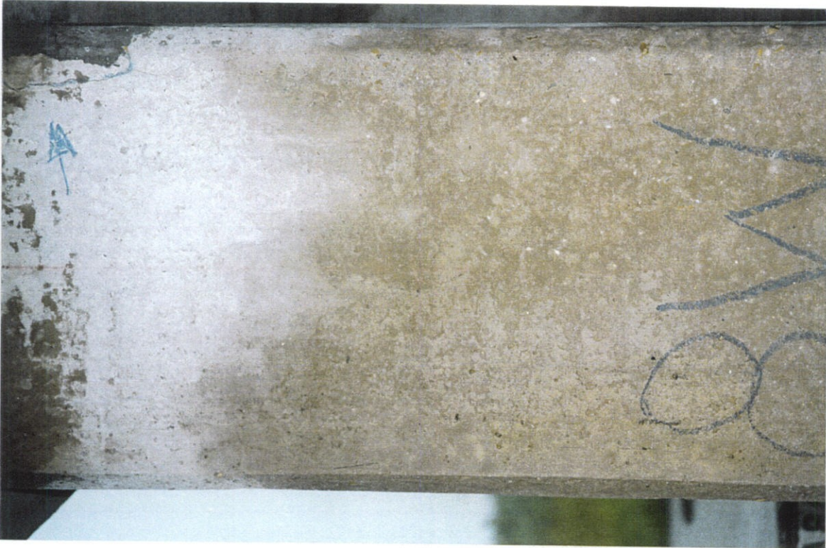
PHOTO NO. 38 - PILE NO. 8, WEST FACE. UPPER PORTION OF PILE. HAIRLINE CRACK AT TOP OF PILE (ARROW). NO OTHER CRACKS OBSERVED ON THIS PILE.
