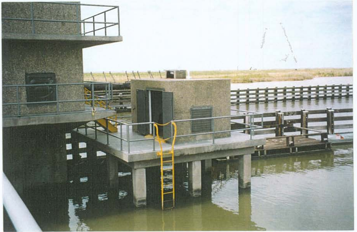
PHOTO NO. 5 – PUMPHOUSE AND PUMP PLATFORM.
