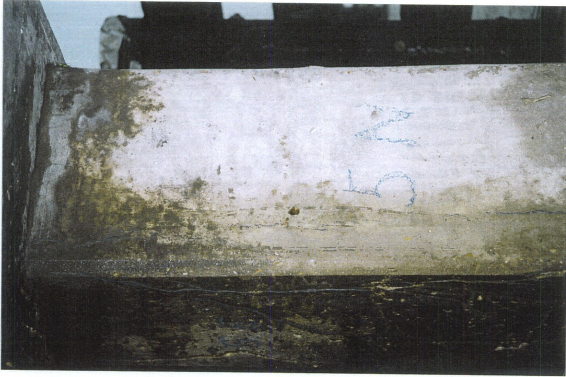
PHOTO NO. 21 - PILE NO. 5, NORTH FACE, UPPER PORTION OF PILE. PATCH AT TOP OF PILE. VERTICAL CRACKS ON LEFT SIDE.
