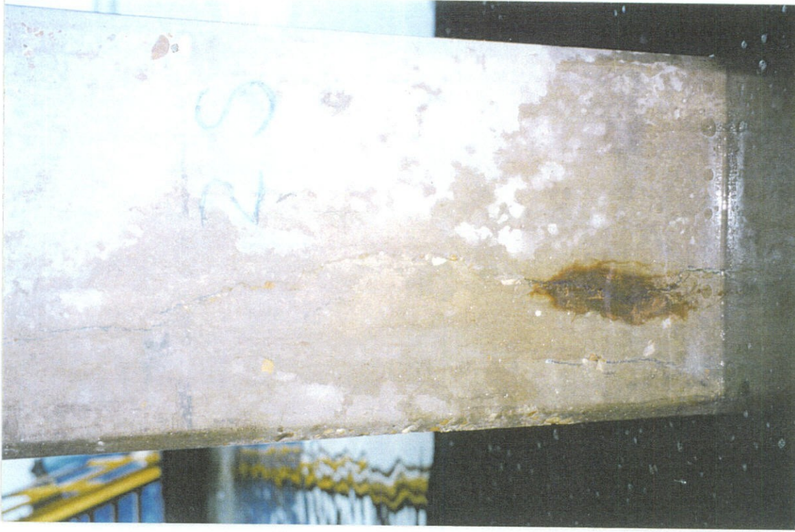
PHOTO NO. 4 - PILE NO. 2, SOUTH FACE. CONTINUATION OF CRACK SHOWN IN PHOTO NO. 3 AND ADDITIONAL CRACK.
