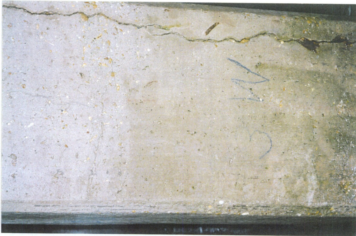
PHOTO NO. 11 - PILE NO. 3, WEST FACE. LOWER PORTION OF PILE. CONTINUATION OF OPEN CRACK SHOWN IN PHOTO NOS. 9 AND 10.
