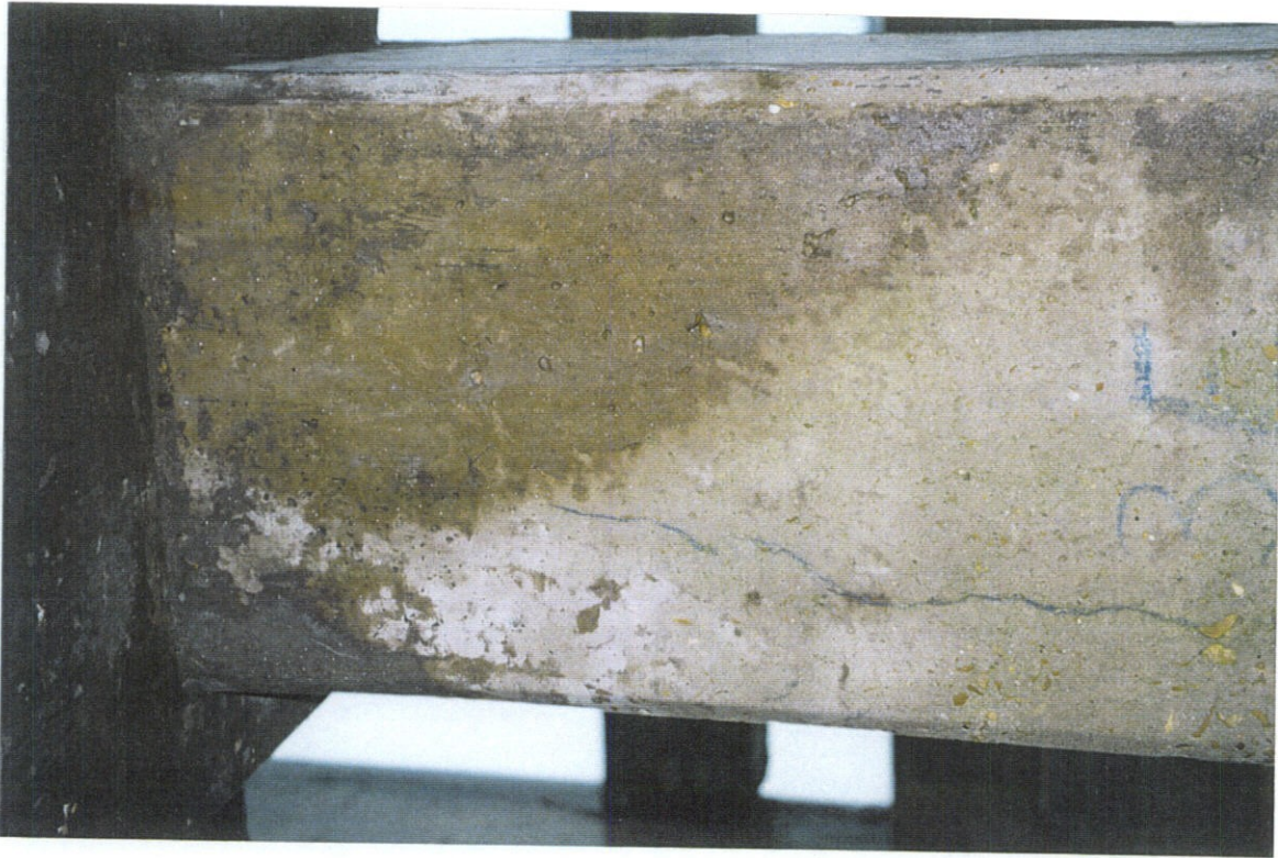
PHOTO NO. 15 - PILE NO. 3, EAST FACE, UPPER PORTION OF PILE. CRACK INCREASES IN SIZE (WIDTH) TOWARD BOTTOM OF PILE.
