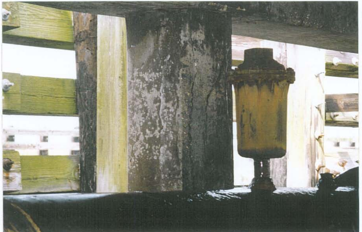
PHOTO NO. 11 – LOOKING NW AT CRACKS IN SOUTH AND EAST FACES OF PUMP PLATFORM PILE NO. 5.
