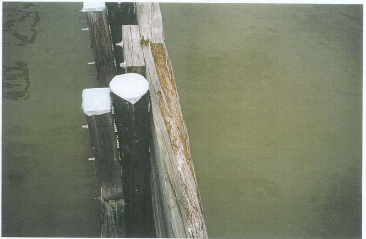
PHOTO NO. 34 – BADLY DETERIORATED TOP FENDER TIMBER ON NORTHWEST GUIDEWALL.
