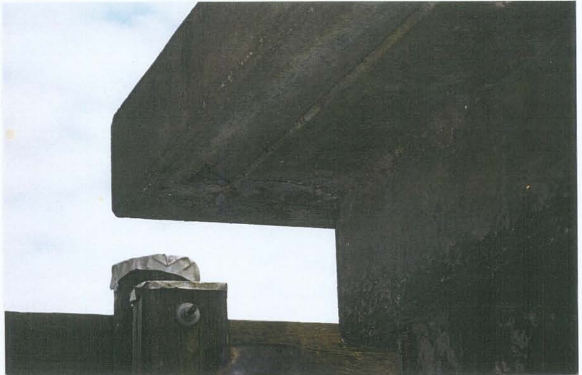
PHOTO NO. 16 – CRACK IN BOTTOM OF PUMP PLATFORM DECK AT SOUTHWEST CORNER.
