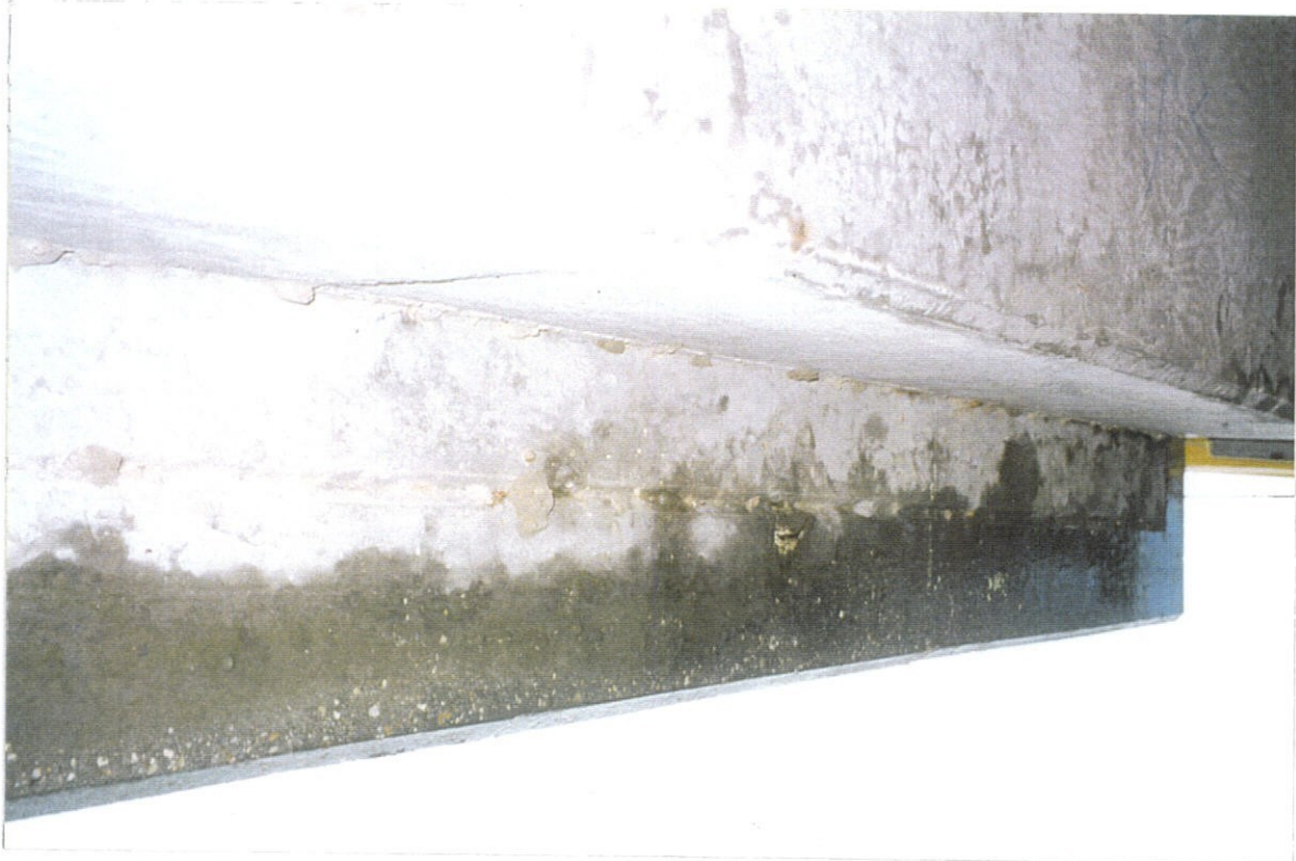
PHOTO NO. 39 - WEST UPPER DECK OVERHANG UNDERSIDE. NOTE CRACK ALONG DRIP STRIP.
