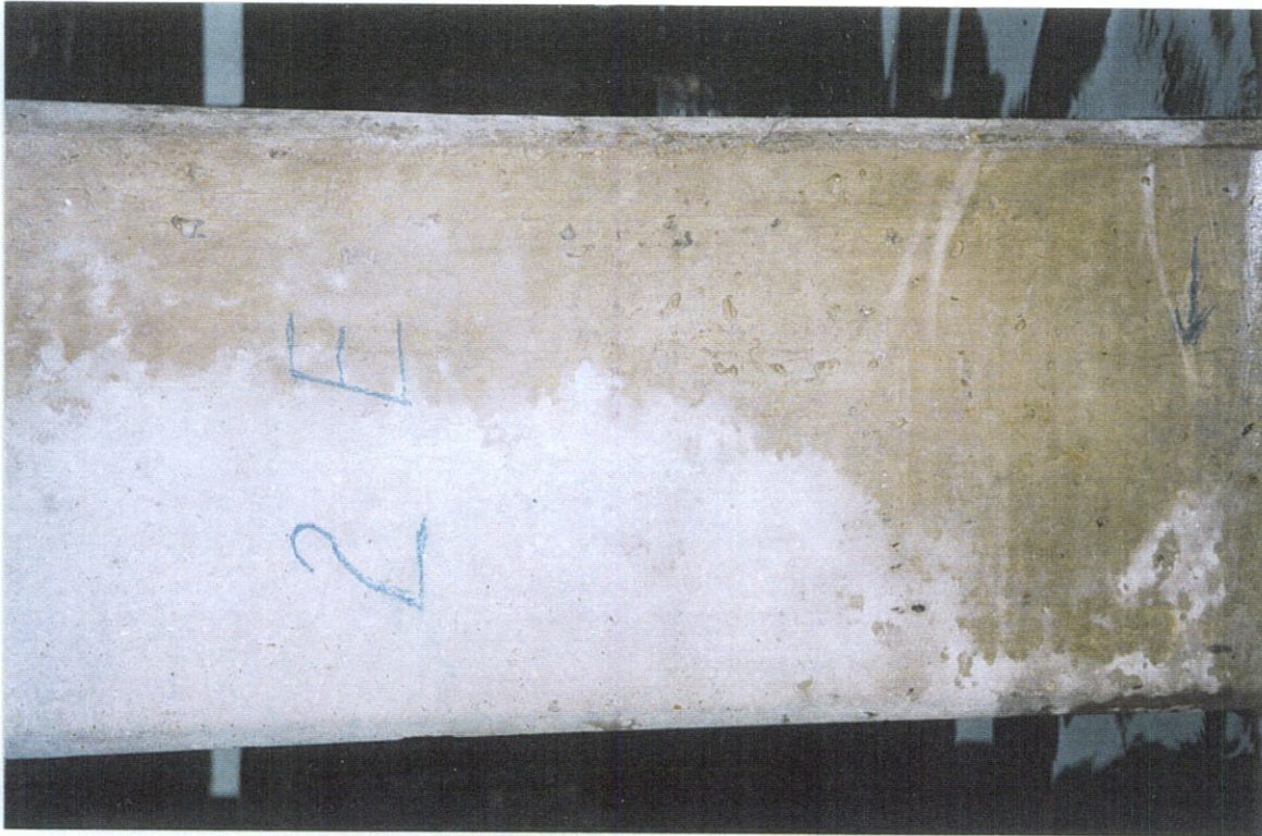
PHOTO NO. 5 - PILE NO. 2, EAST FACE. NO CRACKS. WHAT APPEARS TO BE CRACKS (ARROW) IS STAINS.
