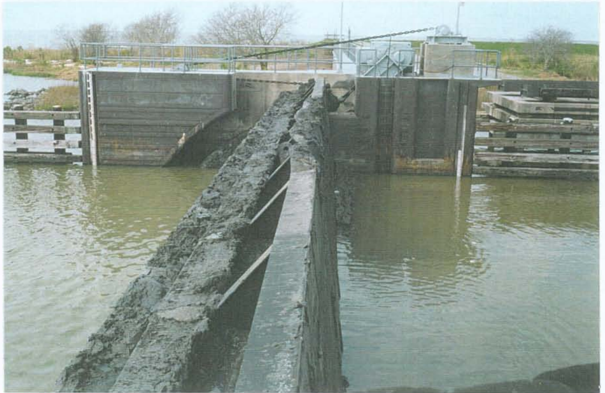
PHOTO NO. 25 – GATE APPROACHING CLOSED POSITION. NOTE COUNTERWEIGHT CHAIN IS PULLING AGAINST GATE CLOSING.
