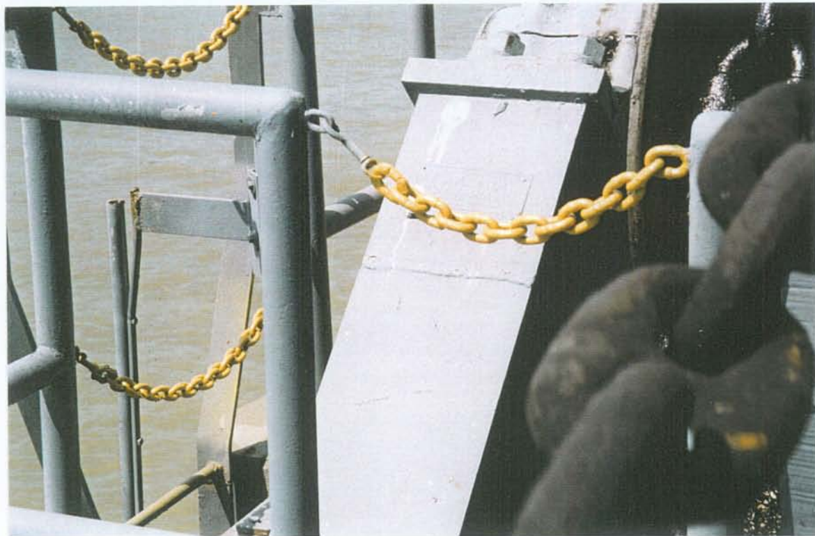
PHOTO NO. 19 – VIEWS OF SAFETY CHAINS ACROSS HANDRAIL OPENINGS. SAFETY CHAINS PAINTED AND IN GOOD CONDITION.
