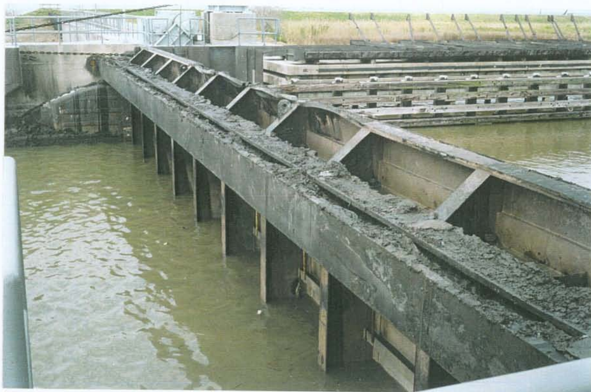
PHOTO NO. 20 – GATE IN FULLY CLOSED POSITION. PAINT SYSTEM IN GOOD CONDITION. NOTE DAMAGE ALONG TOP OF GATE. DAMAGE APPEARS TO BE SAME AS NOTED AT LAST INSPECTION.
