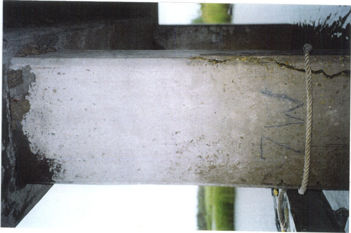
PHOTO NO. 32 - PILE NO. 7, WEST FACE, UPPER PORTION OF PILE. PATCH AT TOP OF PILE. OPEN CRACK AT SOUTHWEST CORNER OF PILE.
