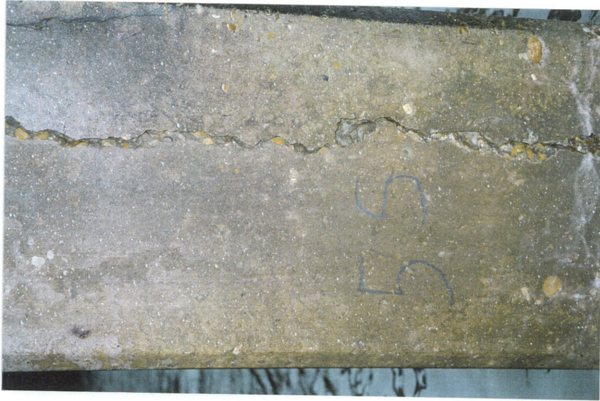
PHOTO NO. 27 - PILE NO. 5, SOUTH FACE, LOWER PORTION OF PILE. CONTINUATION OF CRACKS SHOWN IN PHOTO NO. 26.
