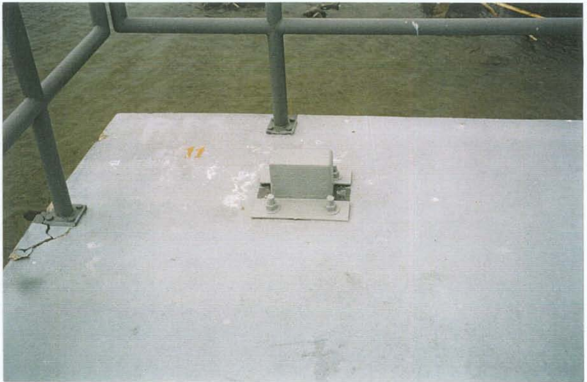
PHOTO NO. 3 – SPALL ON GATE BAY DECK AT HANDRAIL ANCHORAGE. NOTE COVER OVER OUTLET FOR LIGHT POLE THAT HAS BEEN RELOCATED.
