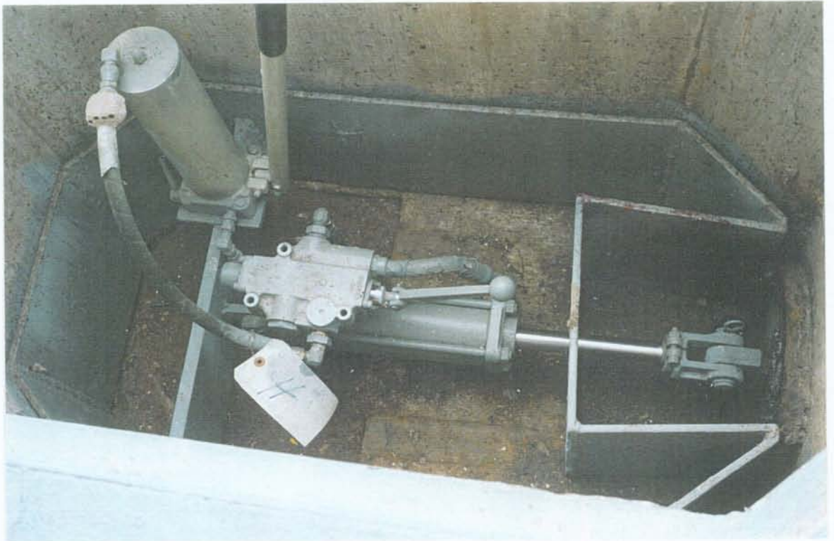
PHOTO NO. 30 – MANUALLY OPERATED GATE LATCHING MECHANISM.
