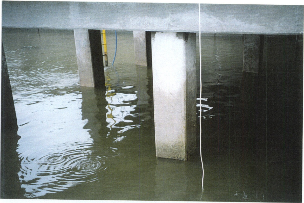
PHOTO NO. 31 - PILE NO. 7, NORTH FACE. VERTICAL CRACK NEAR NORTHWEST CORNER OF PILE.
