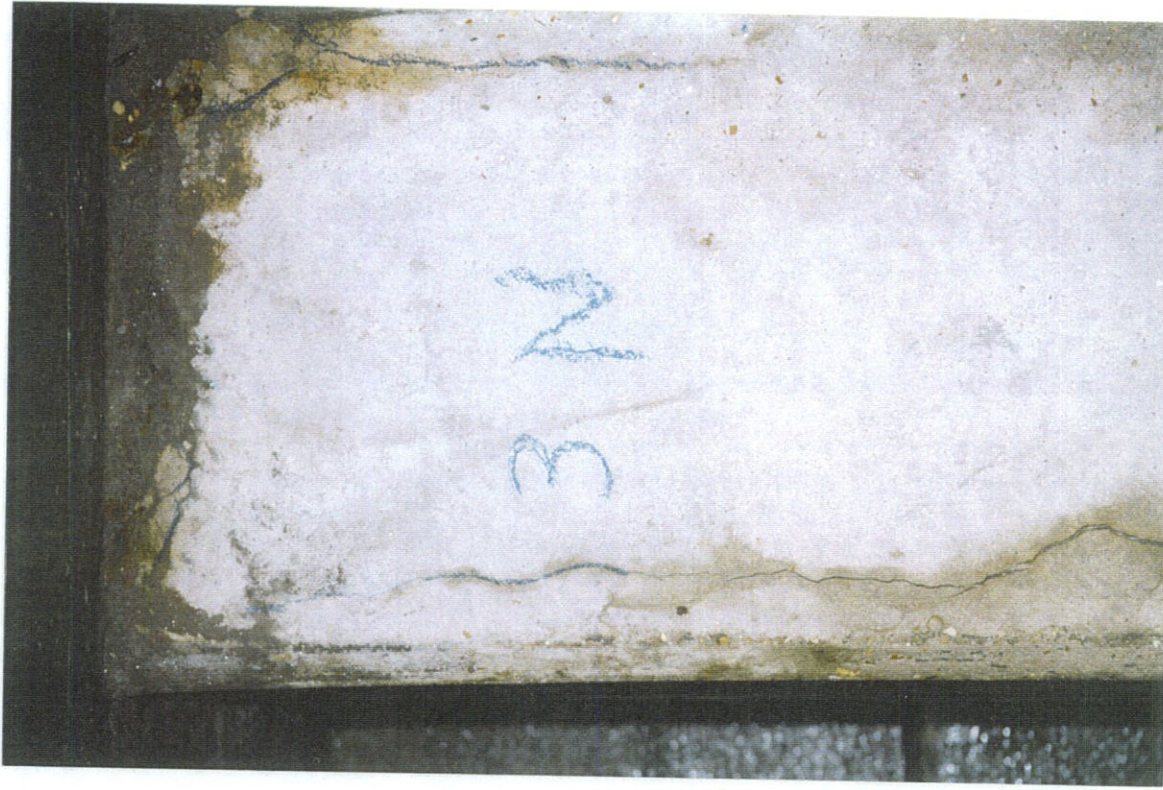
PHOTO NO. 12 - PILE NO. 3, NORTH FACE, TOP PORTION OF PILE. PATCH AT TOP OF PILE. CRACKS NEAR TOP OF PILE. VERTICAL CRACK ON RIGHT, AND UPPER PORTION OF VERTICAL CRACK ON LEFT MARKED WITH LUMBER CRAYON. CRACK ON LEFT IS OPEN EXCEPT UPPER PORTION.
