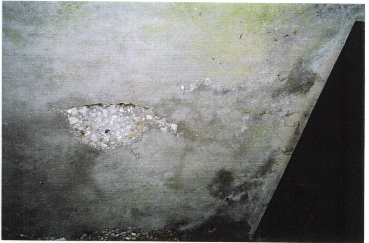
PHOTO NO. 47 - UNDERSIDE OF UPPER DECK, AREA B, LOOKING WEST AT AREA JUST SOUTH OF PUMP COLUMN RECESS. NOTE SPALL AND CRACK FROM PUMP COLUMN RECESS.
