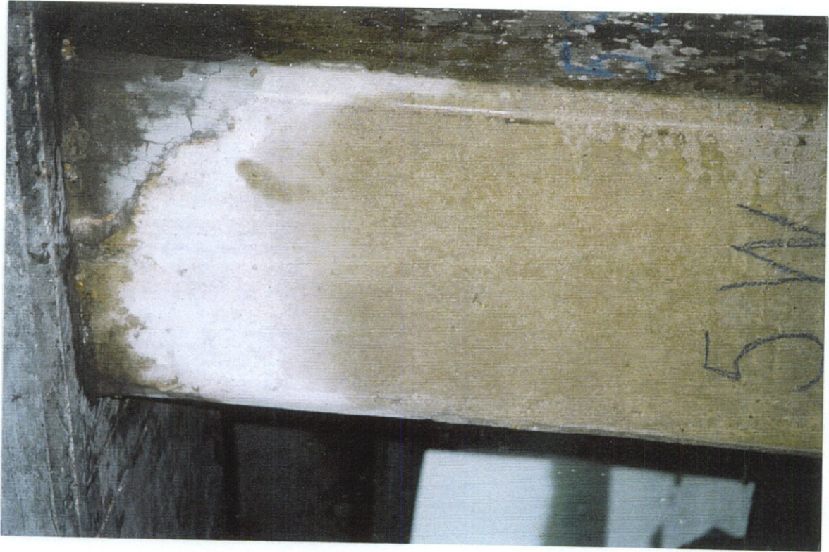
PHOTO NO. 23 - PILE NO. 5, WEST FACE, UPPER PORTION OF PILE. PATCHES AT TOP OF PILE AT BOTH CORNERS. NO CRACKS OBSERVED.
