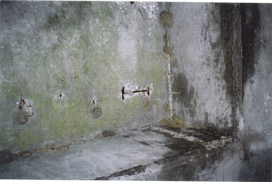
PHOTO NO. 44 - UNDERSIDE OF UPPER DECK, NORTHEAST CORNER OF AREA B (DENOTED ON CRACK SURVEY PLAN SHEET) LOOKING EAST.
