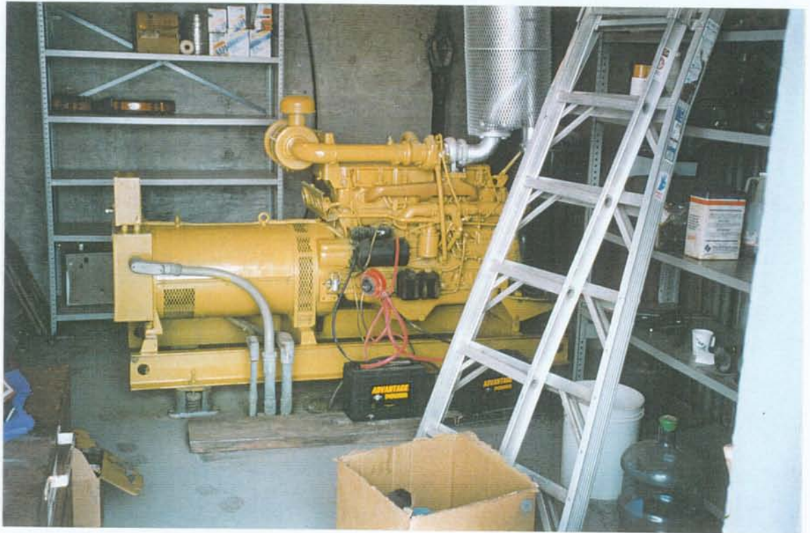
PHOTO NO. 31 – EMERGENCY POWER GENERATOR UNIT.
