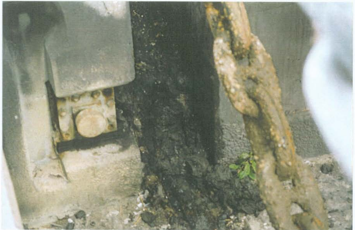
PHOTO NO. 26 – GATE SHOCK ABSORBER STUCK IN FULLY RECESSED POSITION.
