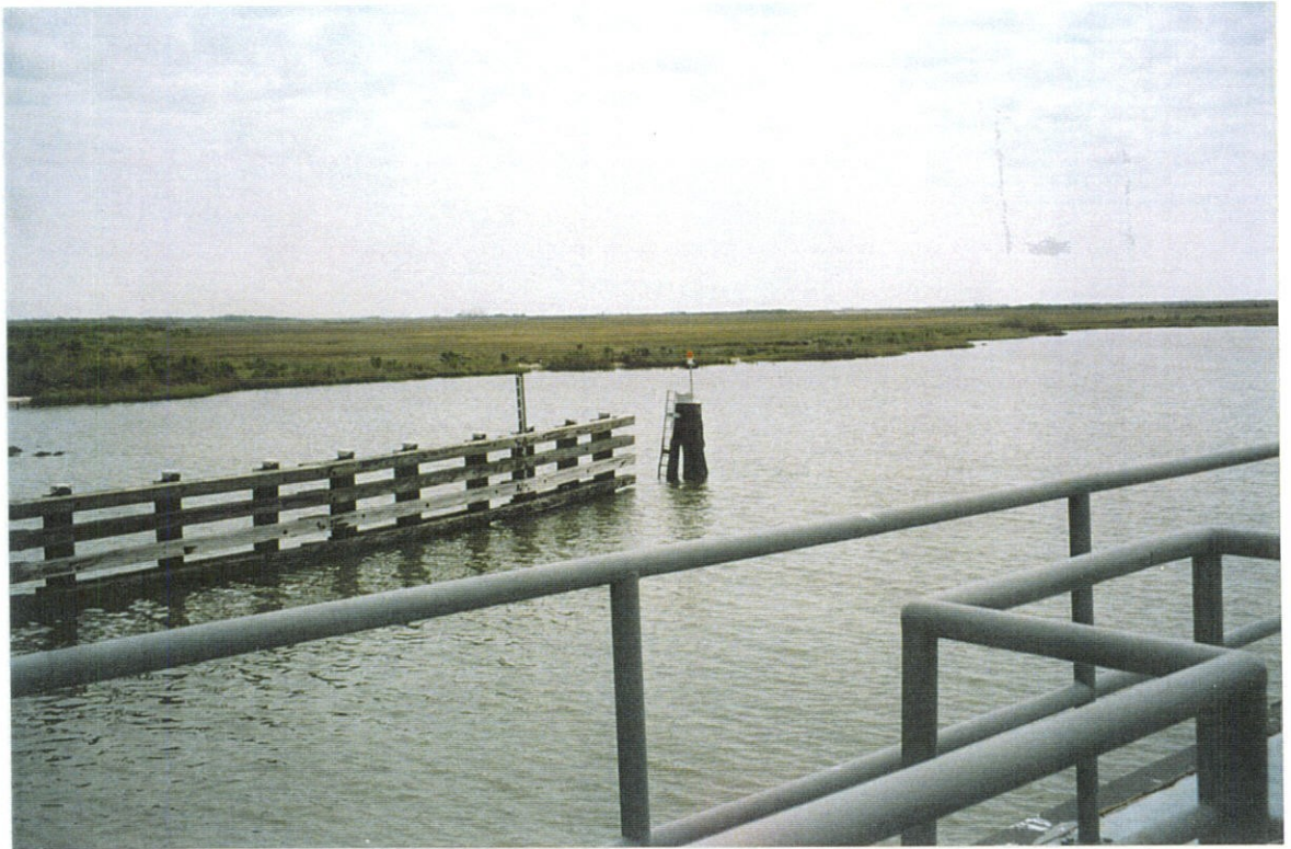
PHOTO NO. 39 – PROTECTED SIDE WEST CHANNEL BANK. NOTE EROSION POCKET APPROXIMATELY 200 FEET NORTH OF NORTH END OF GUIDEWALL.
