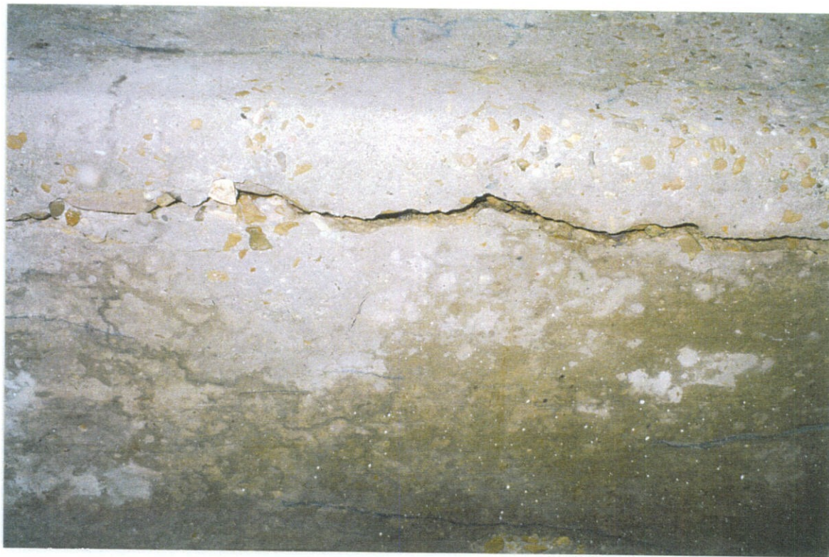
PHOTO NO. 18 - PILE NO. 3, SOUTH FACE, MIDDLE PORTION OF PILE. CONTINUATION OF CRACKS SHOWN IN PHOTO NO. 17.
