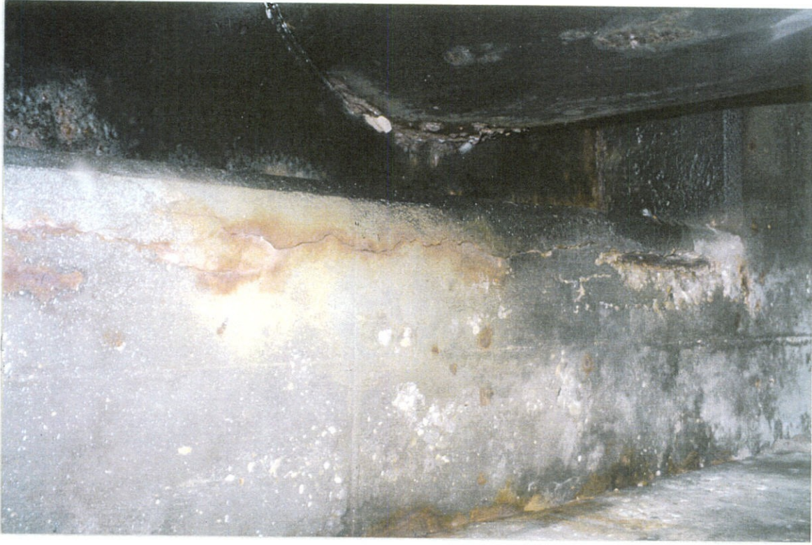
PHOTO NO. 45 - UNDERSIDE OF UPPER DECK, AREA B, JUST WEST OF PUMP COLUMN BLOCKOUT, LOOKING NORTH. PUMP COLUMN ON RIGHT.
