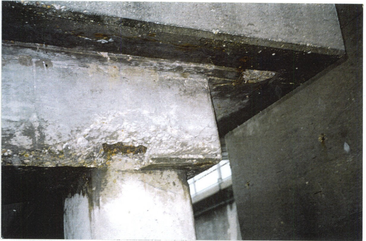
PHOTO NO. 40 – SOUTH END OF WEST NORTH/SOUTH BEAM AND UNDERSIDE OF TOP DECK OVERHANG. NOTE CRACKED AND SPALLED AREA ON BEAM WITH EXPOSED REINFORCEMENT AND SPALL AND CRACK IN DECK OVERHANG.
