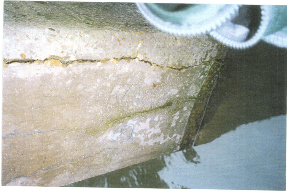
PHOTO NO. 19 - PILE NO. 3, SOUTH FACE, CONTINUATION OF CRACKS SHOWN IN PHOTO NO. 18.
