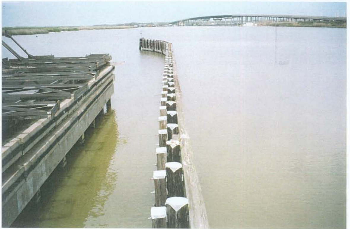
PHOTO NO. 33 – NORTHWEST TIMBER GUIDEWALL. NOTE ALUMINUM CAPS ON TOP OF PILES AND VERTICAL TIMBERS.
