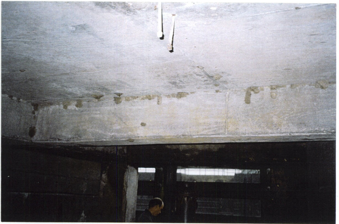
PHOTO NO. 43 - LOOKING WEST AT UNDERSIDE OF UPPER DECK (AREA A AS DENOTED ON CRACK SURVEY PLAN SHEET). NO CRACKS NOTED.
