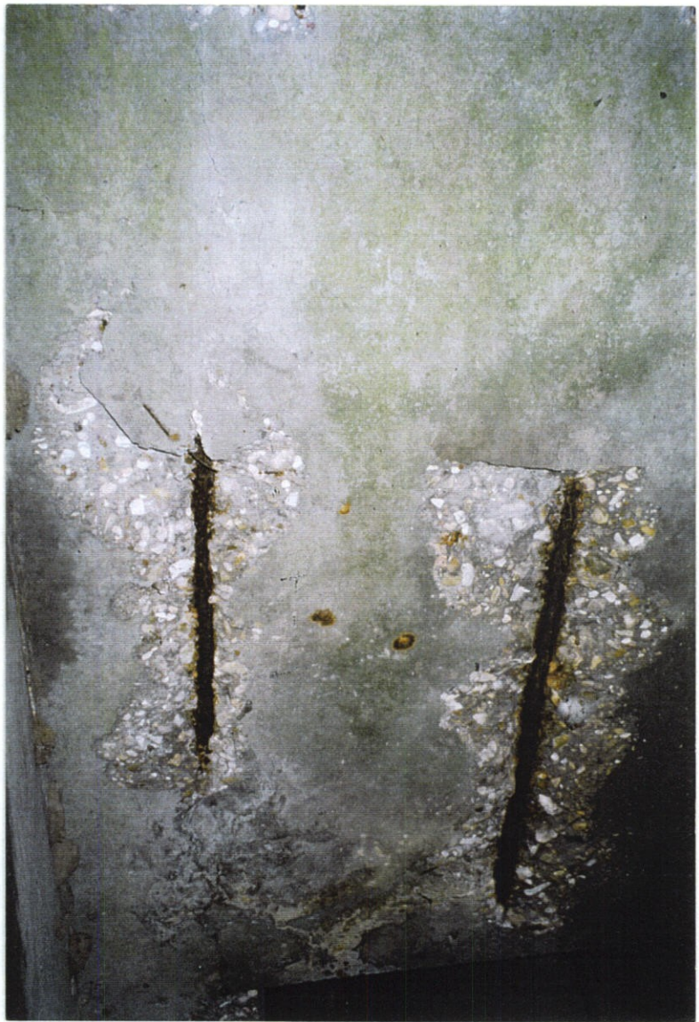
PHOTO NO. 46 - UNDERSIDE OF UPPER DECK, AREA B, LOOKING SOUTH. PUMP COLUMN RECESS (AT BOTTOM OF PHOTO) JUST SOUTH OF EXPOSED REINFORCEMENT.
