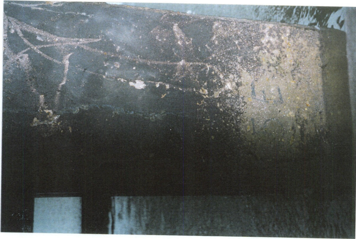
PHOTO NO. 29 - PILE NO. 5, EAST FACE, LOWER PORTION OF PILE. CONTINUATION OF CRACK AT SOUTHEAST CORNER (PHOTO NO. 28) TO WATER SURFACE DOES NOT SHOW EXCEPT NEAR WATER SURFACE DUE TO POOR QUALITY OF PHOTO.
