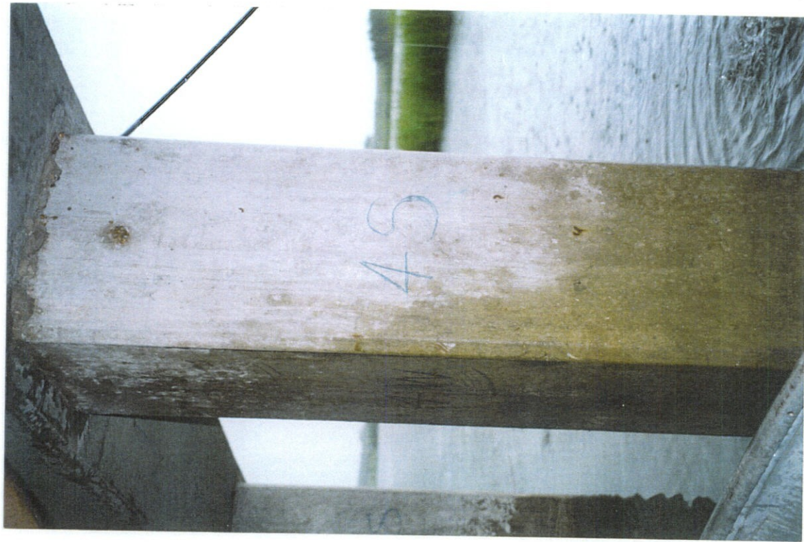
PHOTO NO. 20 - PILE NO. 4, SOUTH FACE, GOOD VISUAL CONDITION. NO CRACKS NOTED ON PILE NO. 4
