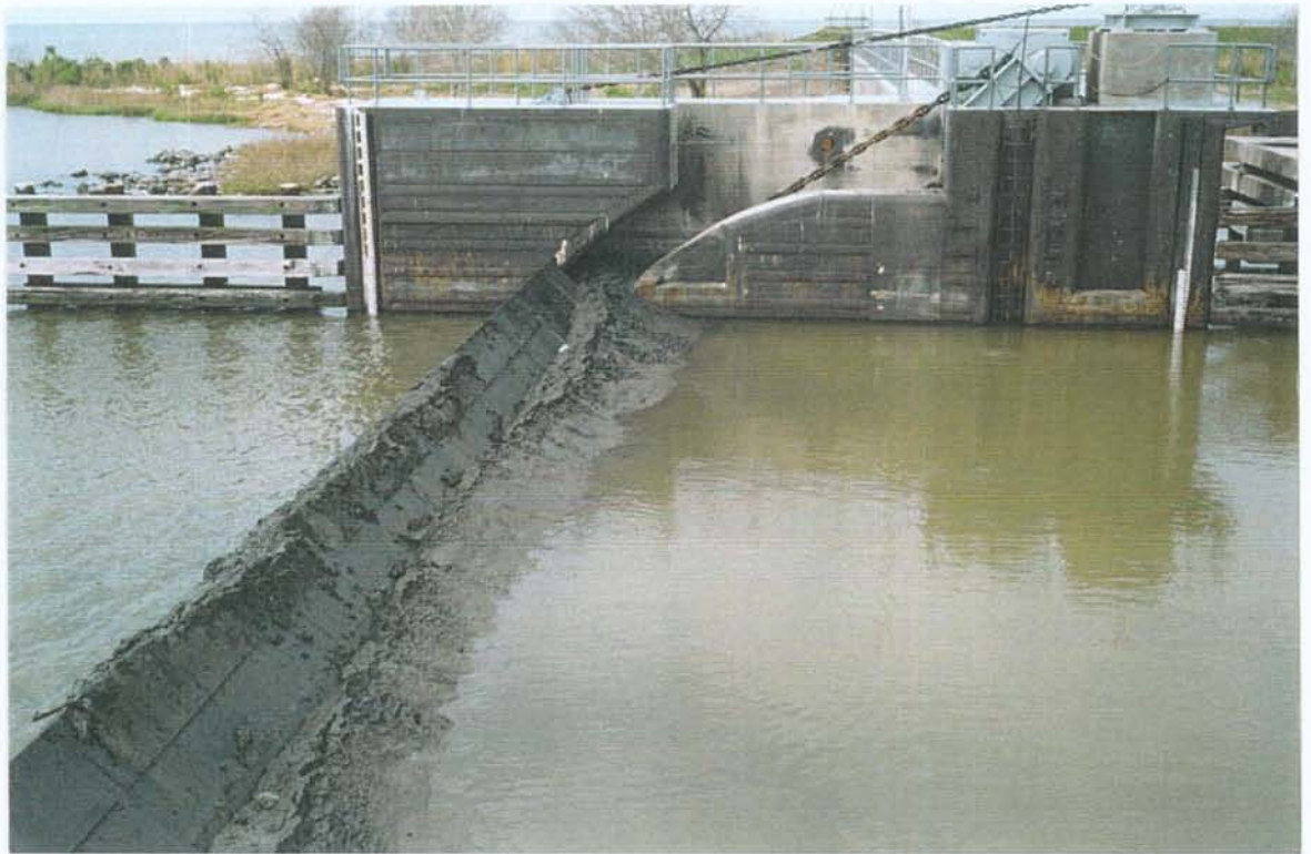
PHOTO NO. 17 – LOOKING WEST AT CHAMBER FACE OF WEST GATE BAY WALL. NOTE CORROSION ON EMBEDDED METAL AT SPLASH ZONE.
