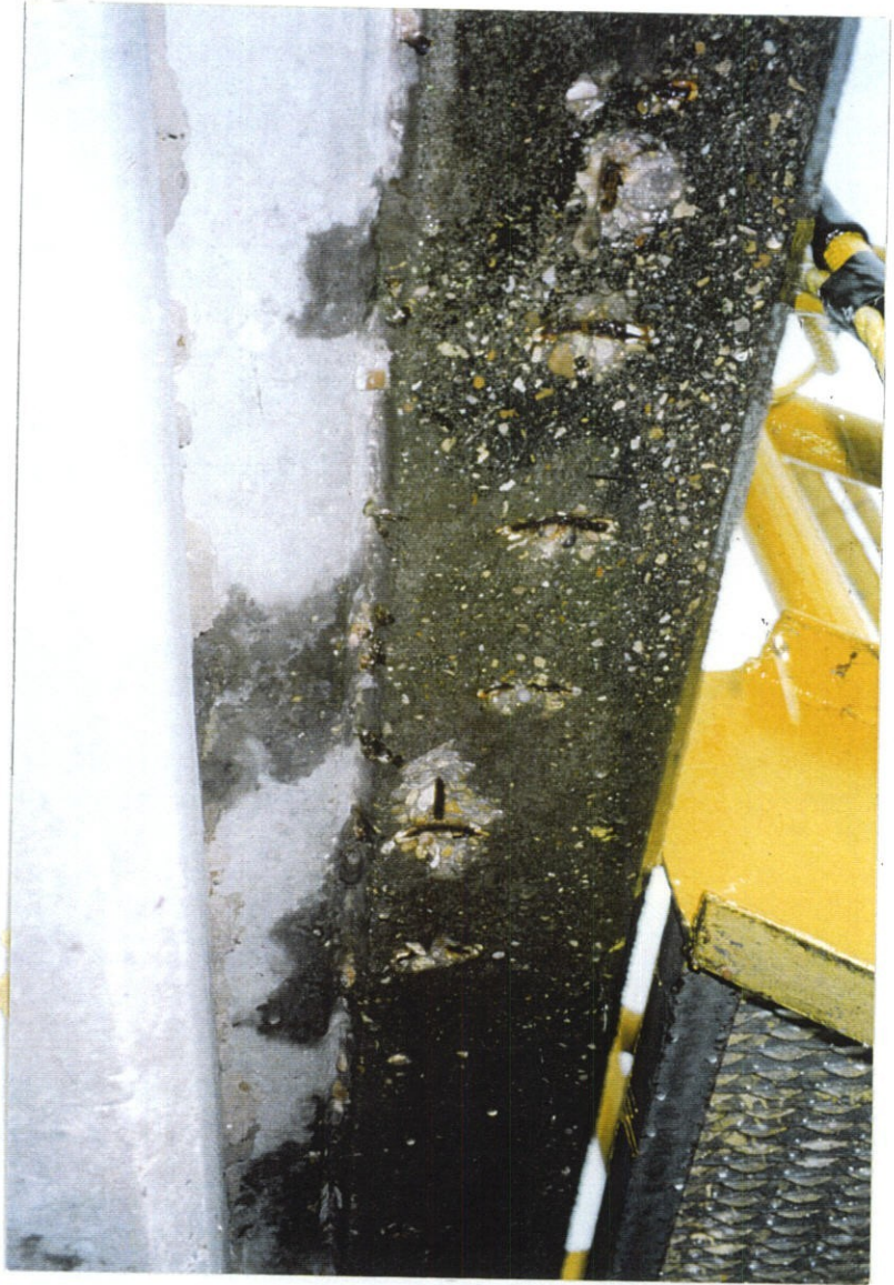
PHOTO NO. 42 - LOOKING WEST AT UNDERSIDE OF UPPER DECK NORTH OVERHANG. NOTE SHALLOW SPALLS WITH WHAT APPEARS TO BE EXPOSED REINFORCEMENT CHAIRS THAT ARE CORRODED.
