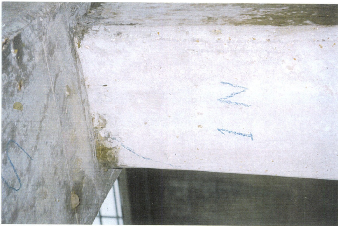
PHOTO NO. 1 - PILE NO. 1, NORTH FACE. NOTE SMALL CRACK (MARKED WITH LUMBER CRAYON) AND PATCH (UPPER LEFT CORNER).
