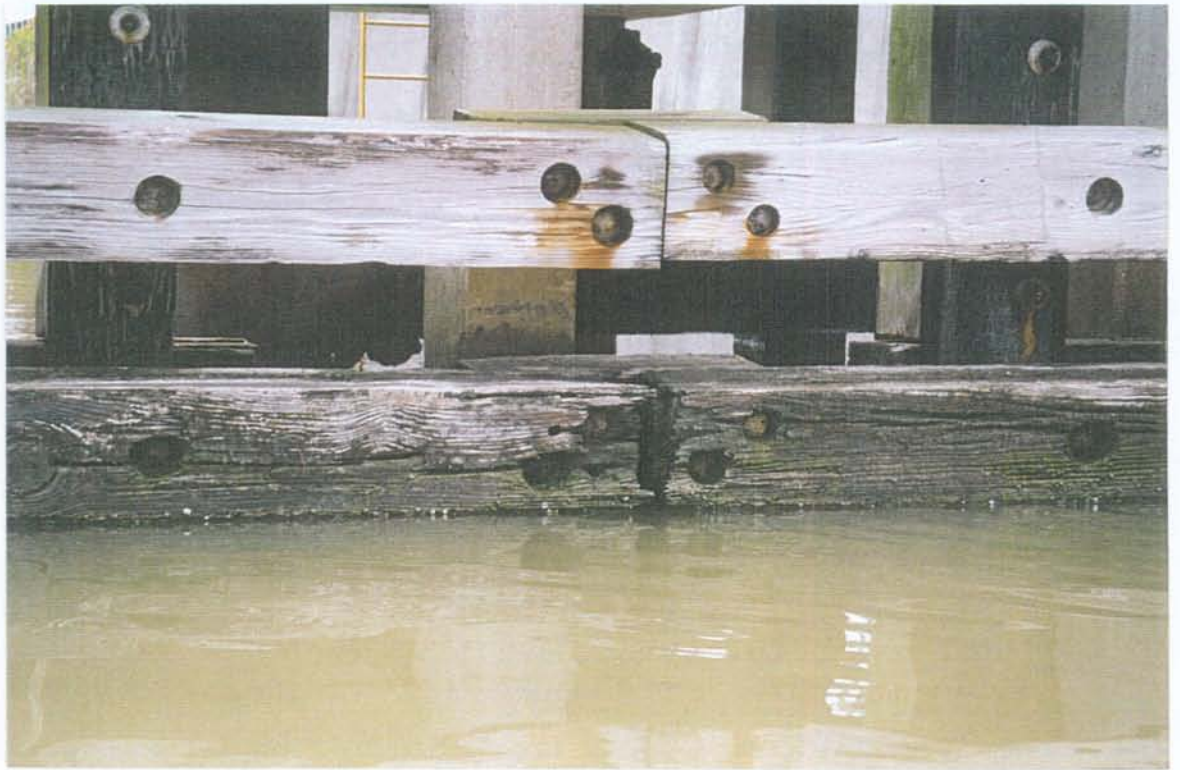
PHOTO NO. 35 – DETERIORATED FENDER TIMBER AT SPLASH ZONE.
