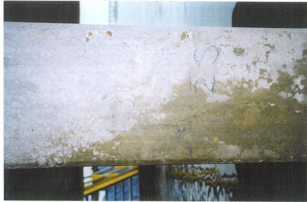
PHOTO NO. 3 - PILE NO. 2, SOUTH FACE. NOTE CRACK.
