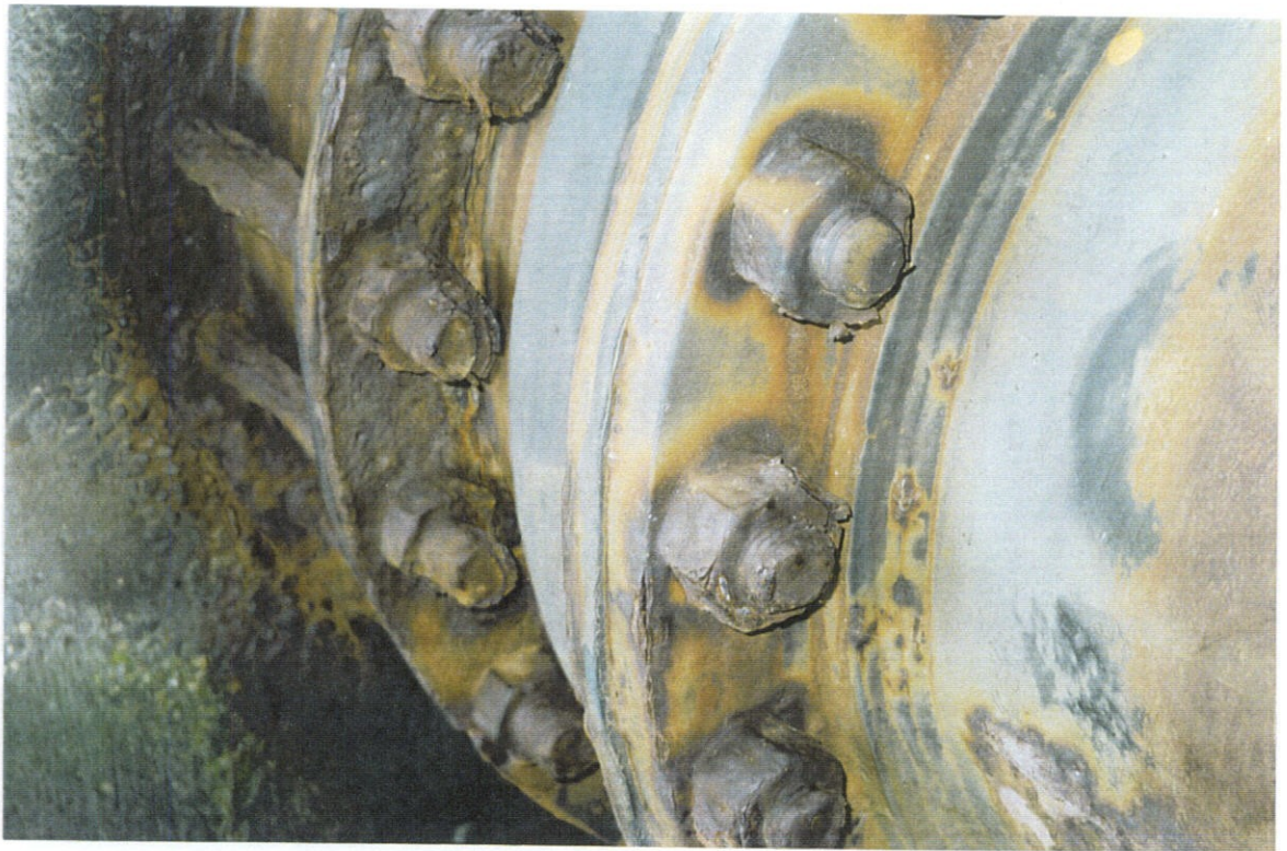
PHOTO NO. 44 - VIEW OF BADLY CORRODED ATTACHMENT RING AND ATTACHMENT BOLTS AND NUTS FOR 24-INCH CHECK VALVE AND EXPANSION COUPLING.
