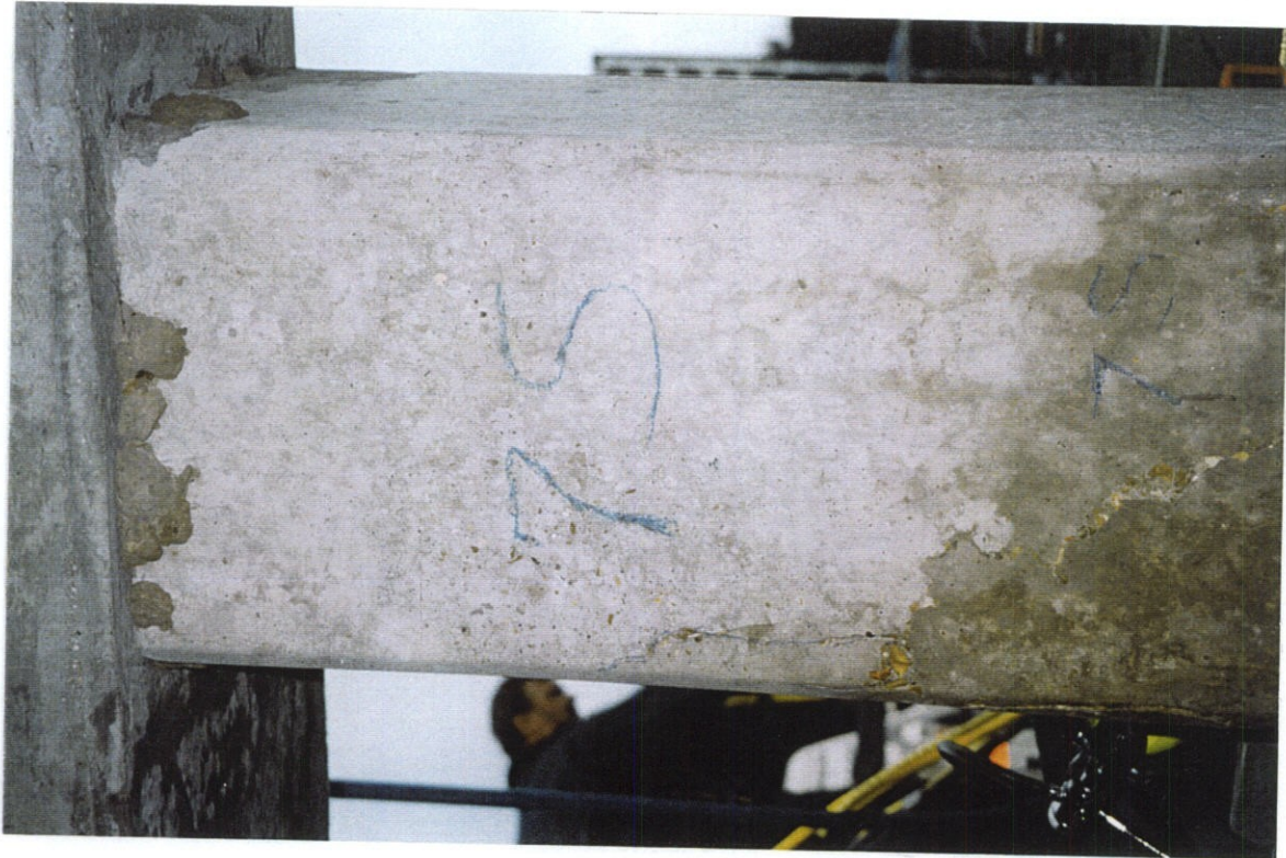
PHOTO NO. 34 - PILE NO. 7, SOUTH FACE, UPPER PORTION OF PILE. PATCHES AT TOP OF PILE. CRACK NEAR SOUTHWEST CORNER AND LEFT OF LOWER "7S."
