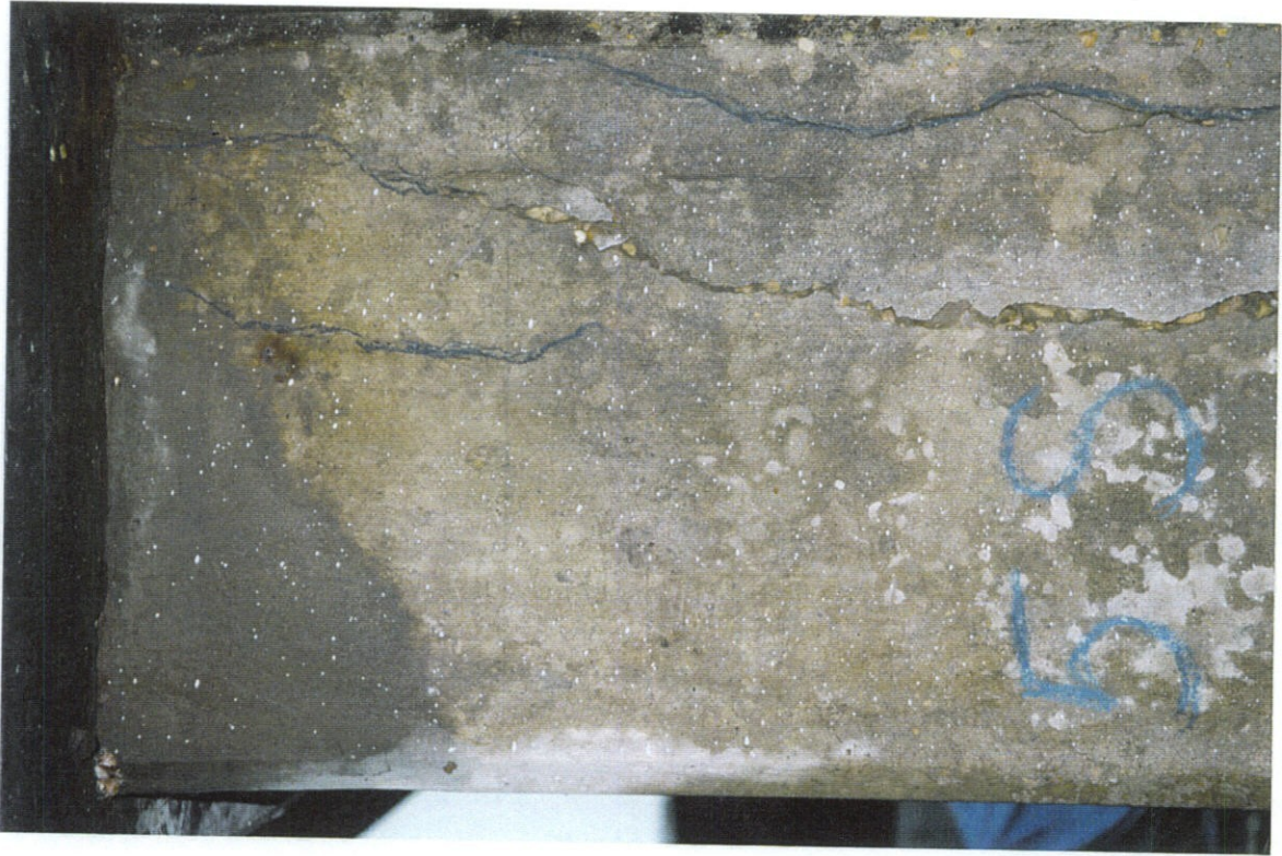
PHOTO NO. 25 - PILE NO. 5, SOUTH FACE, UPPER PORTION OF PILE. LARGE PATCH AT TOP, VERTICAL CRACKS ON RIGHT.
