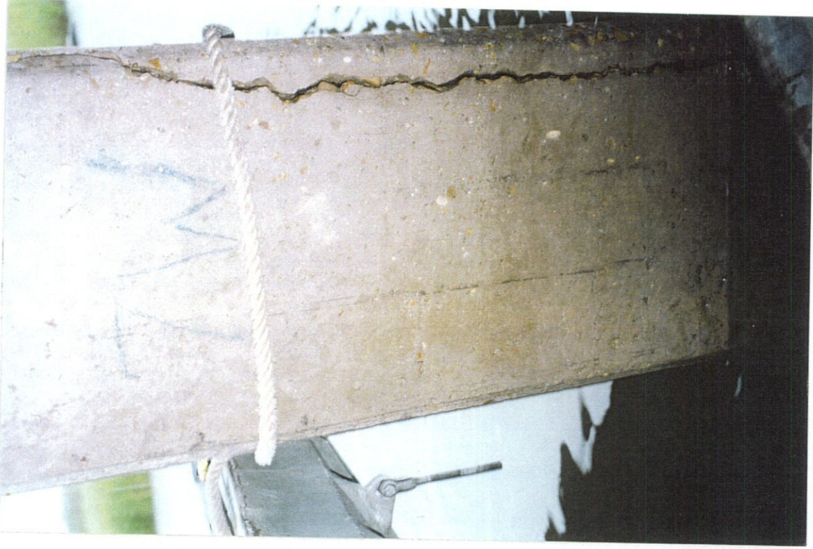
PHOTO NO. 33 - PILE NO. 7, WEST FACE, LOWER PORTION OF PILE. CONTINUATION OF OPEN CRACK SHOWN IN PHOTO NO. 32.
