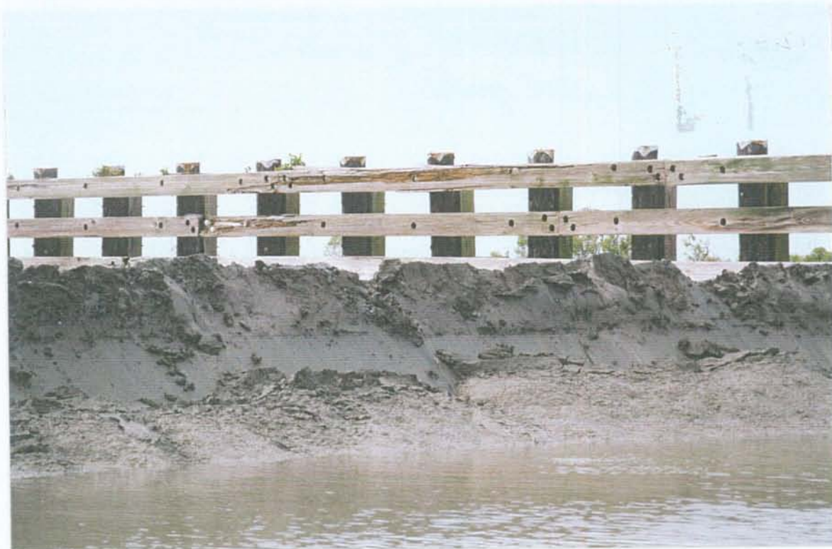
PHOTO NO. 23 – SILT SLIDING OFF GATE AS IT IS BEING CLOSED (RAISED).
