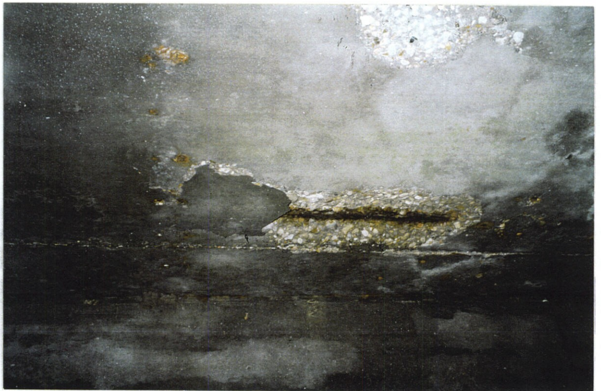
PHOTO NO. 48 - UNDERSIDE OF UPPER DECK, LOOKING WEST AT SOUTHWEST PART OF AREA B, WEST NORTH/SOUTH BEAM IN BACKGROUND. NOTE PATCH AT SOUTH (LEFT) END OF EXPOSED CORRODED REINFORCEMENT.
