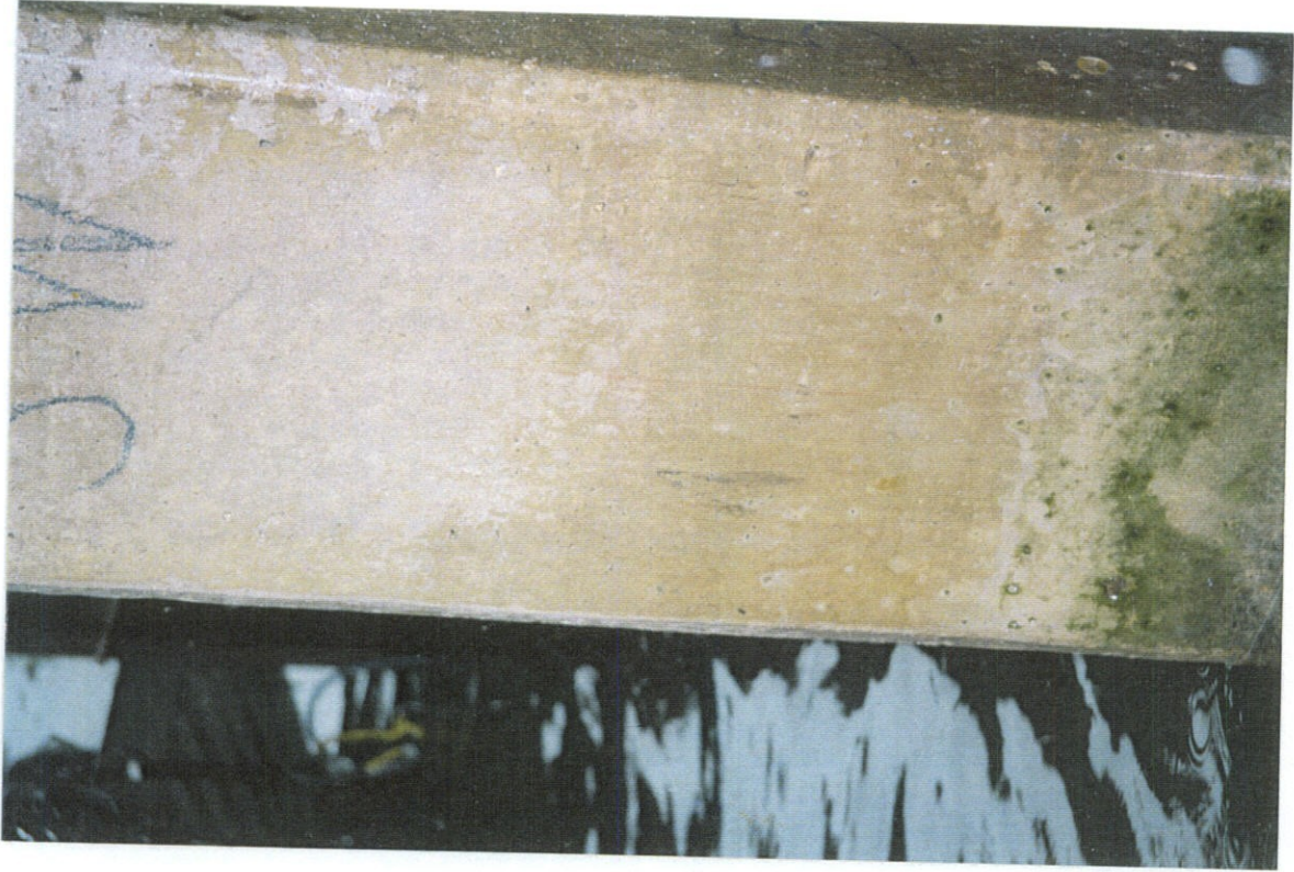
PHOTO NO. 24 - PILE NO. 5, WEST FACE, LOWER PORTION OF PILE. NO CRACKS OBSERVED.
