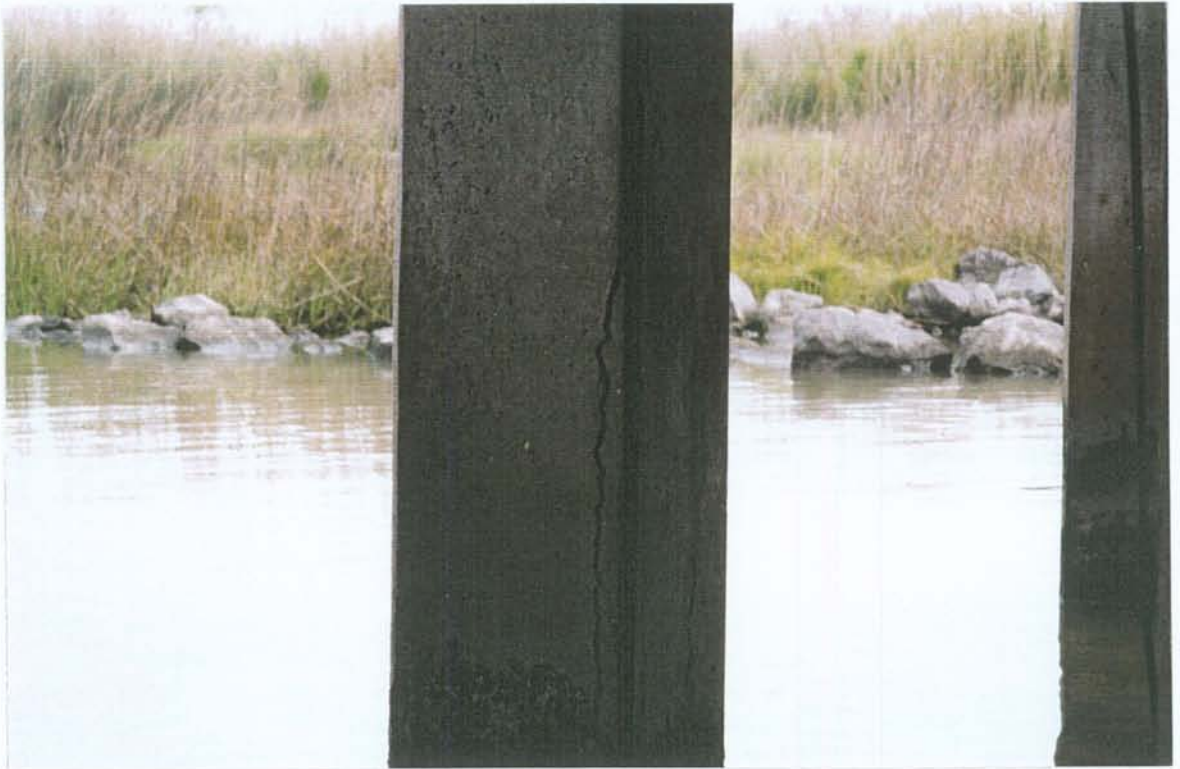
PHOTO NO. 10 – LOOKING ESE AT CRACK IN NORTH FACE OF PUMP PLATFORM PILE NO. 2.
