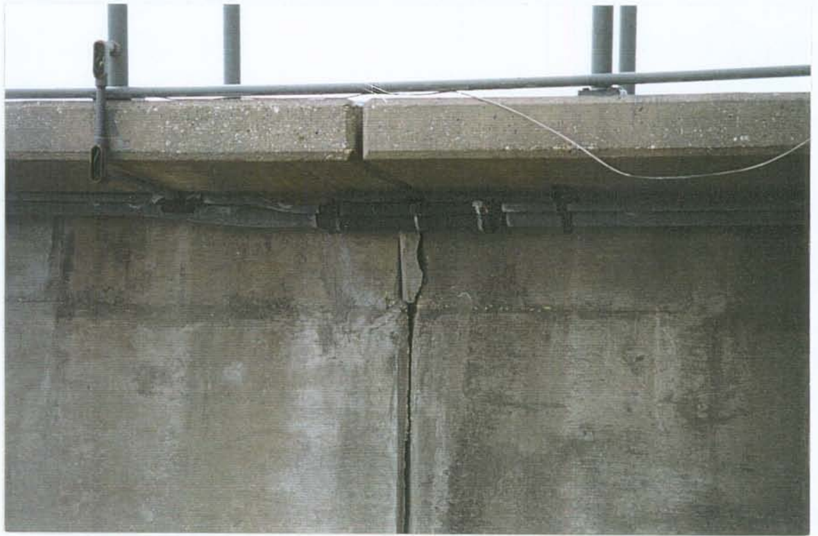
PHOTO NO. 1 – SPALL ON PROTECTED SIDE OF EAST "T" WALL AT JOINT BETWEEN MONOLITHS T-2R AND T-3R.
