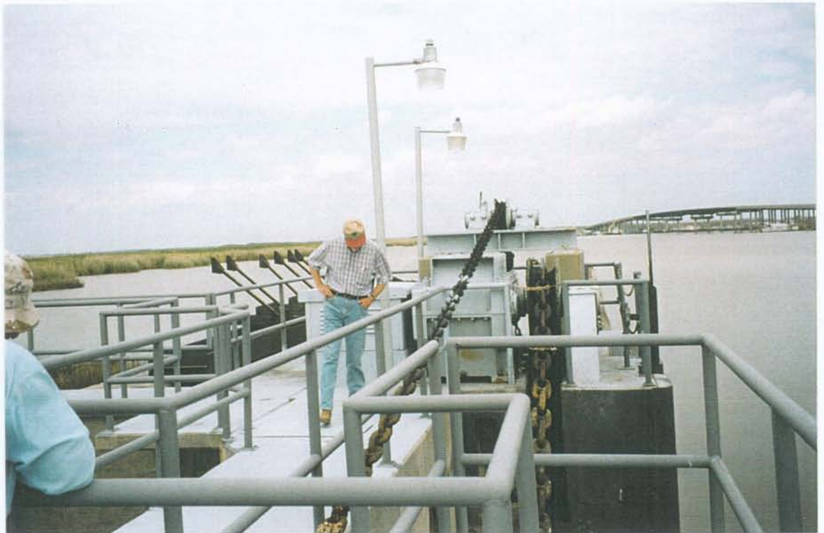
PHOTO NO. 18 – LOOKING NORTH ALONG TOP OF WEST SIDE GATE BAY WALL. NOTE GOOD CONDITION OF PAINT ON HANDRAILS.
