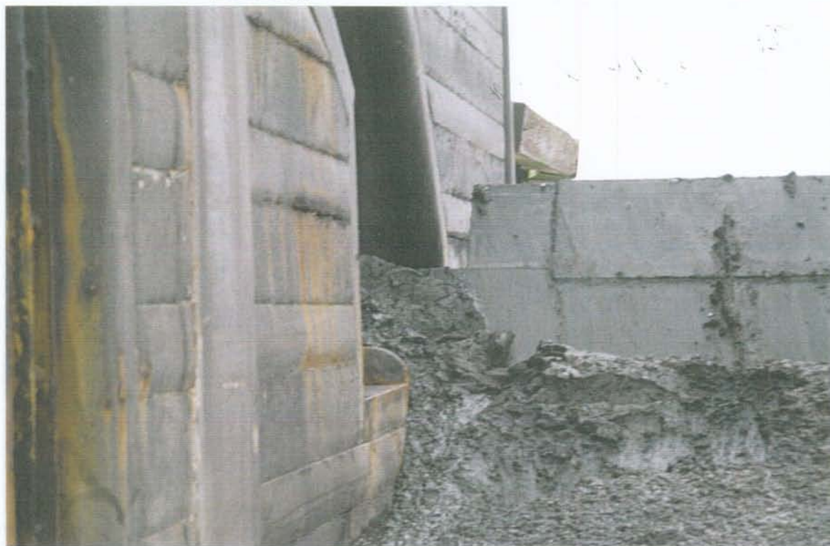
PHOTO NO. 24 – SILT ACCUMULATION AS GATE IS BEING CLOSED (RAISED).
