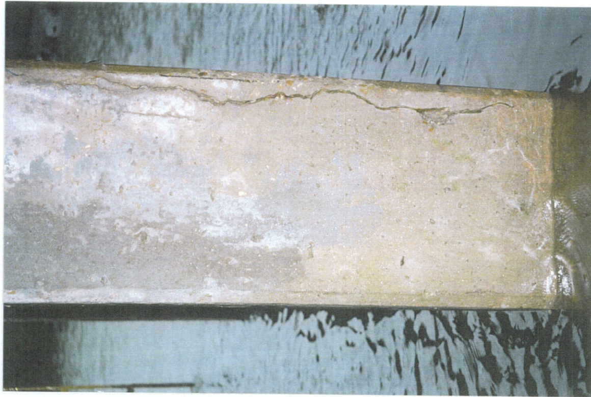
PHOTO NO. 6 - PILE NO. 2, WEST FACE. CRACKS NEAR SOUTHWEST CORNER OF PILE.
