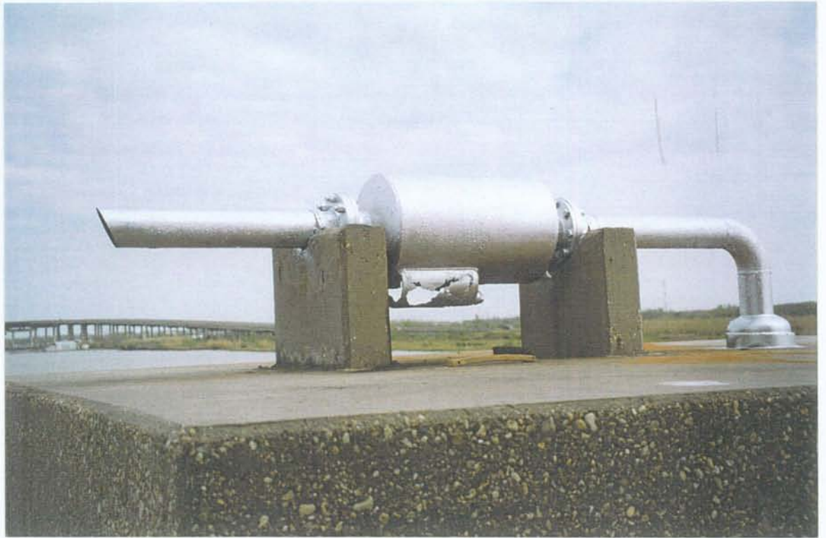
PHOTO NO. 29 – PUMP ENGINE MUFFLER ON TOP OF PUMP HOUSE. MUFFLER BADLY CORRODED ON BOTTOM AND LEAKING EXHAUST.
