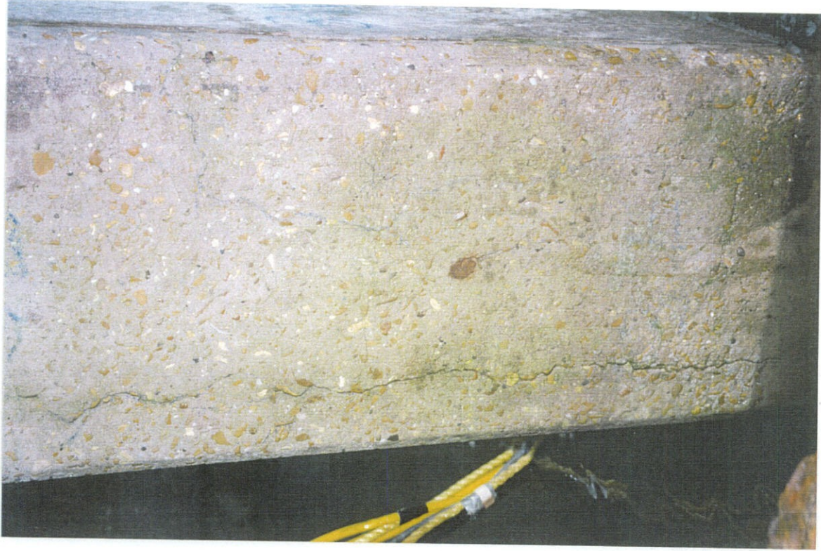
PHOTO NO. 16 - PILE NO. 3, EAST FACE, LOWER PORTION OF PILE. CONTINUATION OF CRACK SHOWN IN PHOTO NO. 15.
