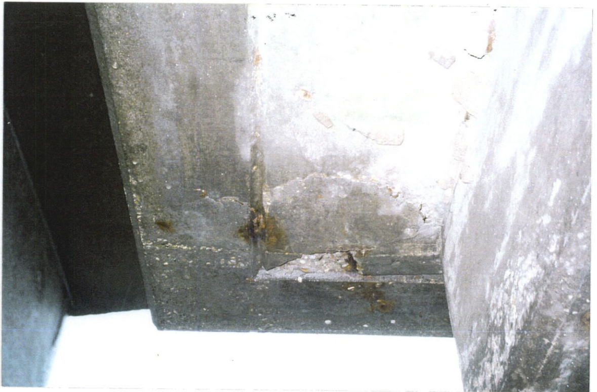
PHOTO NO. 41 – UNDERSIDE OF UPPER DECK SOUTH OVERHANG, PHOTO LOOKING WEST. NOTE SPALL AT DRIP STRIP (SHOWS IN PHOTO NO. 40) AND CRACKS IN UNDERSIDE OF DECK.
