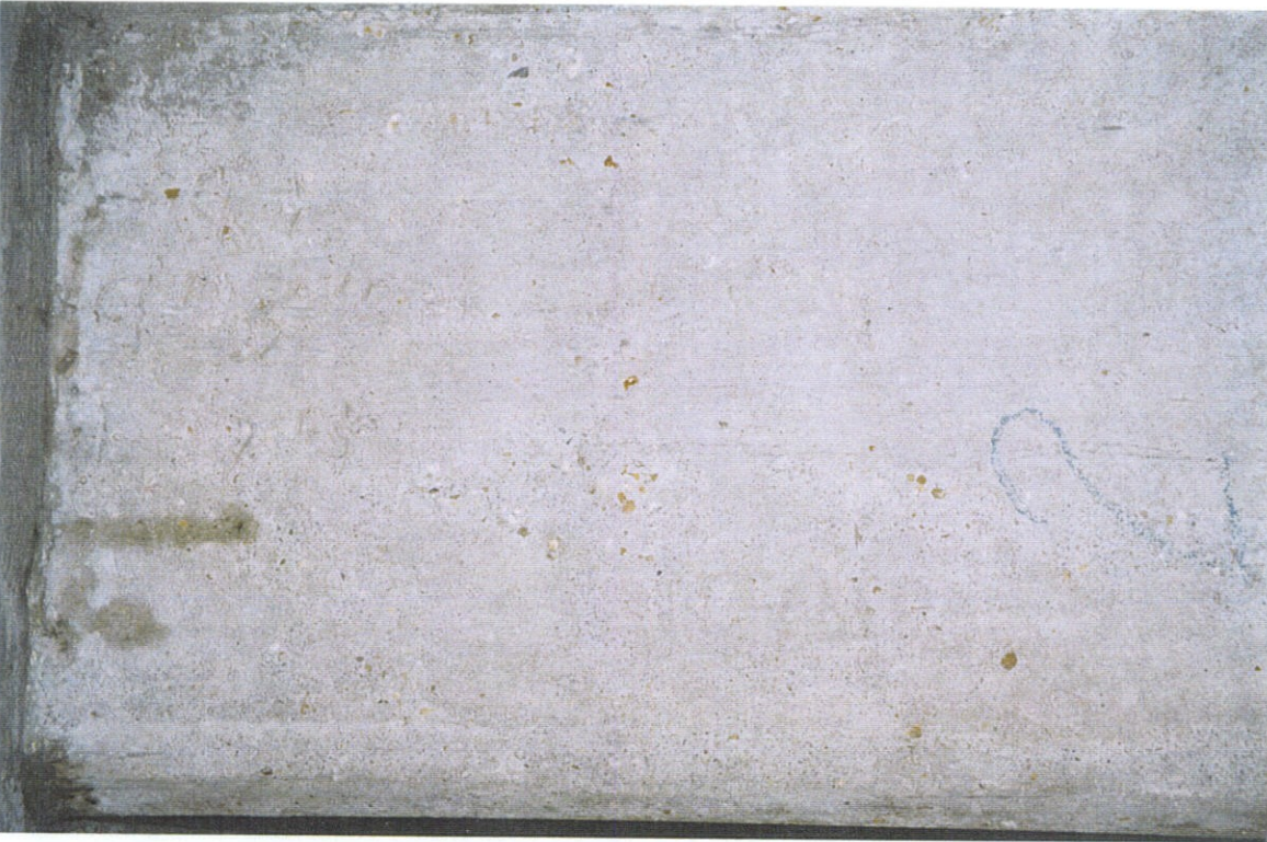
PHOTO NO. 7 - PILE NO. 2, NORTH FACE, UPPER PART OF PILE. NO CRACKS.
