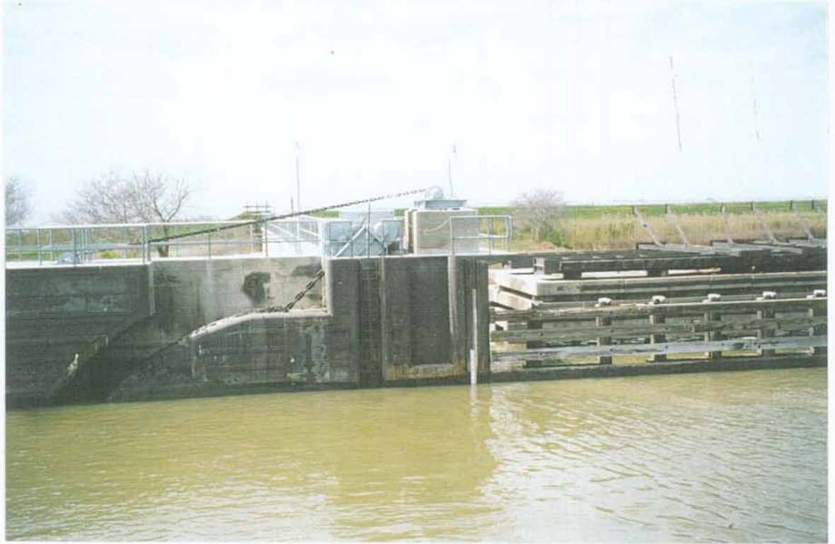
PHOTO NO. 27 – VIEW SHOWING POSITION OF HOIST AND COUNTERWEIGHT CHAINS WITH GATE OPEN (LOWERED).
