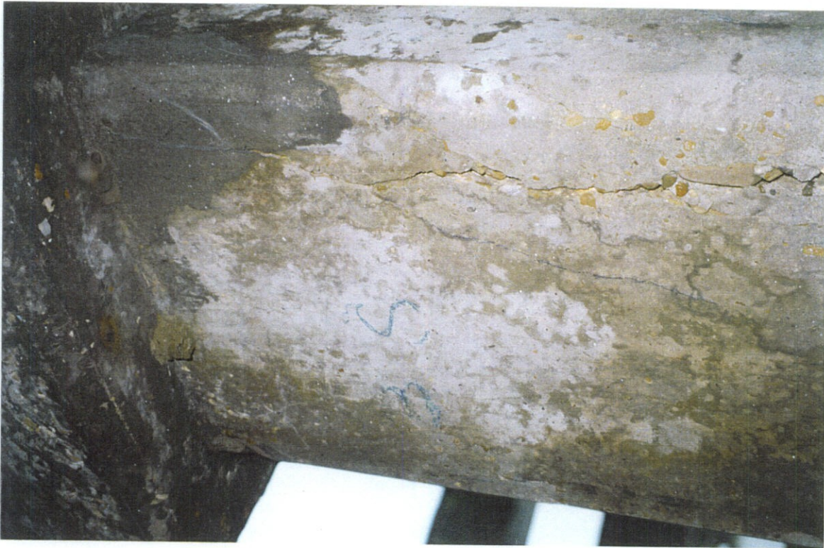
PHOTO NO. 17 - PILE NO. 3, SOUTH FACE, UPPER PORTION OF PILE. PATCH AT TOP OF PILE ON SOUTHEAST CORNER OF PILE. LARGER CRACK IS OPEN.
