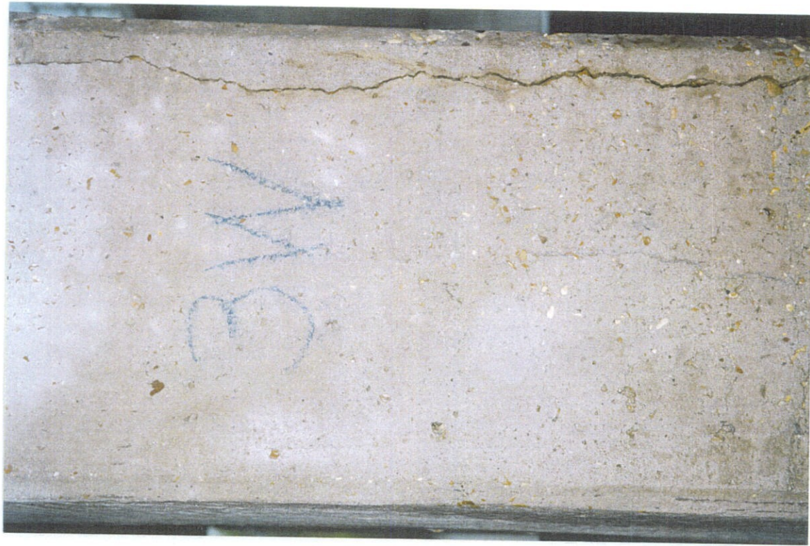
PHOTO NO. 10 - PILE NO. 3, WEST FACE. MIDDLE PORTION OF PILE. CONTINUATION OF OPEN CRACK SHOWN IN PHOTO NO. 9.
