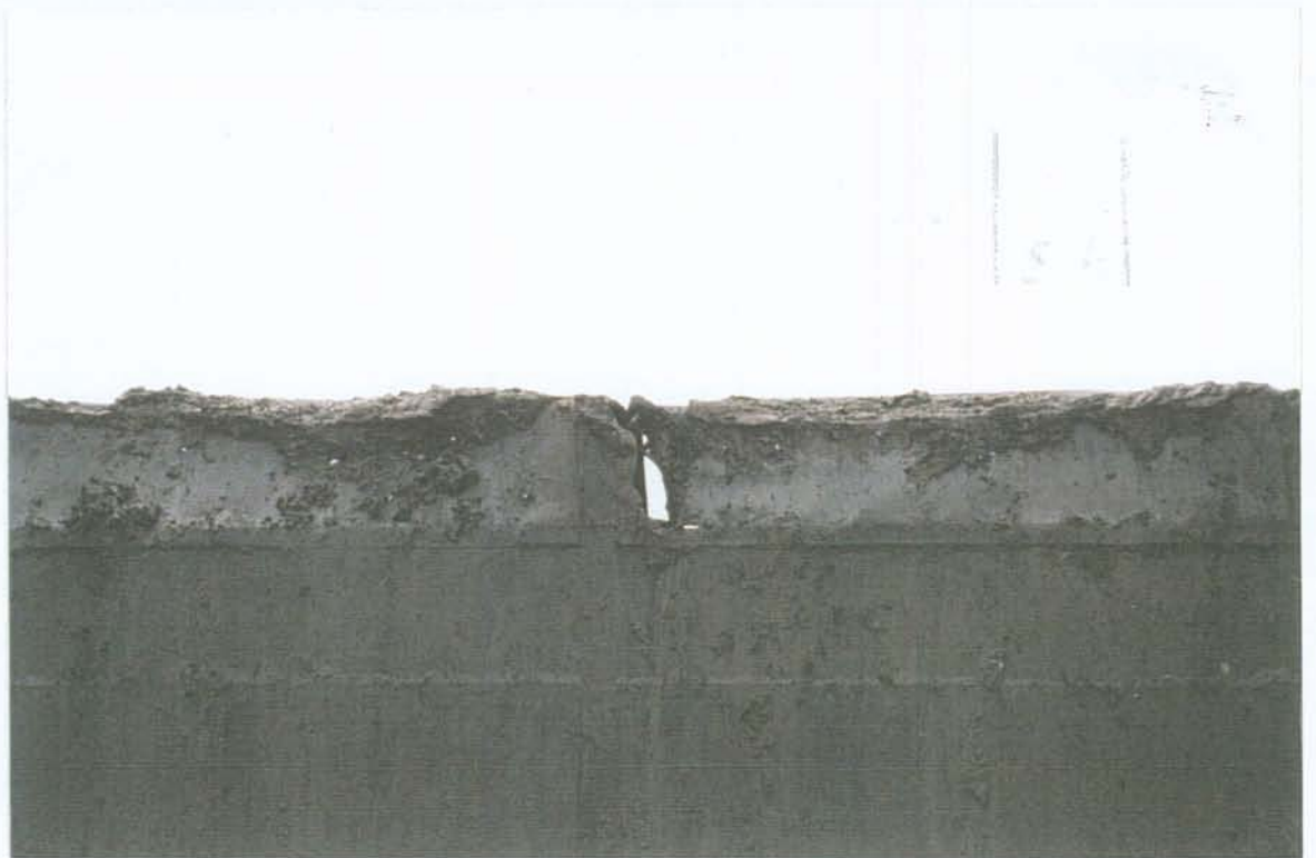
PHOTO NO. 21 - SKINPLATE SIDE OF GATE IN FULLY CLOSED POSITION. PAINT SYSTEM IN GOOD CONDITION. NOTE DAMAGE ON TOP OF GATE.
