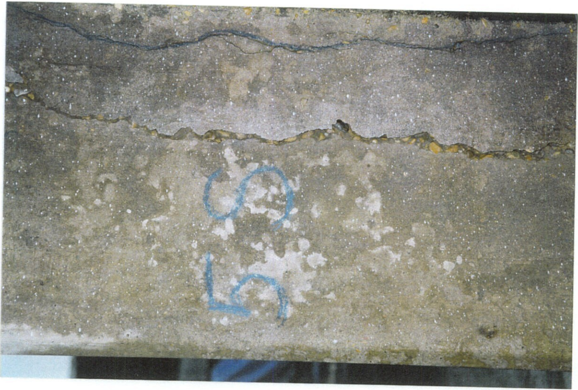
PHOTO NO. 26 - PILE NO. 5, SOUTH FACE, MIDDLE PORTION OF PILE. CONTINUATION OF CRACKS SHOWN IN PHOTO NO. 25.
