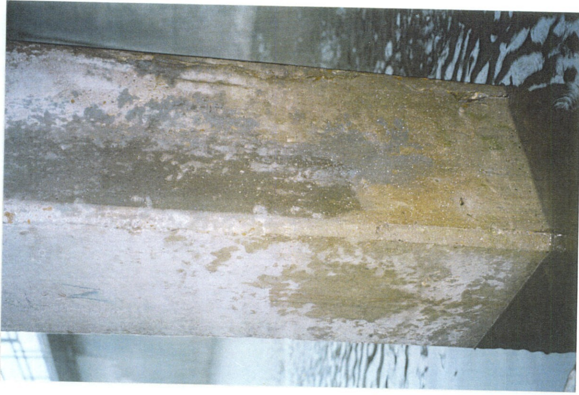
PHOTO NO 8 - PILE NO. 2, NORTH FACE ON LEFT, WEST FACE ON RIGHT. NO CRACKS NOTED IN NORTH FACE. CRACKS IN WEST FACE ALSO SHOWN IN PHOTO NO. 6.
