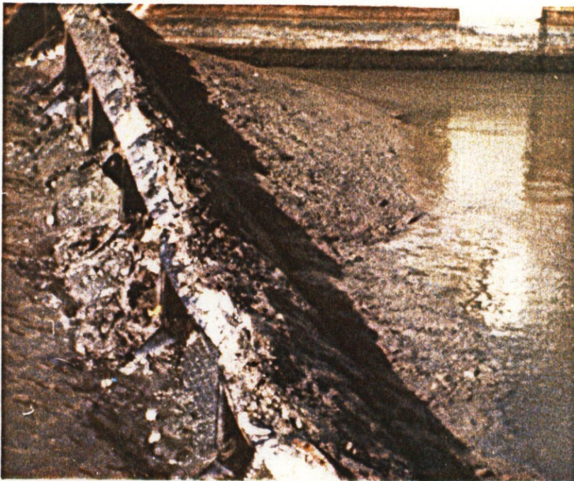
Photo No. 4: Damaged flap gate
