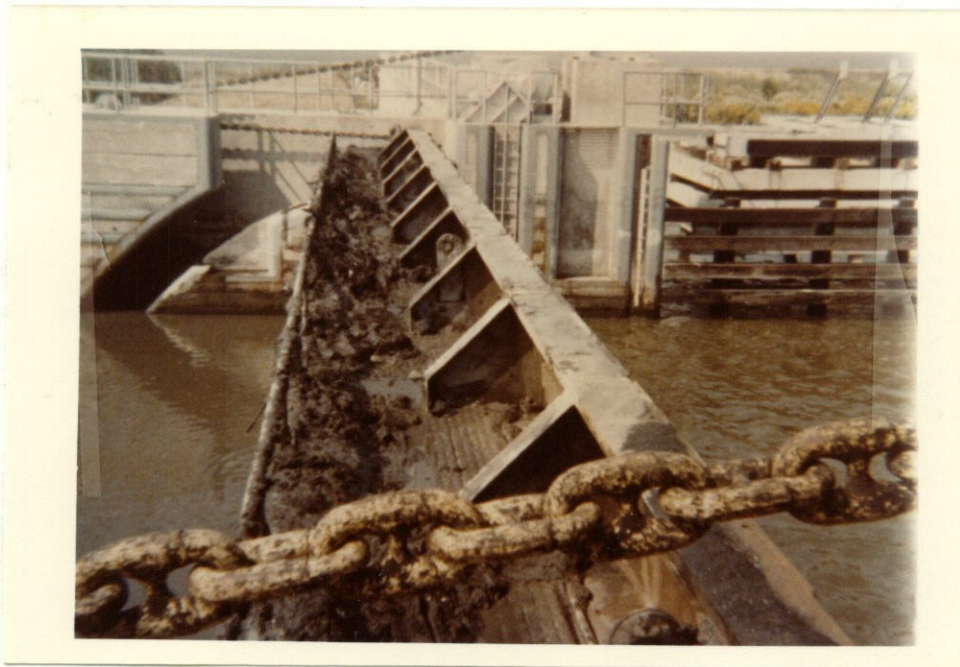
PHOTO NO. 5 - Trapped Soil Deposits on Walkway and Rusted Chain
