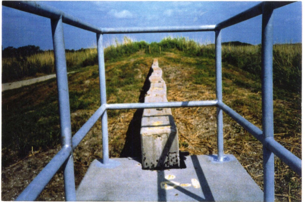
PHOTO 1 - Separation of concrete sheetpile from the T-wall on west side
