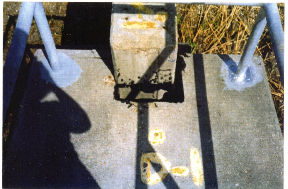
PHOTO 2 - Separation of concrete sheetpile from the T-wall on the west side
