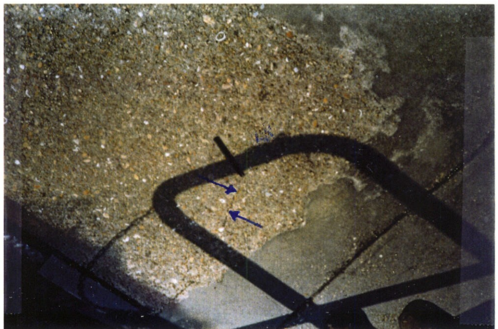
Photo 8 - Typical hairline cracks on top of gatebay monoliths and T-walls on both west and east sides
