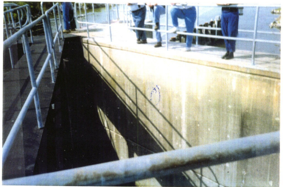
Photo 10 - Efflorescence on channel walls and on both west and east sides of the gatebay structures
