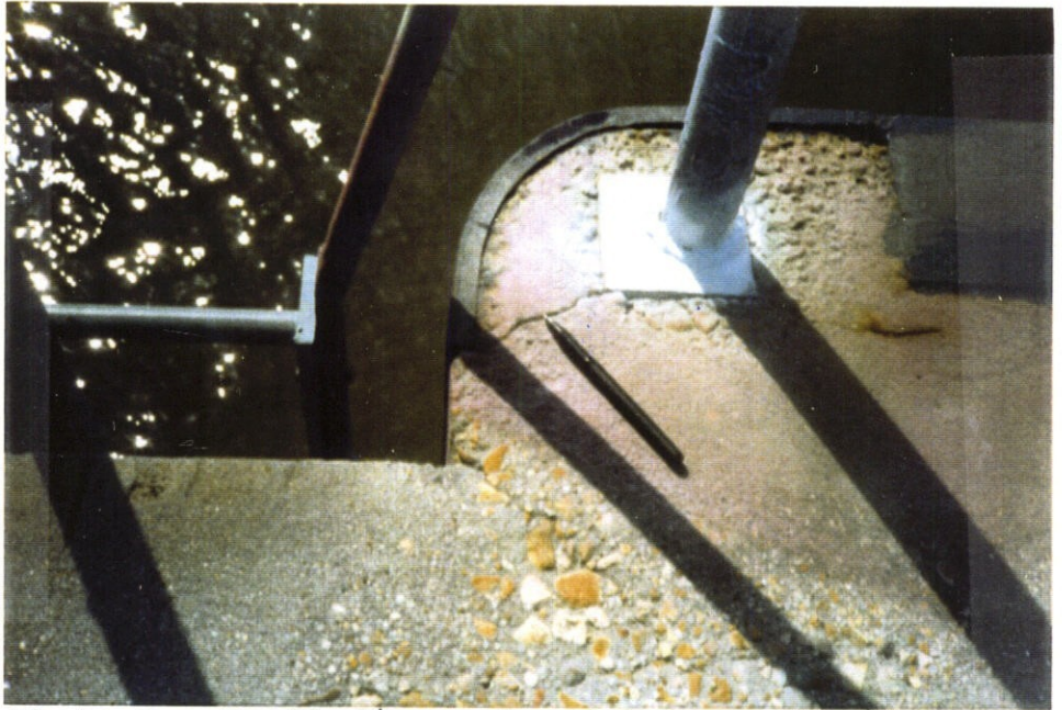
Photo 9 - Small diagonal crack on west side near edge of gatebay structure and handrail
