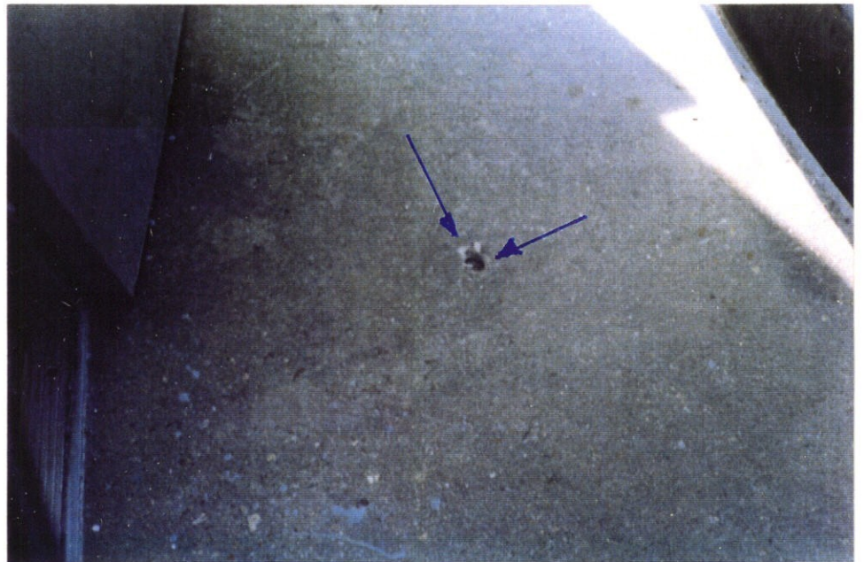
PHOTO 4 - Typical small spalls on top surface of gatebay monoliths and channel walls on both east and west sides
