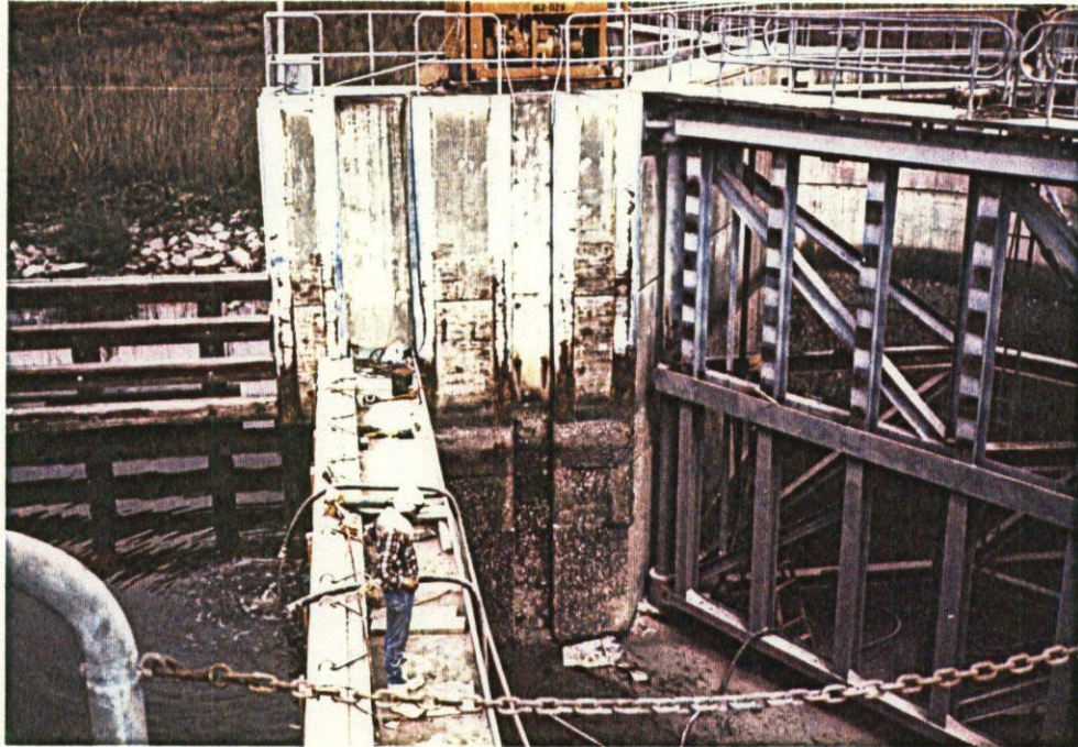
Photo No. 5 - Notice surface corrosion on steel members embedded in concrete. (18 March inspection)
