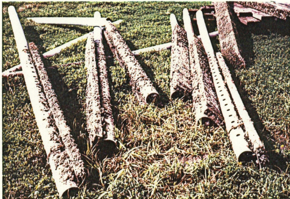
Photo No. 4 - Members of old cathodic protection system. Notice barnacle overgrowth. Old system was entirely replaced. (18 March inspection)
