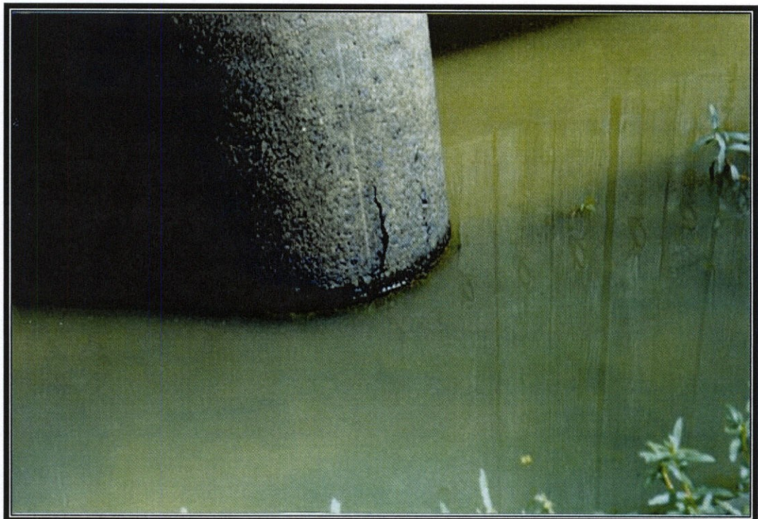
↓ PHOTO NO. 2 - A SPALL IS LOCATED ON THE RIVERSIDE FACE OF PIER 190-191 NEAR THE WATERLINE.
