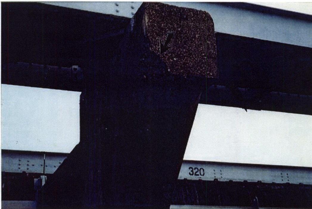
PHOTO 8 - Medium size spall on the riverside bridge bent of pier 319. The spall appeared to be old and no action is required at this time.
