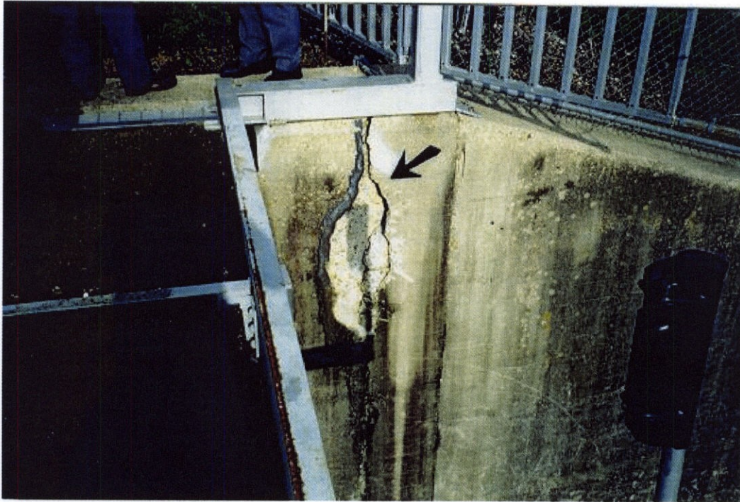
PHOTO 9 - Large spall on west abutment wall, noted during previous periodic inspections appeared to be the same. This spall is about 3 feet down-stream of the lakeside bridge where bridge span no. 1 channel beams rest on the abutment wall and should not affect the bridge.
