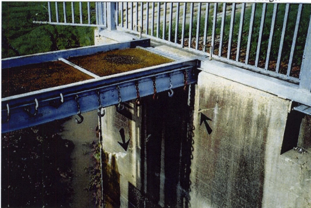
PHOTO 10 - The deep and fine arched crack under the riverside bridge, noted during previous periodic inspections has not changed.
