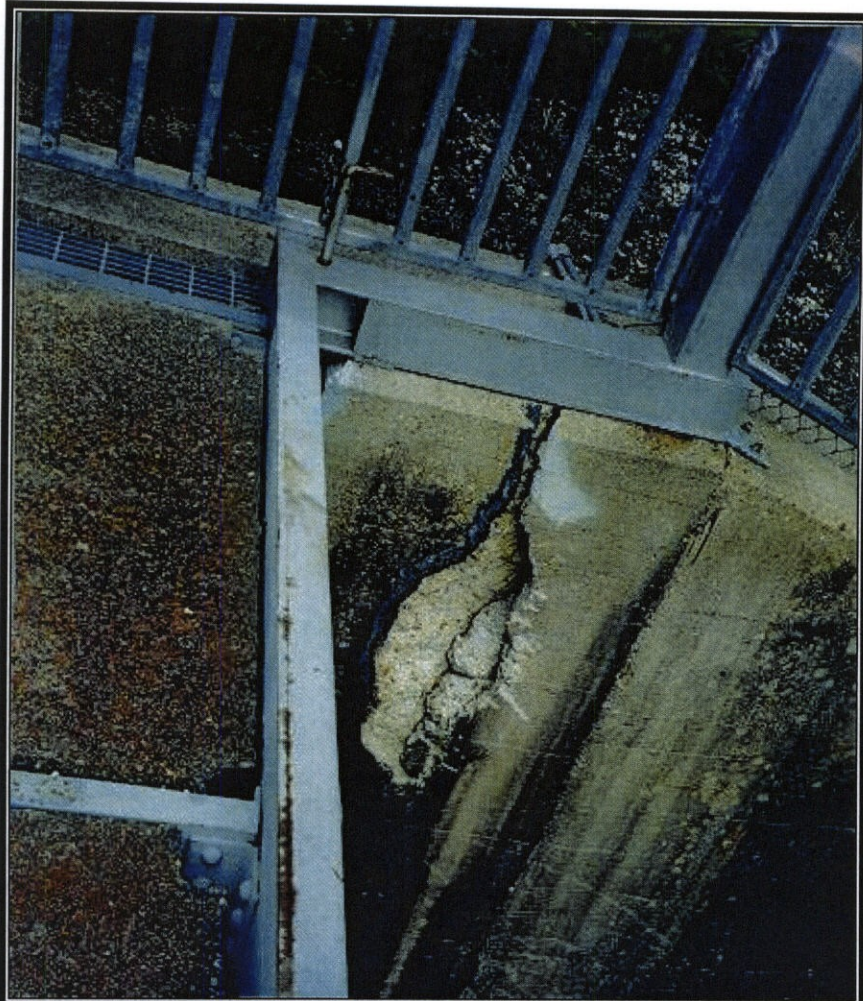
← PHOTO NO. 5 - SHEARED FEMALE KEY ON THE DOWNSTREAM SIDE OF THE ABUTMENT.
