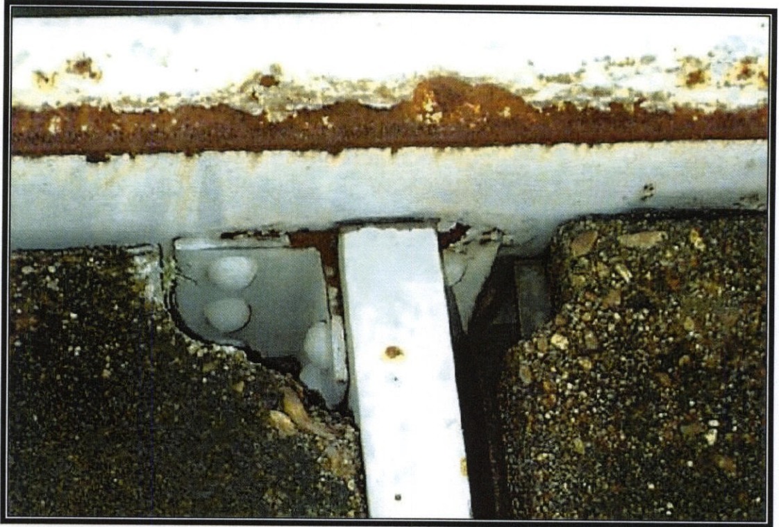
↑ PHOTO NO. 13 – CLOSE-UP OF RUST ON CRANE/SERVICE BRIDGE COMPONENTS.
