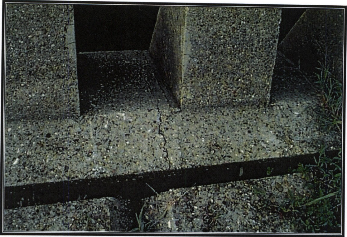
↑ PHOTO NO. 7 – ONE OF SEVERAL CRACKS AT DOWNSTREAM END OF STILLING BASIN.
