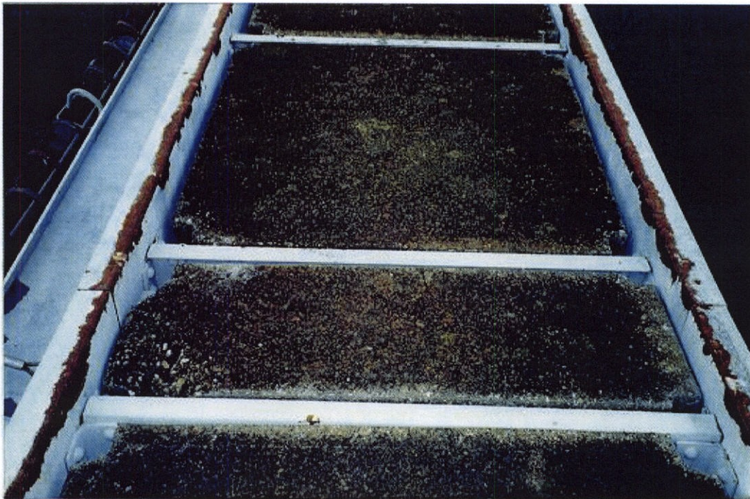
PHOTO 6 - Typical close up of concrete walkway panels, note top portion of the Channel beam (which the crane and engine driven rail car ride) are beginning to show signs of rust.
