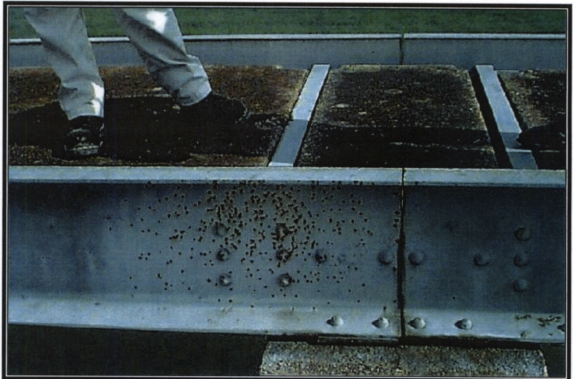
↓ PHOT NO. 14 – TYPICAL SPOT RUSTING ON THE C CHANNELS OF THE CRANE/SERVICE BRIDGE.
