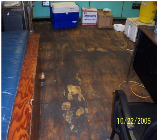
Photo 1 – Missing tiles and damaged floor in control room
