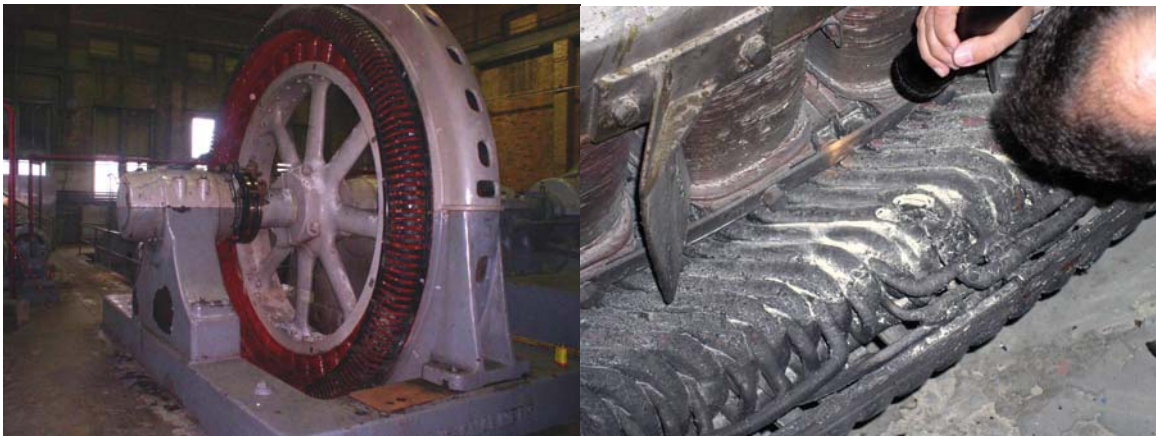
Figure 6. Typical pump motor arrangement
