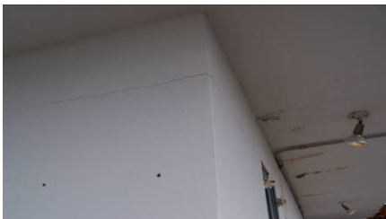
Photo 1—Wall Crack Below Roof
