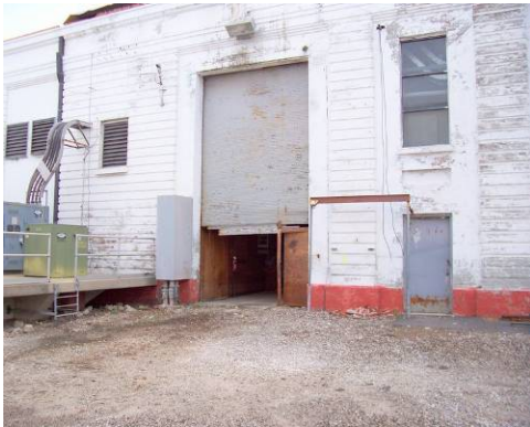
Photo 1 – Damaged roll-up door.
