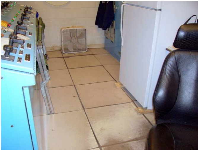
Photo 3 – Damaged tiles in control room.
