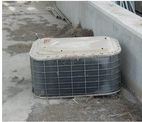
Photo 2—Damaged Air Conditioner
