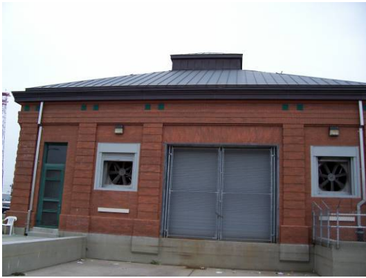
Photo 1 – Roof ridge flashing missing; west end of bldg.
