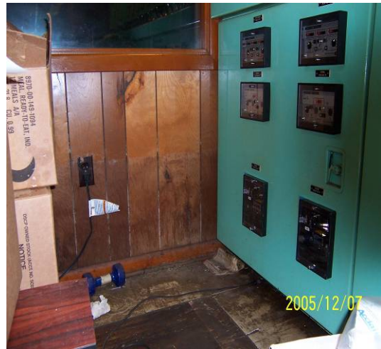
Photo 2 – Damage to walls in control room.
