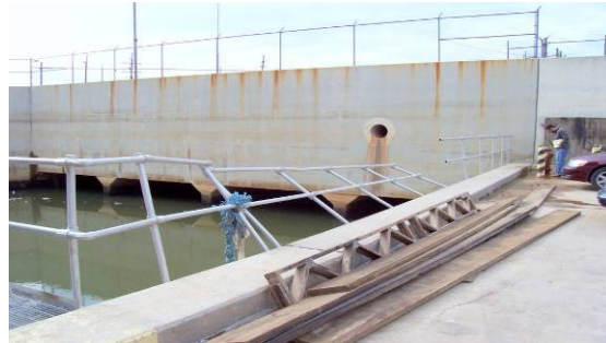
Photo 2—Damaged Pipe Rail
