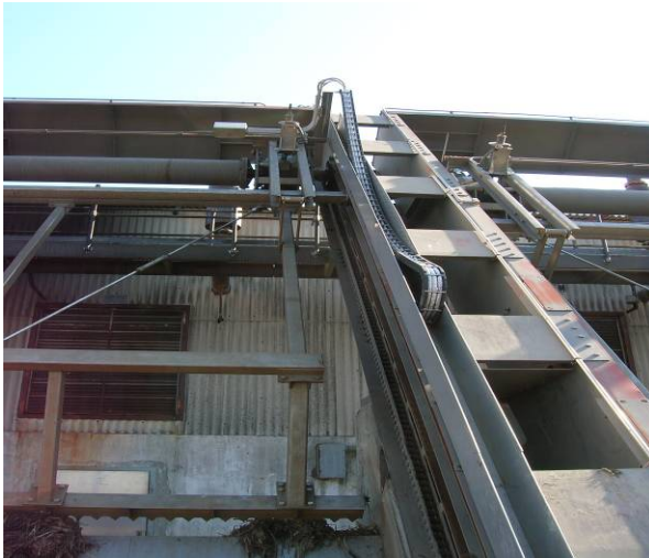
Photo 1—Damaged Trash Rake Cable Tray
