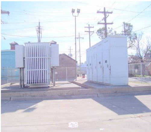
Photo 1—Outdoor Electrical Equipment
