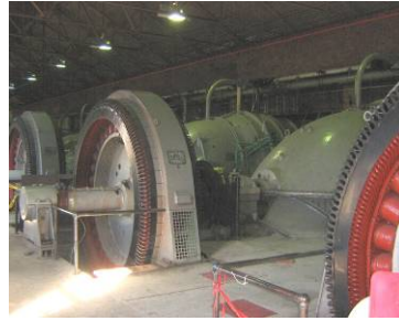
Photo 2 – 25 cycle pump motors to be rewound.
