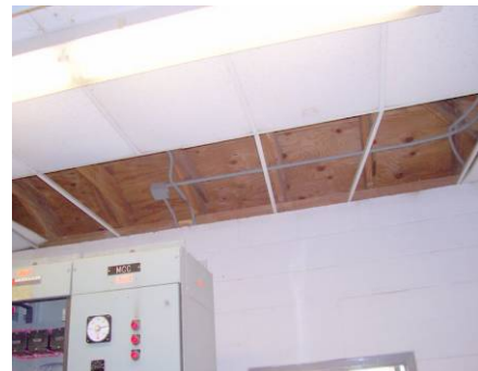
PHOTO 2 – DAMAGED CEILING TILES
