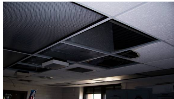
Photo 2—Damaged Ceiling Tiles
