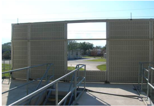
Photo 2 – Damaged Noise Reduction Panels
