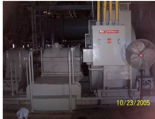
Photo 2 – Motor for drainage pumps A & D.
