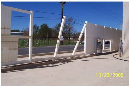
Photo 3 – Damaged vinyl fence.
