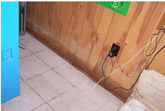
Photo 3—Damaged Floor and Wall
