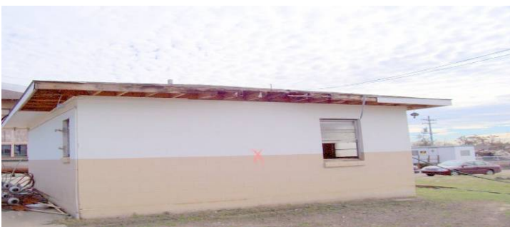
PHOTO 3 – DAMAGED OIL STORAGE BLDG.
