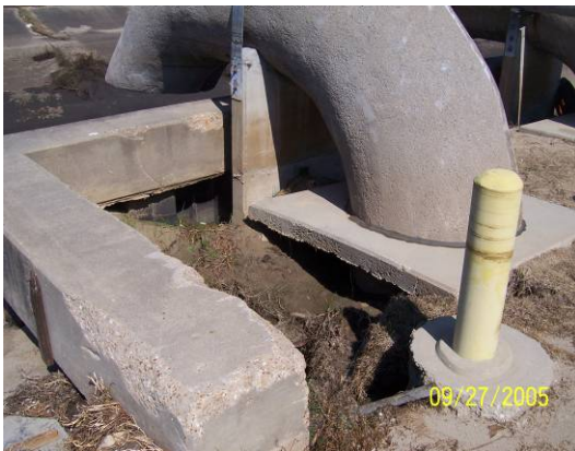
PHOTO 3. SCOUR AT DISCHARGE PIPES
