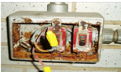
Photo 3. Damaged Low Voltage Wiring
