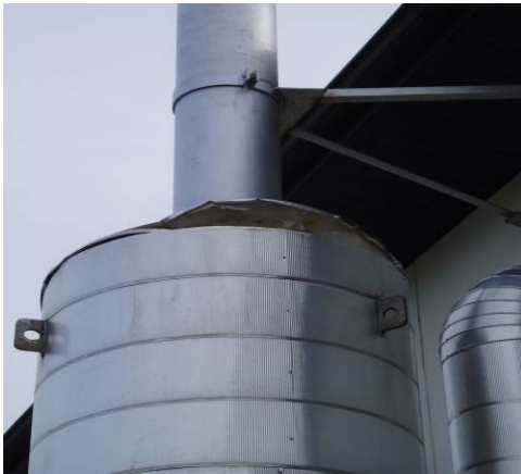
PHOTO. DAMAGED GENERATOR MUFFLER
