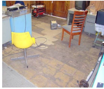
Photo 2 – Damage to control room floor.
