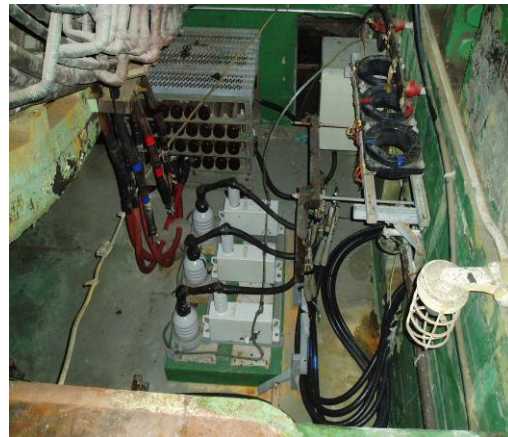
Photo 2 Motor Pit Equipment
