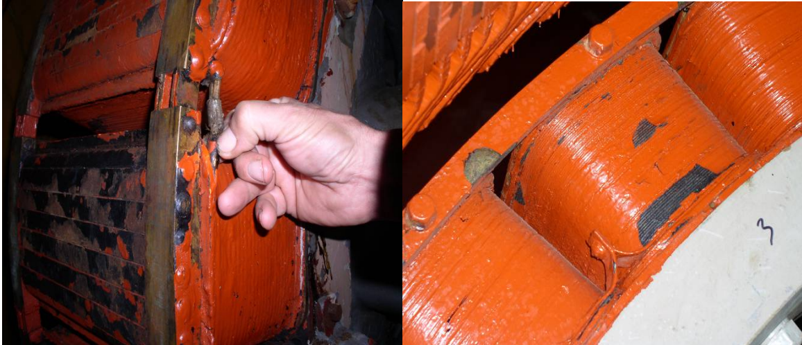
Figure 4. G.E. motor specialist shows sprayer damage Figure 5. Flaking and peeling coil insulation
