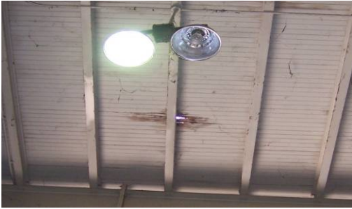
Photo 1 – Damage to roof.
