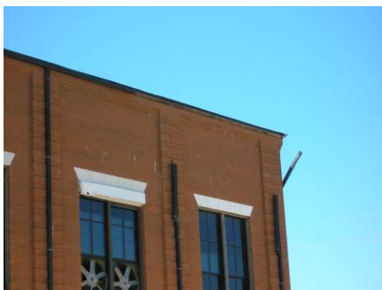
Photo 3—Damaged Gutter and Downspouts
