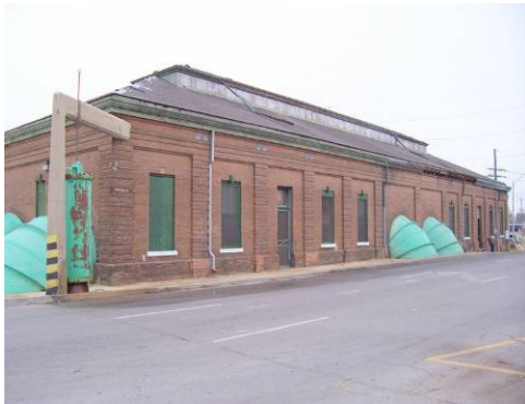
Photo 1 – Roof damage to station bldg.
