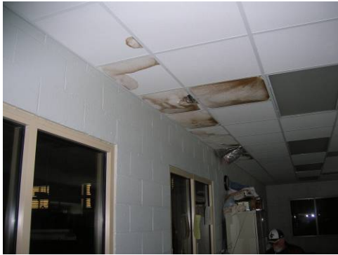
Photo 1 – Damaged ceiling tiles
