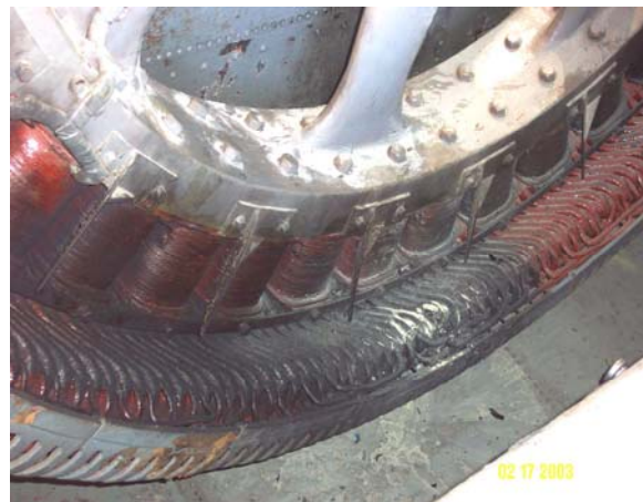
Photo 4 – Burned motor for Pump A.
