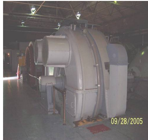
Photo 2—Pump D Protective Shroud
