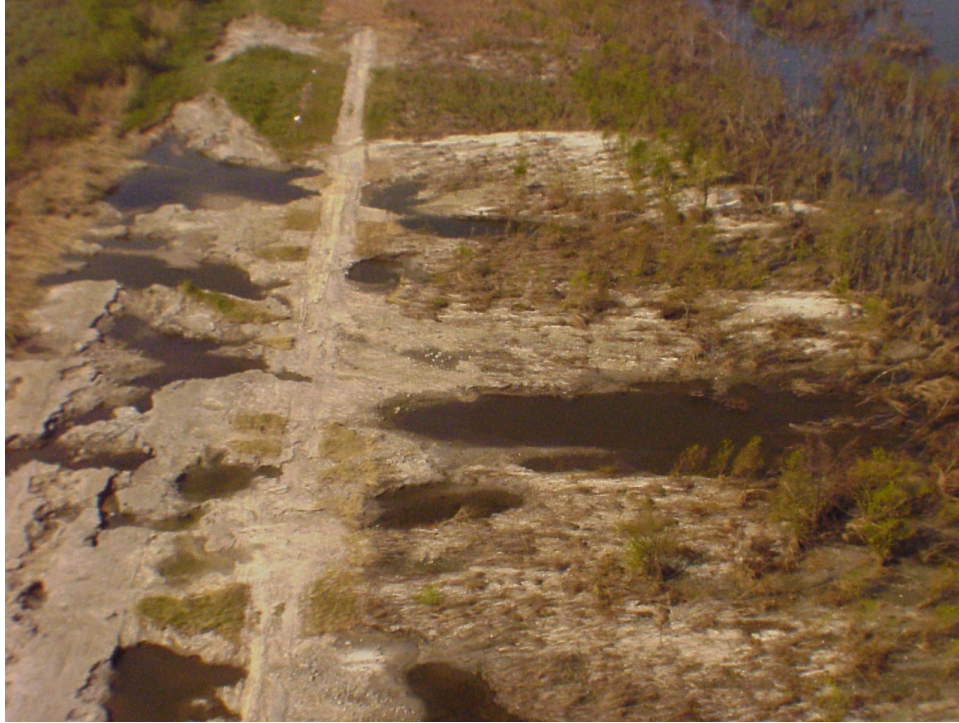
Figure J-B7. Failure of Levee by Overtopping East of PS #15 (East Back Levee)
