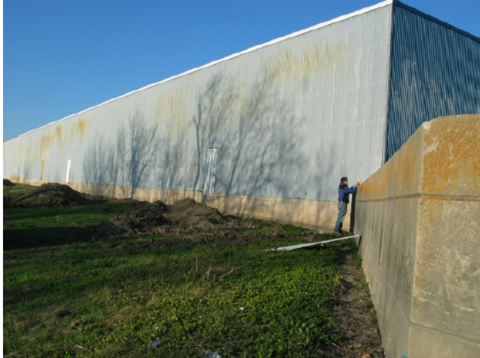
Figure J-B13. Floodwall Serves as Building Foundation (Dupuy Storage Facility – IHNC East)
