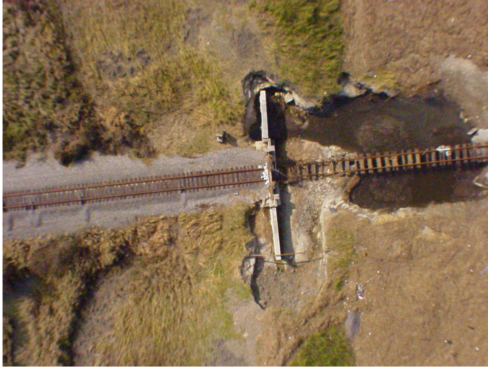
Figure J-B6. Aerial View of Damage at RR Closure Along East Levee (Point NOE12c on System Map)
