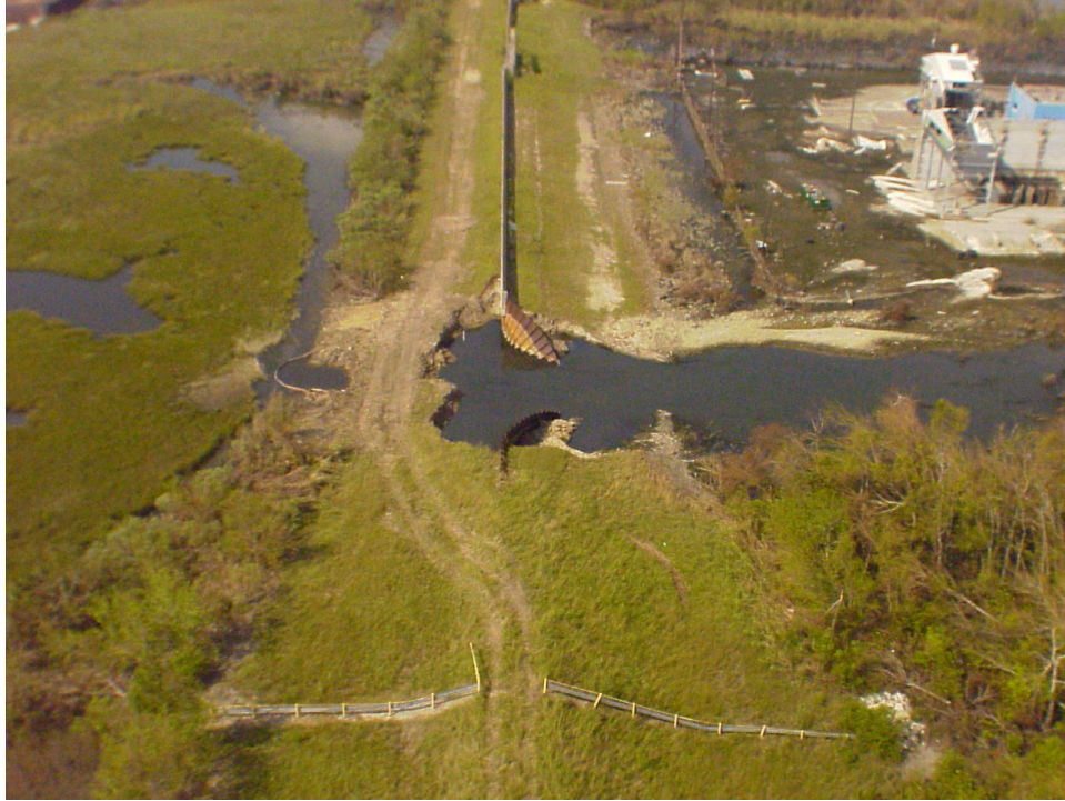
Figure J-B9. Floodwall Failure at East End of Michoud Canal FW
