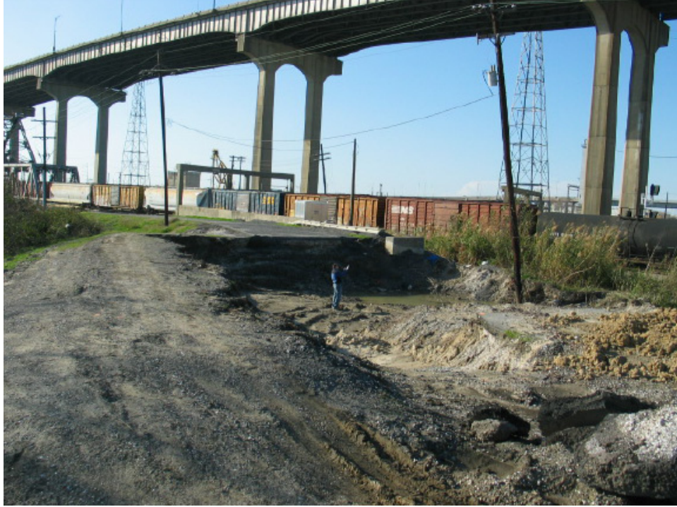
Figure J-B12. Major Washout Area from Overtopping Near I-10 Overpass (Citrus Back Levee)
