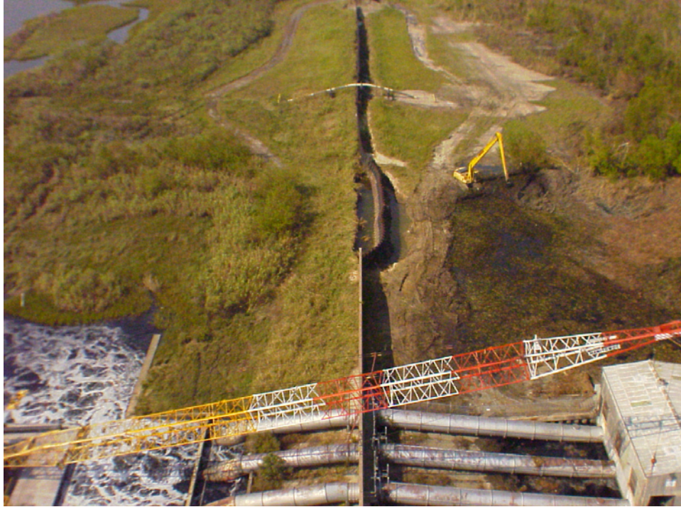
Figure J-B8. Floodwall Failure Near Orleans Pump Station #15
