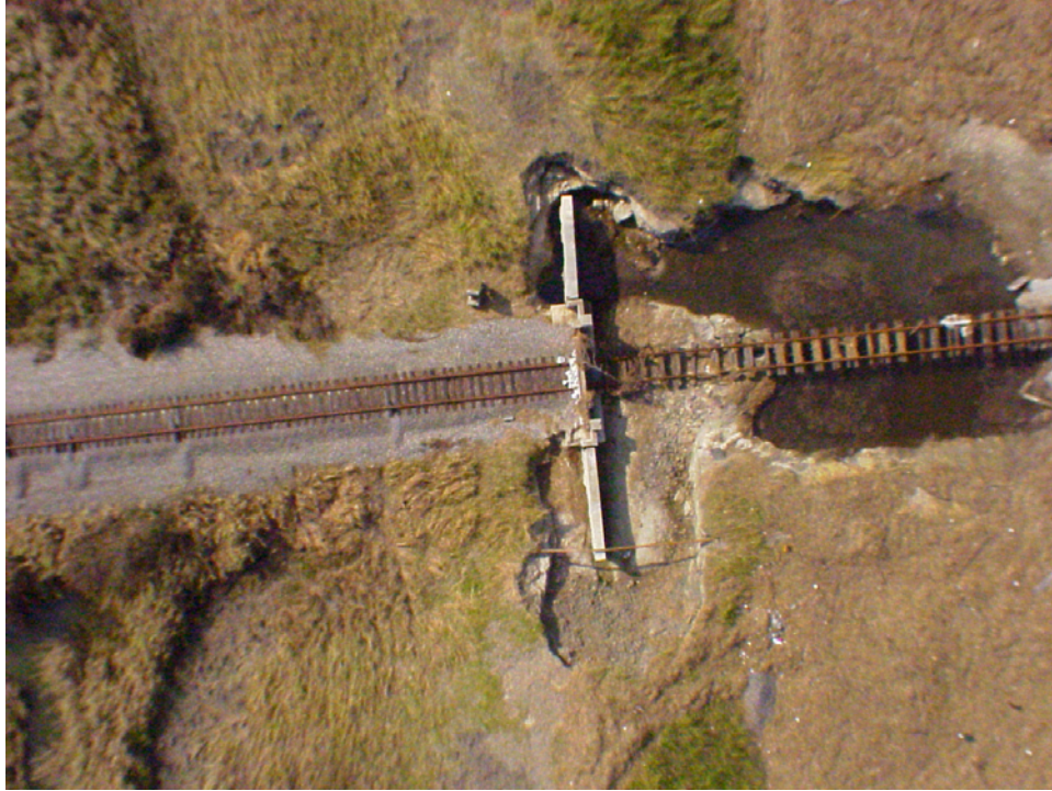
Figure J-B6. Aerial View of Damage at RR Closure Along East Levee (Point NOE12c on System Map)
