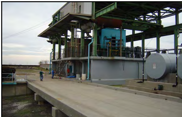
Post-Hurricane Katrina – View from the Inlet Canal
