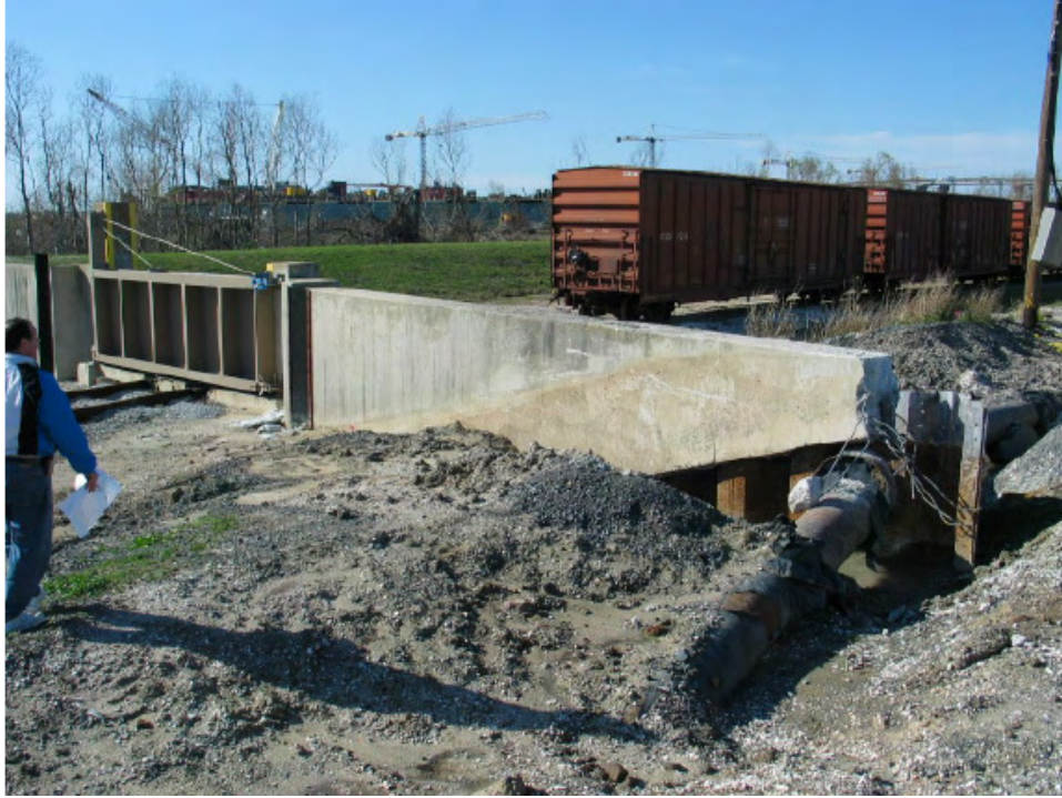
Figure J-B11. Erosion Damage Around RR Closure (Citrus Back Levee)
