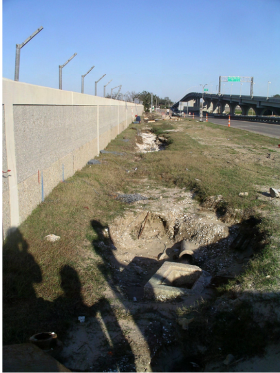
Figure J-B3. Scour Behind Lakefront Airport FW from Overtopping
