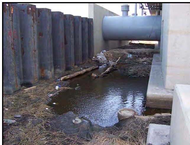
Post-Hurricane Katrina – Erosion
