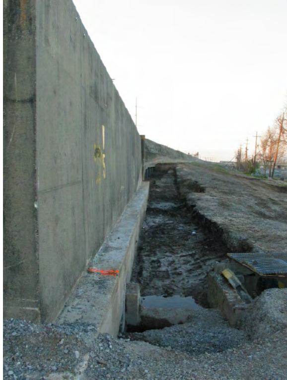
Figure J-B14. Erosion Behind Floodwall Adjacent to Gate E-13 (IHNC East)
