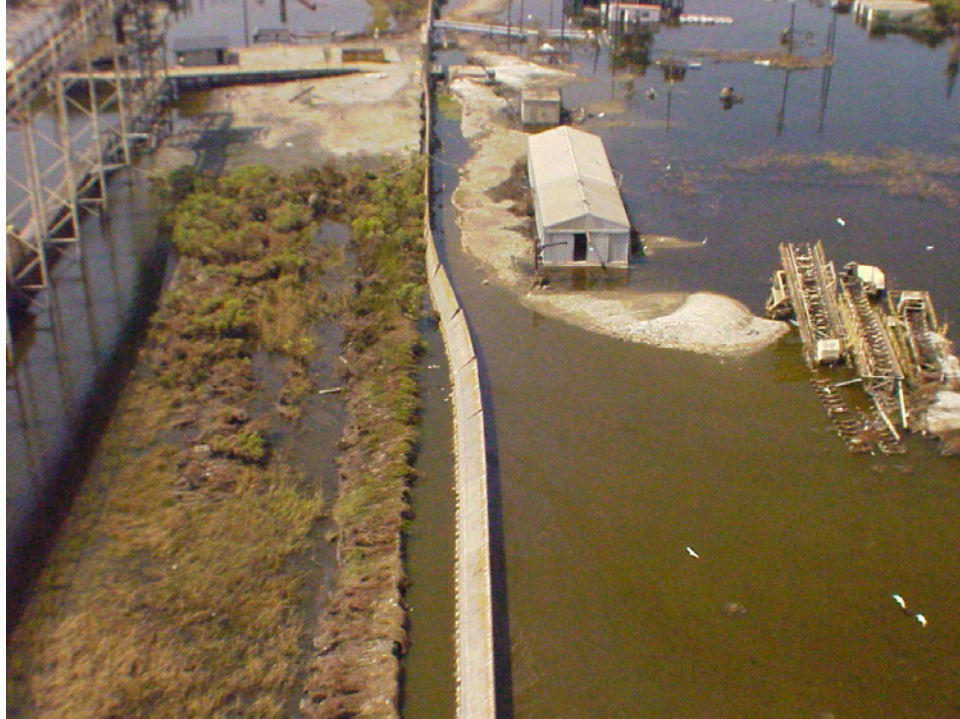
Figure J-B10. Floodwall Failure at Bulk Loading Facility/Elaine PS
