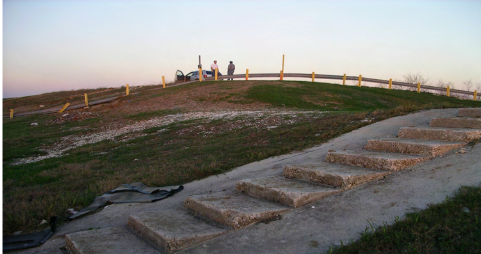
Figure J-B5. Begin Lakefront Levee at Citrus Lakefront and Paris Road (Lakefront Levee @ El. 19.0 +/- and Citrus Lakefront Levee @ 13.5+/-)
