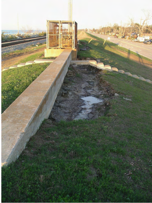
Figure J-B4. Minor Scour from Overtopping at Jahncke Pump Station
