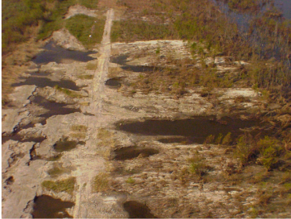
Figure J-B7. Failure of Levee by Overtopping East of PS #15 (East Back Levee)
