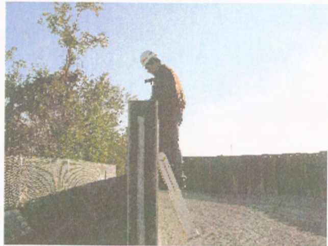
Photo 6 (Fig. 4) - Vertical downward impact to top of wall
