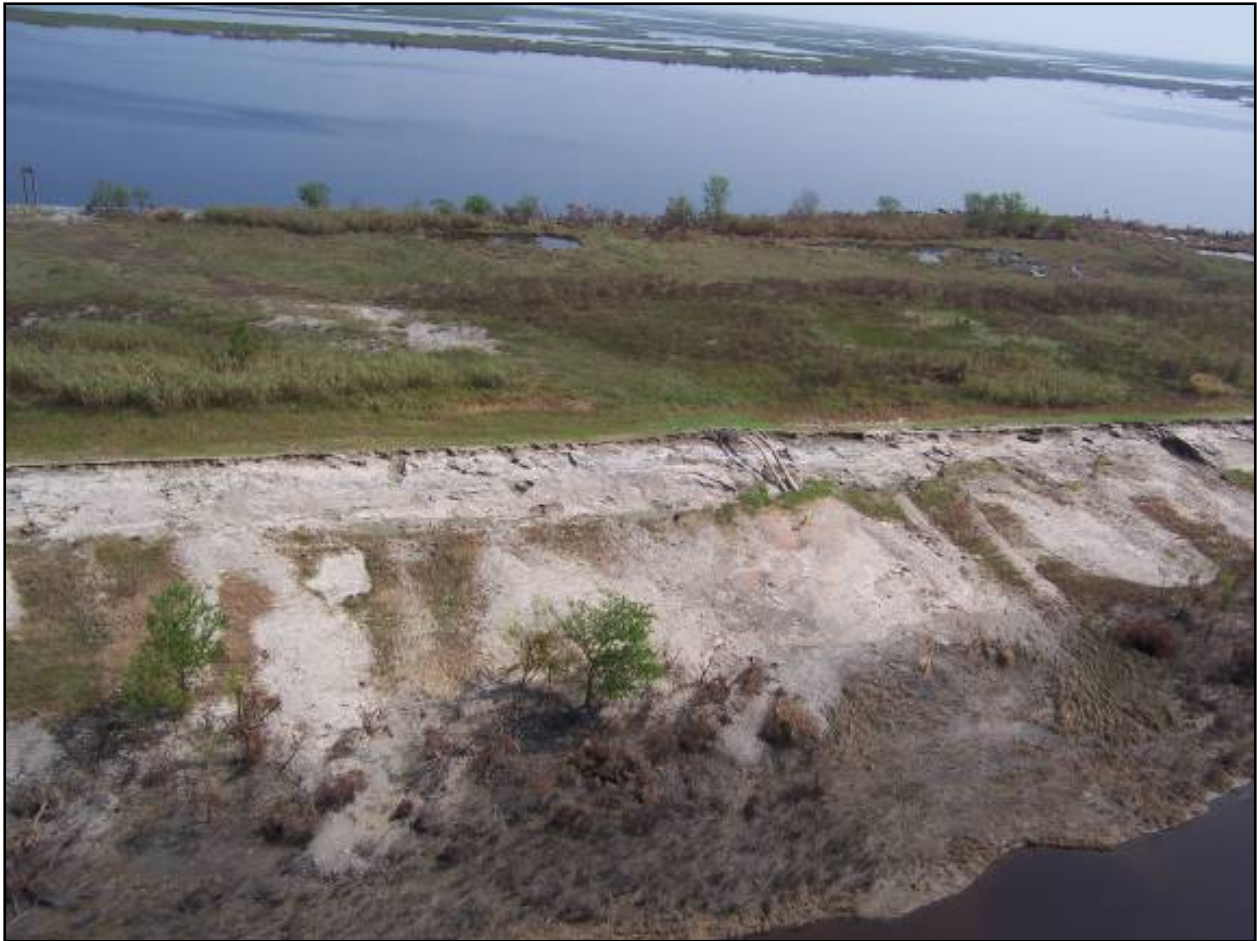
Figure 25. Stage D erosion between Bienvenue and Dupre structures, St. Bernard Parish
