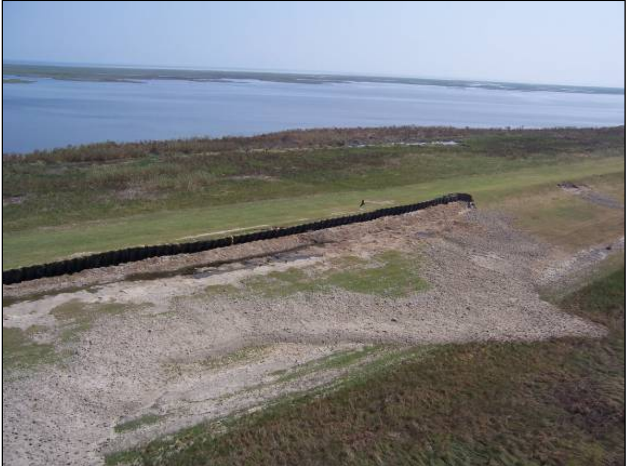
Figure 40. Sheetpile-to-levee transition showing significant scour behind the sheetpile and minimal erosion on the levee southeast of Dupre.
