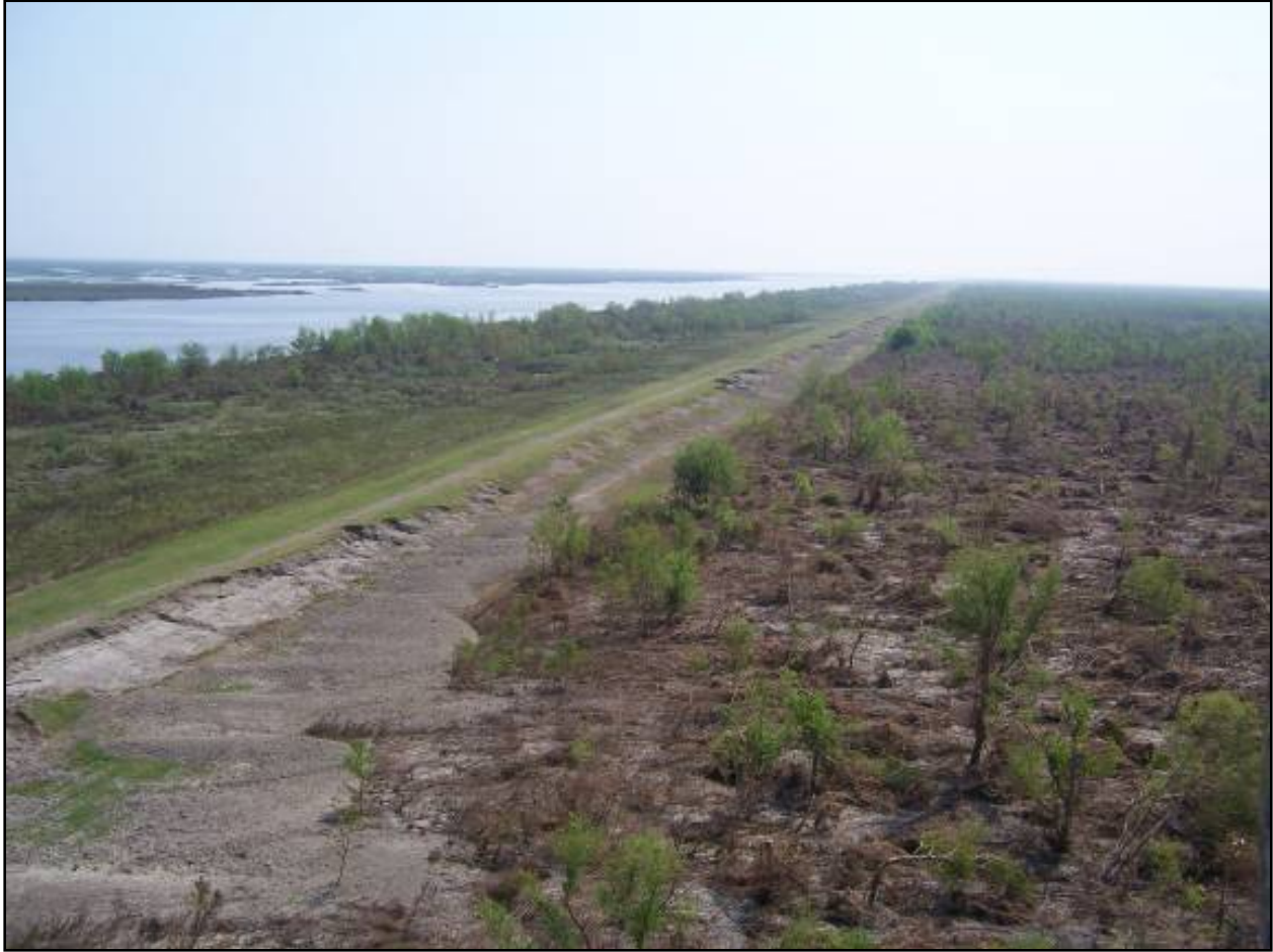
Figure 37. 2,500 ft. of levee from Dupre Control Structure to Sta 1007+91 that lost approximately 8' of elevation.
