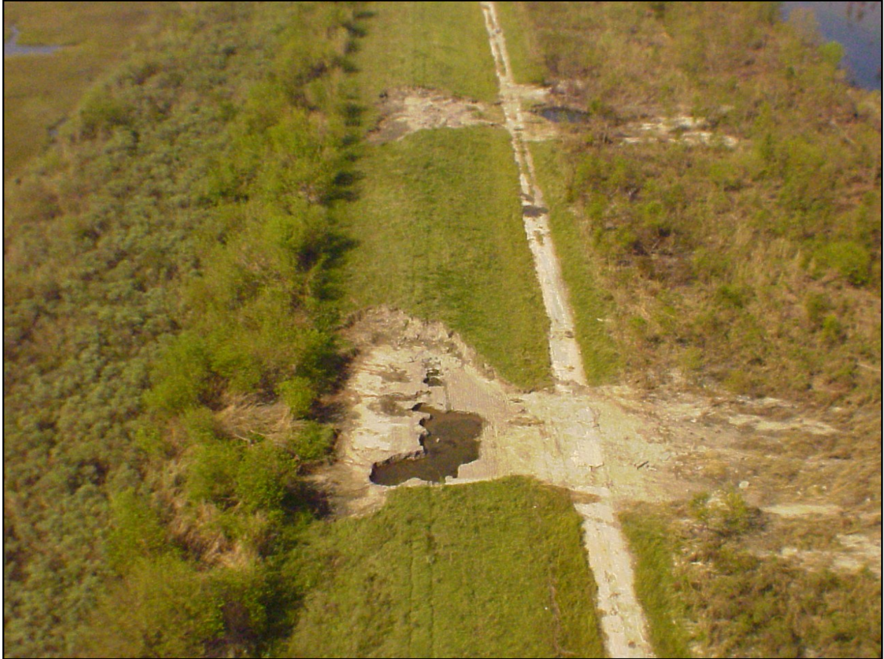
Figure 24. Localized Stage D breach east of pump station 15 on the East Back levee
