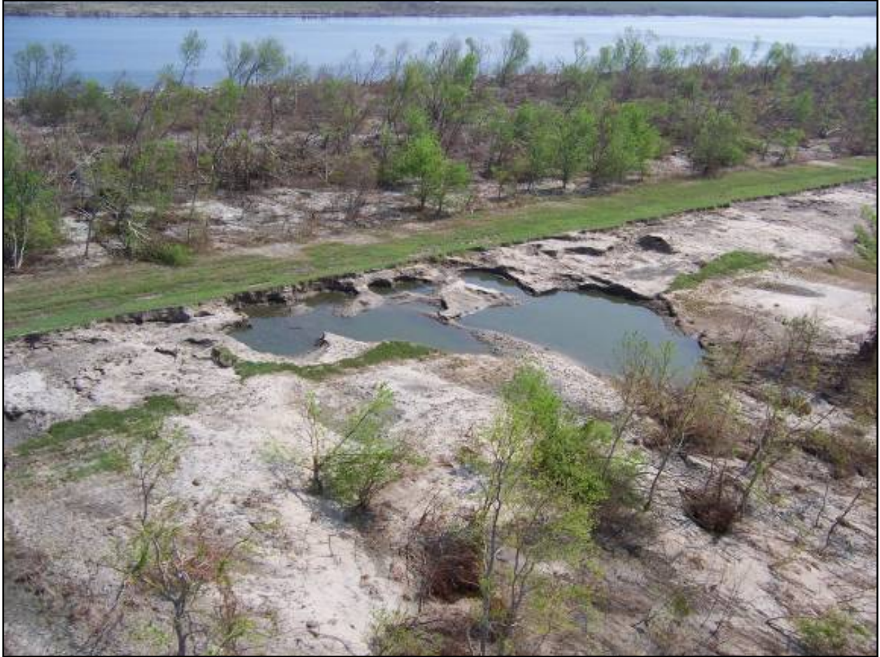
Figure 36. Stage D erosion southeast of Dupre Control Structure
