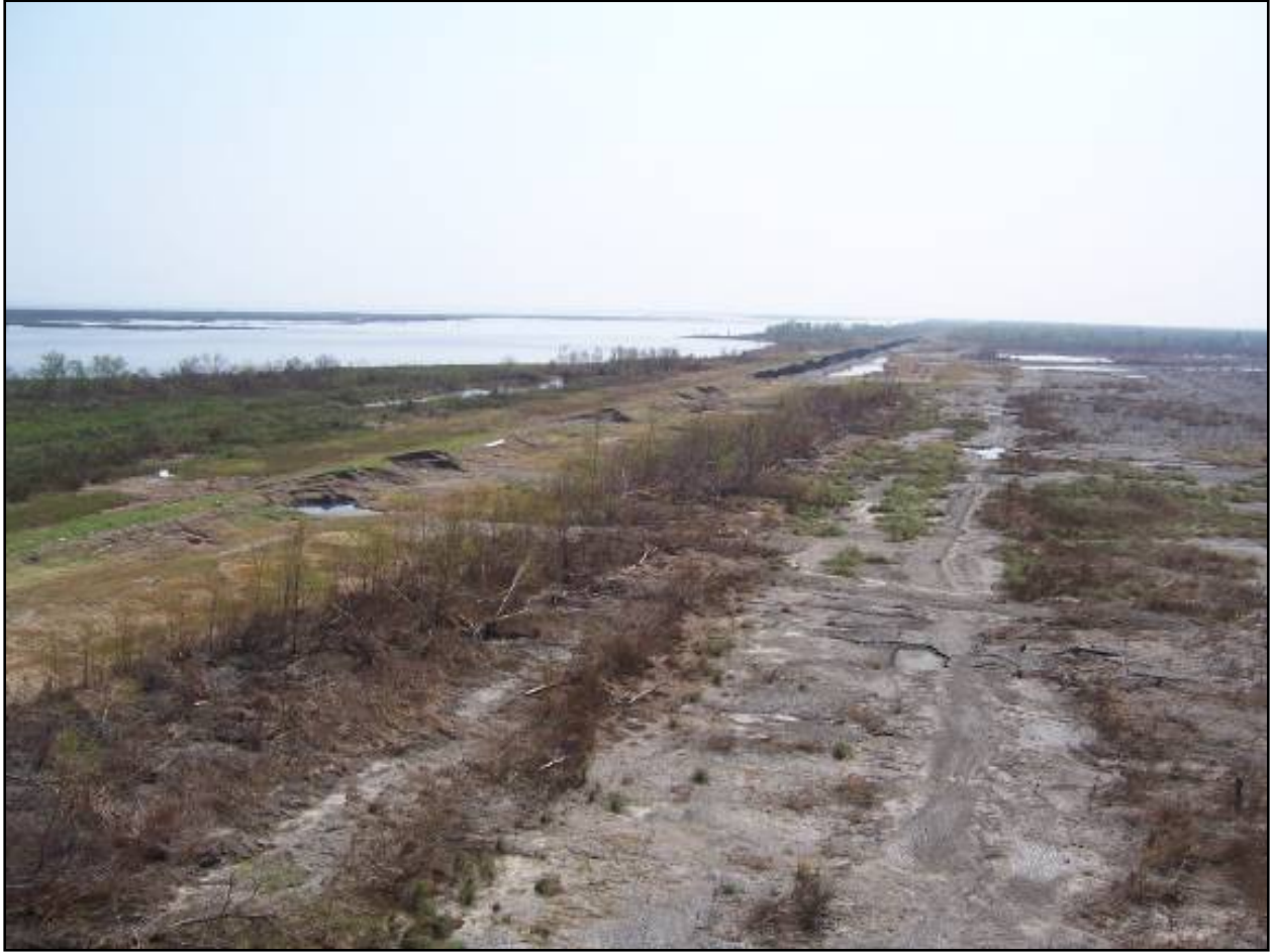
Figure 15. Stage B crown erosion on remaining levee southeast of Bienvenue Control Structure
