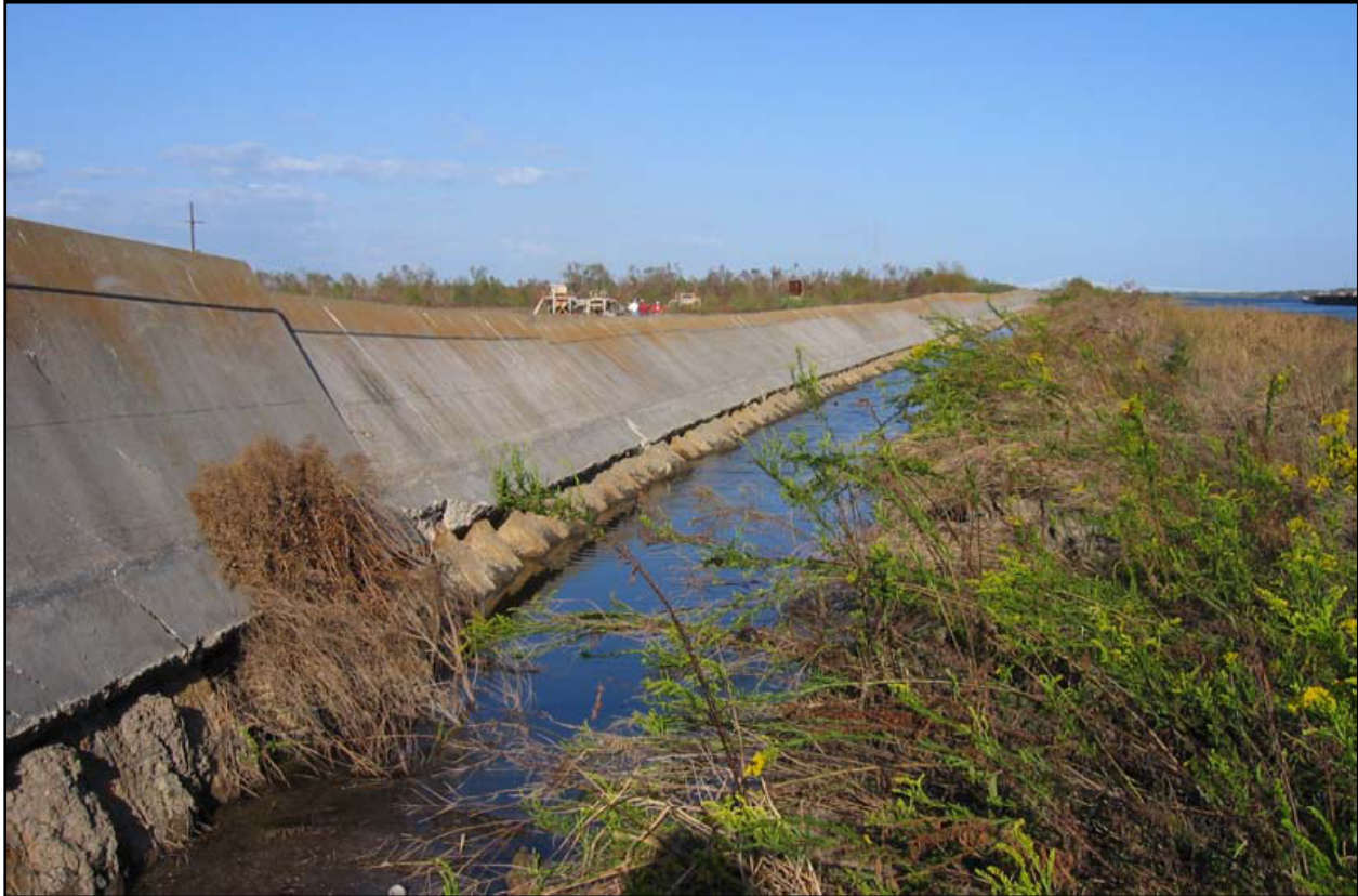
Figure V-17-40. Deflection and tilting of Citrus Back Levee I-wall
