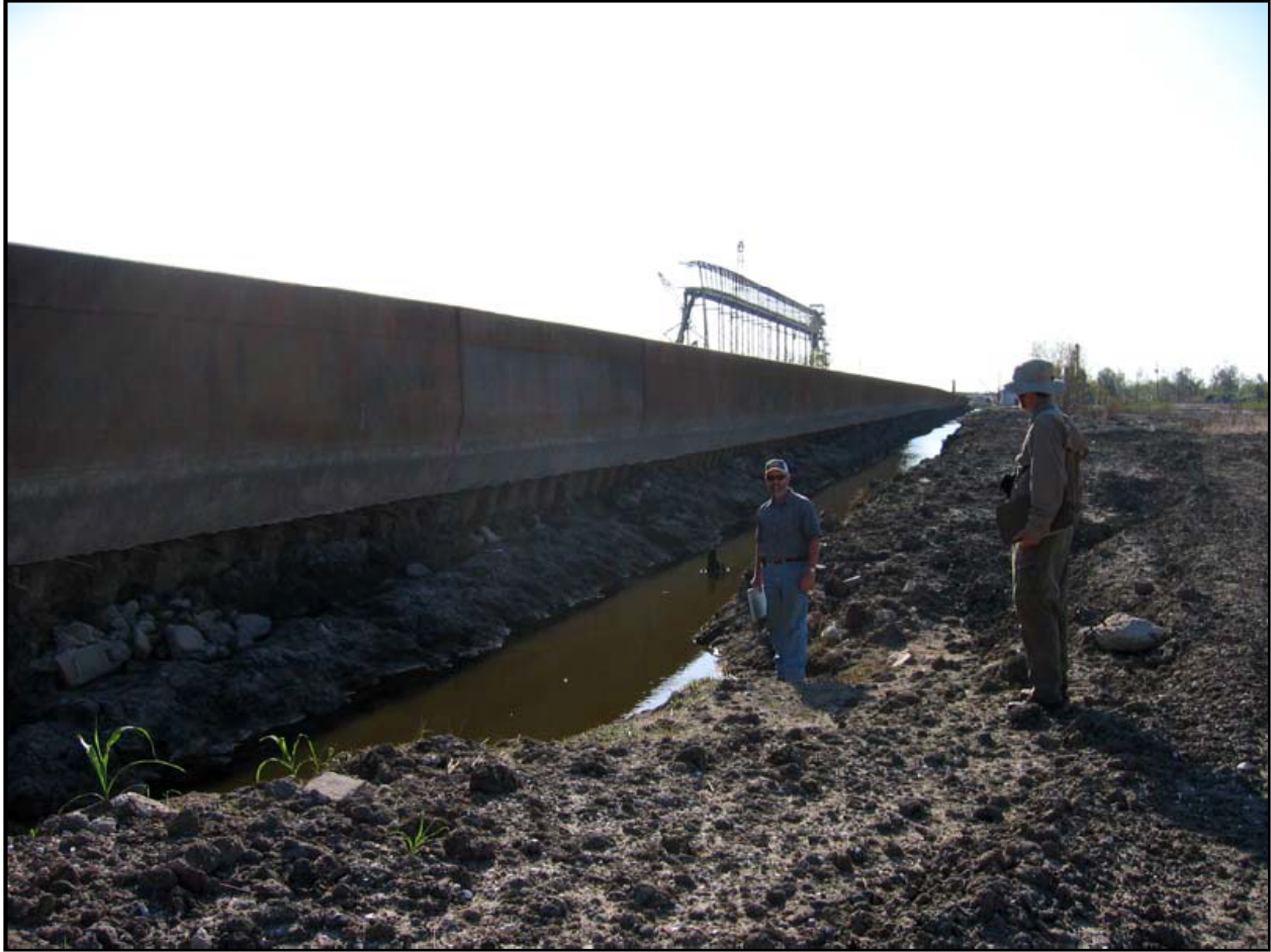
Figure V-17-38. Scour trench on the protected side of Citrus Back Levee I-wall. (Figure 7.14, NSF-Berkeley report (ILIT Final Report, July 31, 2006)
