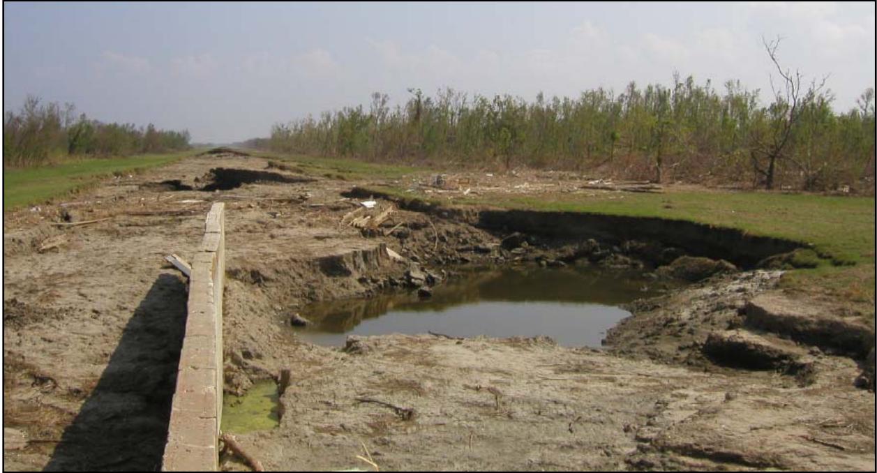
Figure 35. Stage D scour at the floodwall / levee at the southeast side of Bayou Dupre control structure
