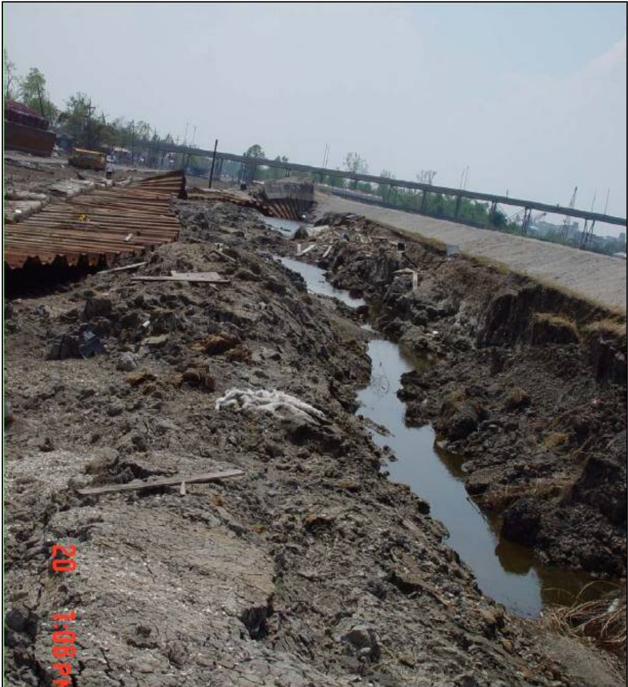
Figure V-17-37. Scour and Erosion Leading to the Failure of the I-Wall on the IHNC adjacent to the South Breach (Lower Ninth Ward)
