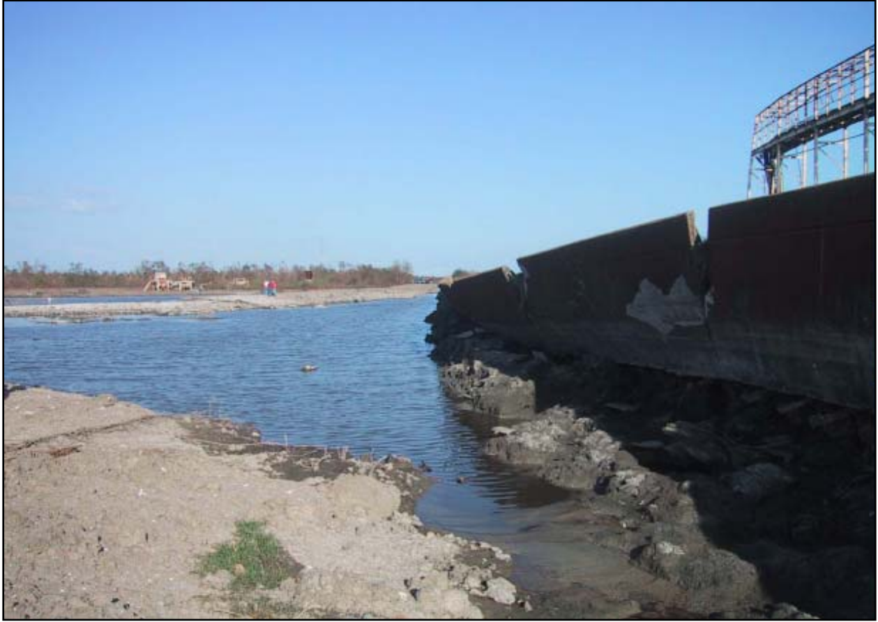
Figure V-17-39. Another section of the Citrus Back Levee I-wall showing erosion of the levee, lateral deflection, and tilting from overtopping
