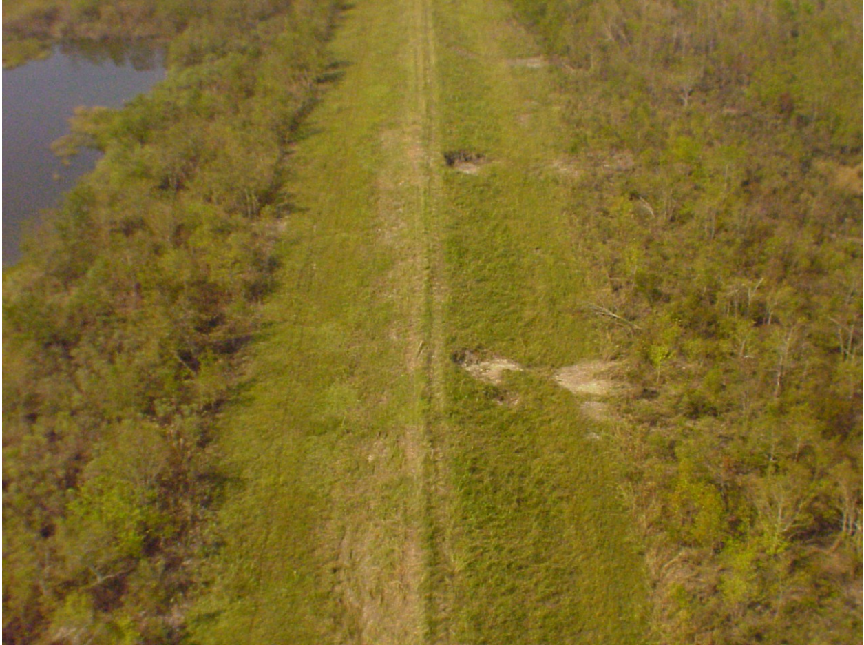
Figure 5. Stage A erosion on the Citrus Back Levee
