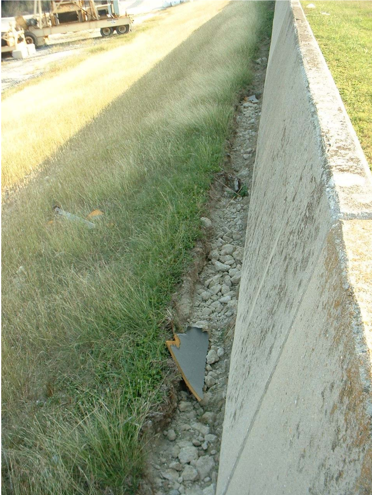
Figure 2b. Post-Katrina Photographs of Michoud Canal I-Wall showing erosion from overtopping waves.
