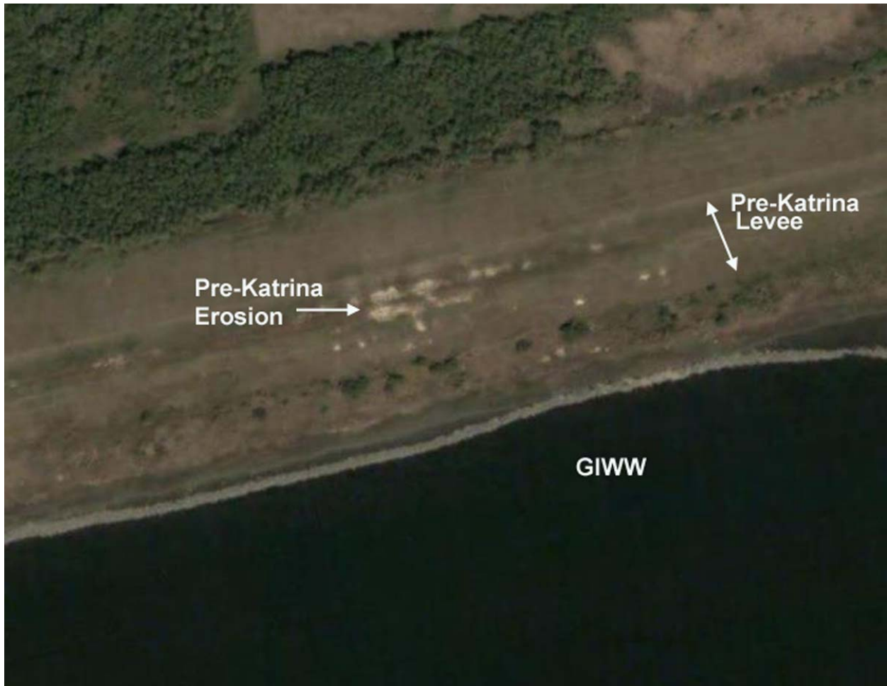
Figure 8. Possible pre-existing surface erosion on levee slopes along the north bank of the GIWW (Citrus Back Levee) at N 30deg 0 min 7 sec W 89deg 58min 31 sec. (pre-Katrina image from GoogleEarth website). Possible erosion is evidenced by vegetation distress and bare spots along the levee.
