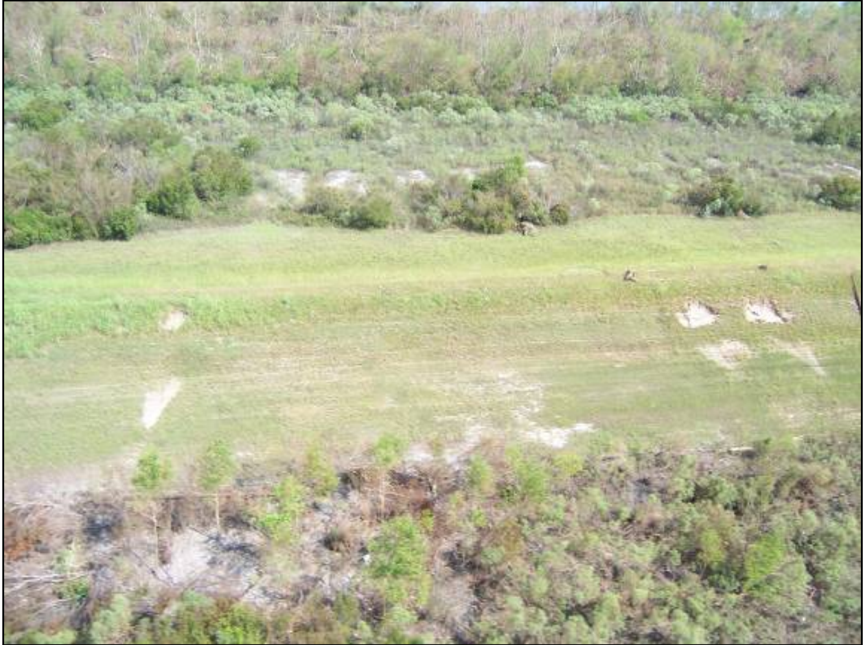
Figure 9. Stage A erosion on south bank GIWW levee, St. Bernard Parish
