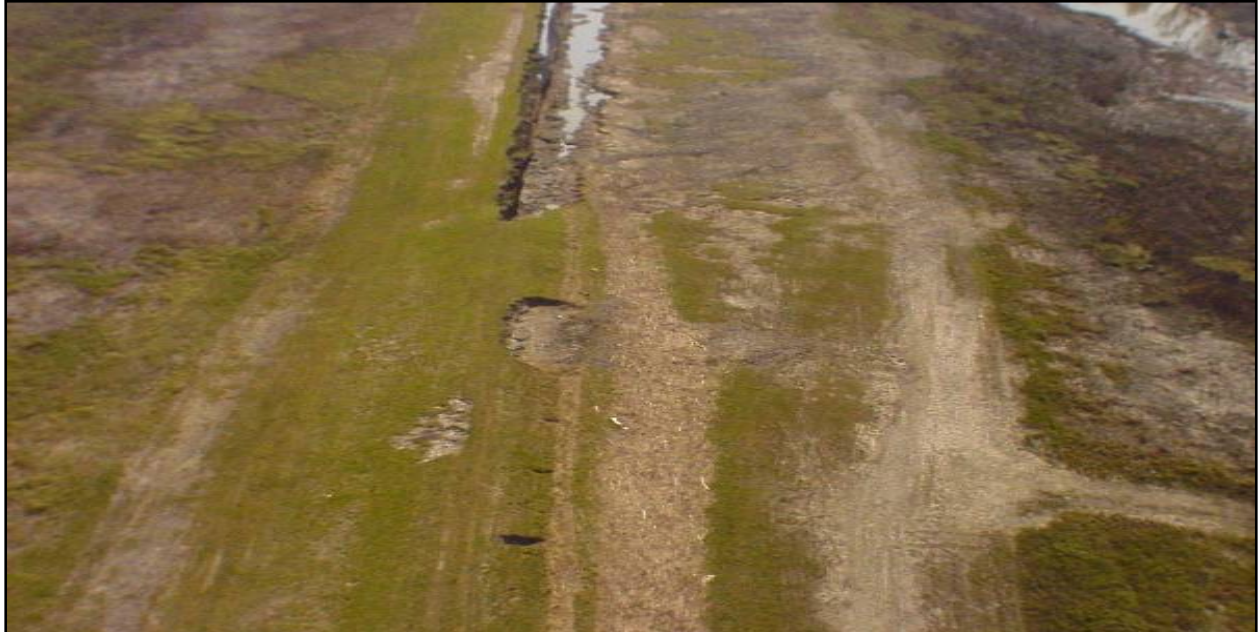
Figure 18. Stage C breach development on short reach of levee between Verret and Caernarvon
