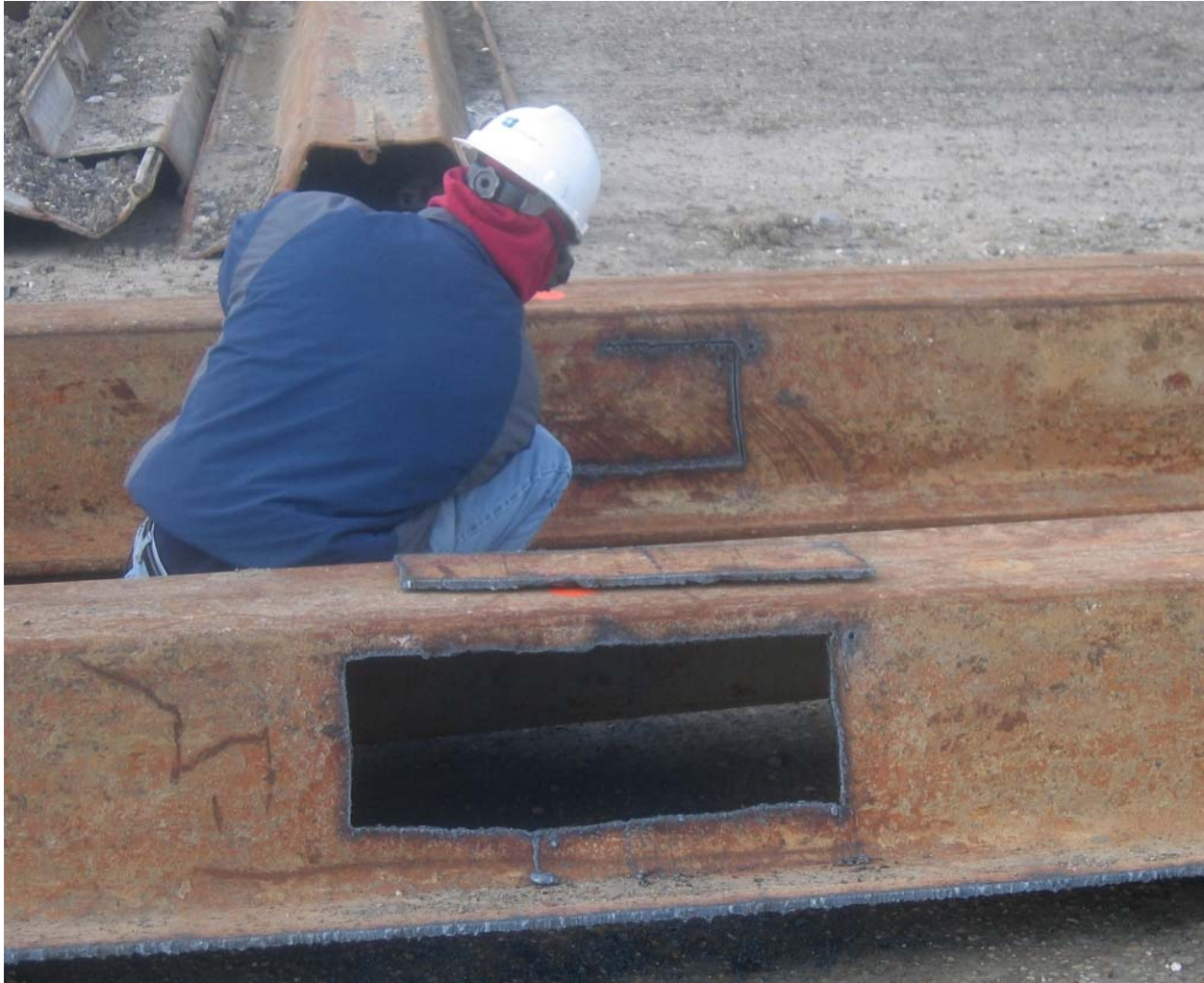
Figure 16-3. Flame Cutting Material Samples from Sheet Piling IHNC-SP-WS-B1
