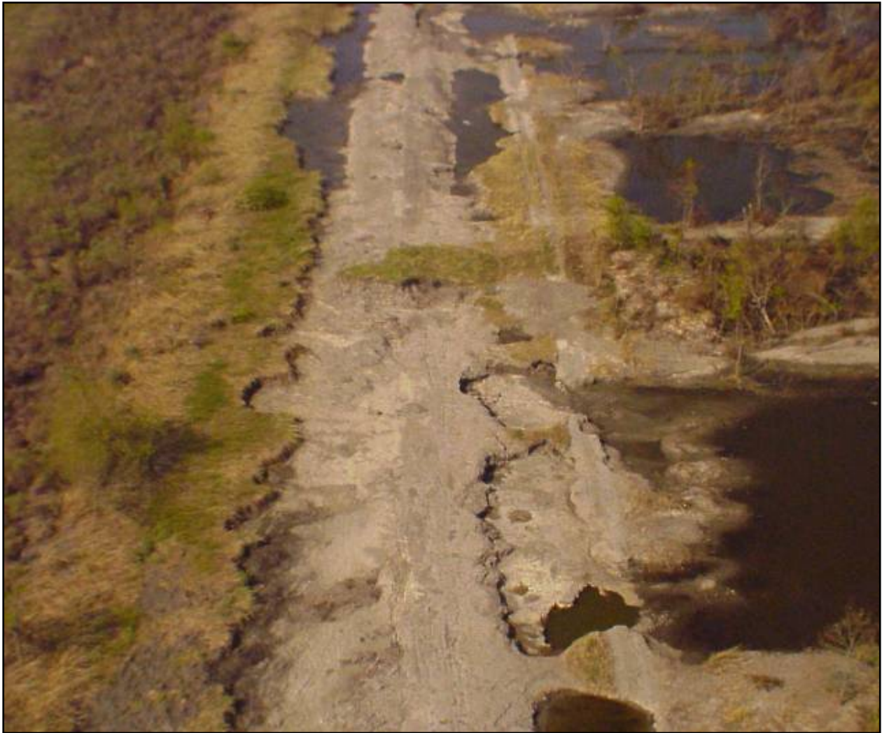
Figure 21. Stage D erosion east of pump station 15, N.O. East Back levee
