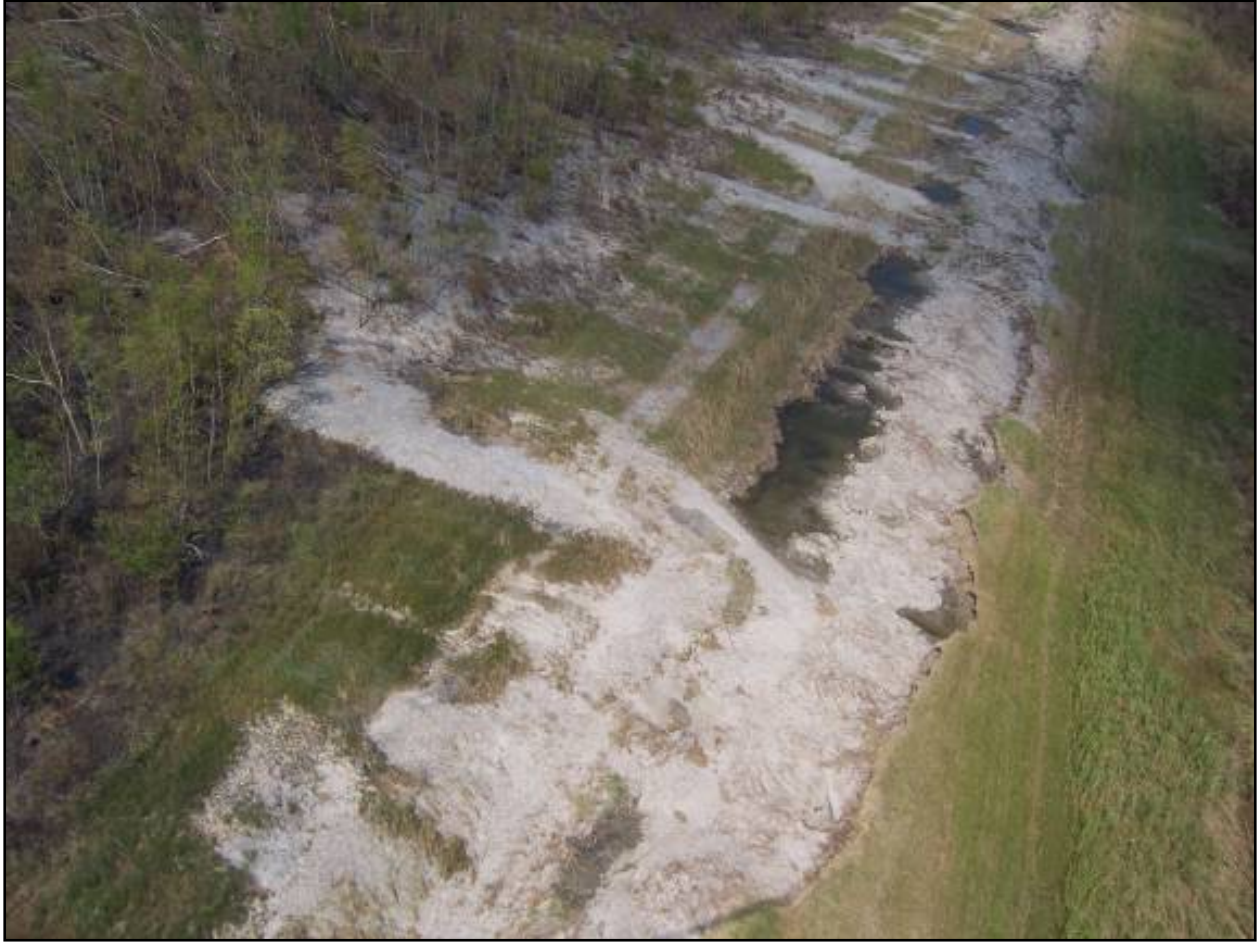
Figure 26. 2,300 ft. of levee between Bayou Bienvenue (Sta 383+00) and Bayou Dupre (Sta 704+00) that only lost 50% of original height.
