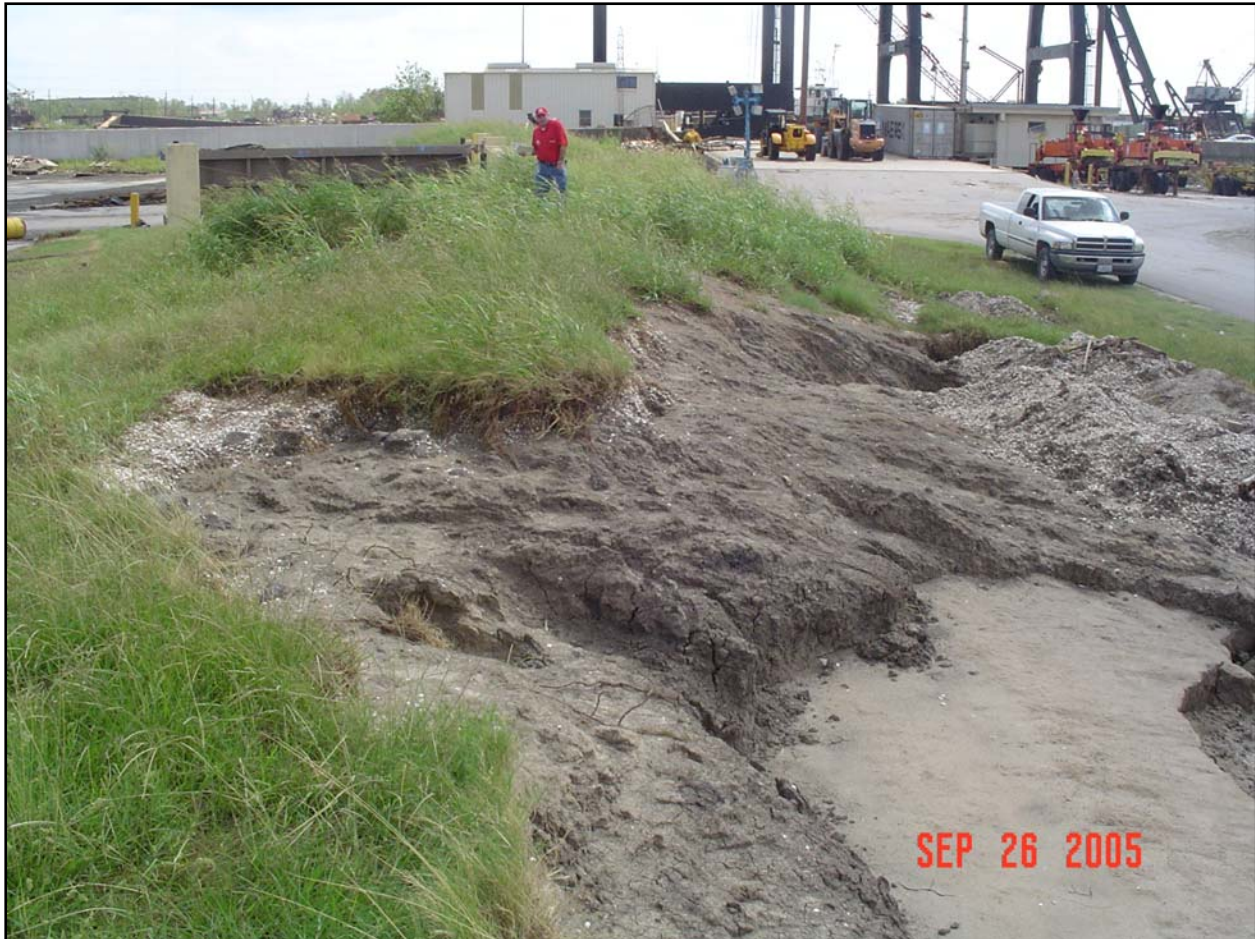
Figure 14. Crown erosion (stage B) on the remaining west side IHNC levee between IHNC and France Rd. ramp
