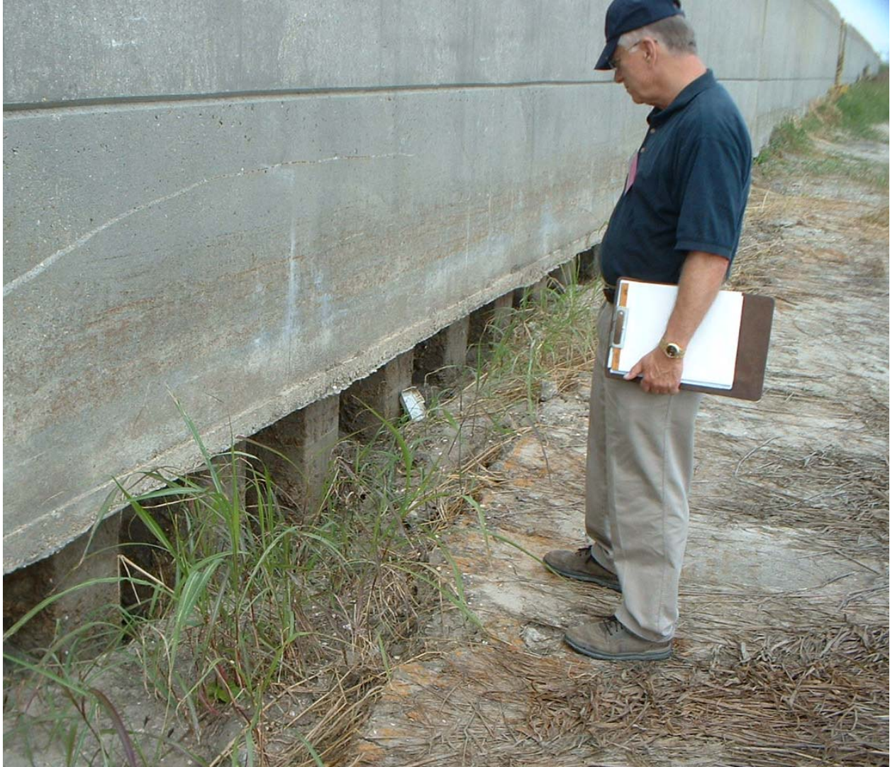
Figure 2a. Post-Katrina photographs of Michoud Canal I-Wall at pump station.
