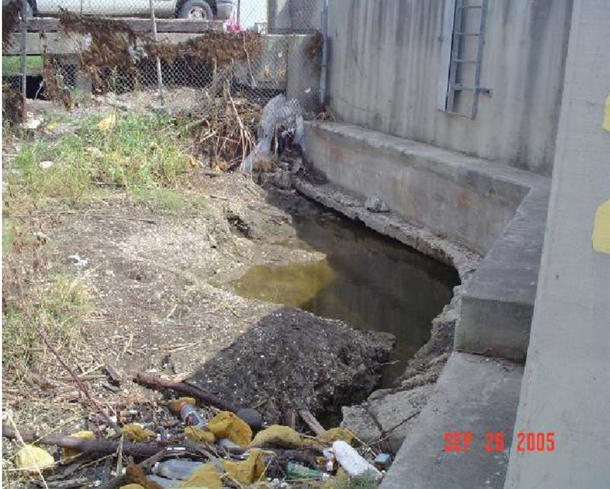
Figure 13-17. Scour at T-Wall Base of Gate W23, West Side IHNC
