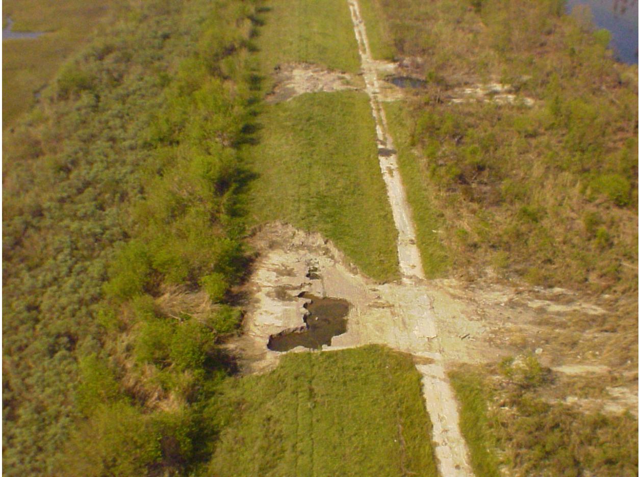
Figure 13-62. Partial Breach East of Pump Station 15
