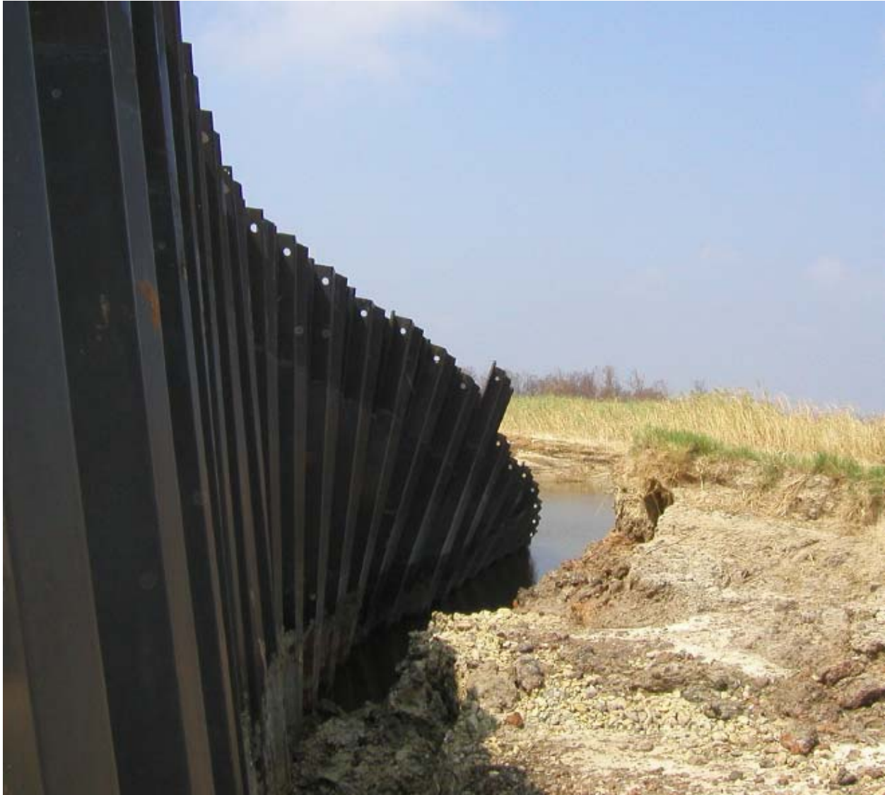
Figure 13-27. Closeup of Adjacent Breached Sheetpile with Backside Scour. Note the stratified layers in the soil profile representing existing hydraulic fill historically dredged from the MRGO
