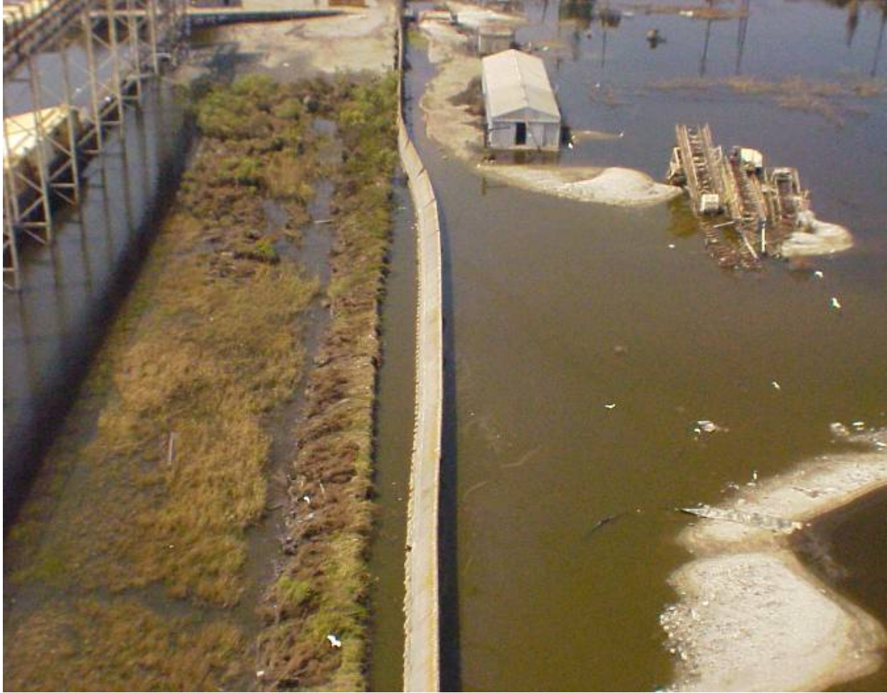
Figure 13-34. Bulk Loading Facility I-Wall Breach (2000' near Elaine St. at GIWW, near Sta 271+55 B/L, Citrus Back Levee, north bank GIWW). Scour depths were 6 to 10 ft on both floodside and protected side of the I-wall. Pre-existing wall elevation was approximately 15 ft (MSL), and levee elevation was approximately 9 ft (MSL), for an exposed wall height of approximately 6 ft. Storm surge ranged from elevation 15 to 17 ft
