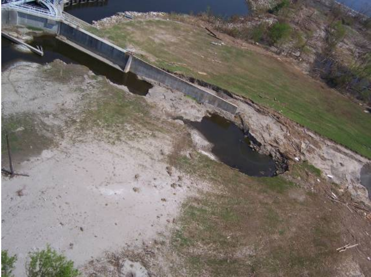
Figure 14-141. Severe Scour on East Side of Structure
