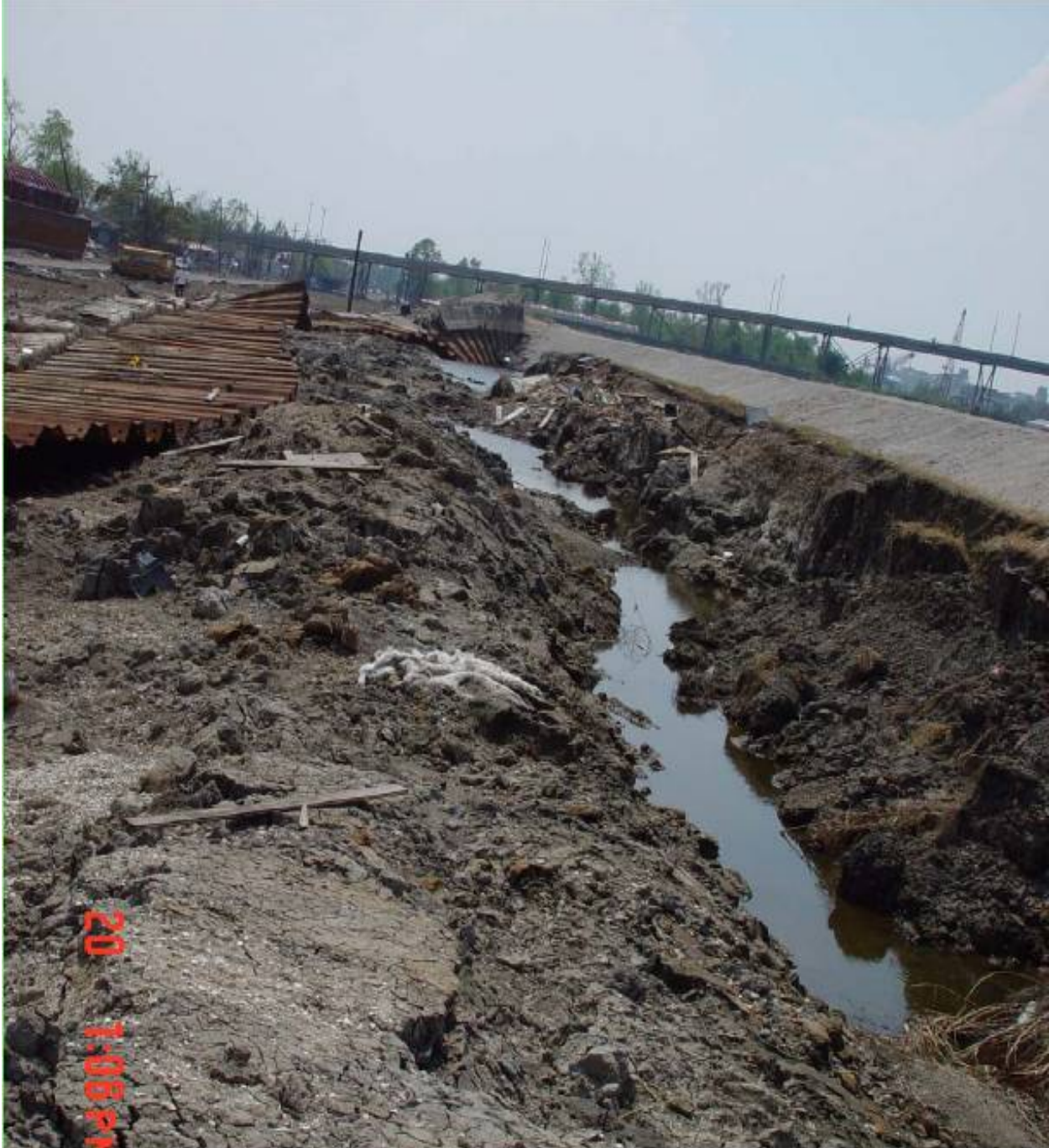
Figure 11-5. Scour and Erosion Leading to the Failure of the I-Wall on the IHNC Adjacent the South Breach (9th Ward)
