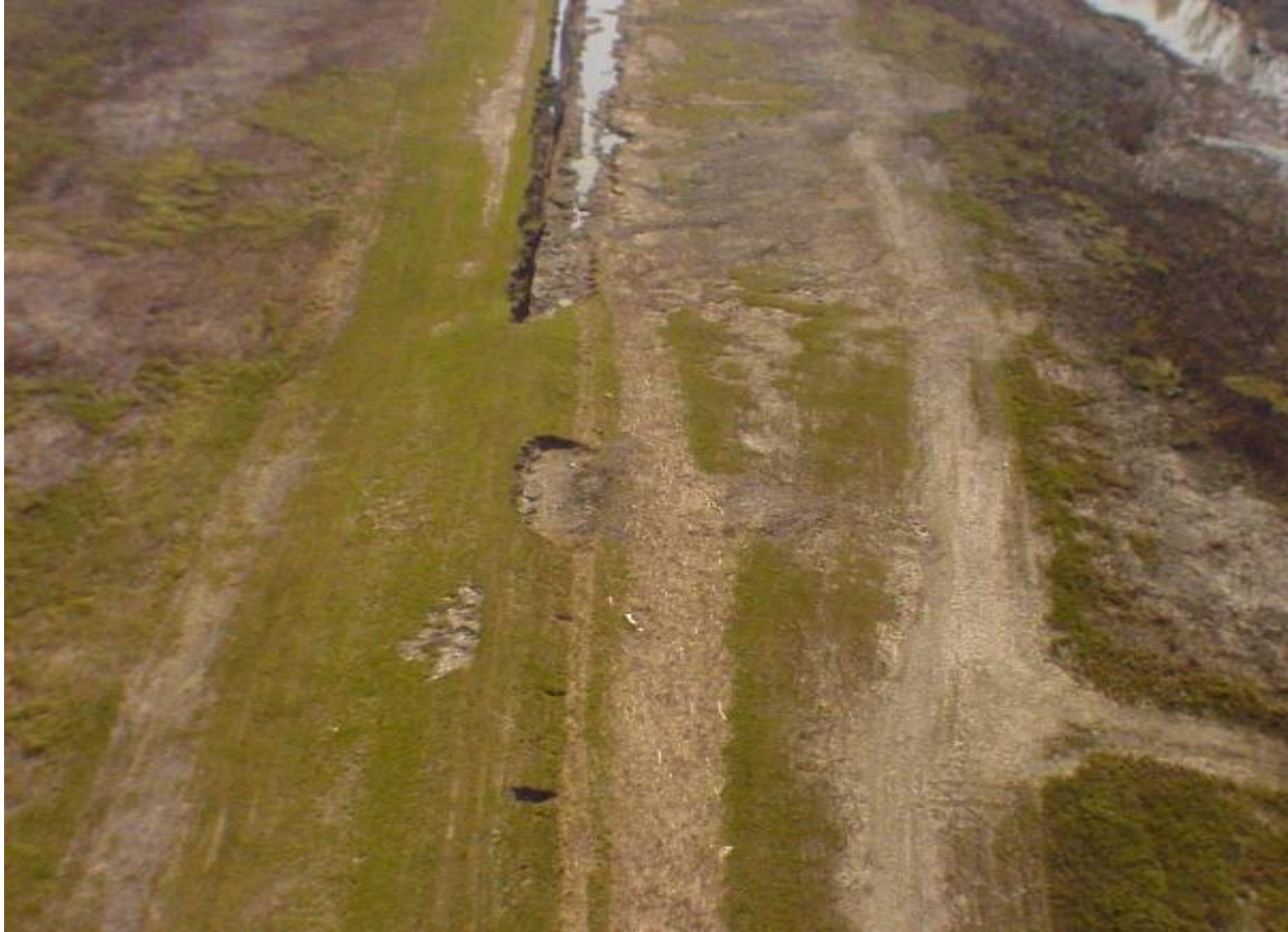
Figure 13-56. Crown Scour Along Approximate B/L Sta 1203+00 to Sta 1230+00, St. Bernard Levee Between MRGO and Miss. River. Crown was Approximate Elevation 15 ft
