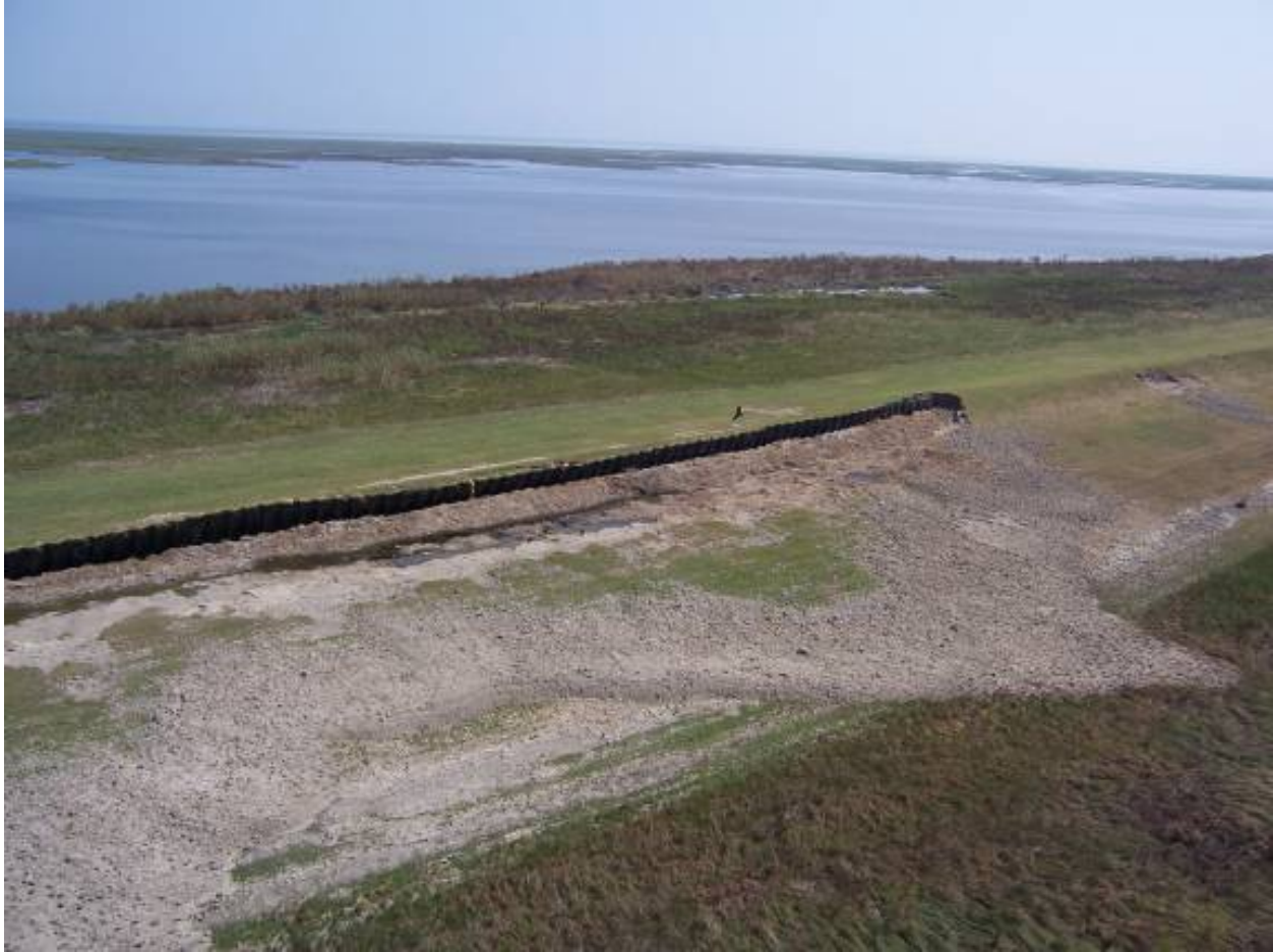
Figure 13-76. End of Sheetpile Wall at B/L Sta 980+58, along the MRGO (St. Bernard Parish). Note that scour occurred along the sheetpile wall and minimally beyond the levee transition. Approximate sheetpile elevation was 17 ft and levee crown elevation was 13 ft. Beyond the transition, the levee crown elevation was approximately 17 ft. The approximate storm surge overtopping crest was 4 ft over the sheetpile and 1 ft over the transition levee
