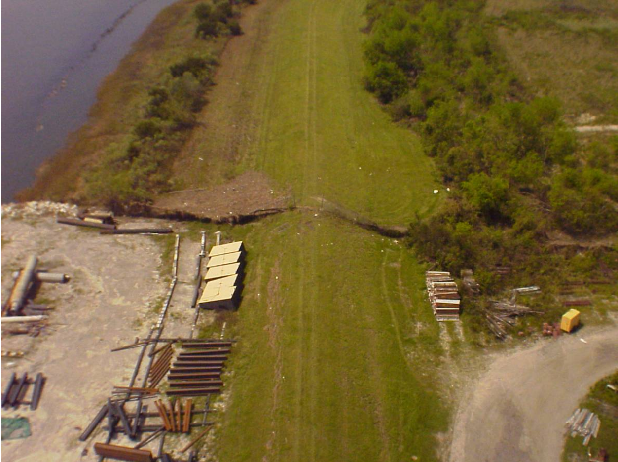
Figure 12-75. NOEX_V. Narrow Localized Breach at Pre-Existing Pipeline Crossing. Coords 30 deg 00 min 10.66 sec N, 89 deg 57 min 49.31 sec W (Approximate Sta 349+00 B/L)
