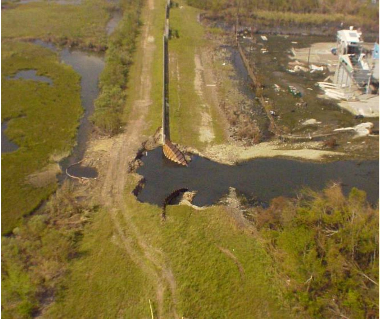
Figure 13-32. Air Products Sheetpile Breach
