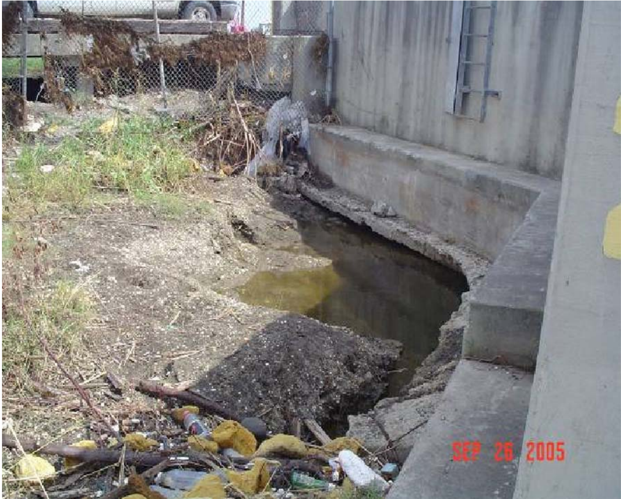
Figure 14-72. Scour at T-Wall Base of Gate W23
