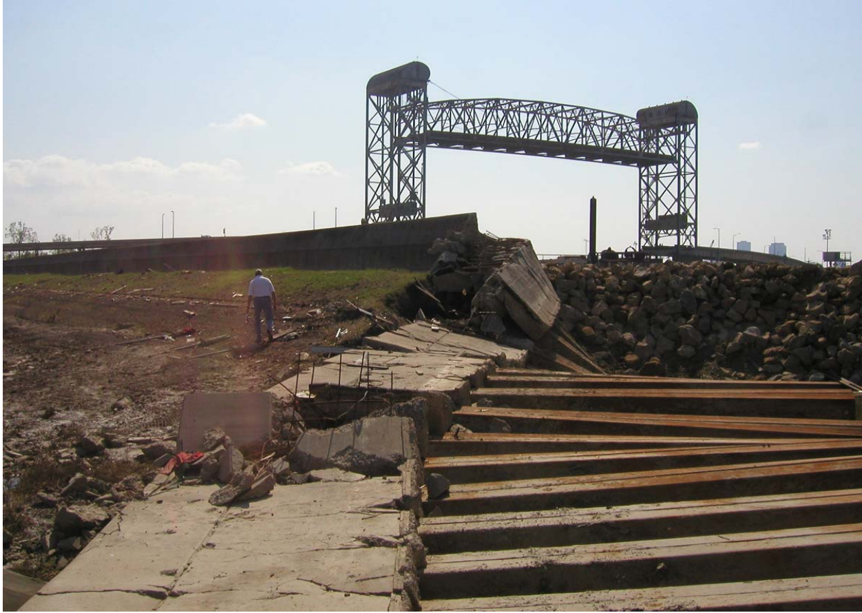
Figure 14-25. Transition From Failed Wall to Intact Wall, View Toward Claiborne Ave.
