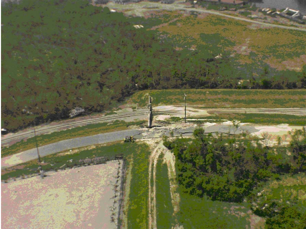
Figure 14-43. Scour at Railroad Gate Closure Structure E4 at Southernmost IHNC03 Project. 29 deg 59 min 48.76 sec N, 90 deg 01 min 11.6 sec W (Sta 176+75.9)
