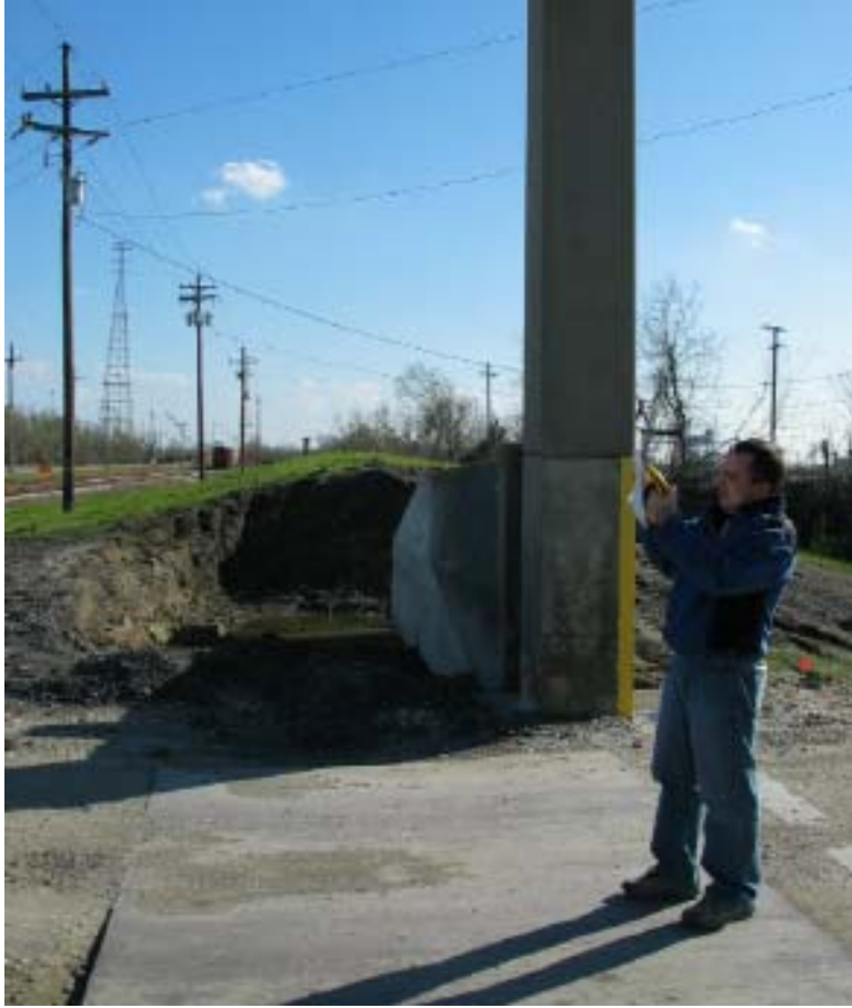
Figure 14-42. Gate E5 Looking South From Inside the Protected Area. Scour damage 7' (w) x 7' (d) around adjacent flood wall. Top of wall at gate is Elev. 13.2 +/-
