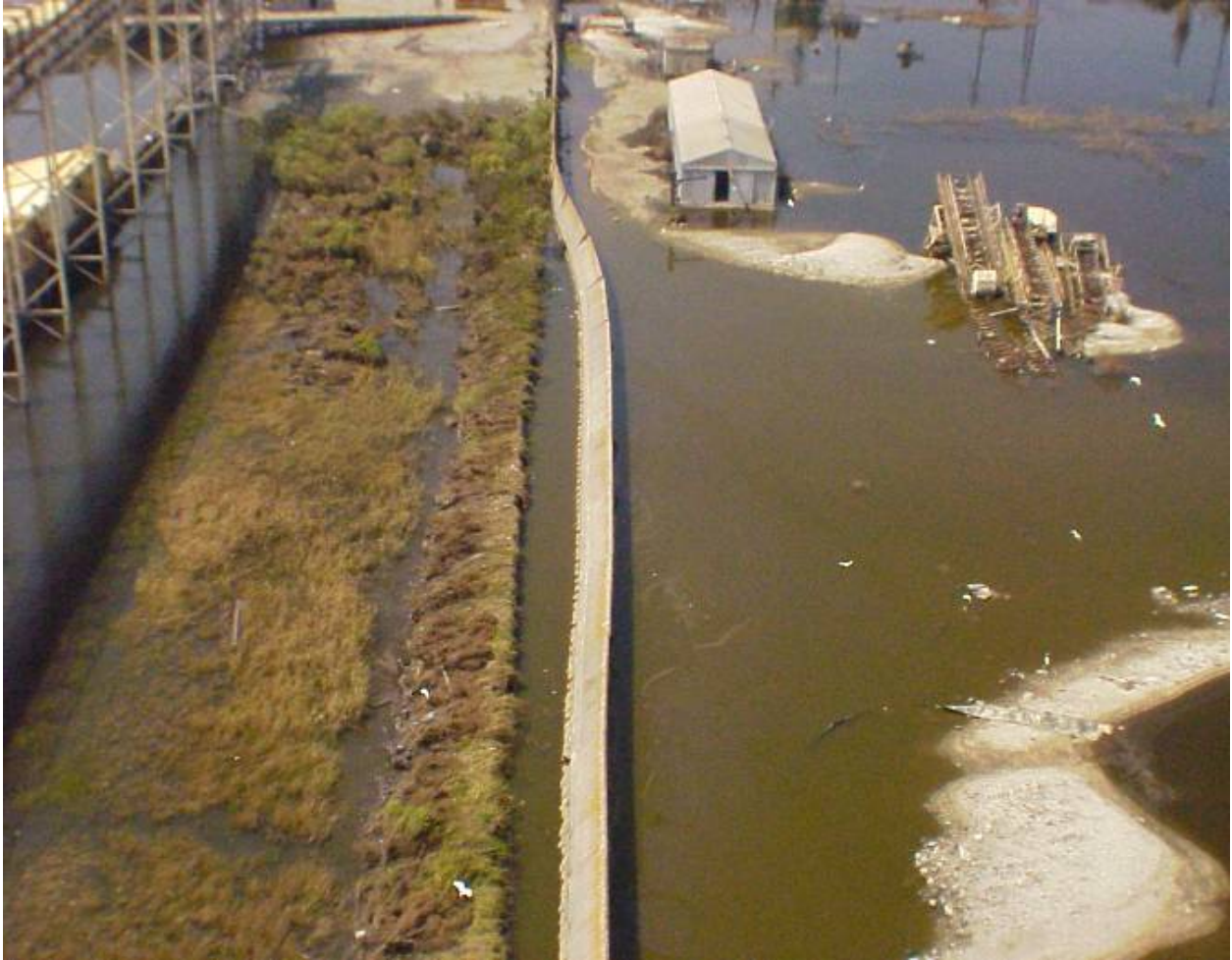
Figure 12-55. NOE4_B. Bulk Loading Terminal Facility I-Wall Failed by Rotation with Attendant Scour and Erosion (2000' near Elaine St. at GIWW), near Sta 271+55 B/L (Citrus Back Levee), Immediately Adjacent to the Tool Shed Metal Building
