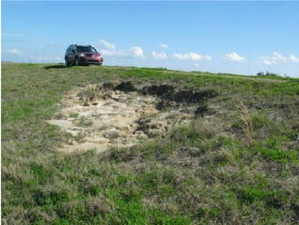
Figure 13-44. Closeup of Landside Slope Erosion at N 30deg 0 min 2.29sec W 89deg 58min 27.29sec
