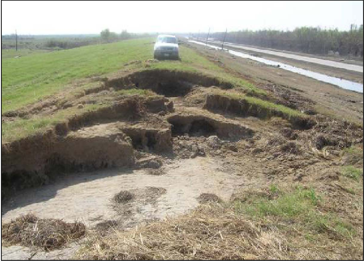
Figure 13-59. Plaquemines Parish East Bank Back Levee Erosion
