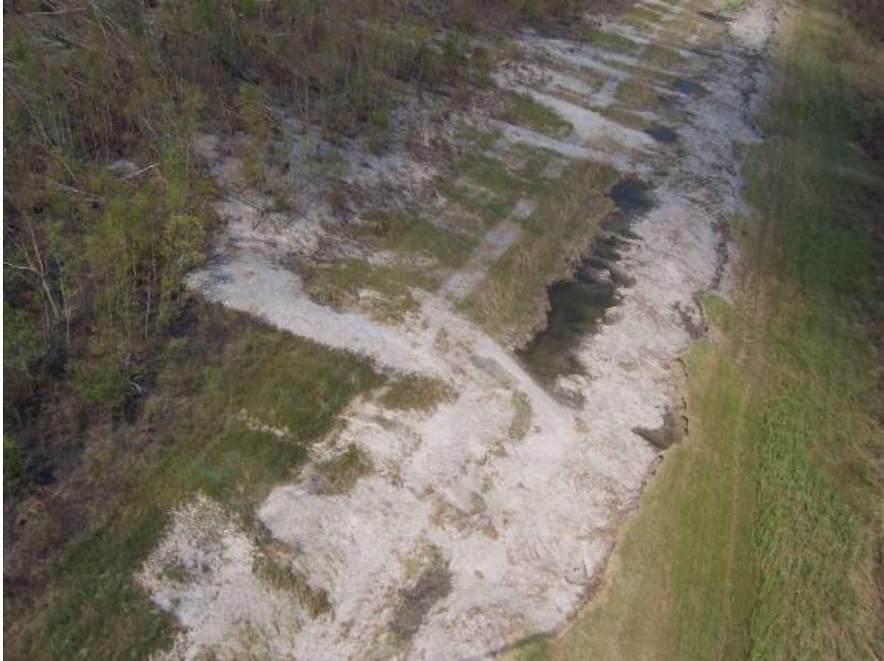
Figure 14-117. More Missing Levee
