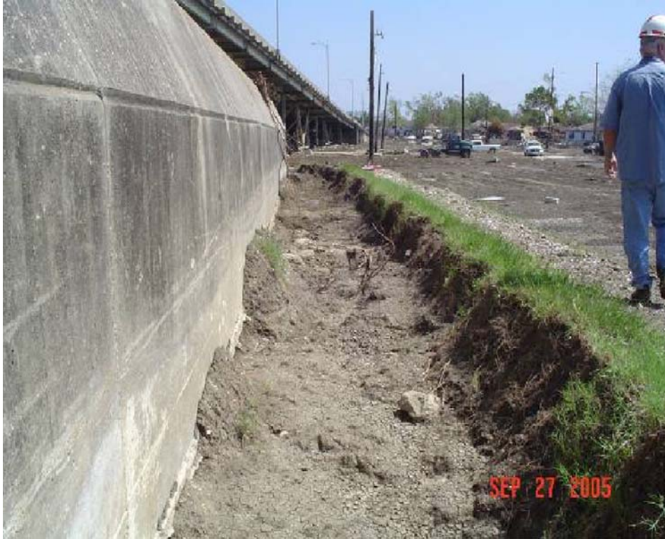
Figure 13-5. Scour Pattern "A" on East Side IHNC near N. Claiborne Ave. Bridge
