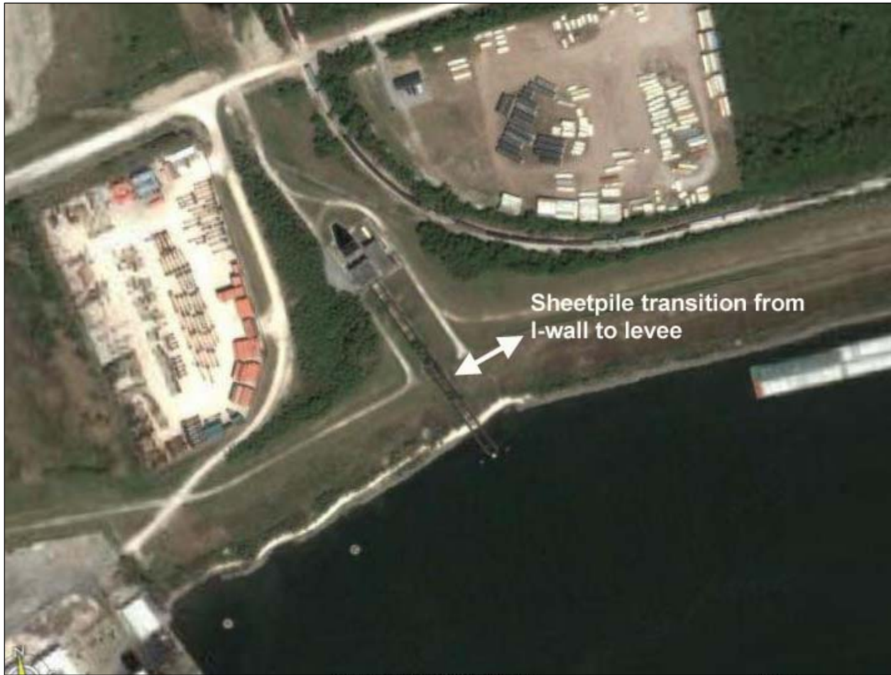
Figure 12-72. NOEX_S. Plate 2 of DM2-Gen Design Citrus Back Levee (Aug 1967) IHNC to NASA.pdf Shows Original Borings and Profile at Above Picture Location. Note that overtopping scour occurred at the intersection of the dirt road and levee crown as seen in Figure 12-NOEX-Q above
