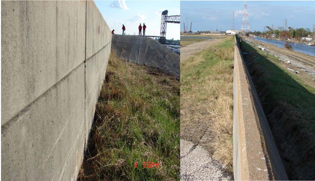
Figure 11-6. IHNC East Bank – South Breach – Wall Movement
