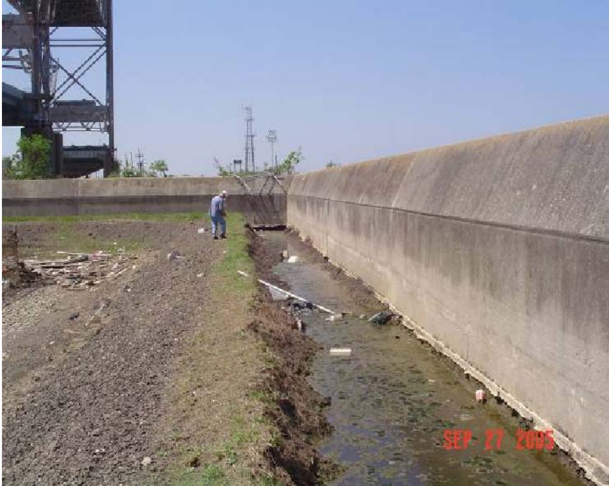
Figure 13-8. IHNC East, Approximate B/L Sta 7+00 (DM3 Chalmette Area Plan), North of the Claiborne Avenue Bridge. Depth of scour was to the bottom of the I-wall concrete cap. I-wall elevation was designed 15 ft above mean sea level (MSL), bottom of concrete was elevation 7 ft (MSL), and levee crown was elevation 9 ft (MSL). Actual wall height was reported to be 12.5 ft converted to local mean sea level (LMSL), and storm surge height was reported to be up to 15 ft. As an approximation of the overtopping water impact, a 2.5 ft crest of water cascaded from a 6-ft height onto the levee crown. Nearby soil boring 2U (Figure 13-9) indicates the upper 5 ft was fat clay (CH) with sand / silt lenses
