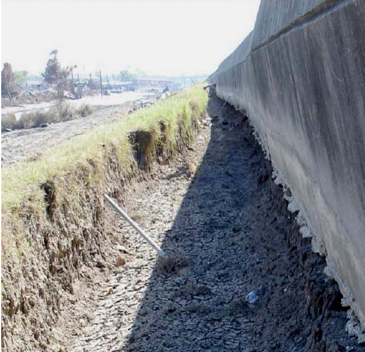
Figure 11-4. Scour and Erosion on the Protected Side of the IHNC Adjacent to the Ninth Ward in the Vicinity of the South Breach
