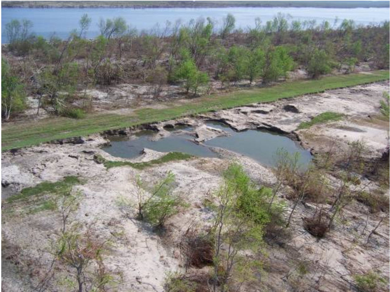
Figure 14-144. Major Scour on Levee Protected Side (Landside)
