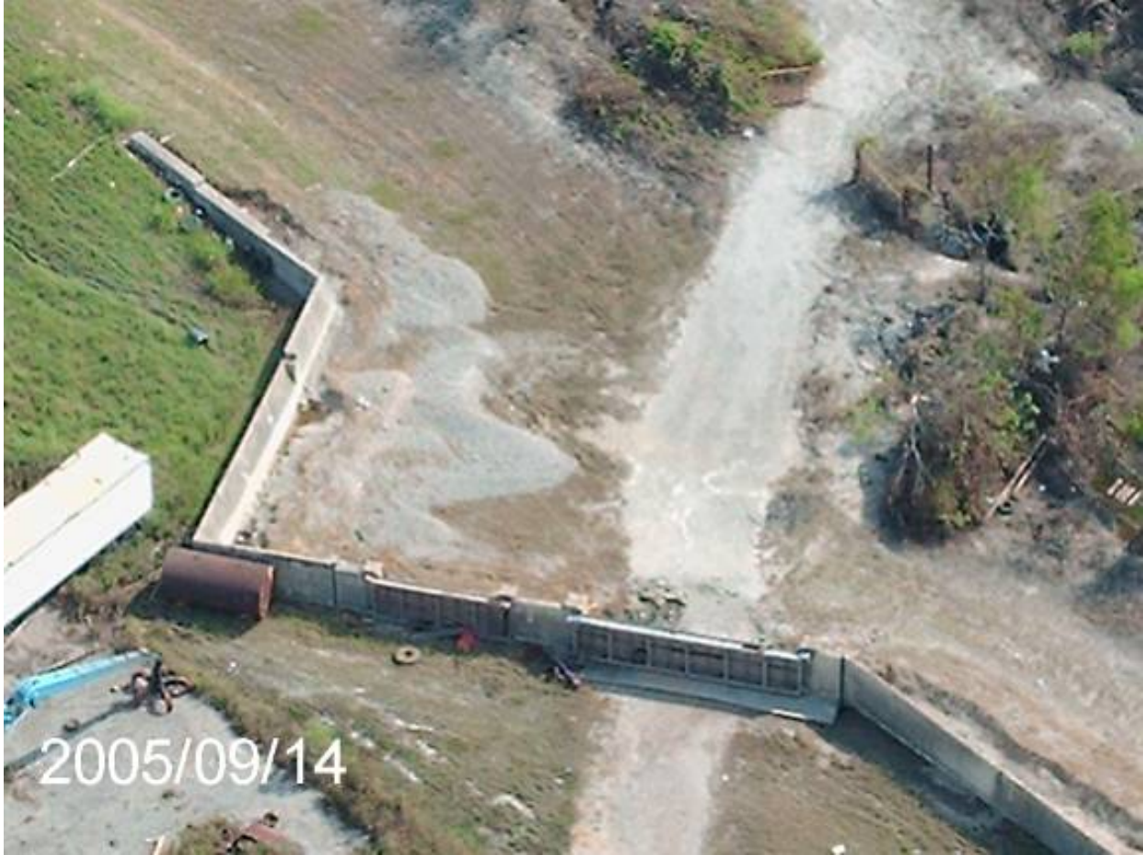
Figure 14-86. View of Scour Outside Gates S2 and S3. IHNC/GIWW and Southern Scrap sites are on the left side of photo
