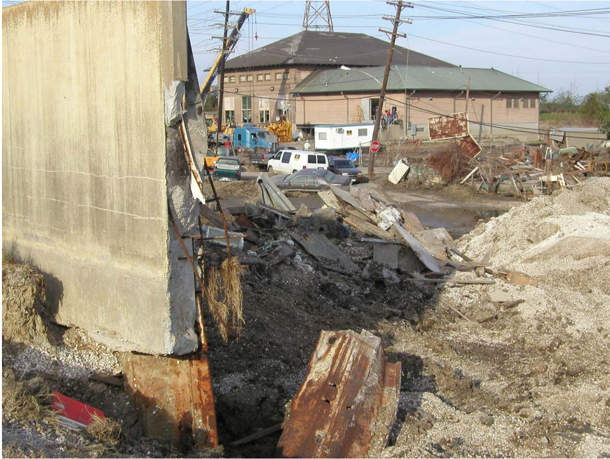
Figure 14-32. Northernmost I-Wall Failure Transition Between Florida Ave and Claiborne Ave., View Toward Pump Station on the Protected Side
