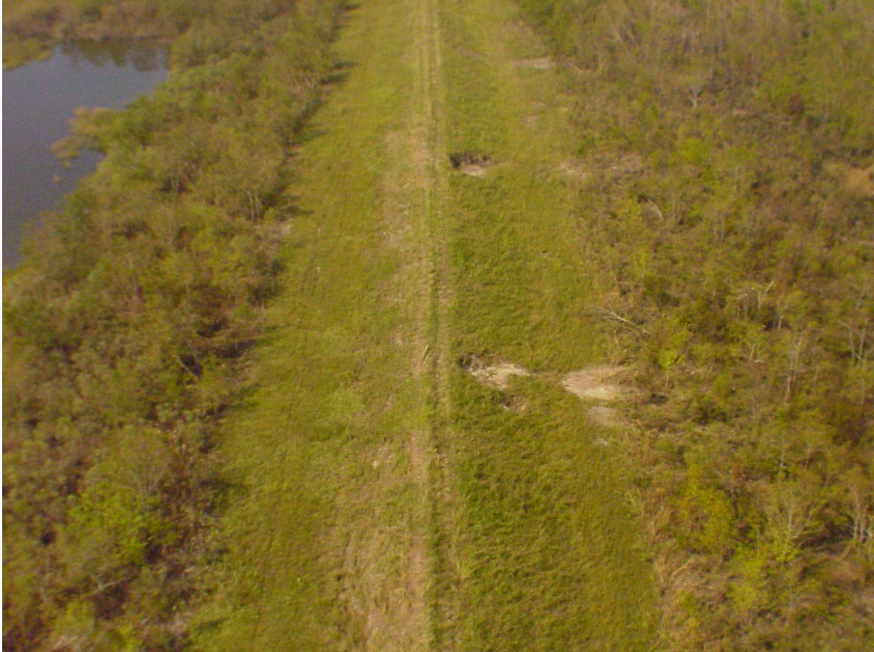
Figure 13-42. Backside Levee Erosion Pattern “B” on the Citrus Back Levee, N.O. East
