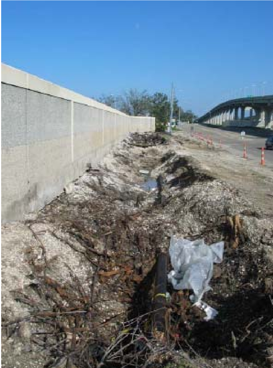
Figure 13-12. Scour Along Lakefront Airport Floodwall Measures 305' (L) x 14' (w) x 48" (d). Existing levee crown appears to be composed of sandy material, based on visual observation. Nearby soil boring 1-C (5/29/1969) at Sta. 8+85, 57 ft right of B/L shows sand, silt, and lean clay lenses to 9-ft depth. Soil boring 4-A (11/3/1970) at Sta 18+00, 200 ft landside of B/L also shows sand, silt, and lean clay lenses to 9-ft depth
