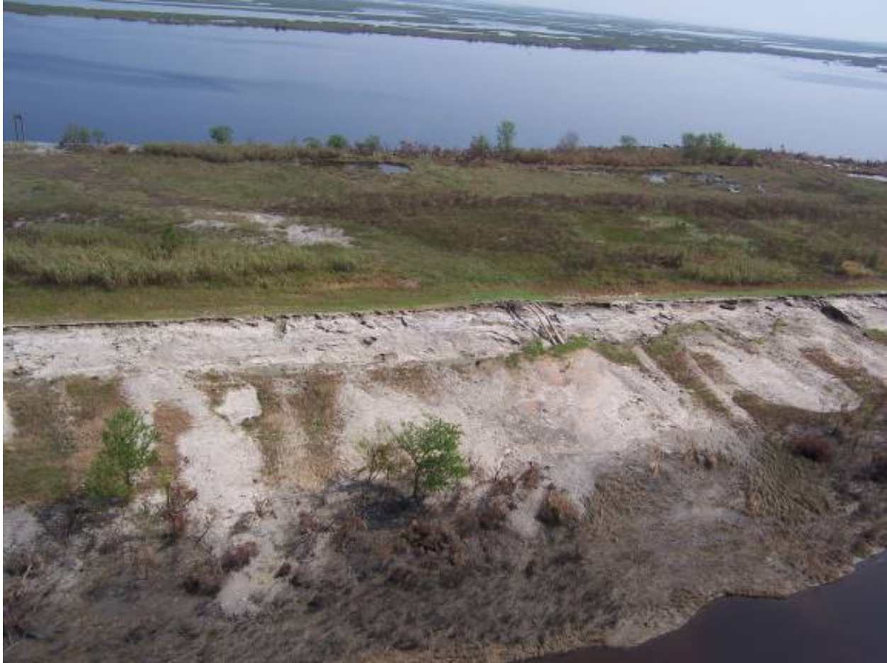
Figure 14-116. Levee Completely Eroded Away
