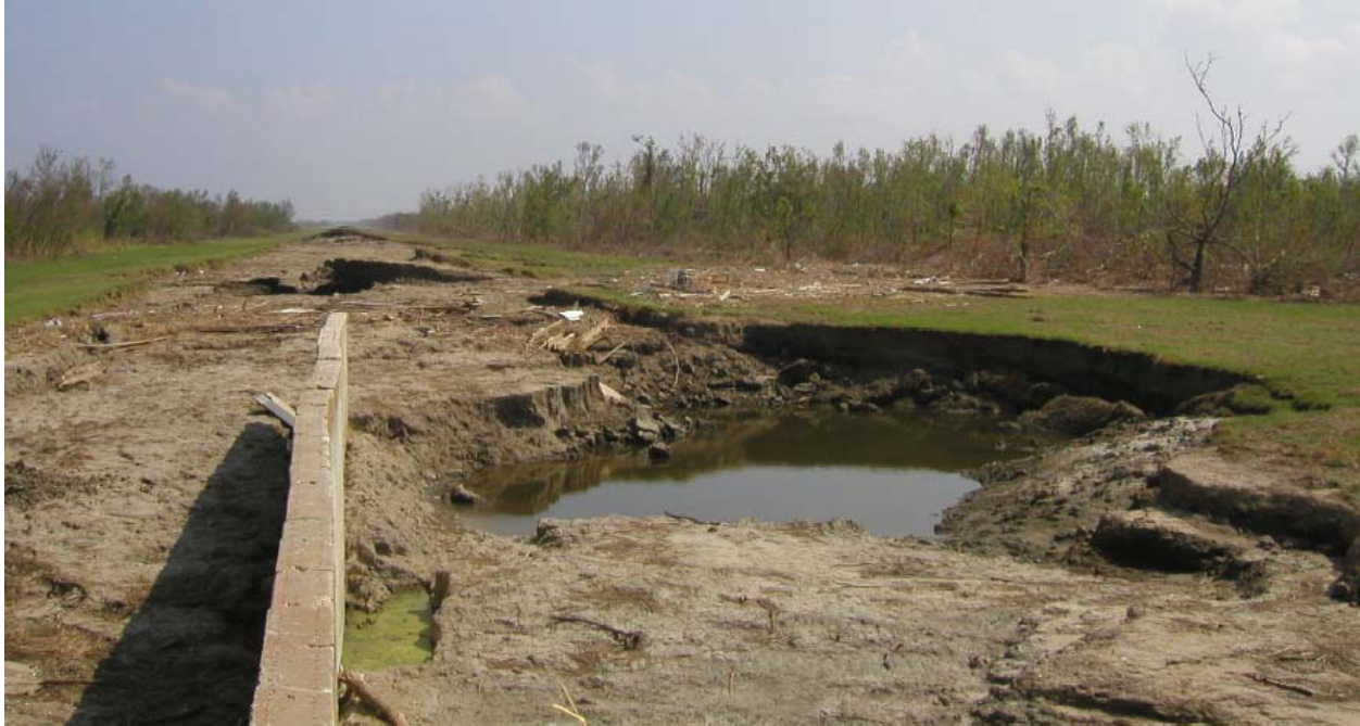
Figure 14-142. Closeup of East View, End of Concrete Wall, Showing Major Scour Holes and Complete Erosion of Levee
