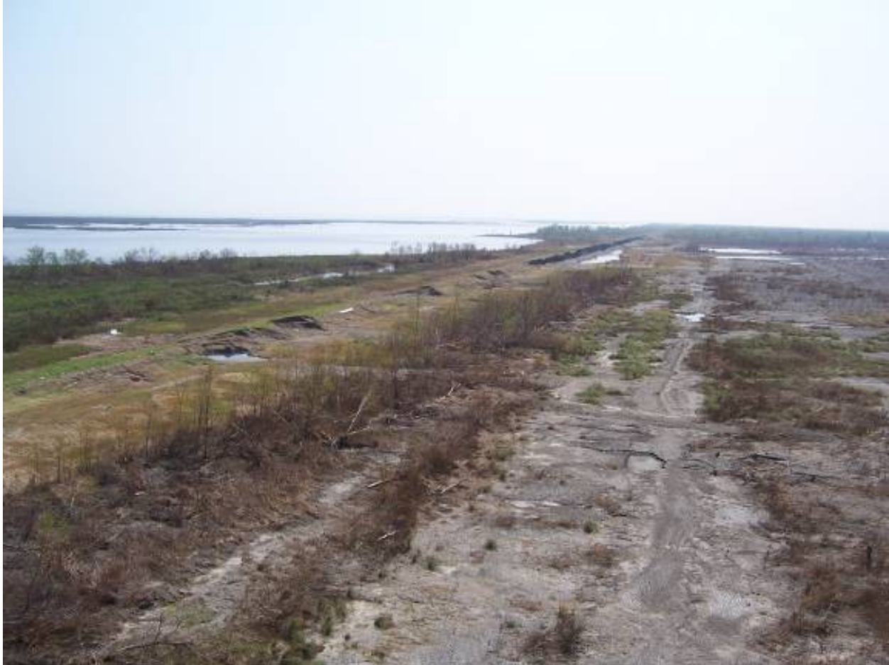
Figure 13-55. Levee with Eroded Crown Between Bienvenue and Dupre Bayous, View South From Approximate B/L Sta 570+00. MRGO is to the Left of Photo
