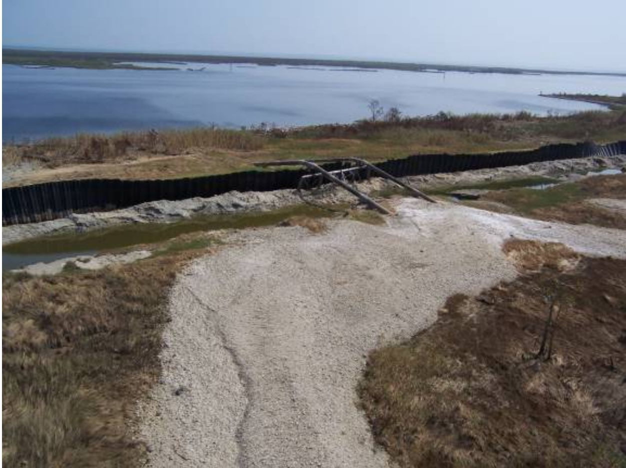
Figure 13-23. Pattern "A" Scour on the Backside of Exposed Sheetpile Wall Along the MRGO South Bank in St. Bernard Parish
