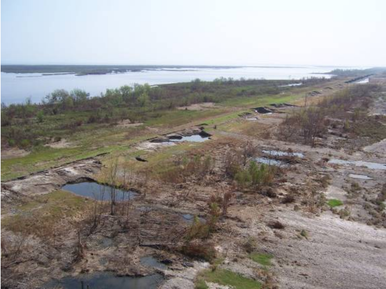
Figure 14-118. Partial Levee Eroded
