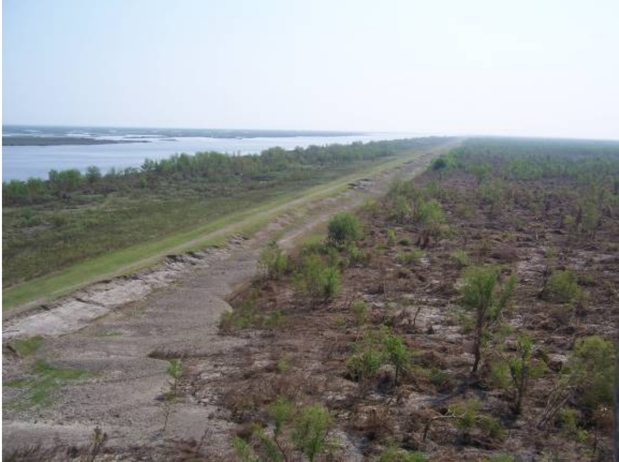
Figure 13-68. 2,500 ft. of levee along MRGO from Bayou Dupre to Sta 1007+91 that lost approximately 8' of elevation
