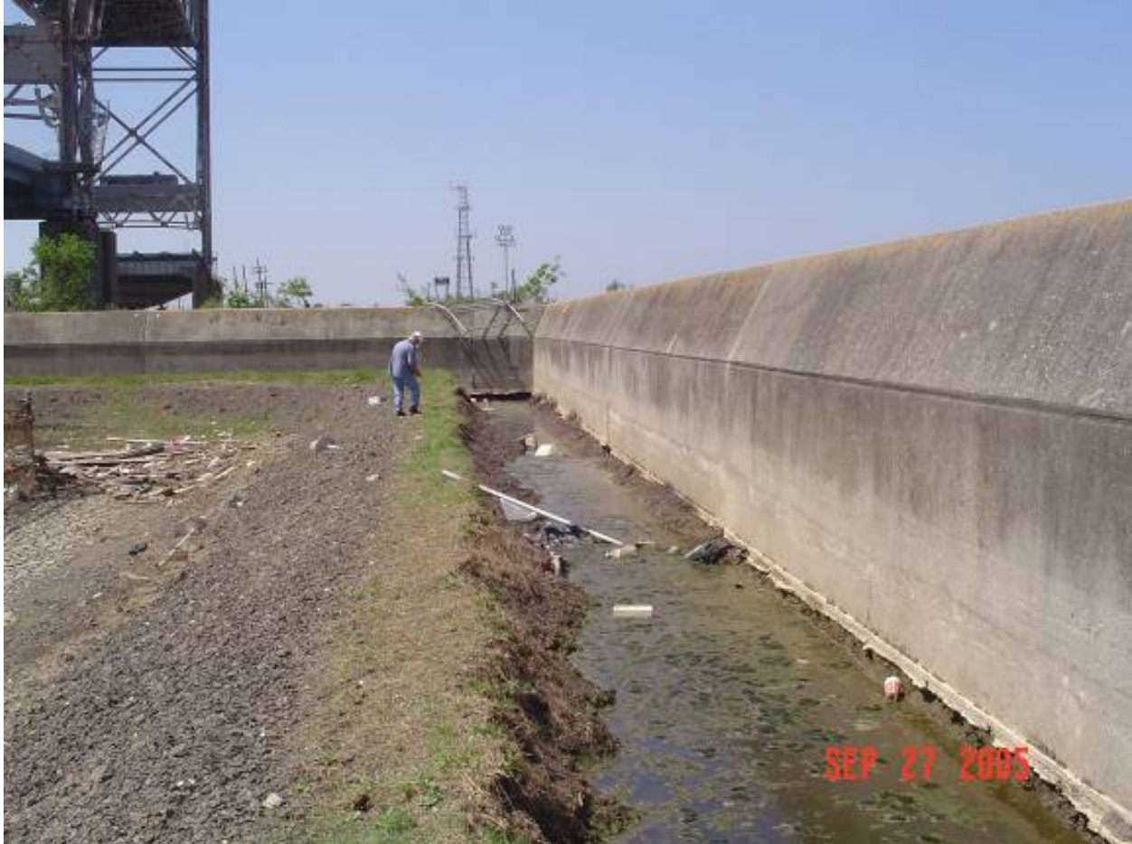
Figure 14-47. Approximate B/L Sta 7+00, View Toward Claiborne Ave. Bridge. Depth of scour was to the bottom of the I-wall concrete cap. Nearby soil boring 2U indicates the upper 5 ft was fat clay (CH) with sand / silt lenses
