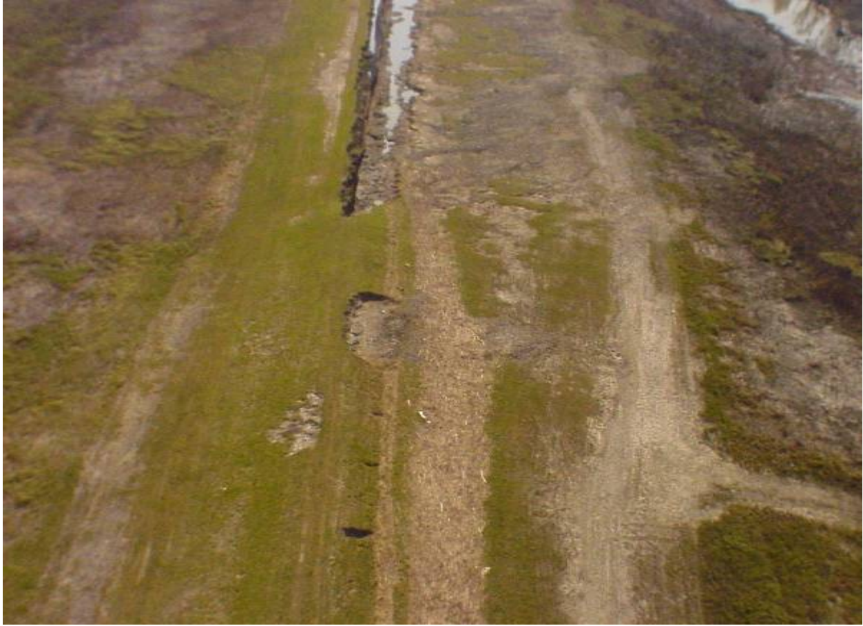
Figure 14-155. Crown Scour Along Approximate B/L Sta 1203+00 to Sta 1230+00
