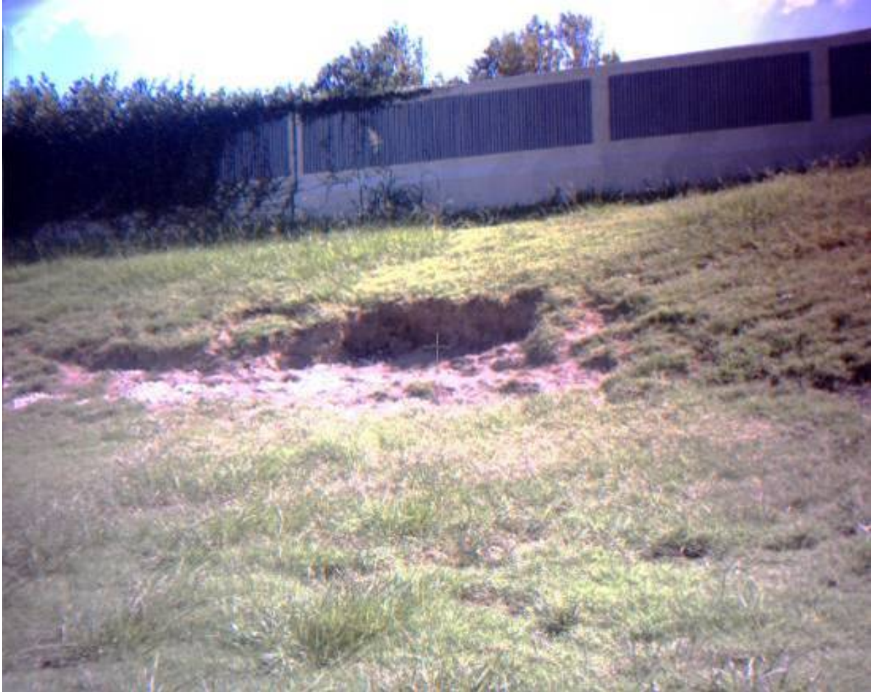
Figure 13-52. New Orleans East Bank Lake Pontchartrain Floodwall Scour, 20ft long x 10ft wide x 2ft deep. GPS coords N90 deg 05min 17.3 sec, W30deg 01 min 39.3 sec
