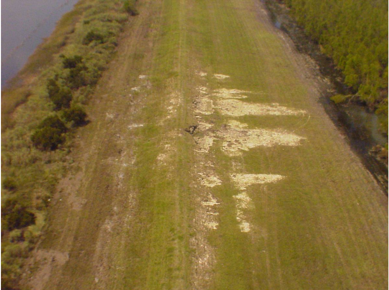
Figure 12-76. NOEX_W. 600' Reach of Levee with Landside Scouring
