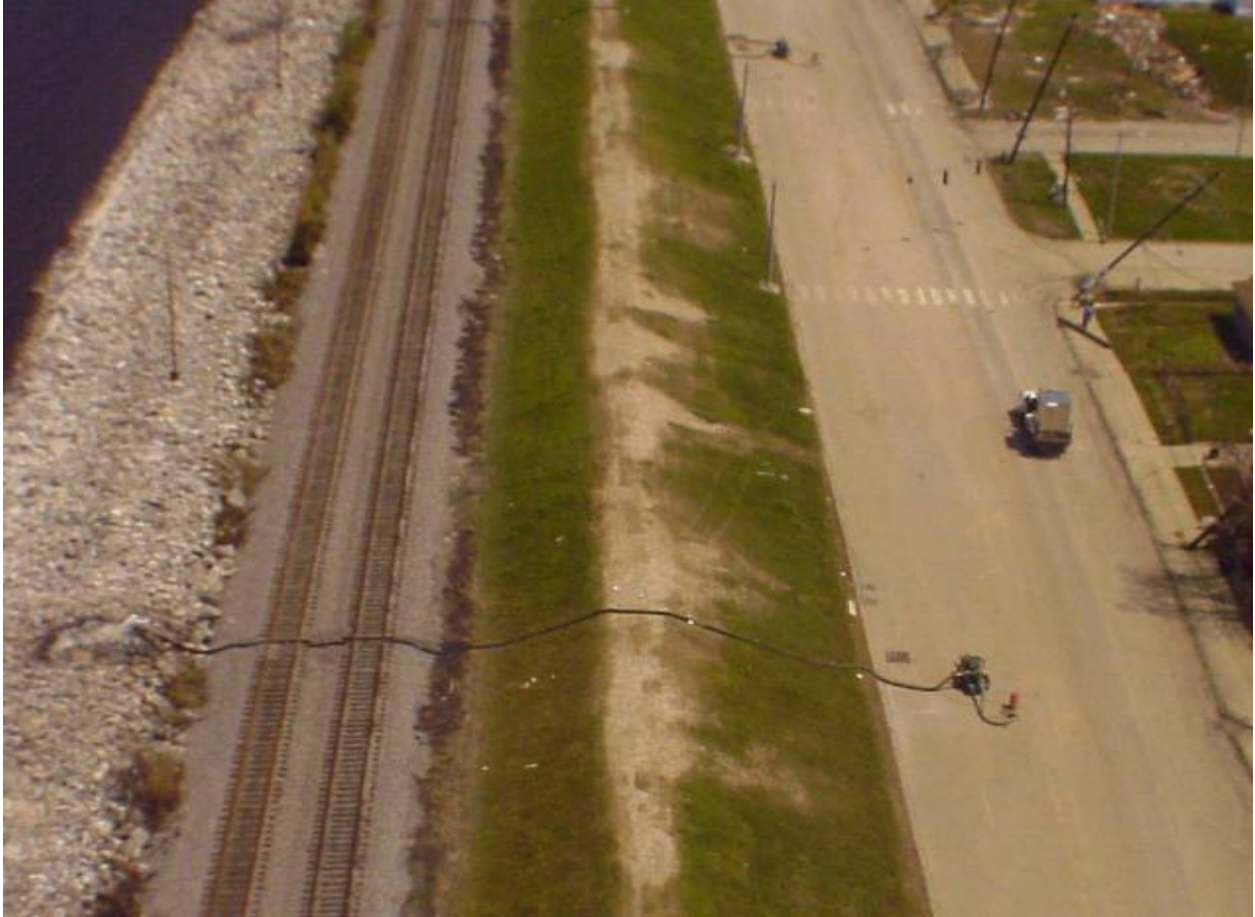
Figure 12-10. NOE7_B Typical Crown and Landside Scouring
