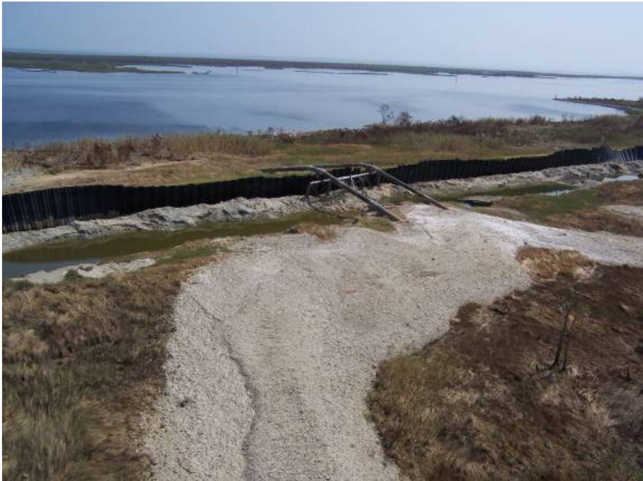
Figure 14-121. Damaged Sheetpile Section (Utility Crossing), With Scour on the Protected Side. B/L Sta 590+70 is centerline of the two pipelines
