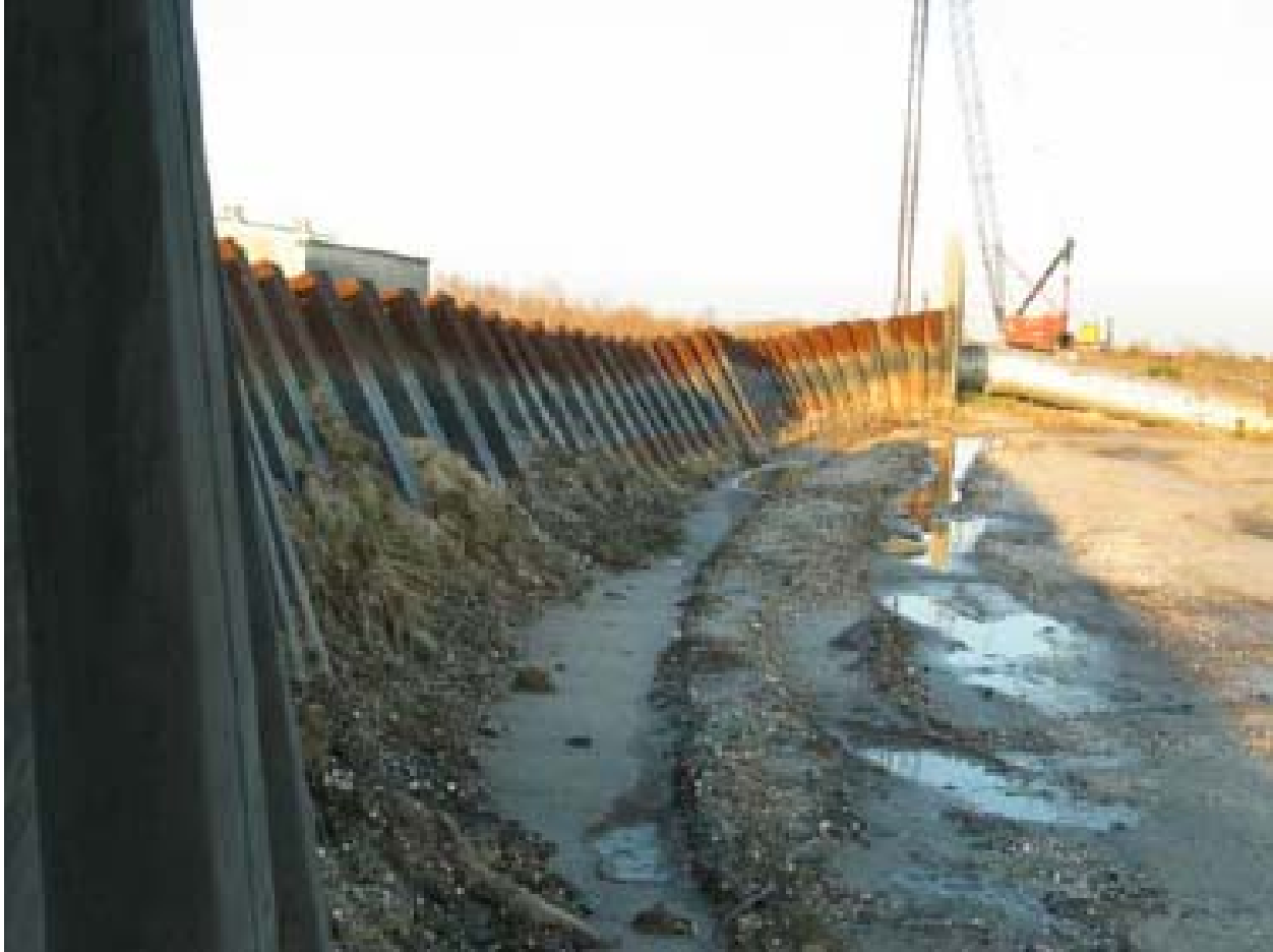
Figure 12-23. NOE2_C Closeup of Sheet Pile Damaged by Scour/Rotation/Sliding Failure
