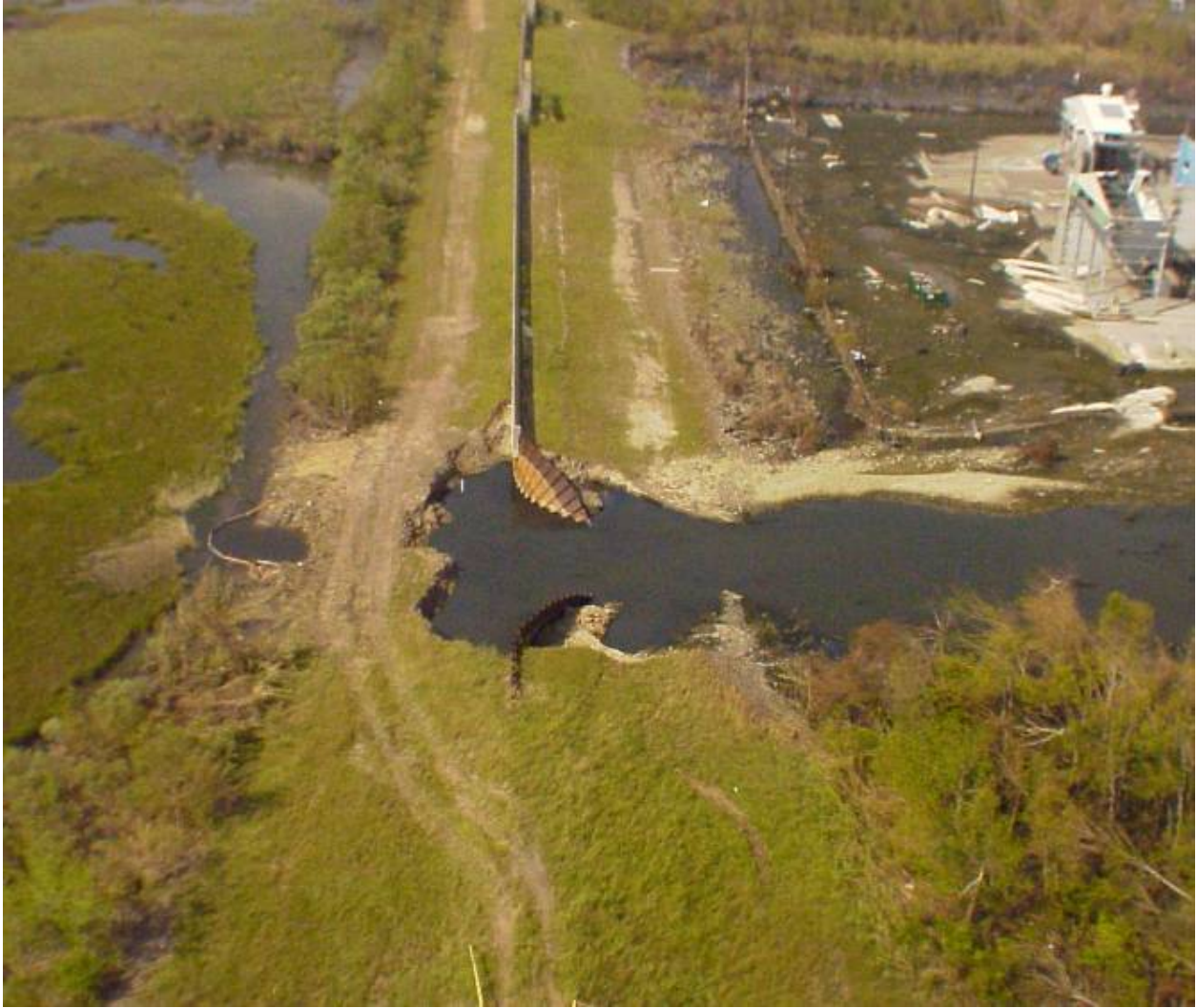
Figure 12-44. NOE3_D Sheetpile Wall Failure (near Sta 772+00 B/L New Orleans East Back Levee) (Coordinates 30 deg 01 min 04.30 sec N, 89 deg 53 min 49.36 sec W)
