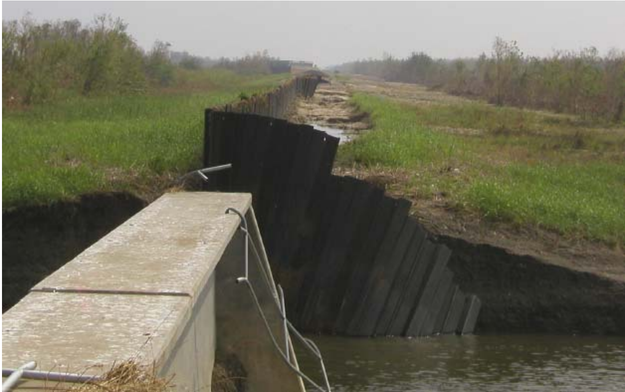
Figure 13-20. View Looking Southeast from the Bayou Bienvenue Control Structure Showing Backside Scour Beyond the Structure
