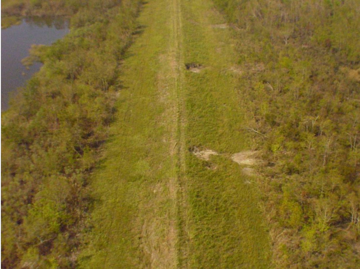
Figure 12-40. NOE1_G Localized Scour Typical of Several Locations
