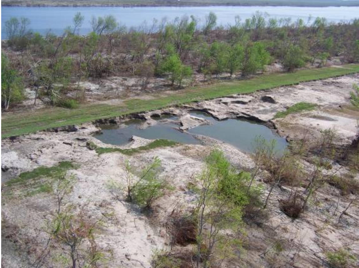
Figure 13-66. 8,000 ft. section of the levee immediately southeast of Bayou Dupre (St. Bernard Parish) that was severely damaged and not only lost approximately 12 feet of levee height but also part of the original levee foundation
