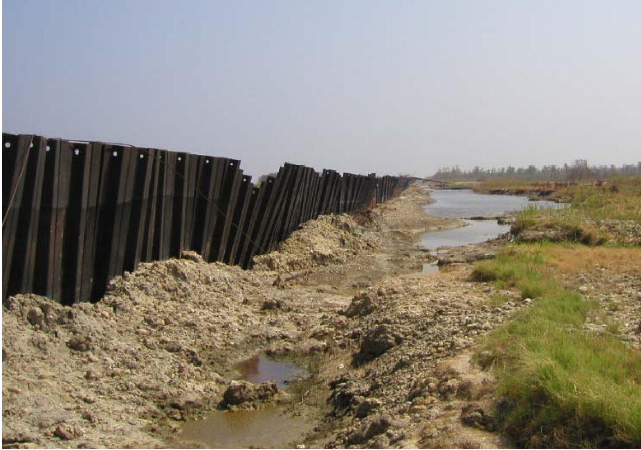
Figure 13-28. Sheetpile Between Bienvenue and Dupre Control Structures. Note the sheetpile elevation differences
