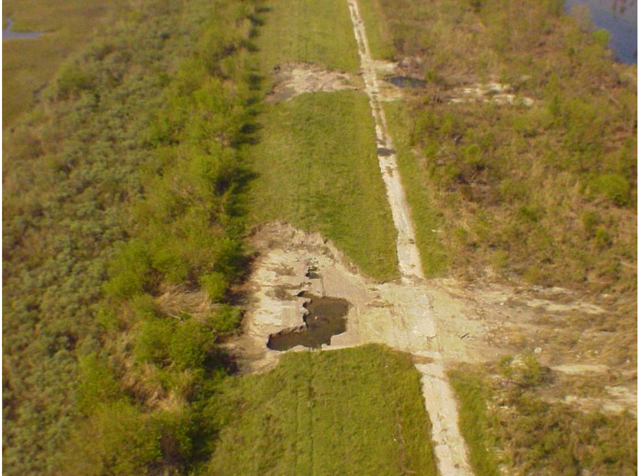
Figure 12-38. NOE1_E Partial Breach East of Pump Station 15
