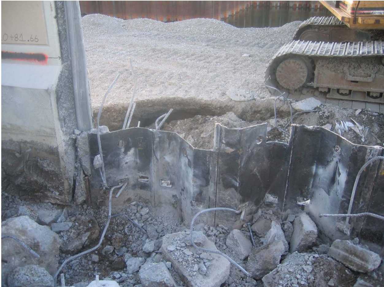
Figure 15-26. Lower Top Elevation of Sheet Piling at Expansion Joint
