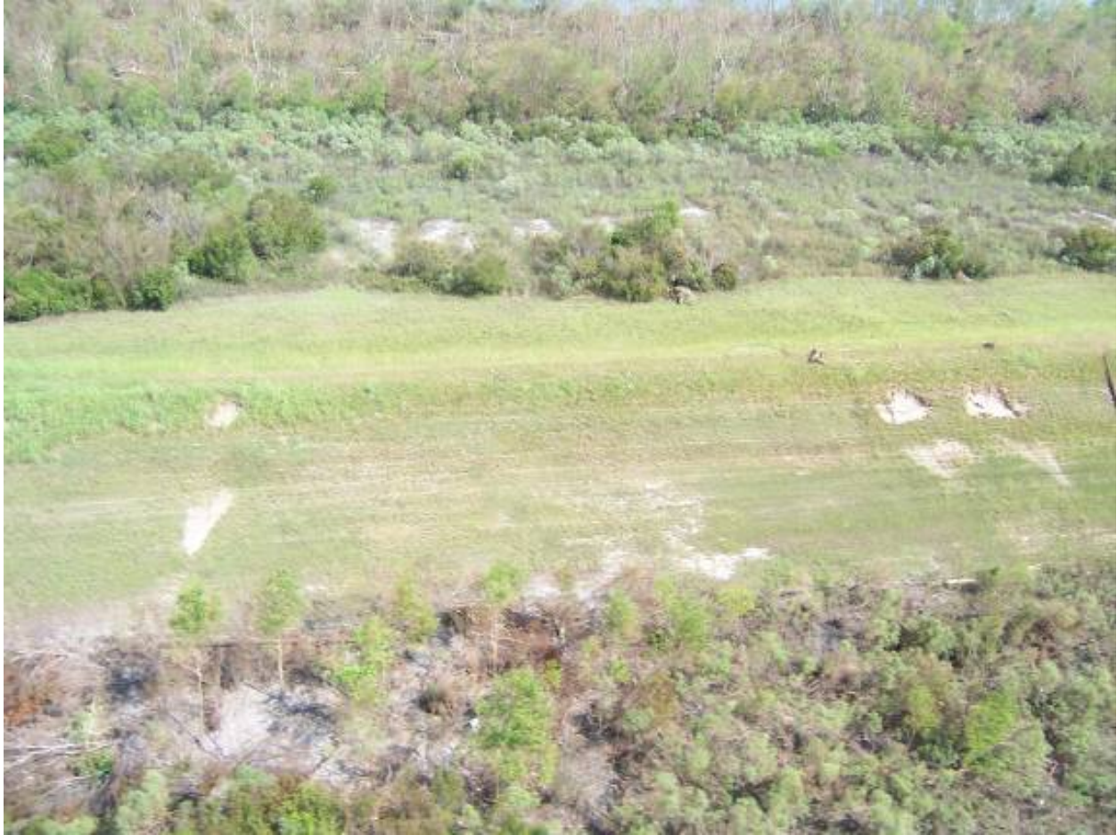
Figure 14-91. Localized Scour on the Levee South of the GIWW, Between IHNC and Paris Rd.
