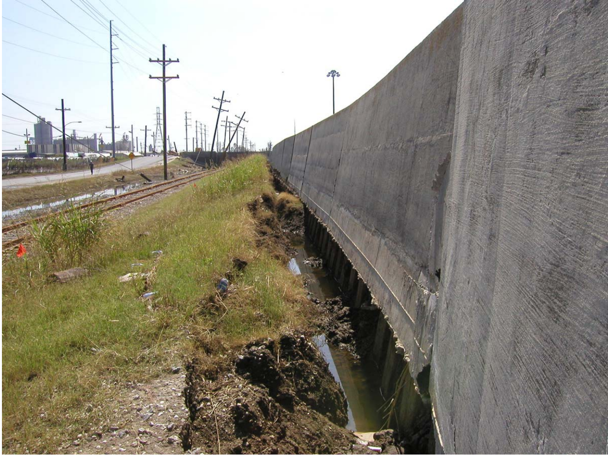
Figure 13-18. IHNC West Side, View South from Benefit St. Gate Toward France Rd Ramp. Approximate W/L Sta 5+56 (B/L Sta 205+44). Top of I-wall elevation 15 ft, levee crown 9 ft, bottom of concrete 7 ft, bottom of pre-existing Z-27 sheet pile (installed by the Orleans Levee Board) at -10ft (MSL). From drawing file H-2-24111, plate IV-15. Nearest soil boring (Figure 13-19) is 30W at B/L Sta 203+00. The I-wall rotated and floodside levee deformation occurred, probably as a result of sheetpile rotation opening up a floodside tension crack. This picture represents scour pattern "C" which is a pre-breaching failure mode
