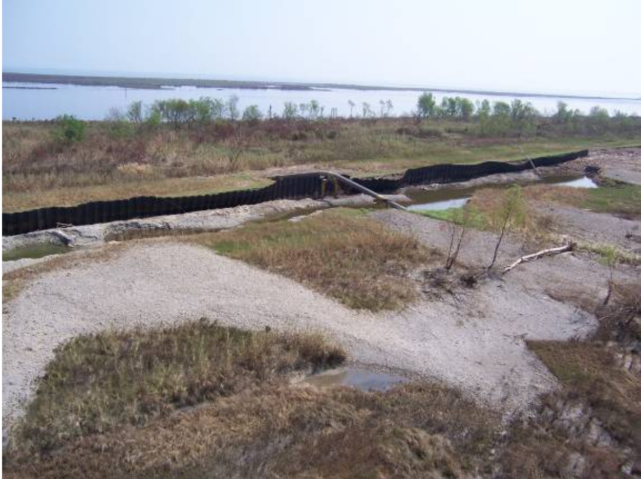
Figure 13-29. Sheetpile Reach Along the MRGO Southeast of Bayou Bienvenue at Approximate B/L Sta 600+00. Top of sheetpile was elevation 17 ft (MSL) and levee crown elevation was approximately 12 ft (MSL), for an exposed sheetpile height of approximately 5 ft. Storm surge on the MRGO was approximately 18 ft, resulting in approximate overtopping velocity of 20 ft per second with approximate 250 lbs/ft impact force. The end of the sheetpile section with transition to the severely eroded levee is approximate B/L Sta 604+15
