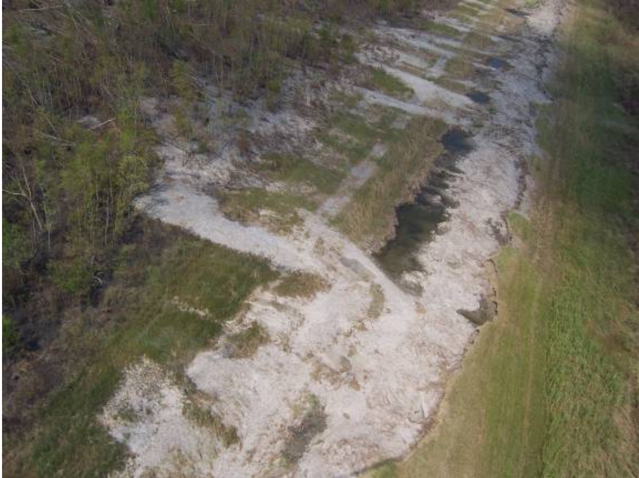
Figure 13-64. 2,300 ft. of Levee Between Bayou Bienvenue (Sta 383+00) and Bayou Dupre (Sta 704+00) That Only Lost 50% of Height
