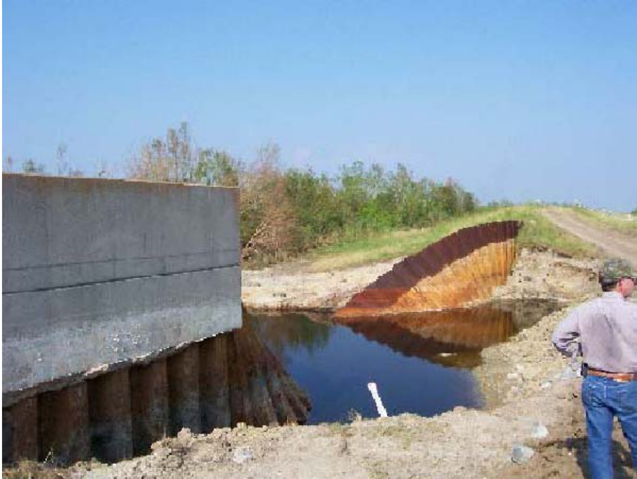
Figure 12-47. NOE3_G. West of Failure Looking East. Drawings from NOE3 Contract Solicitation Show Scour Depth And Outline
