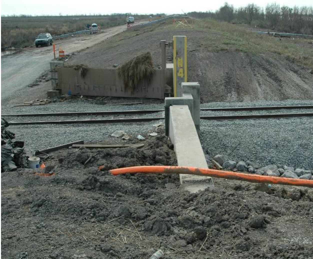
Figure 12-20. NOE5_C. Filled-In Scour Holes
