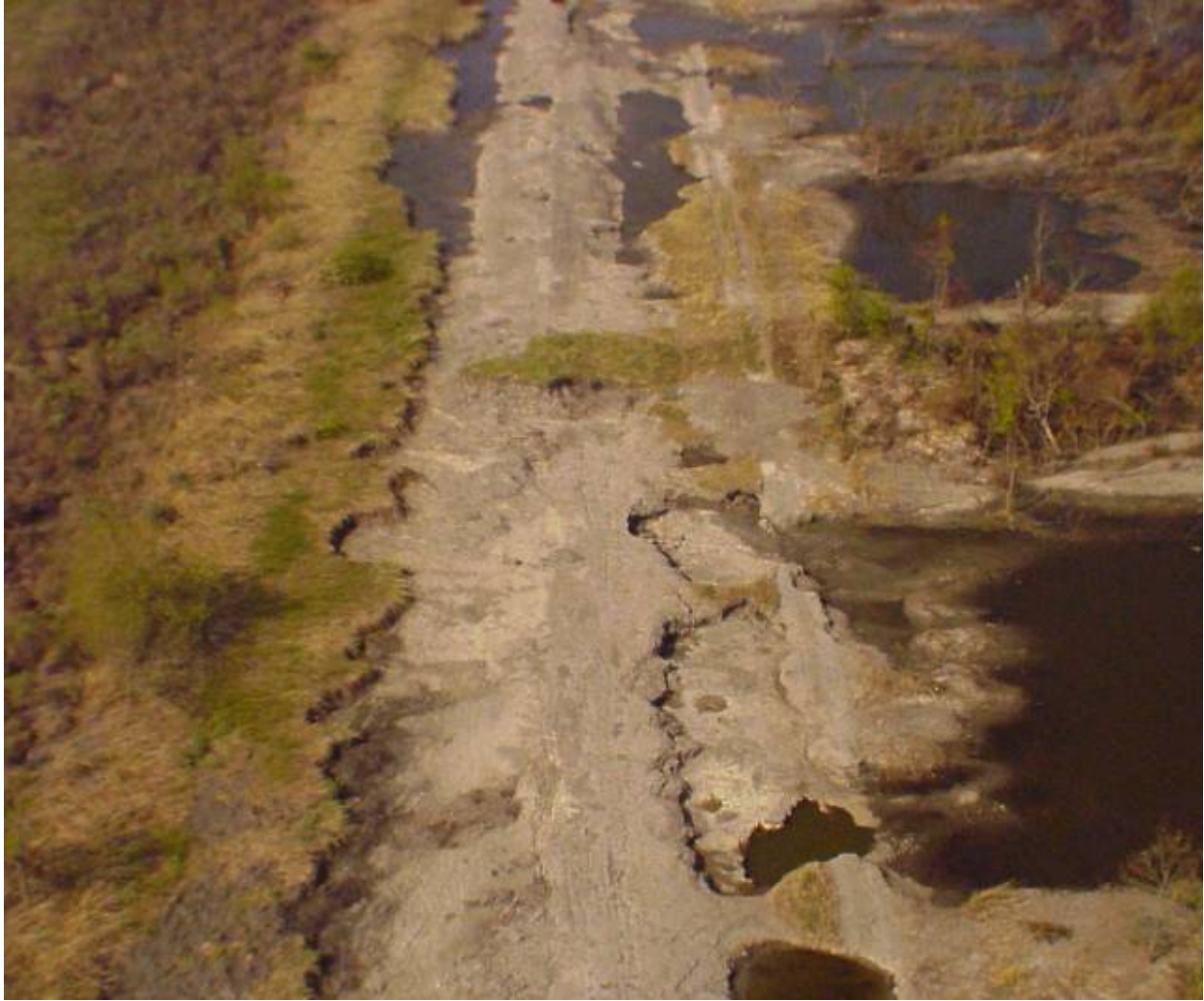
Figure 12-36. NOE1_C Complete Breach East of Pump Station 15
