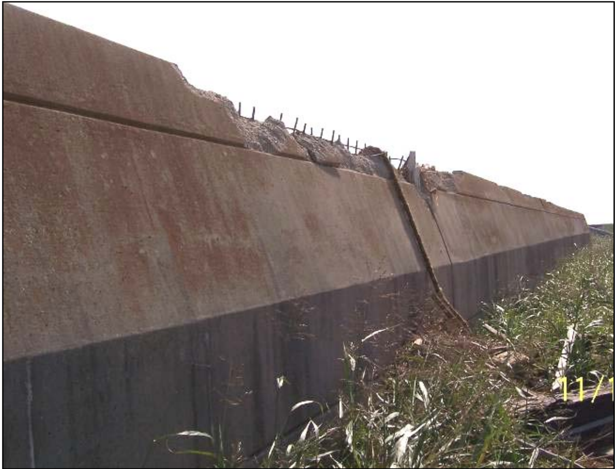
Figure 12-53. NOE9_C. I-Wall Damage Likely Due to Impact
