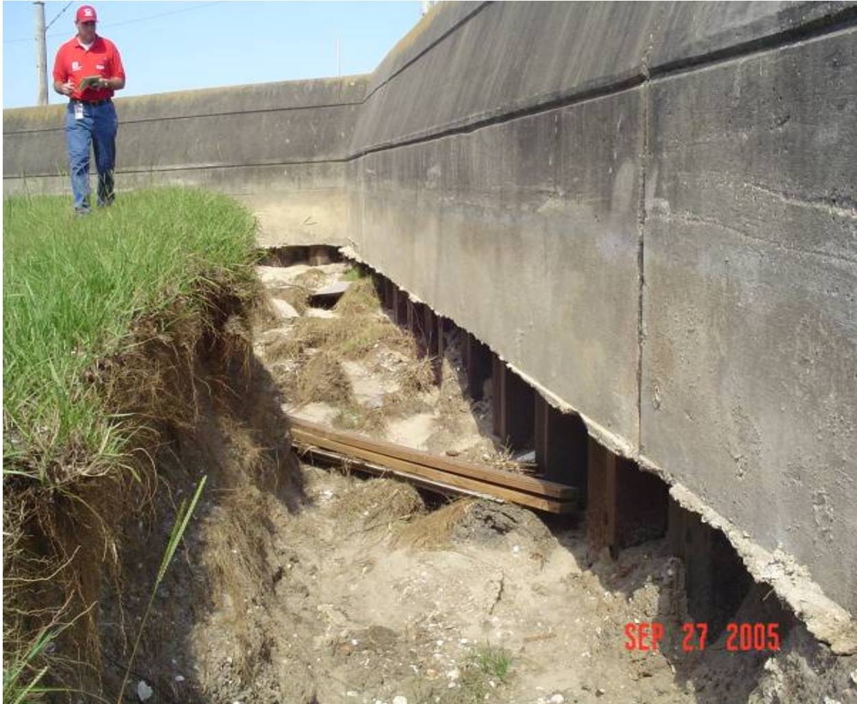
Figure 14-37. Approximate B/L Sta 101+00. Top of I-wall is elev 14.75, bottom of concrete is elev 7, and levee crown is elev 9. Nearest B/L boring is Sta 96+00 (No. 9EU), 500 feet distant
