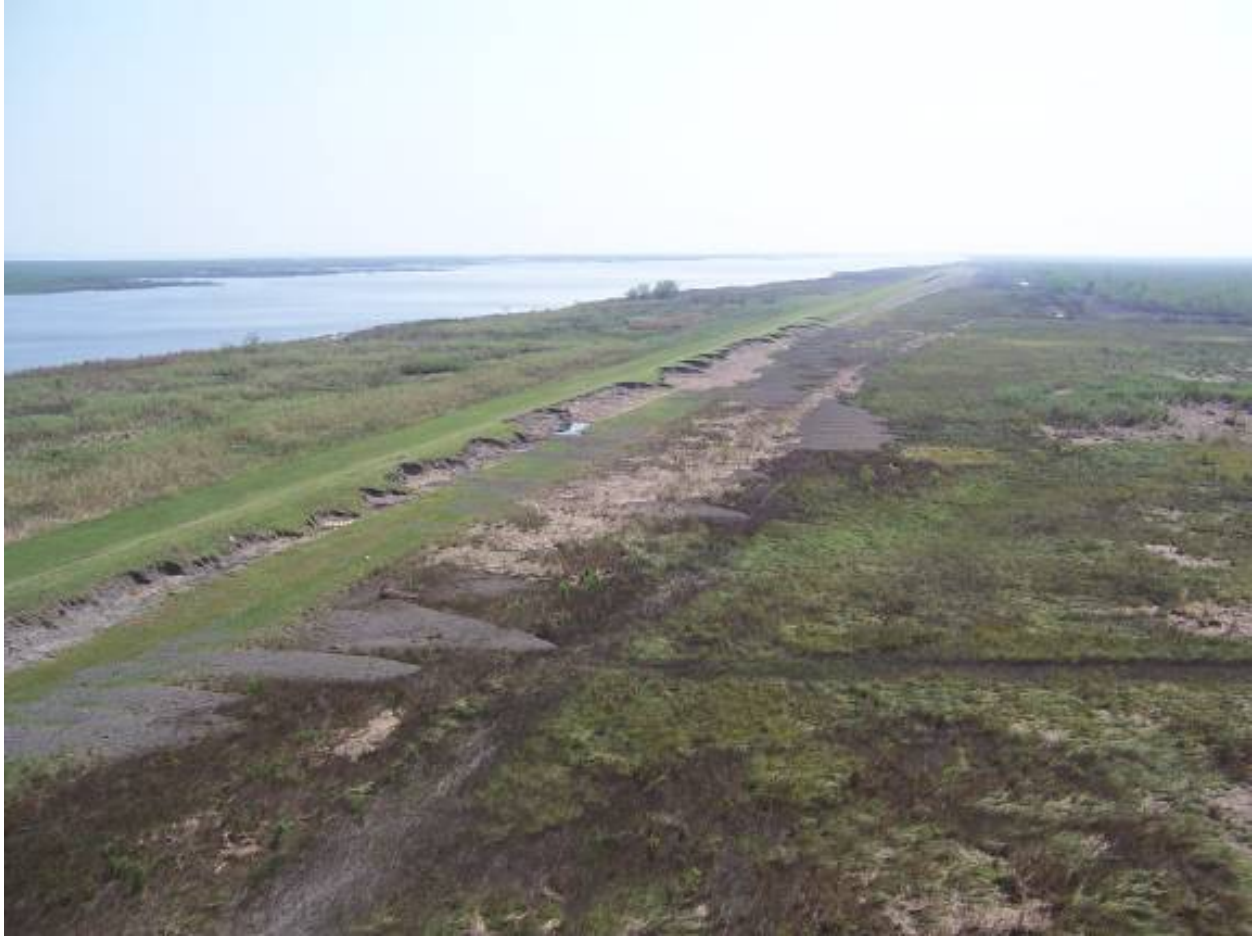
Figure 14-147. Major Scour on Protected Side of Levee
