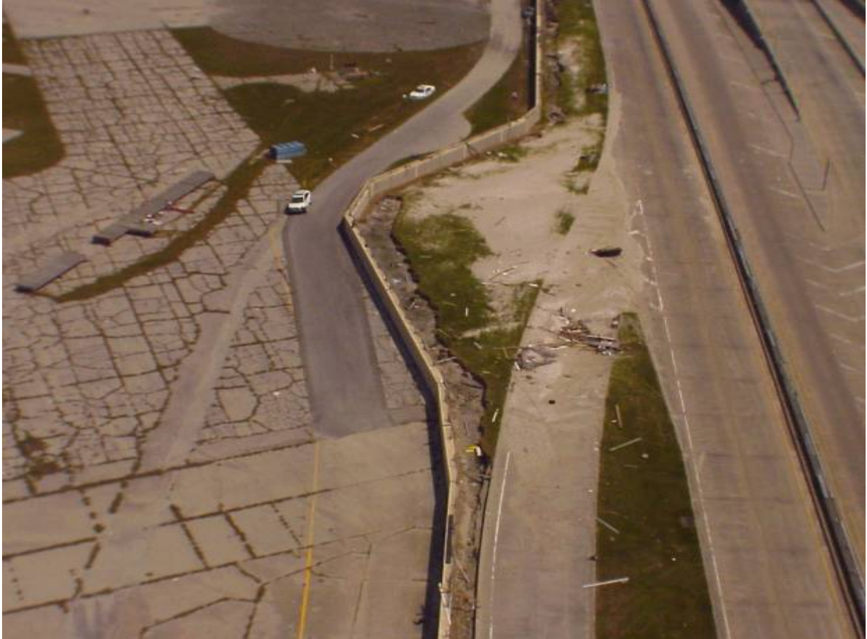
Figure 13-13. Lakefront Airport Floodwall. Scour is approximately 11 ft wide by 2 ft deep. Floodwall elevation is approximately 13.5 ft, ground elevation is approximately 6 ft, and wall height is approximately 7.5 ft
