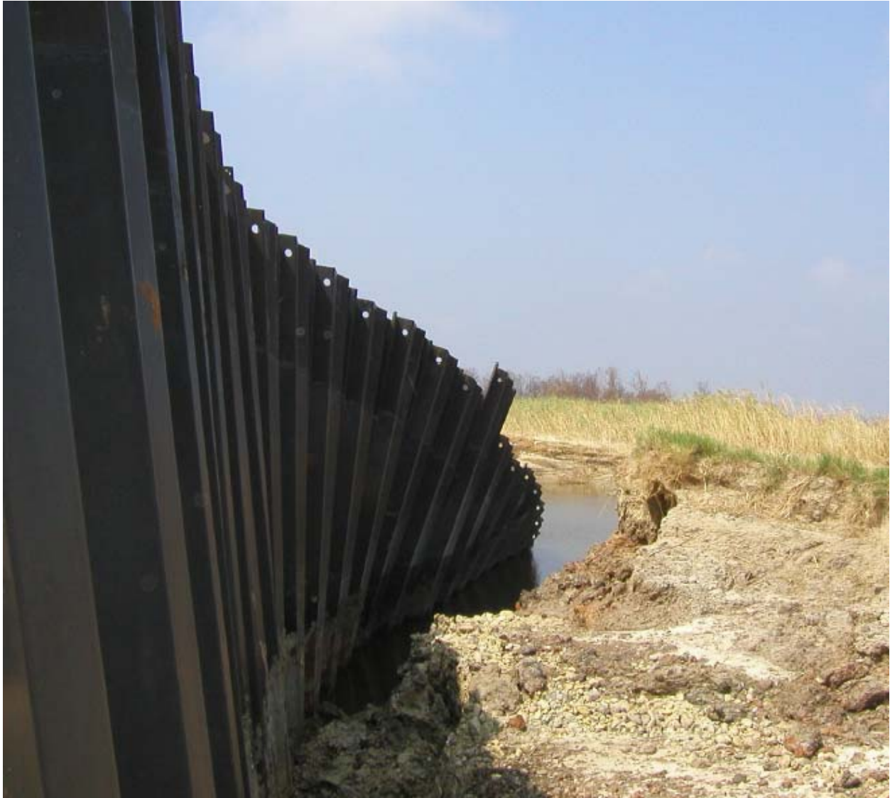
Figure 14-122. Closeup of Damaged Sheetpile and Scour. Note stratified layers in adjacent soil profile of existing hydraulic fill from the MRGO
