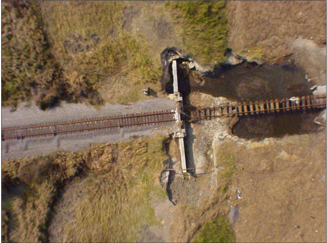
Figure 12-19. NOE5_C. View of Scour Around T-Wall
