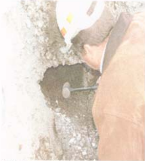
Photo 3 (Fig. 1) - Horizontal impact to sheet pile at 0.5 ft below concrete wall - protected levee side
