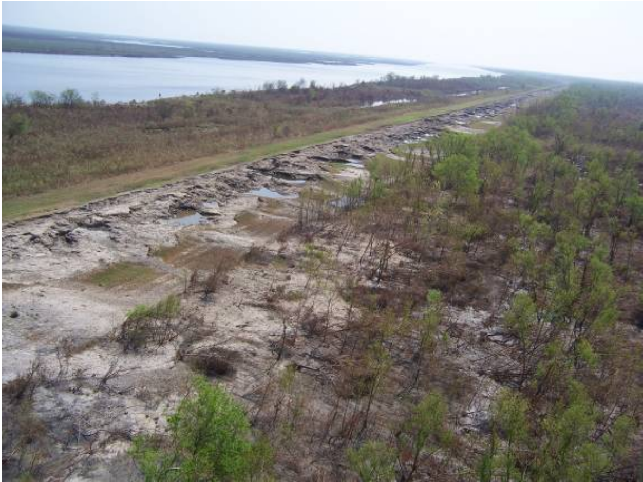
Figure 14-145. Scour Depths Below the Original Levee Footprint
