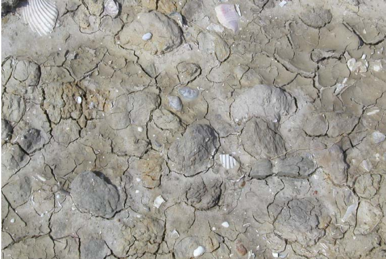
Figure 13-31. Exposed Soil Layer (final eroded surface) on Sheetpile Wall Backside Appears to be In-Situ Fat Clay with Embedded Shell Hash, Possibly an Exposed Estuarine Deposit
