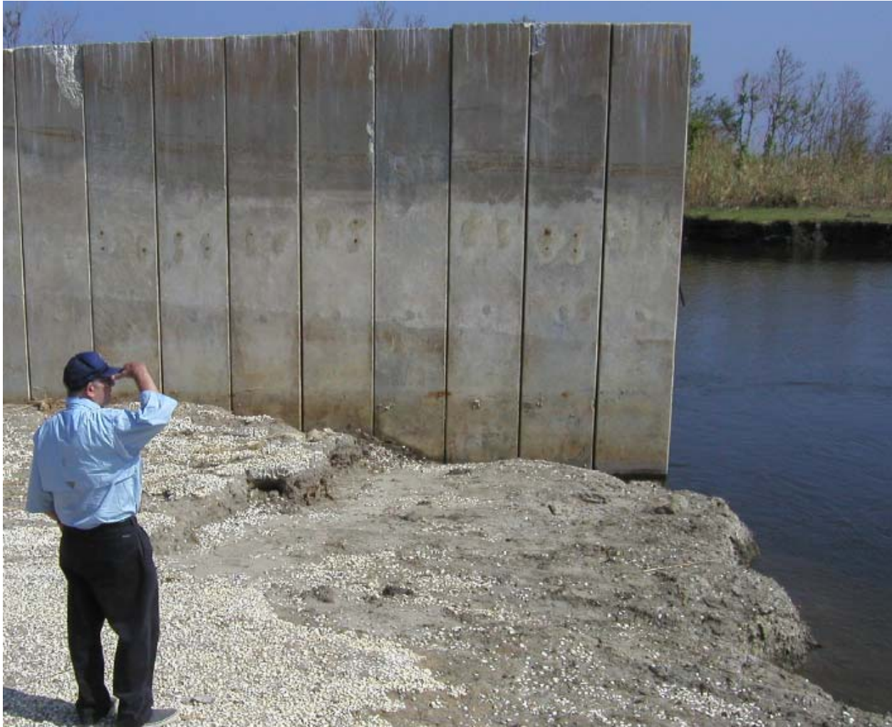
Figure 14-140. Missing Levee and Part of Wall on West Side of Control Structure
