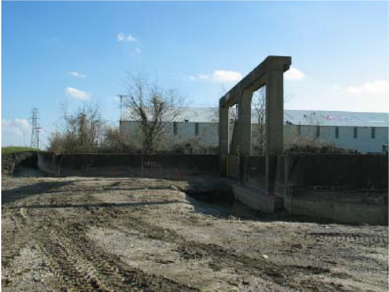
Figure 14-41. Scour at Gate 7E; Scour Measures 7' (w) x 30" (deep). Top of wall is at elev. 13.1 +/-
