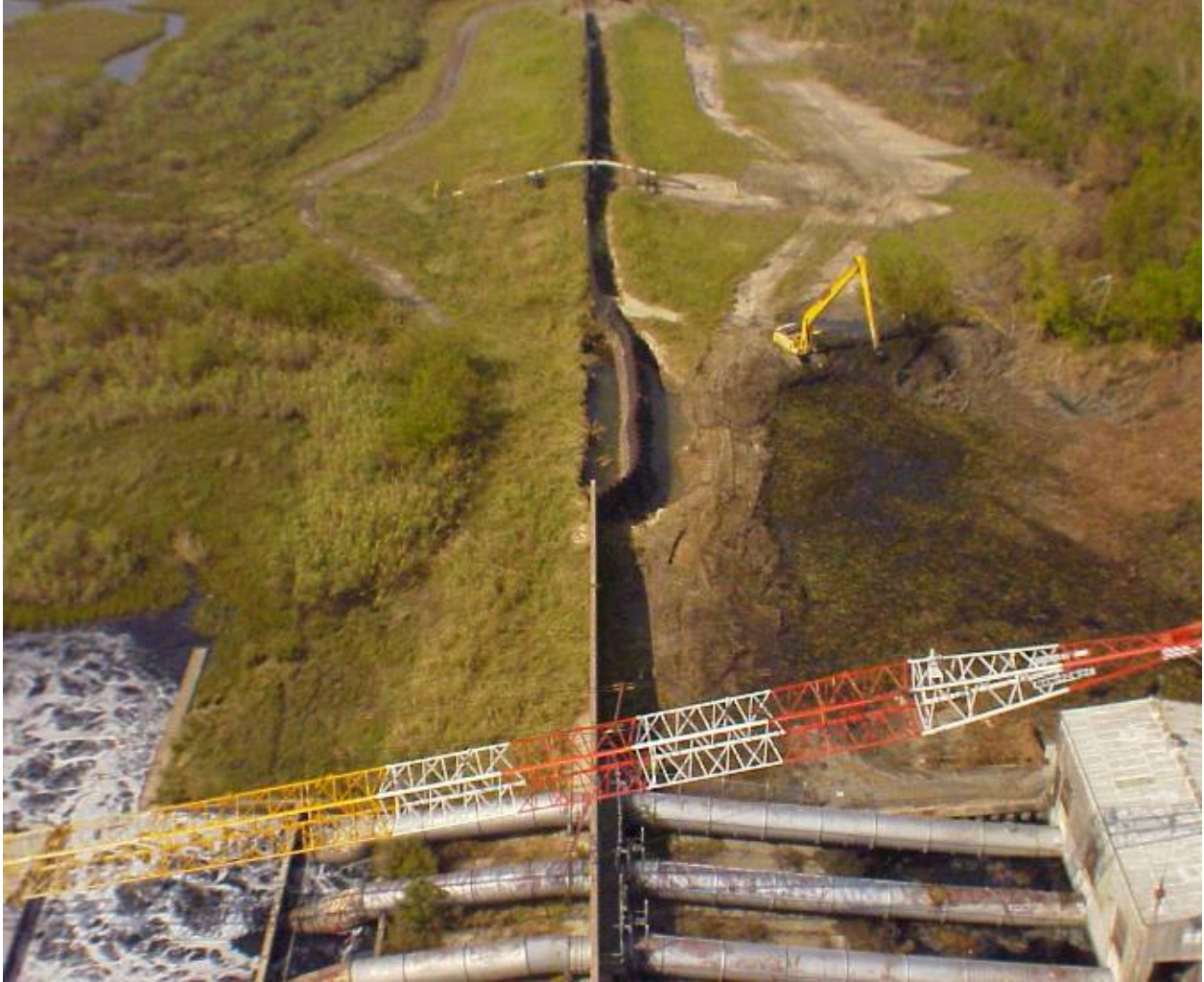
Figure 13-36. New Orleans East Basin, Pump Station 15 on the North Bank GIWW. Failed sheetpile between B/L Sta 874+40 and Sta 875+60 (N.O. East Back Levee). Pre-Katrina elevations ranged from 17.5 to 19.5 ft in this reach
