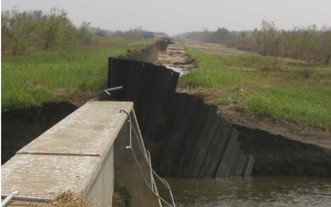
Figure 14-112. View Looking East of the Bayou Bienvenue Control Structure Showing Sheetpile Damage From Scour. From this picture there is no obvious layer stratification in the scoured section profile
