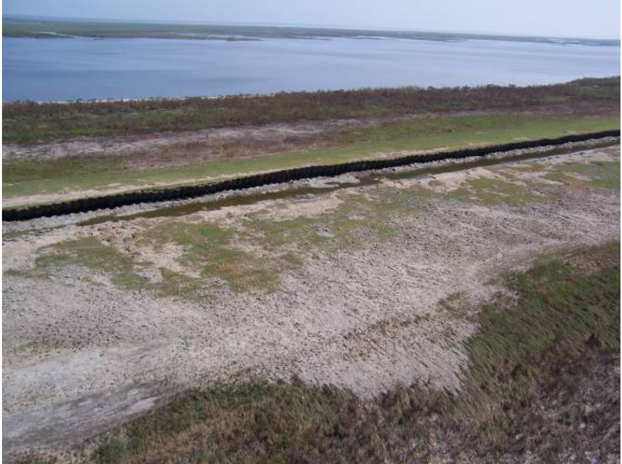
Figure 14-150. Scour on Protected Side of Sheetpile Wall
