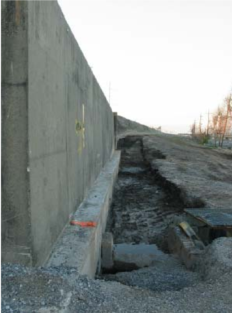
Figure 13-10. T-Wall Base Scour on Backside, East IHNC Near Lakefront Airport
