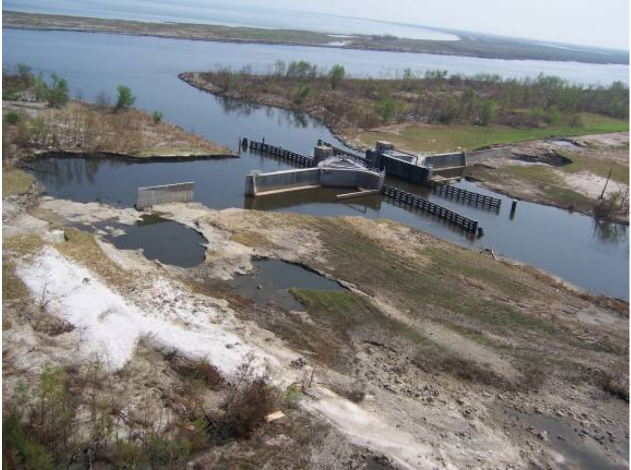
Figure 14-139. Bayou Dupre Control Structure, Post-Katrina. View toward MRGO. Note the missing levees on both sides of the structure
