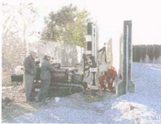
Photo 1 - Geoprobe Rig for PS/SCPT testing at South End of Breach of 17 th Street Levee at Station 17+78 where sheet piles were exposed by USACE PS Cased Borehole (white PVC cap visible)
