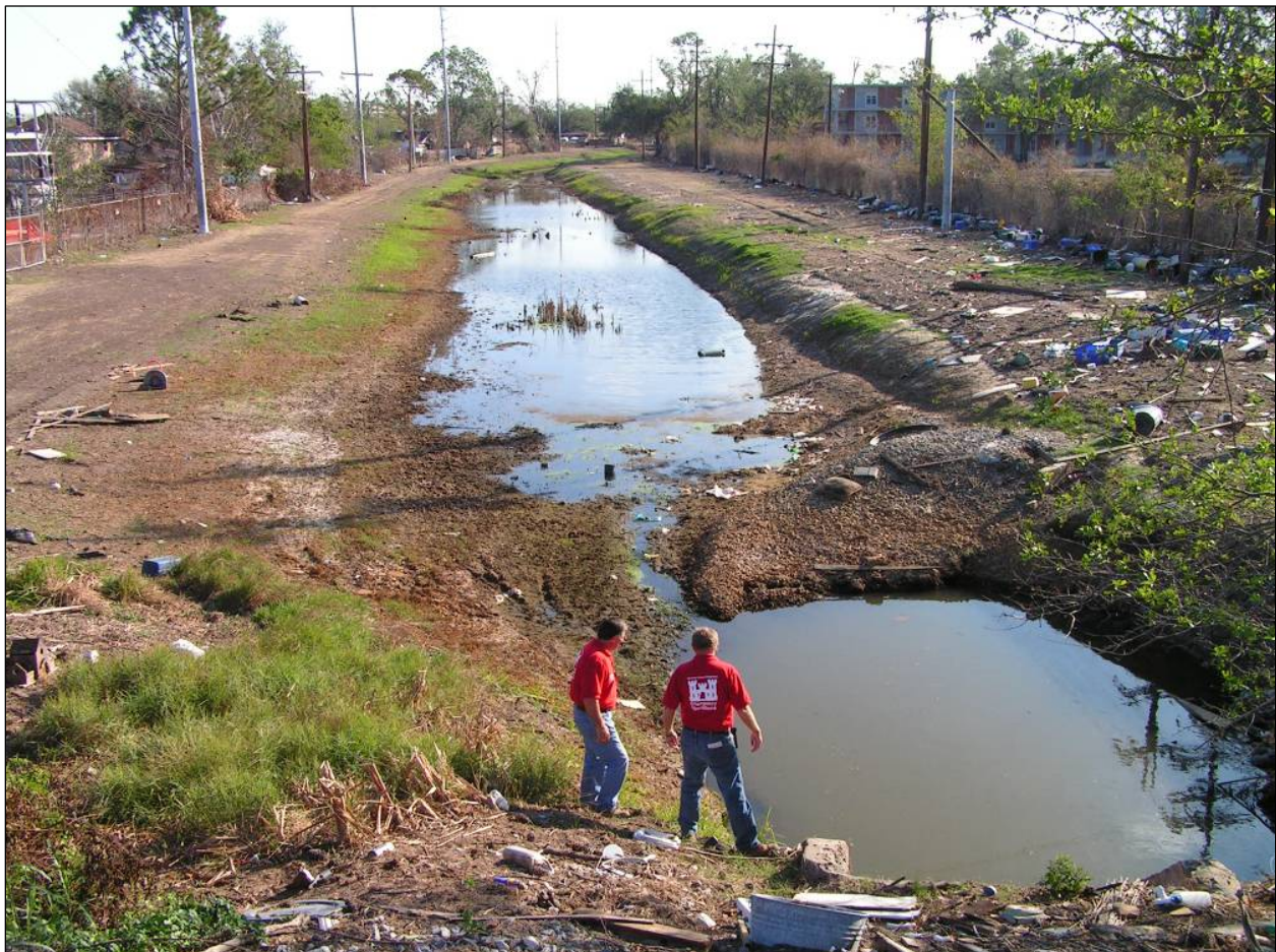
Figure 131. Scour hole east of railroad grade indicating flow from Peoples Canal into the Bartholomew Golf Course area.
