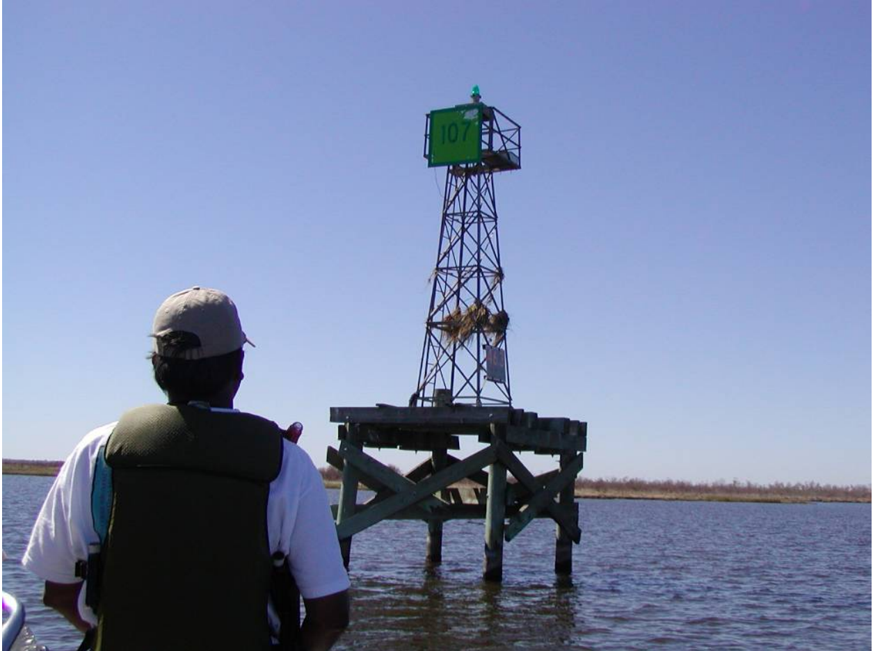
Figure 20. LA 1155 on MRGO. Debris on tower.
