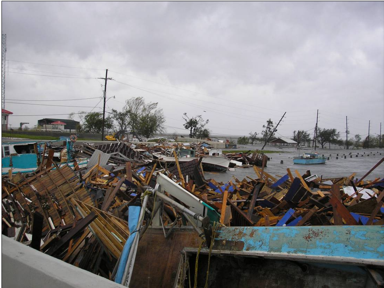
Figure 118. This image shows debris accumulated on north side of Hammond Highway bridge over the 17th Street Canal shortly before 2000 UTC (3:00 p.m. CDT) on Monday, 29 August 2005. The bridge railing is visible in lower left corner.
