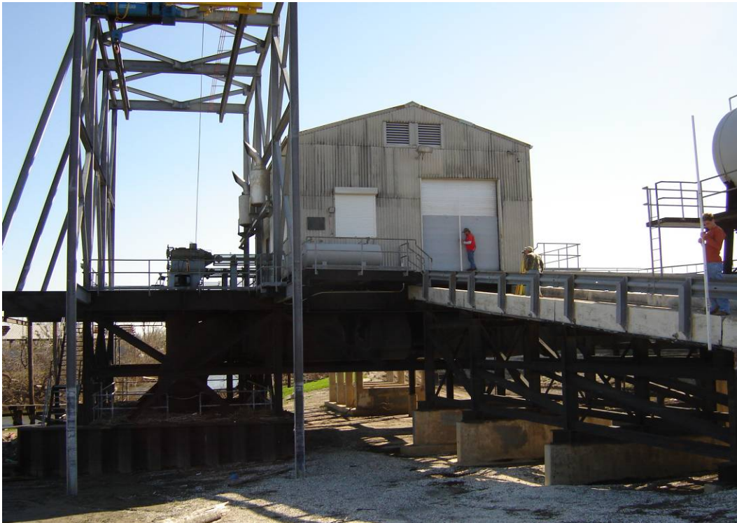
DUVIC(VENICE) PUMP STATION
