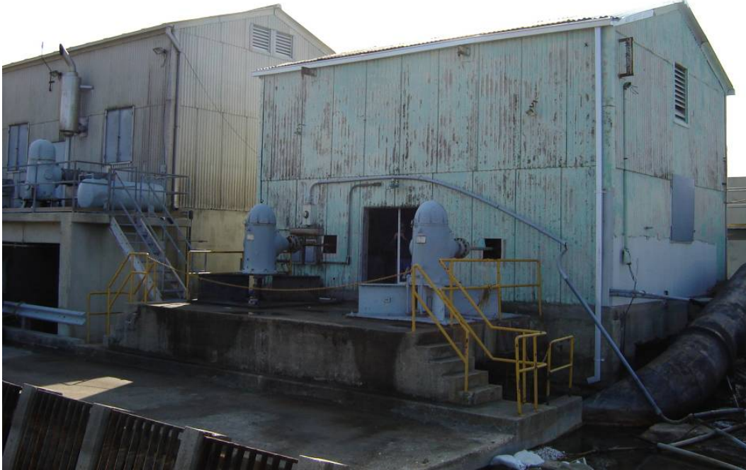
SUNRISE #1 PUMP STATION
