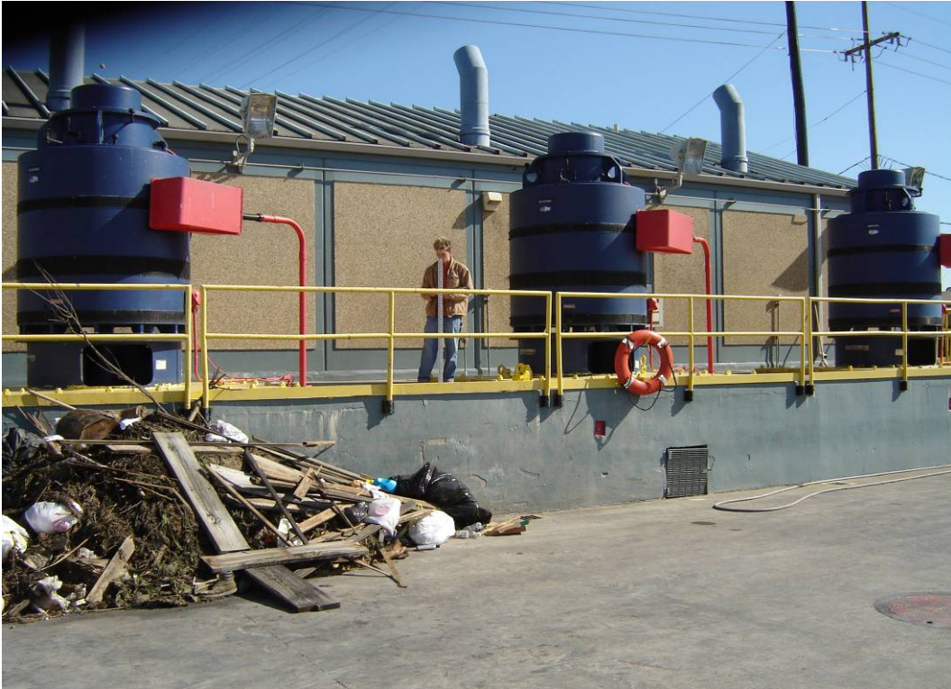
Harvey Pump Station
