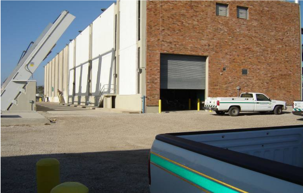
Pump Station JP-02
