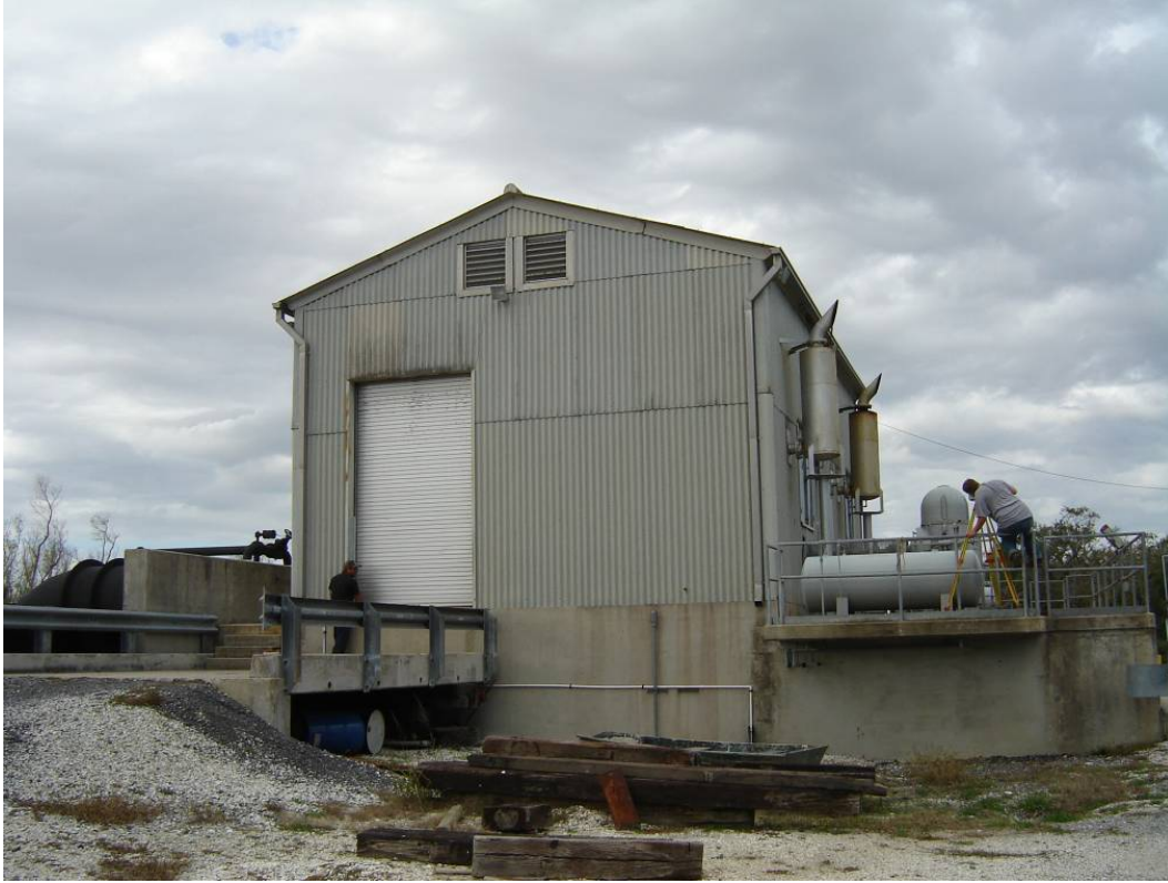
OLLIE #2 PUMP STATION
