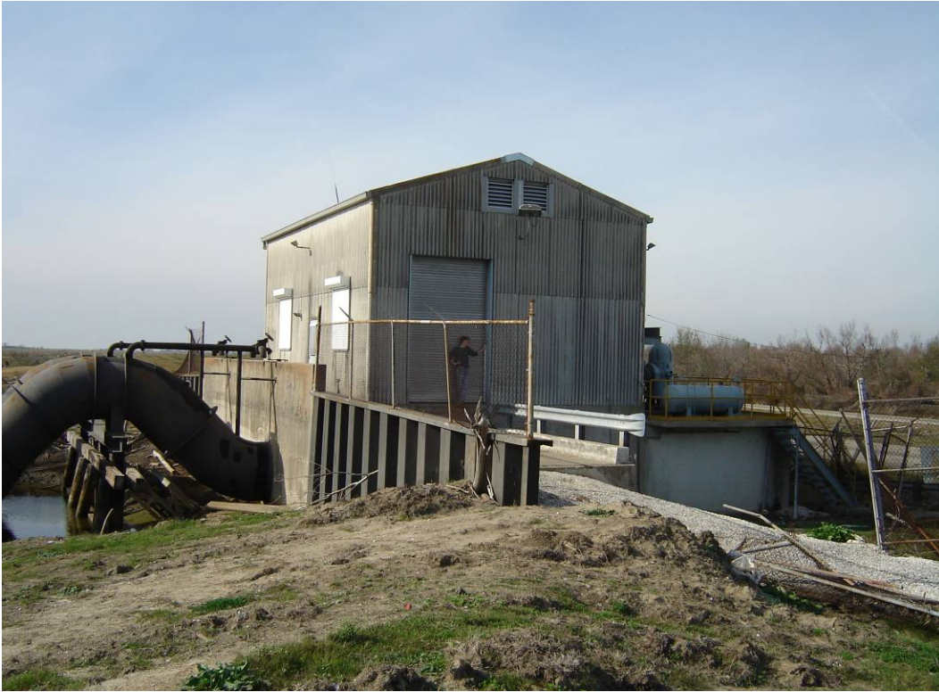
DIAMOND PUMP STATION
