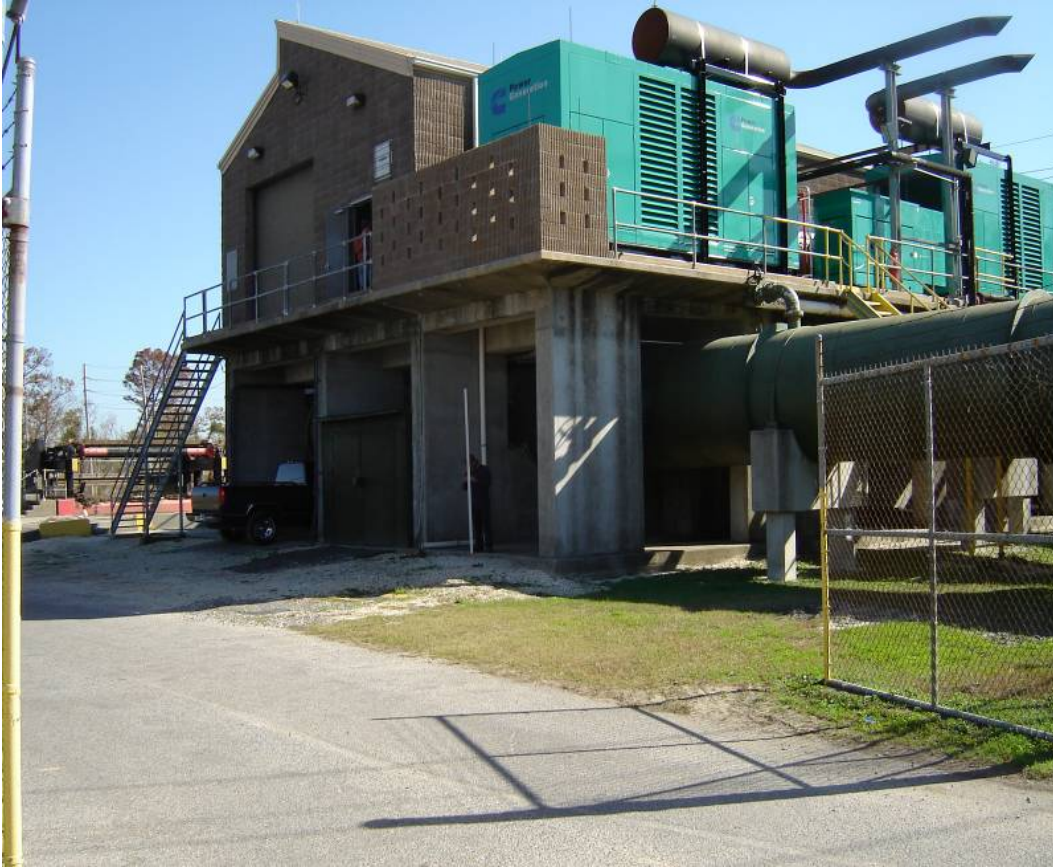
Parish Line Pump Station
