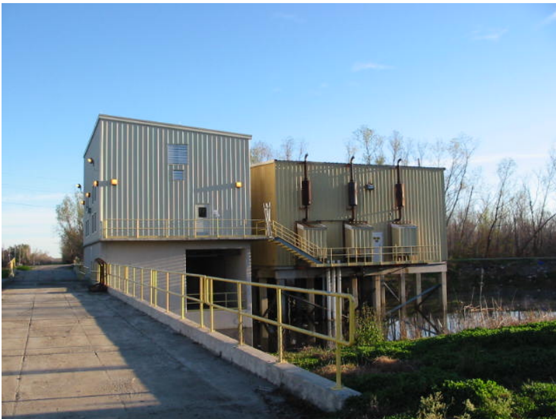
DESTREHAN #1 Pump Station
