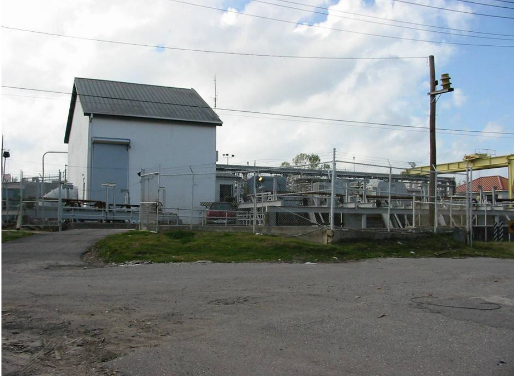
OP #4 Pump Station
