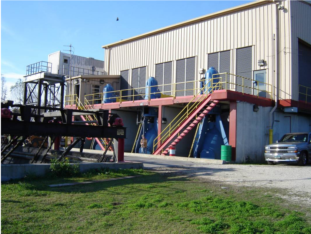
Westwego #2 Pump Station
