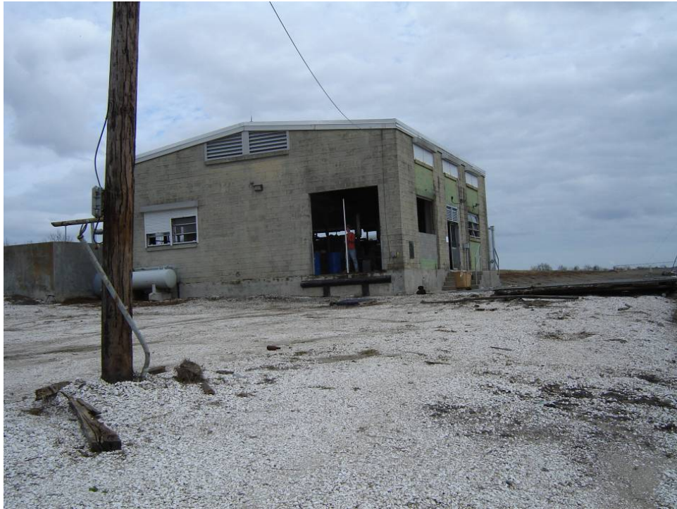
POINTE A La HACHE EAST PUMP STATION
