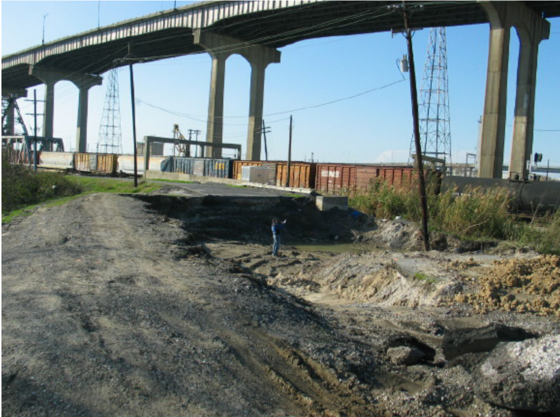
Figure 2-12. Major Washout Area from Overtopping Near I-10 Overpass (Citrus Back Levee)
