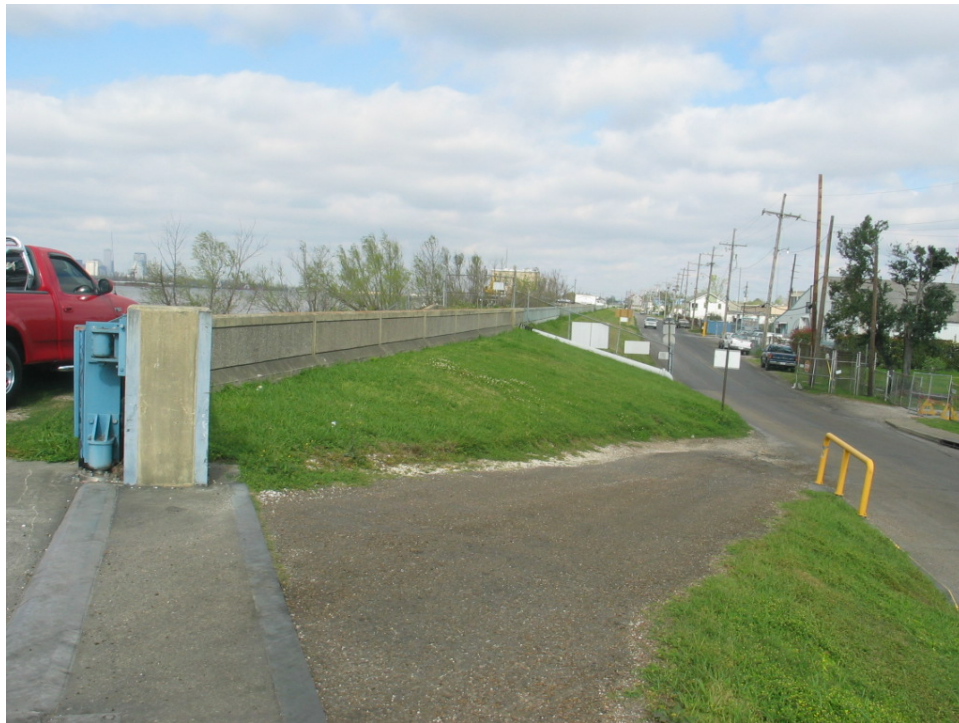
Figure 6-21. Concrete Capped I-wall Near Domino Sugar Plant (Closure represents key point within this reach)
