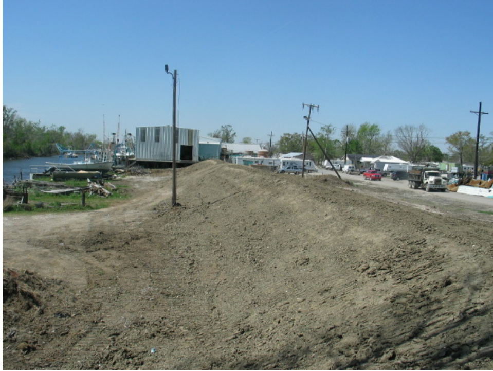
Figure 6-40. Repairs and Levee Raising to Reach STB39 Along Violet Canal (Viewed looking west from end of Reach STB38)
