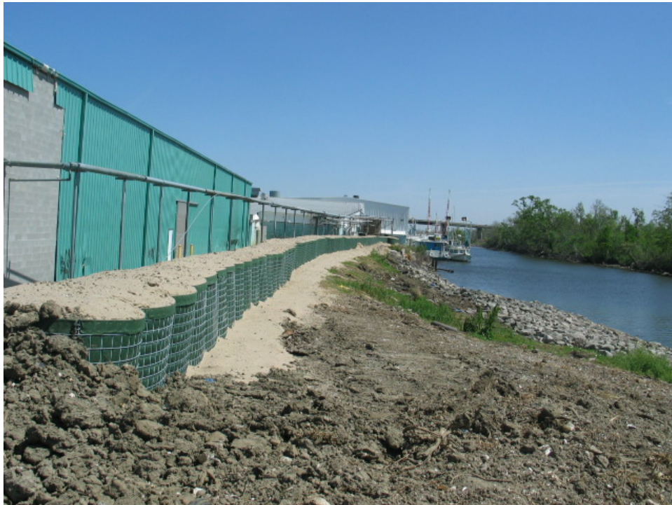
Figure 6-41. Gabion Basket Repairs to Reach STB40 (Viewed from west side of reach)
