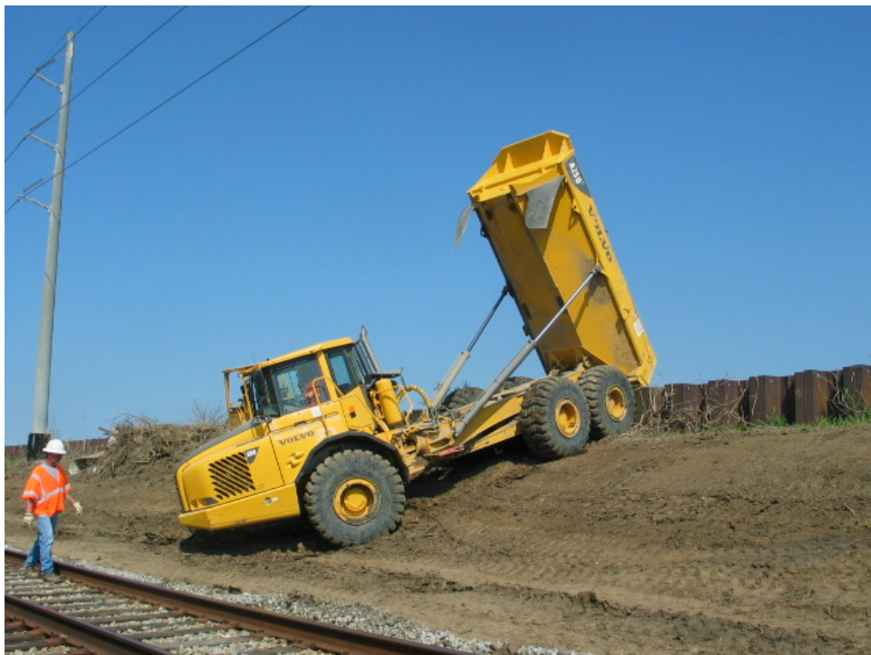
Figure 6-39. Repairs to ILL Along Reach STB33 Near Parish Border (Note: This section is being returned to pre-Katrina conditions)
