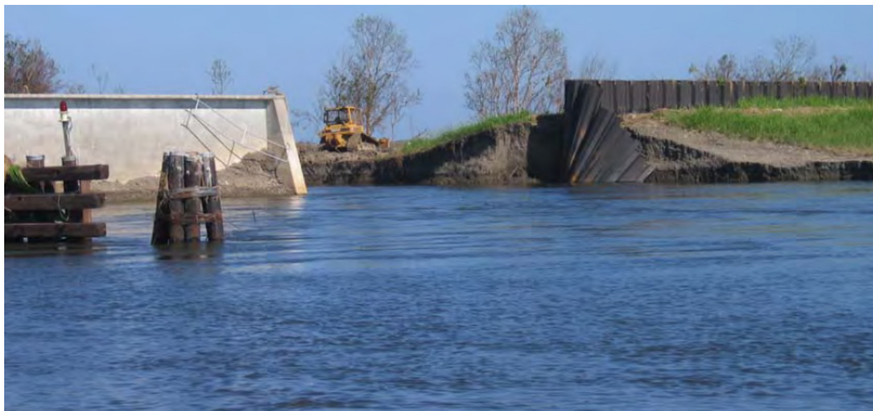
Figure 6-14. Picture of Failed Bienvenue I-wall from Protected Side
