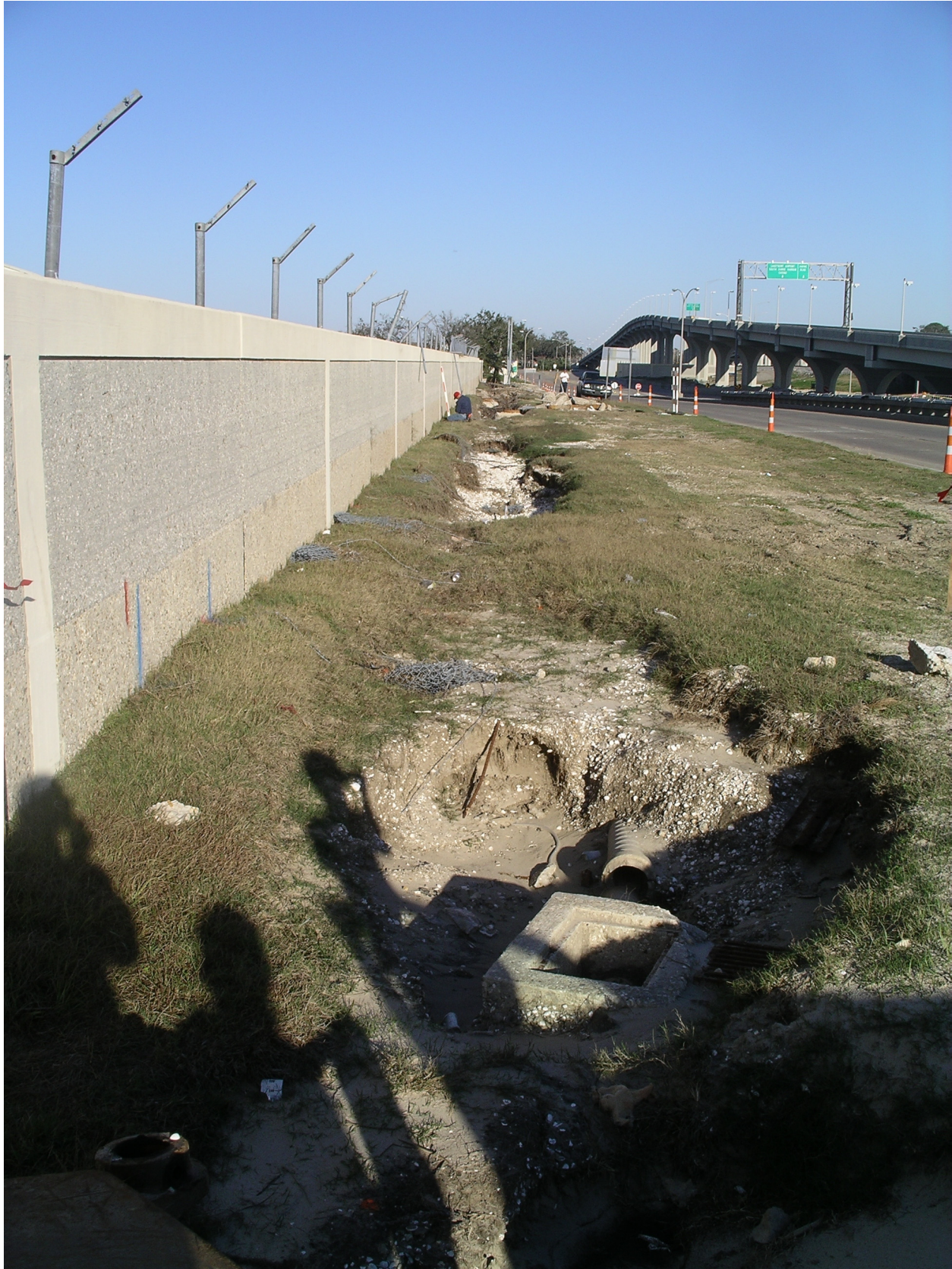
Figure 2-3. Scour Behind Lakefront Airport FW from Overtopping
