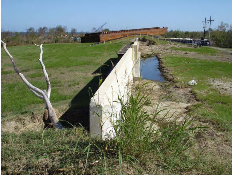
Figure 6-11. Floodwall Northwest Bienvenue Structure (Reach STB10) (Looking southeast toward Bayou Bienvenue just after Katrina)
