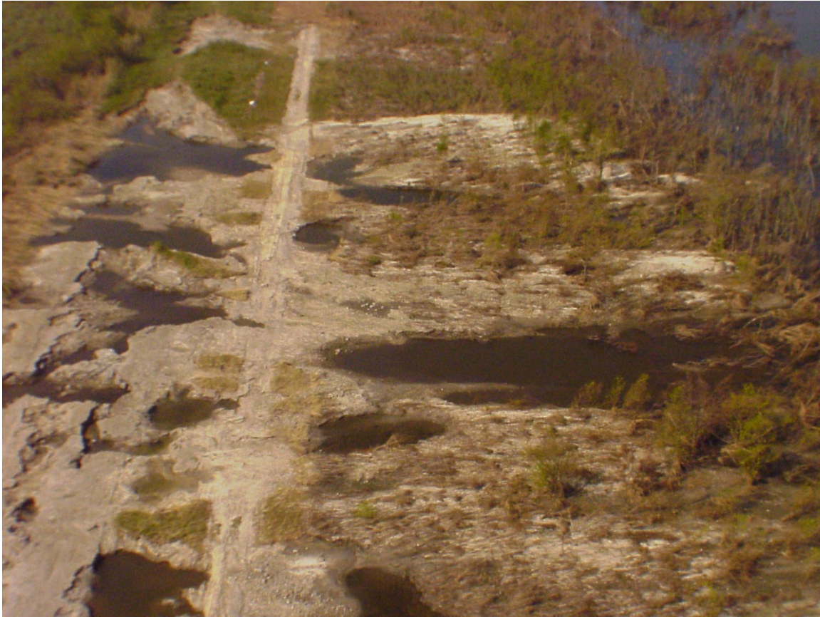
Figure 2-7. Failure of Levee by Overtopping East of PS #15 (East Back Levee)
