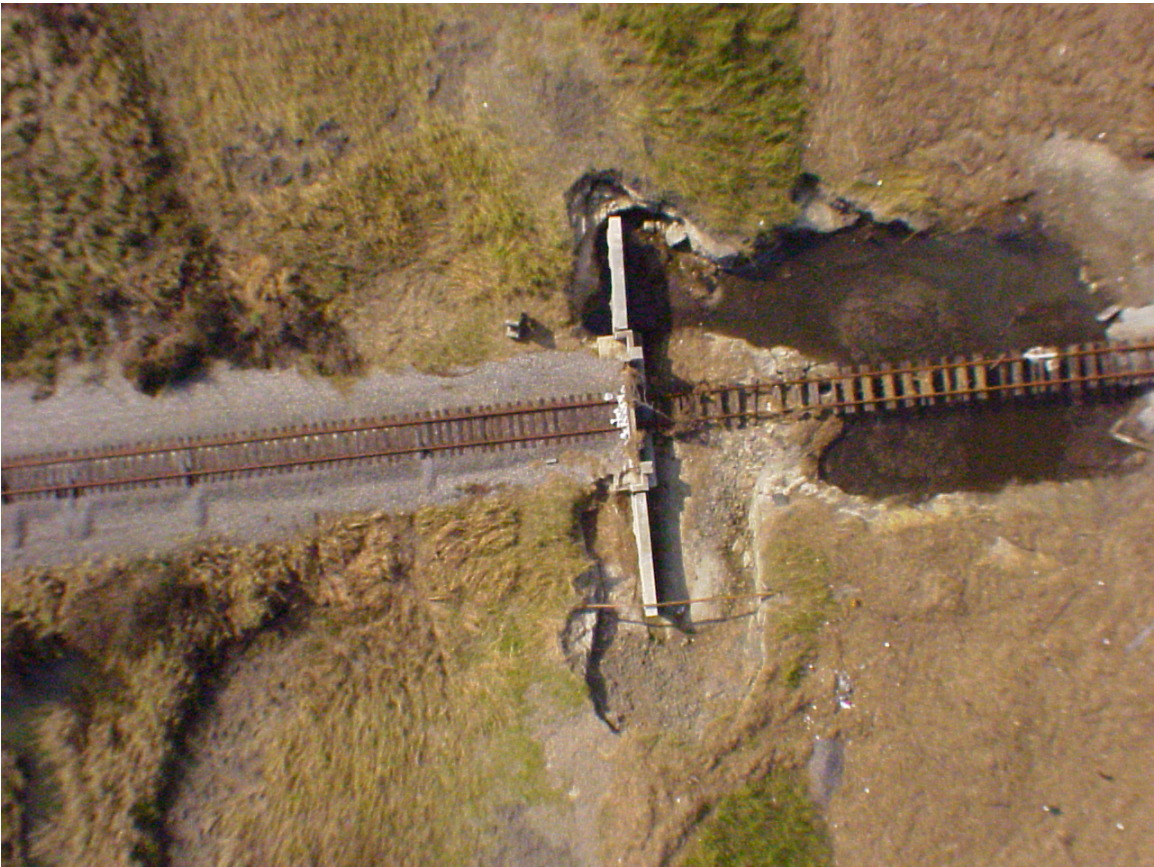
Figure 2-6. Aerial View of Damage at RR Closure Along East Levee (Point NOE12c on System Map)
