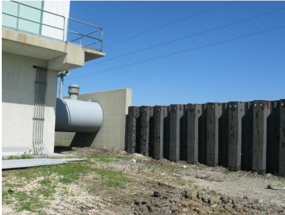
Figure 6-26. T-wall and I-wall offset at Pump Station #7 Along ILL (Note: wall offset is approximately 3 ½ feet)
