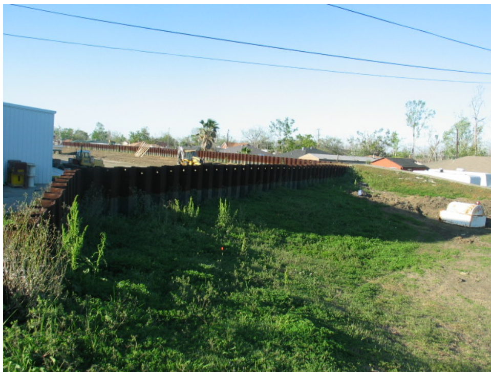
Figure 6-18. Uncapped Sheet Pile I-wall Near Caernarvon Canal (Building on left side is on flood side)
