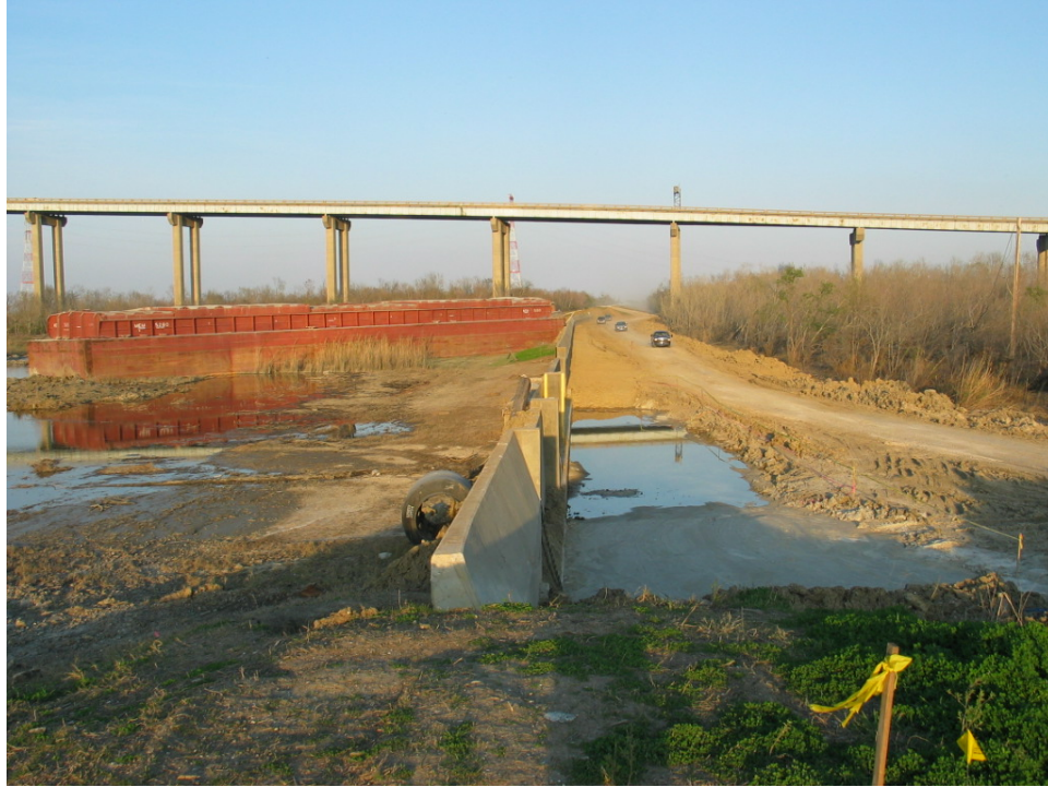
Figure 6-10. Paris Road Floodwall (Reach STB8) (Looking east from the west end of the floodwall)
