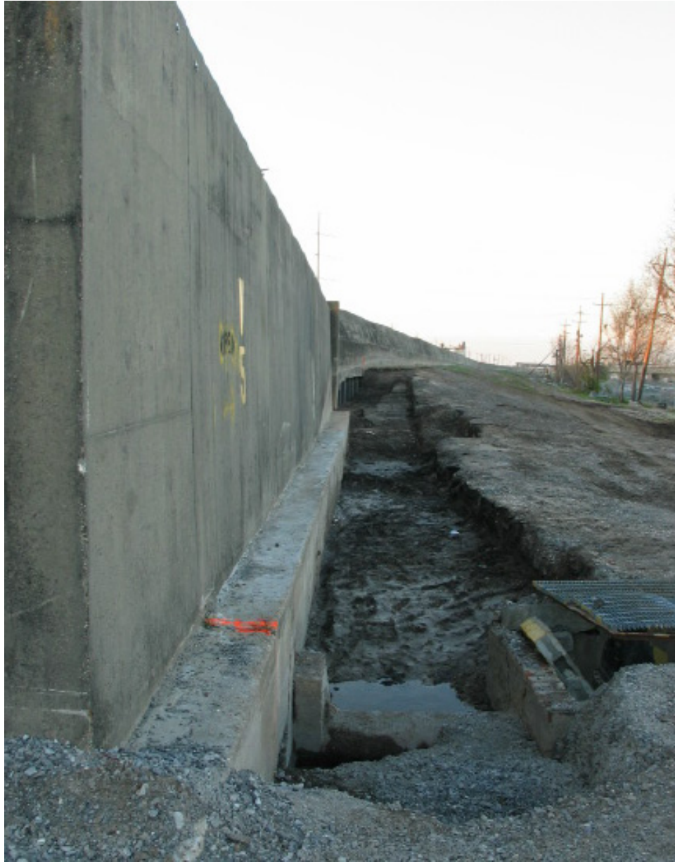
Figure 2-14. Erosion Behind Floodwall Adjacent to Gate E-13 (IHNC East)
