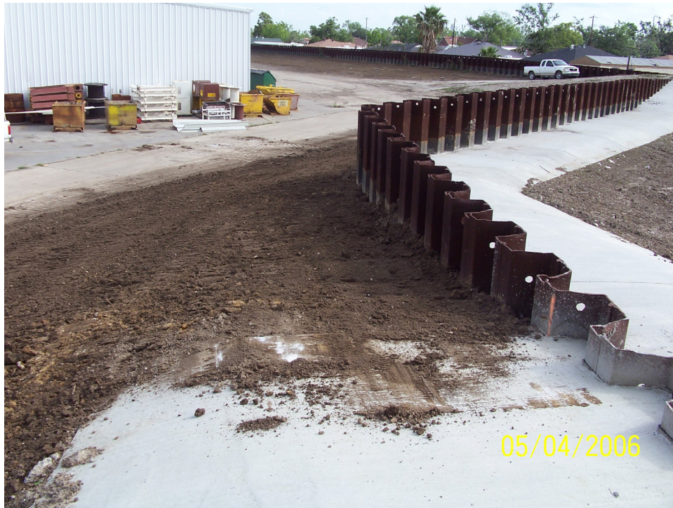
Figure 6-38. Scour Repairs to Caernarvon Sheet Pile I-wall Area (Note: compare to pre-Katrina condition shown in Figure 6-18)
