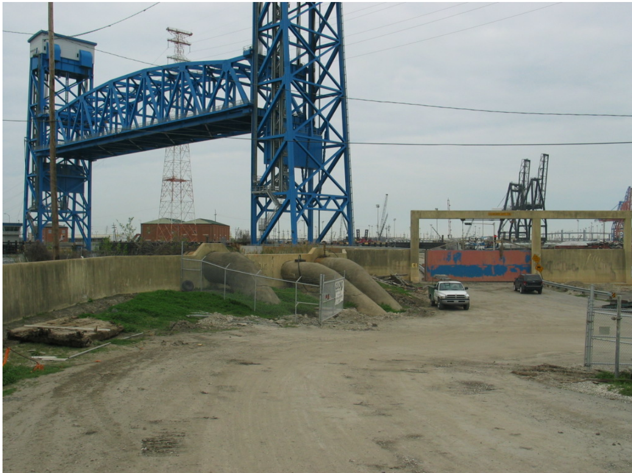
Figure 6-8. Existing T-wall Near Florida Ave. Bridge (Reach STB3) (Looking from protected side towards IHNC)
