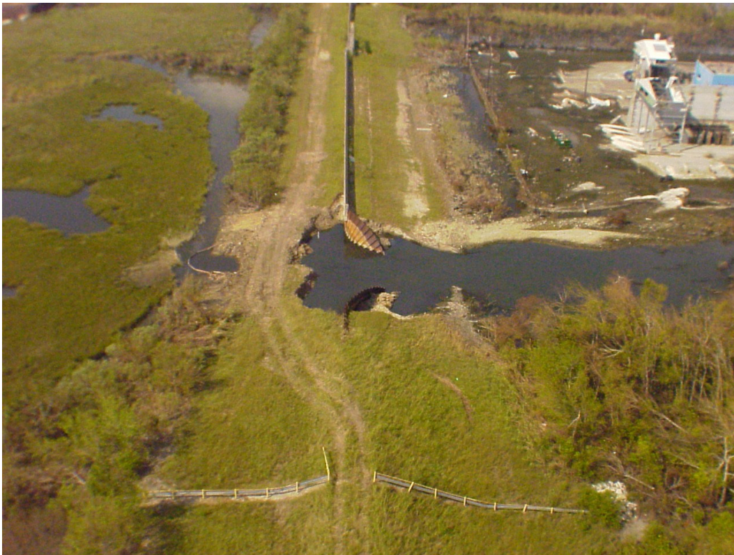
Figure 2-9. Floodwall Failure at East End of Michoud Canal FW
