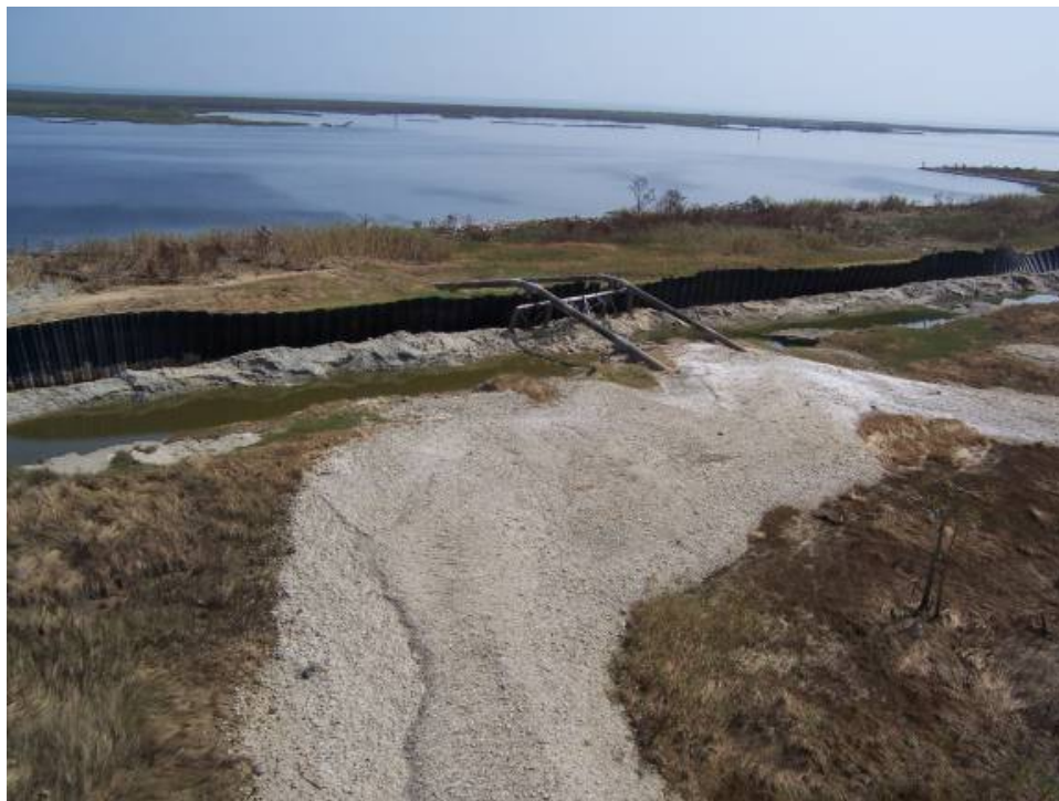
Figure 6-15. Failed I-wall Along MR-GO
