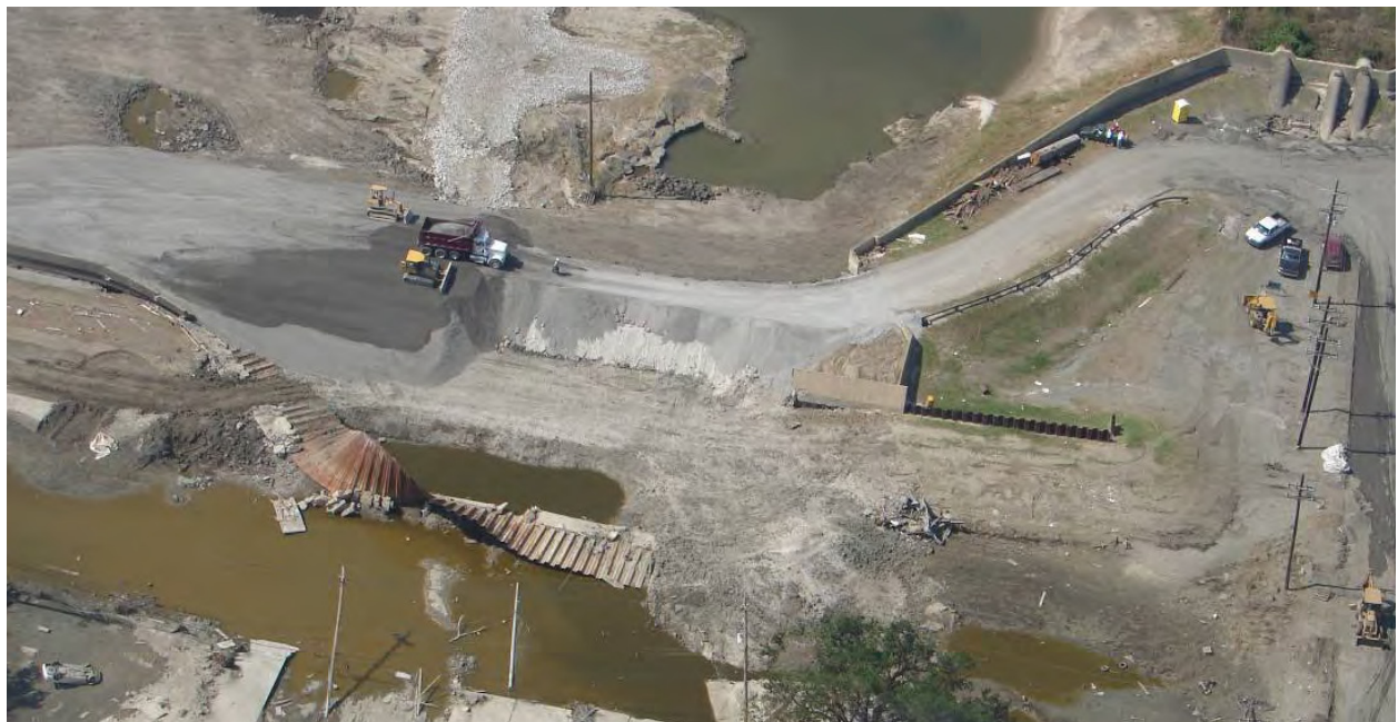
Figure 6-7. North I-wall Failure within Lower 9th Ward (Reach STB2) (Note: pipes on right side of photo are associated with Pump Station #5)
