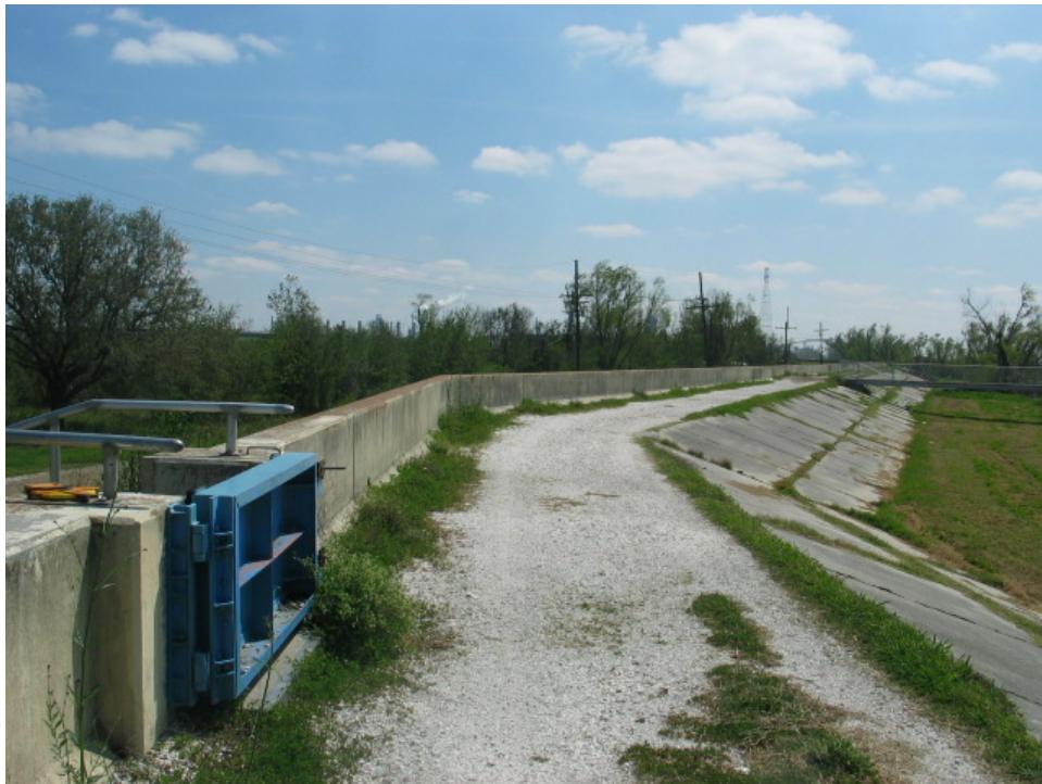
Figure 6-20. Concrete Capped I-wall Along Miss. River Near Battlefield (Access closure gate is key point within this reach)
