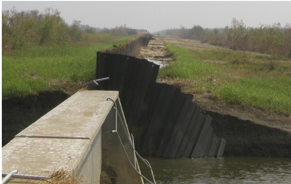
Figure 6-13. Failed Uncapped I-wall Section on Southeast Side of Bayou Bienvenue Control Structure (Looking southeast along the MR-GO)
