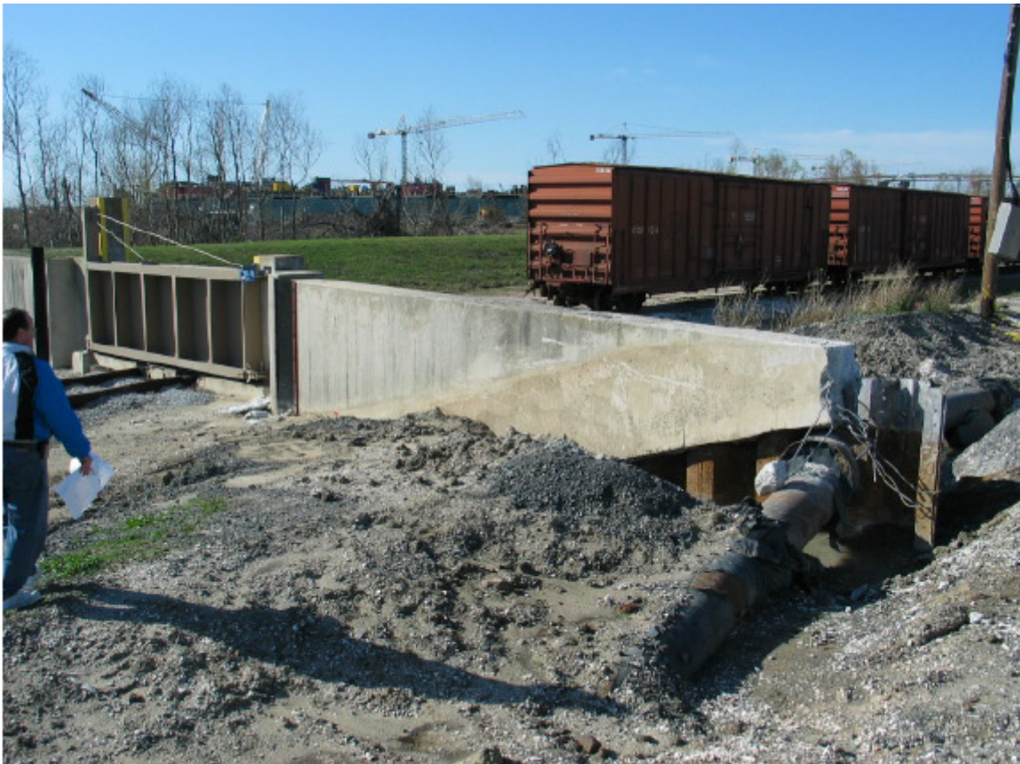
Figure 2-11. Erosion Damage Around RR Closure (Citrus Back Levee)
