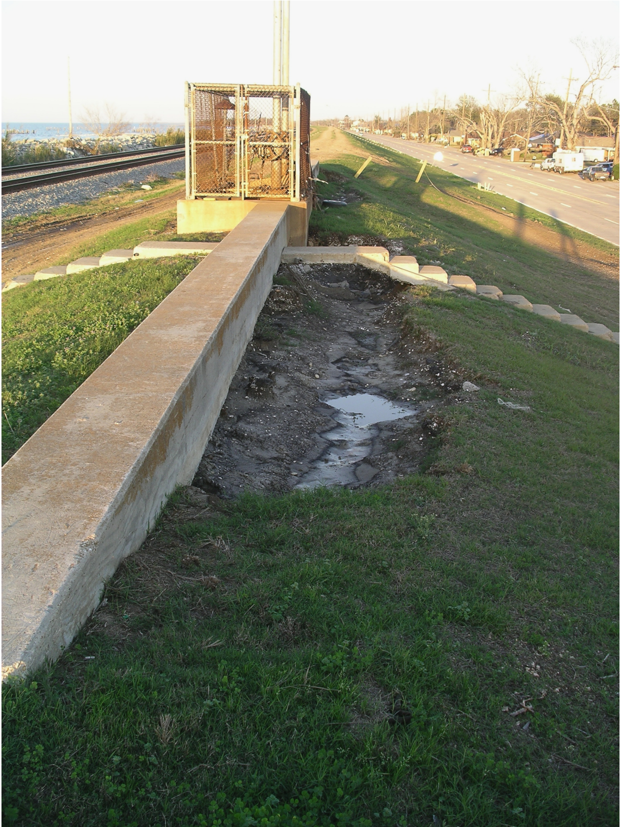
Figure 2-4. Minor Scour from Overtopping at Jahncke Pump Station
