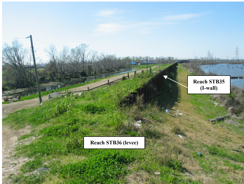
Figure 6-25. End of Reach STB35 @ Beginning of Reach STB36 (Interior Local Levee near Paris Road)
