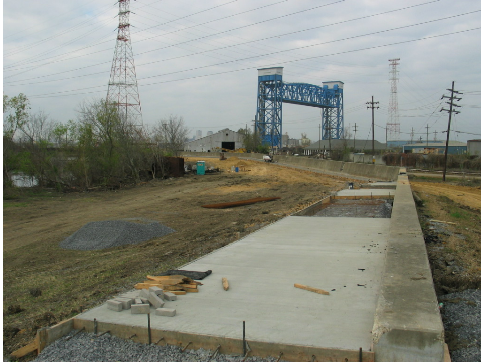
Figure 6-30. New Scour Protection Pad (Typical) (Photo taken at end of Reach STB4 looking back toward IHNC)
