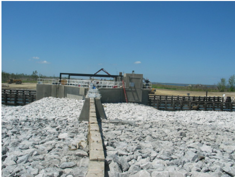
Figure 6-37. Repairs to Southeast Adjoining Walls at Bayou Dupre (Viewed from southeast side looking northwest along the MR-GO)
