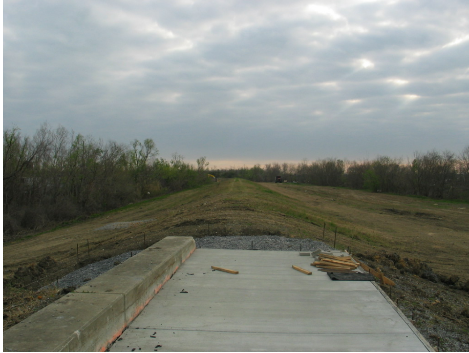
Figure 6-9. Beginning of Reach STB5 at End of I-wall (Note TFG improvements to Reach STB4 in foreground)
