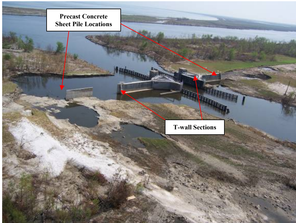
Figure 6-16. Damage at Bayou Dupre Control Structure (Note failed section of precast concrete pile wall)
