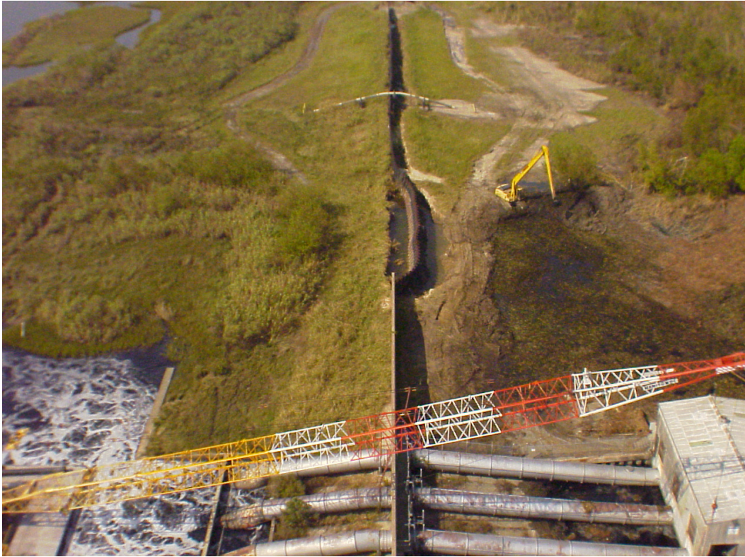
Figure 2-8. Floodwall Failure Near Orleans Pump Station #15
