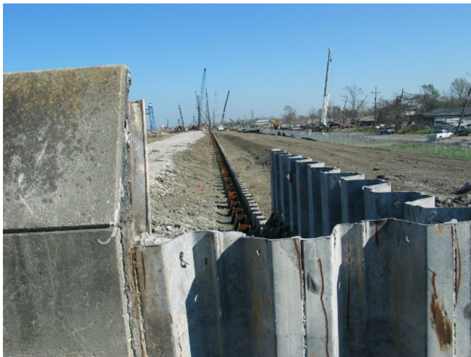
Figure 6-28. New T-wall Being Constructed Along IHNC (Reach STB2) (Looking north along the IHNC)
