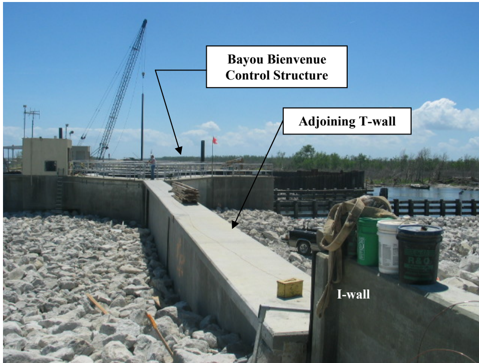
Figure 6-34. Riprap Placement Around Northwest Floodwall Adjoining Bayou Bienvenue Control Structure (Looking southeast along MR-GO)
