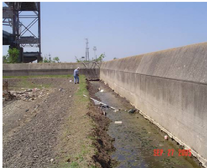
Figure 6-4. Section of Reach STB1 Overtopped During Katrina (Location is just north of Claiborne Avenue Bridge)
