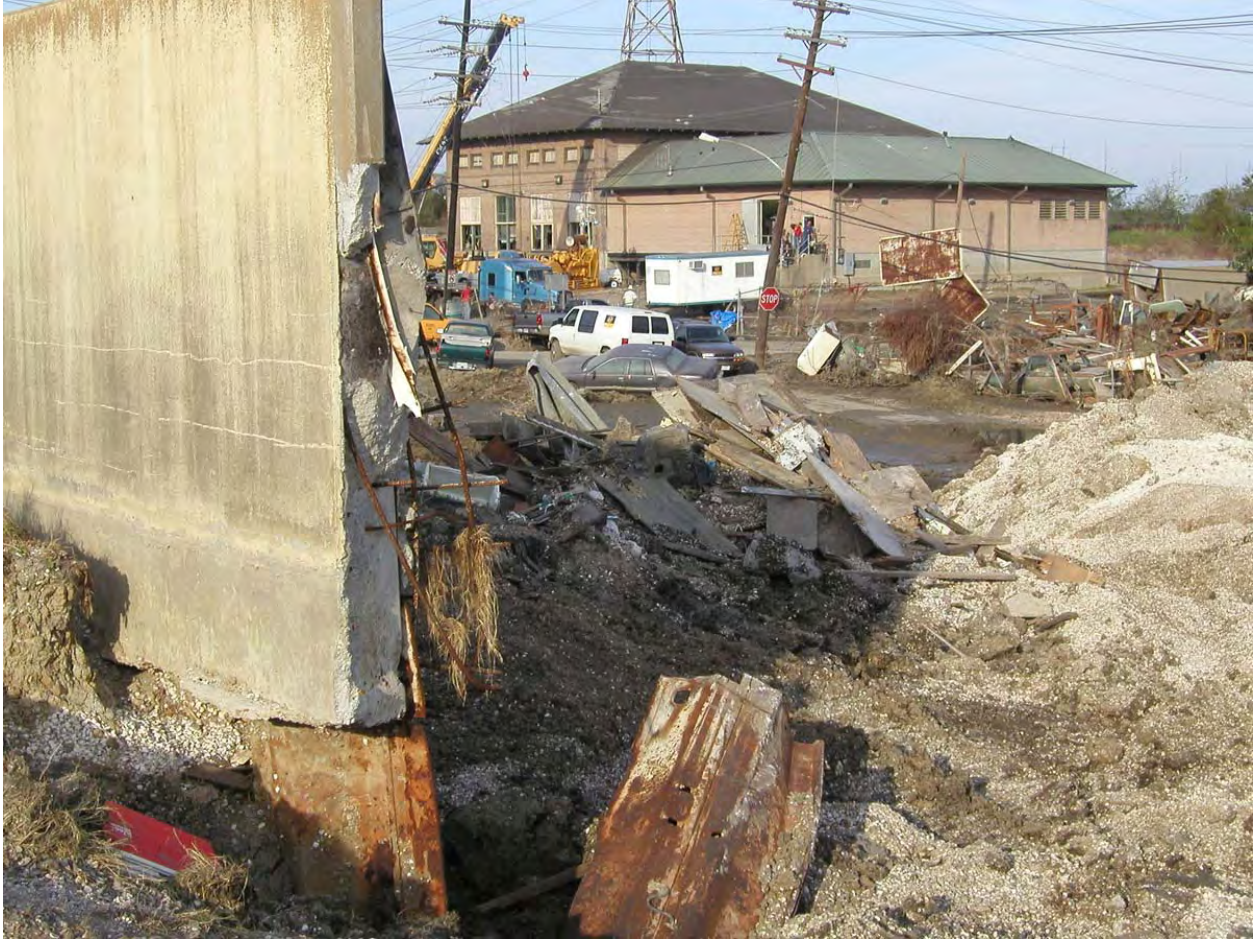
Figure 14-32. Northernmost I-Wall Failure Transition Between Florida Ave and Claiborne Ave., View Toward Pump Station on the Protected Side
