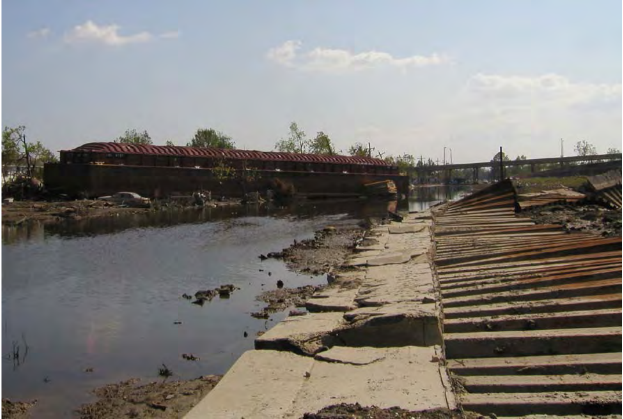
Figure 14-24. Closeup of Flattened I-Wall and Barge, View Toward Claiborne Ave.
