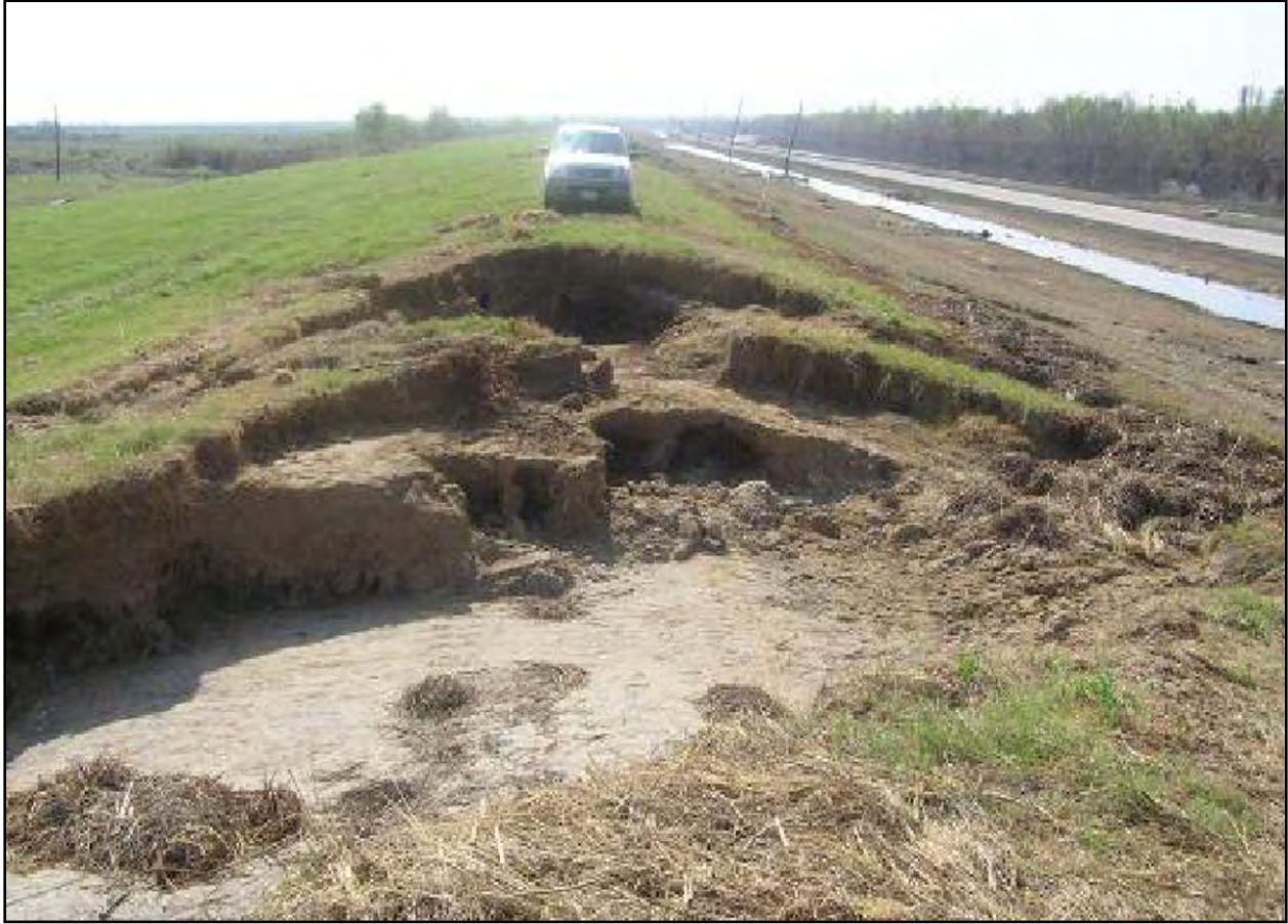
Figure 13-59. Plaquemines Parish East Bank Back Levee Erosion
