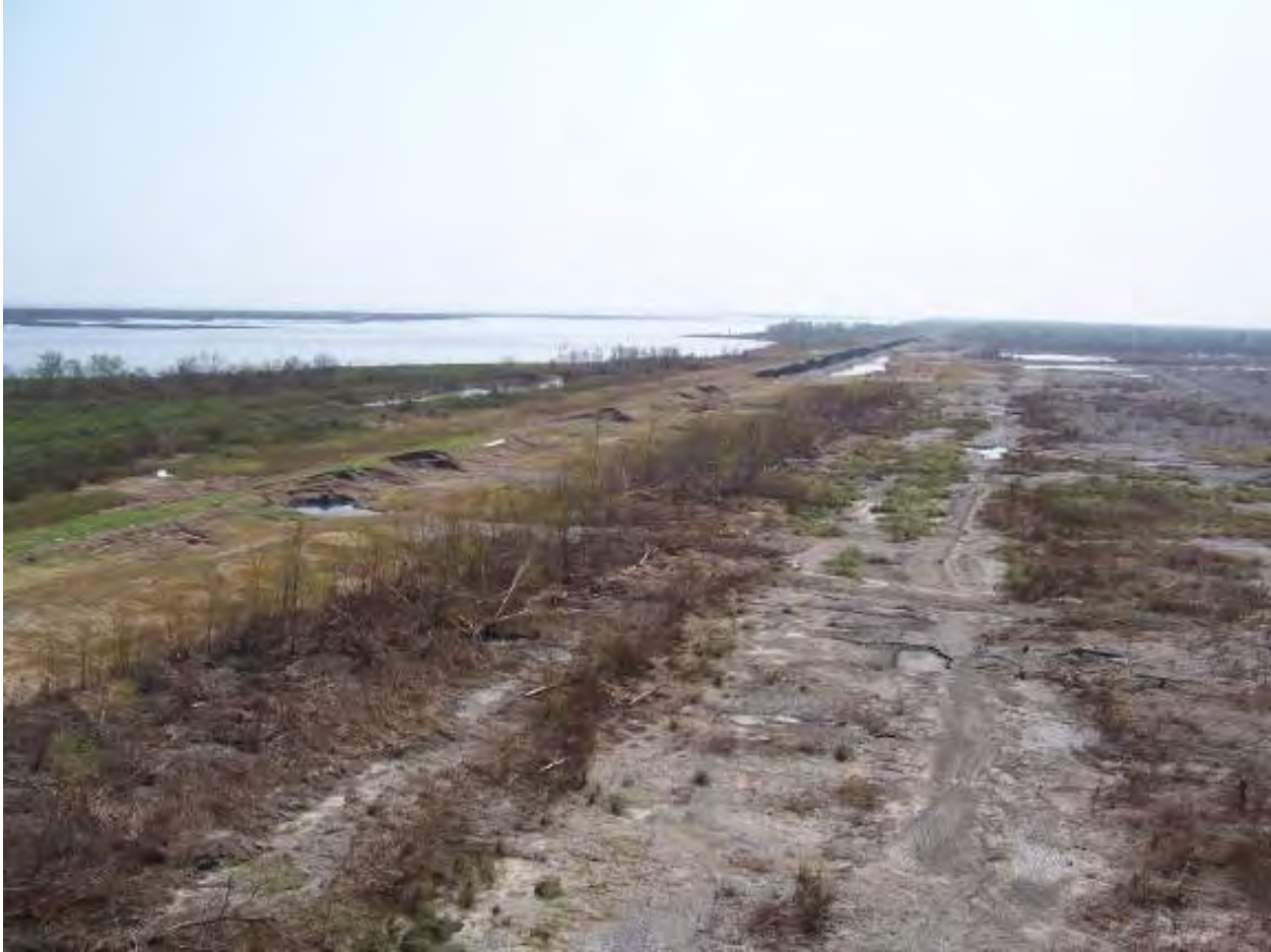
Figure 13-55. Levee with Eroded Crown Between Bienvenue and Dupre Bayous, View South From Approximate B/L Sta 570+00. MRGO is to the Left of Photo
