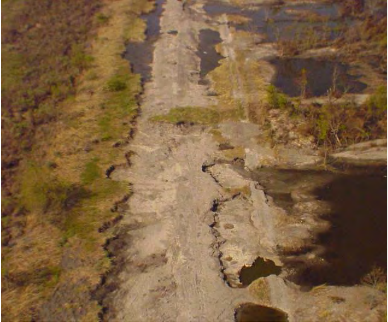
Figure 13-60. East of Pump Station 15 (N.O. East Back Levee), North Bank of GIWW. 12,750 feet of levee east of Pump Station #15 was completely degraded (Station 876+87 B/L to 1101+90 B/L). West of the pump station, 9,800 feet of levee was completely degraded (approx Sta 778+00 to 876+00). The levees in these reaches were constructed from GIWW hydraulic fill in stages over three years
