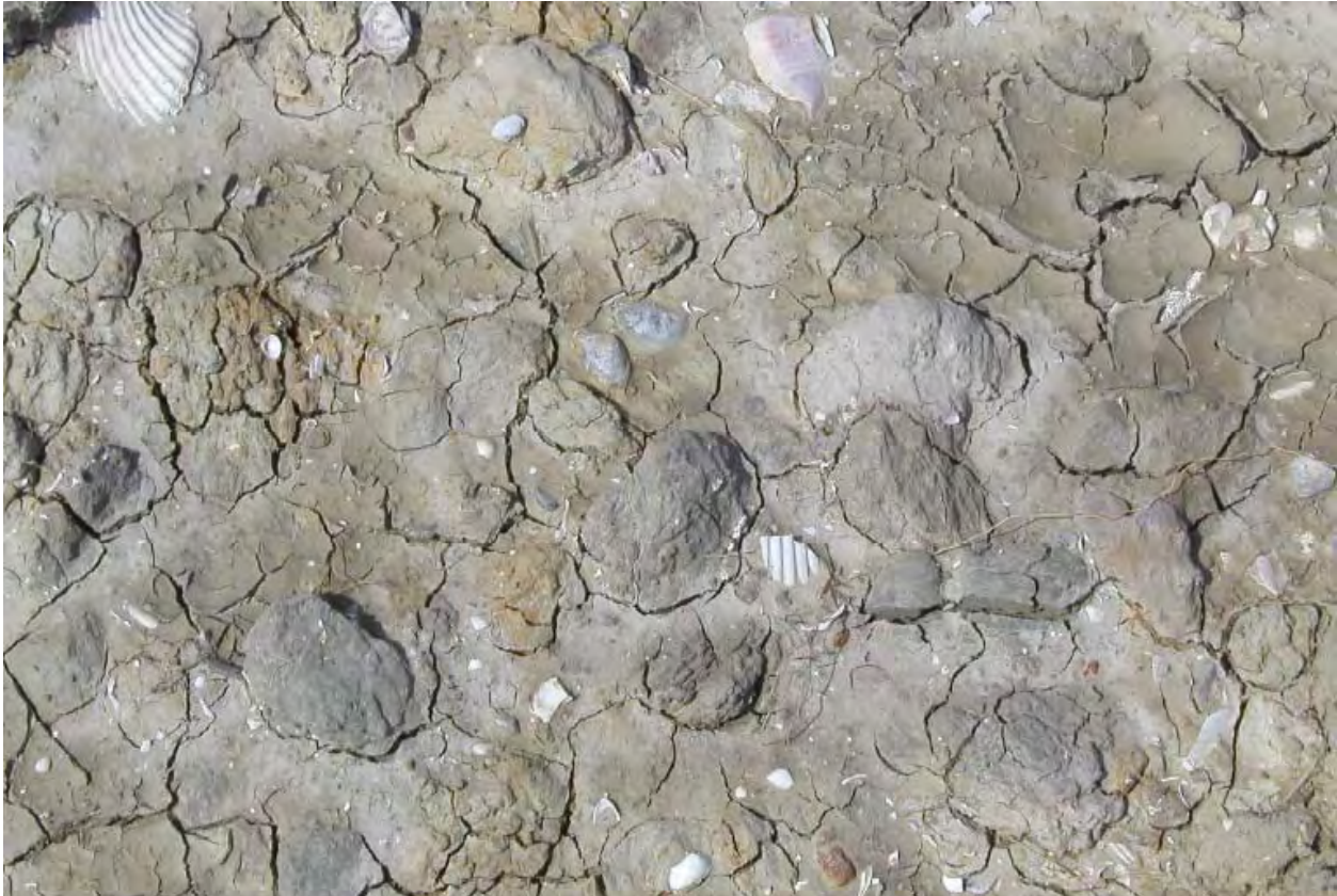
Figure 13-31. Exposed Soil Layer (final eroded surface) on Sheetpile Wall Backside Appears to be In-Situ Fat Clay with Embedded Shell Hash, Possibly an Exposed Estuarine Deposit
