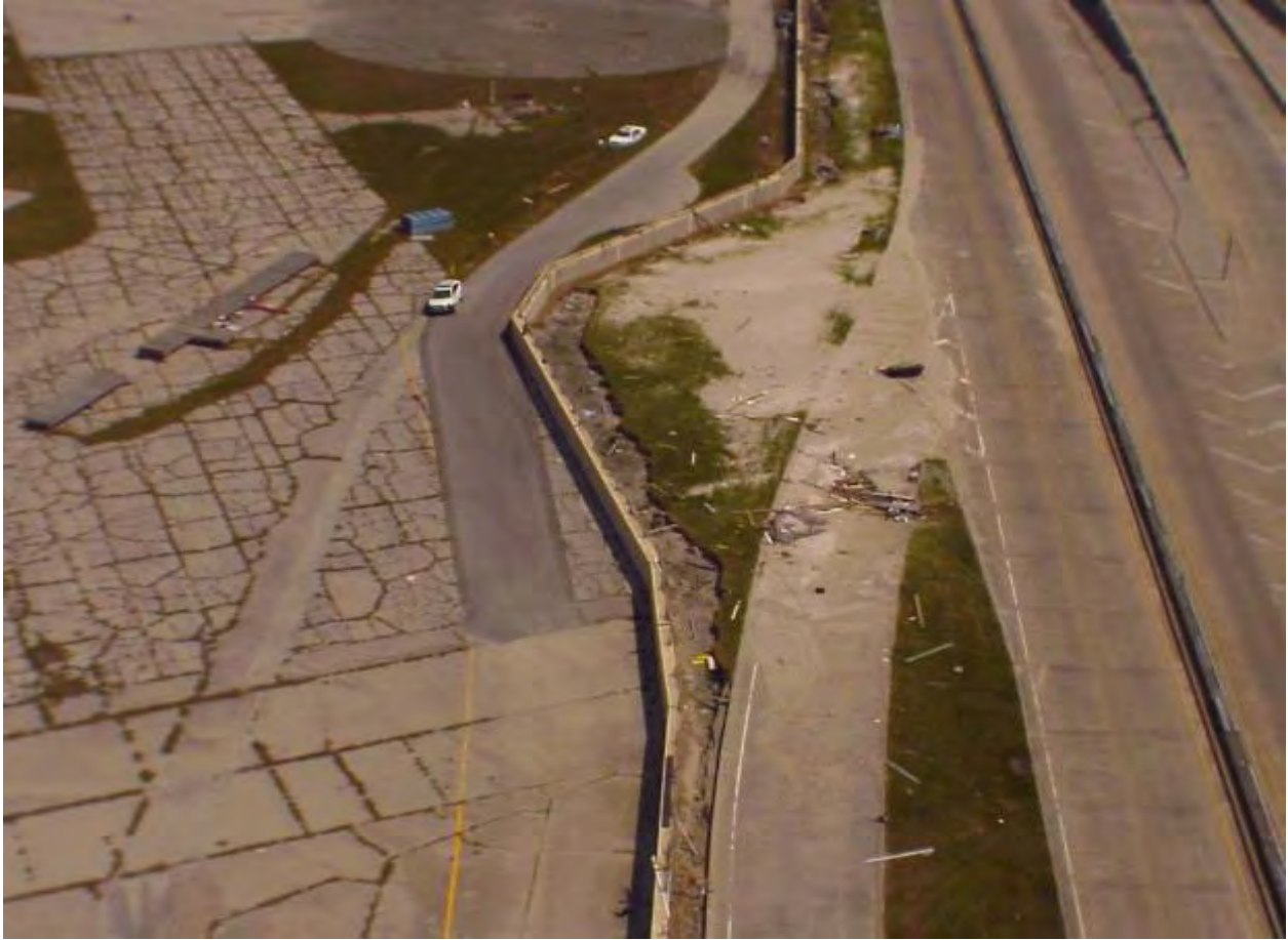
Figure 12-6. NOE6_B. Scoured Section on Protected Side at Lakefront Airport Floodwall
