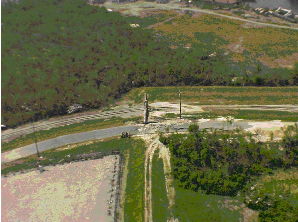
Figure 14-43. Scour at Railroad Gate Closure Structure E4 at Southernmost IHNC03 Project. 29 deg 59 min 48.76 sec N, 90 deg 01 min 11.6 sec W (Sta 176+75.9)
