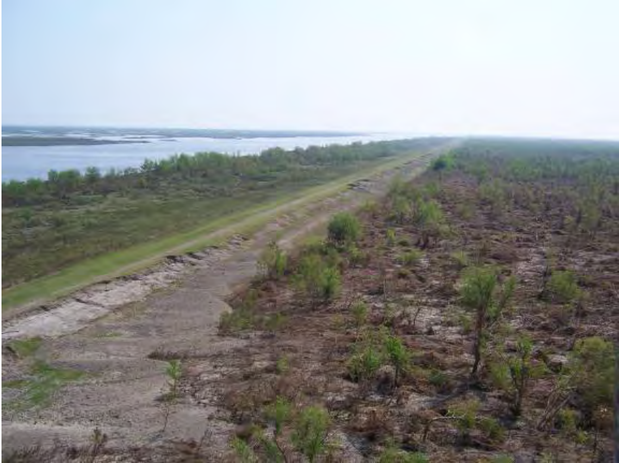
Figure 13-68. 2,500 ft. of Levee Along MRGO from Bayou Dupre to STA 1007+91 That Lost Approximately 8' of Elevation
