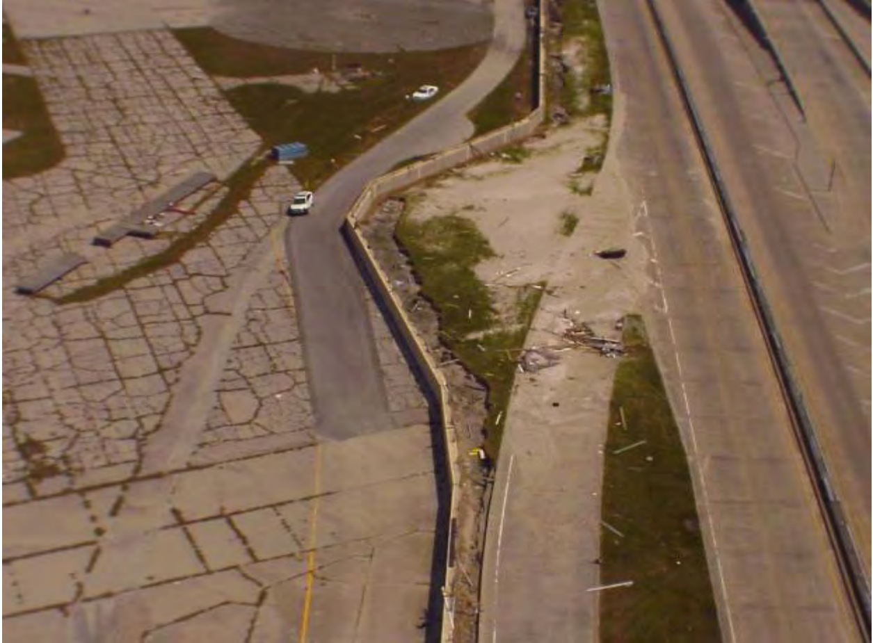
Figure 13-13. Lakefront Airport Floodwall. Scour is approximately 11 ft wide by 2 ft deep. Floodwall elevation is approximately 13.5 ft, ground elevation is approximately 6 ft, and wall height is approximately 7.5 ft
