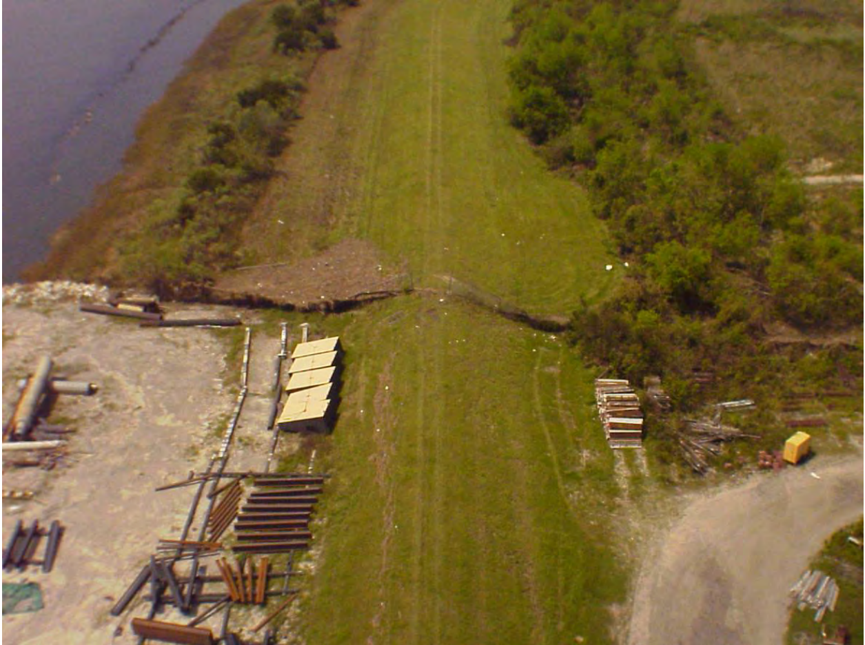
Figure 12-75. NOEX_V. Narrow Localized Breach at Pre-Existing Pipeline Crossing. Coords 30 deg 00 min 10.66 sec N, 89 deg 57 min 49.31 sec W (Approximate Sta 349+00 B/L)
