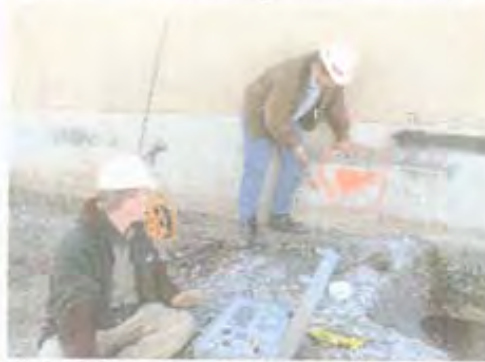
Photo 4 (Fig. 2) - Horizontal impact to side of concrete wall at el. 5 about 0.5 ft below chamfer
