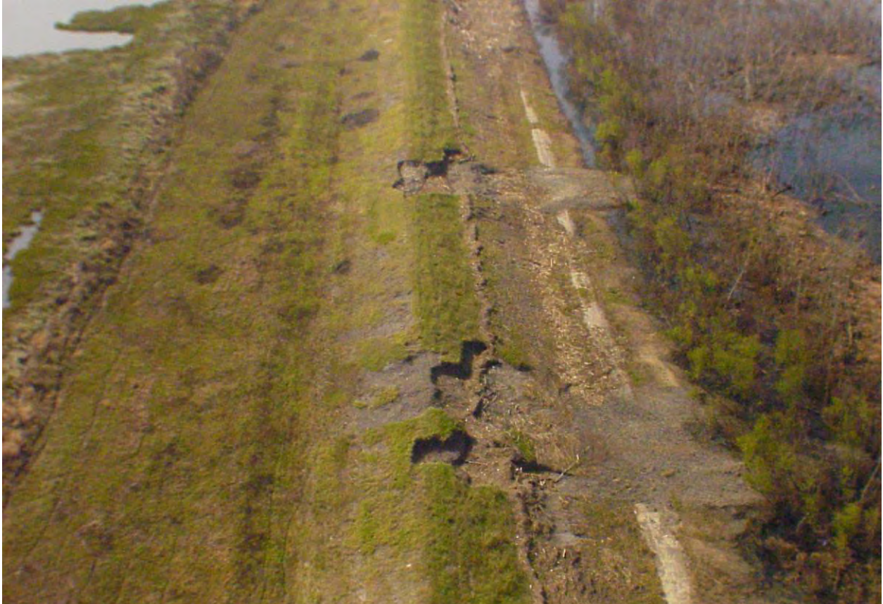
Figure 12-74. NOEX_U. Overtopping Erosion on Flood Side and Land Side
