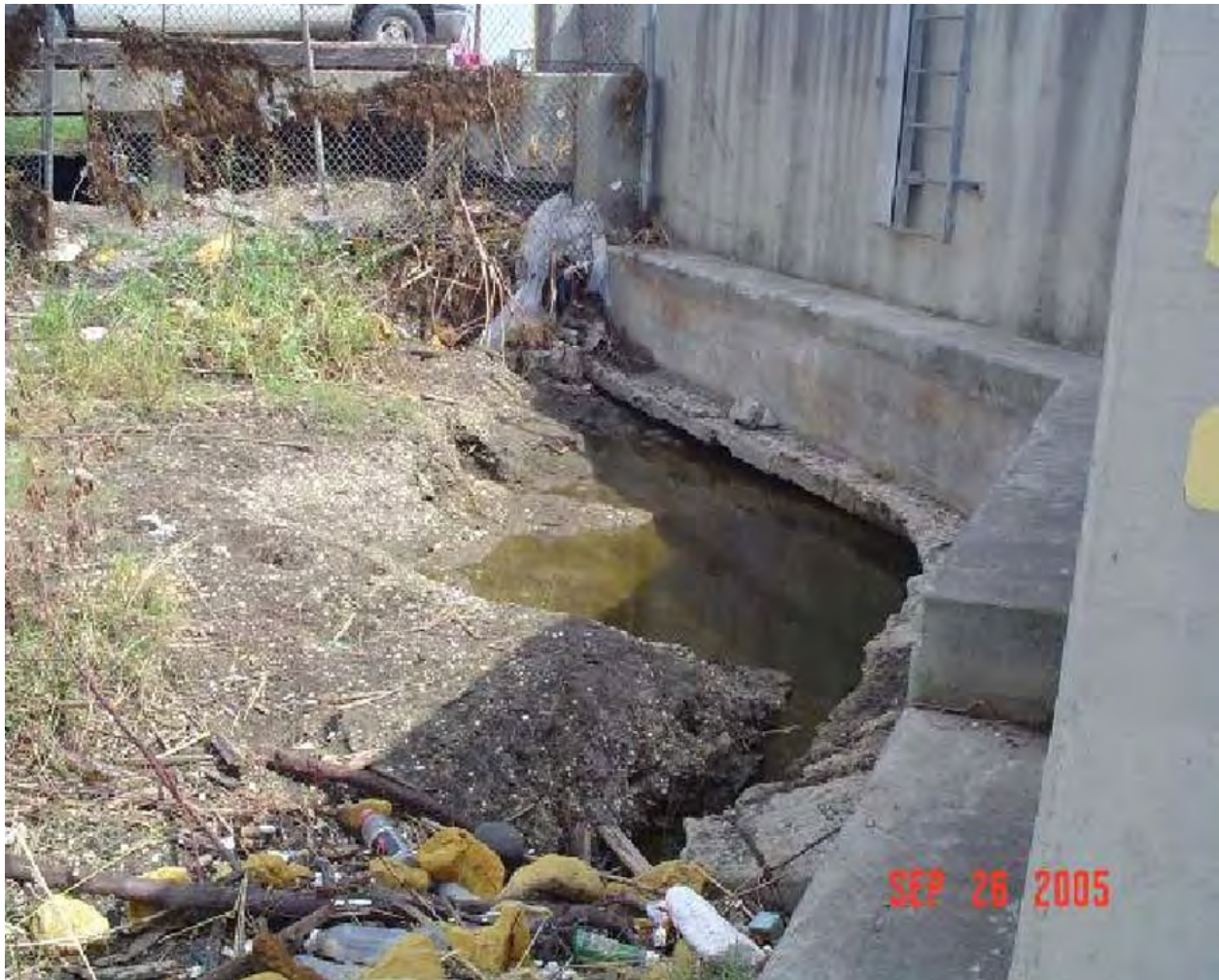
Figure 14-72. Scour at T-Wall Base of Gate W23
