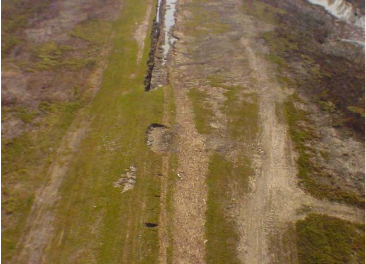
Figure 13-56. Crown Scour Along Approximate B/L Sta 1203+00 to Sta 1230+00, St. Bernard Levee Between MRGO and Miss. River. Crown was Approximate Elevation 15 ft
