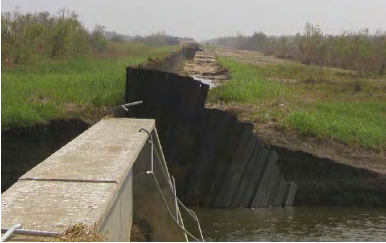
Figure 14-112. View Looking East of the Bayou Bienvenue Control Structure Showing Sheetpile Damage From Scour. From this picture there is no obvious layer stratification in the scoured section profile
