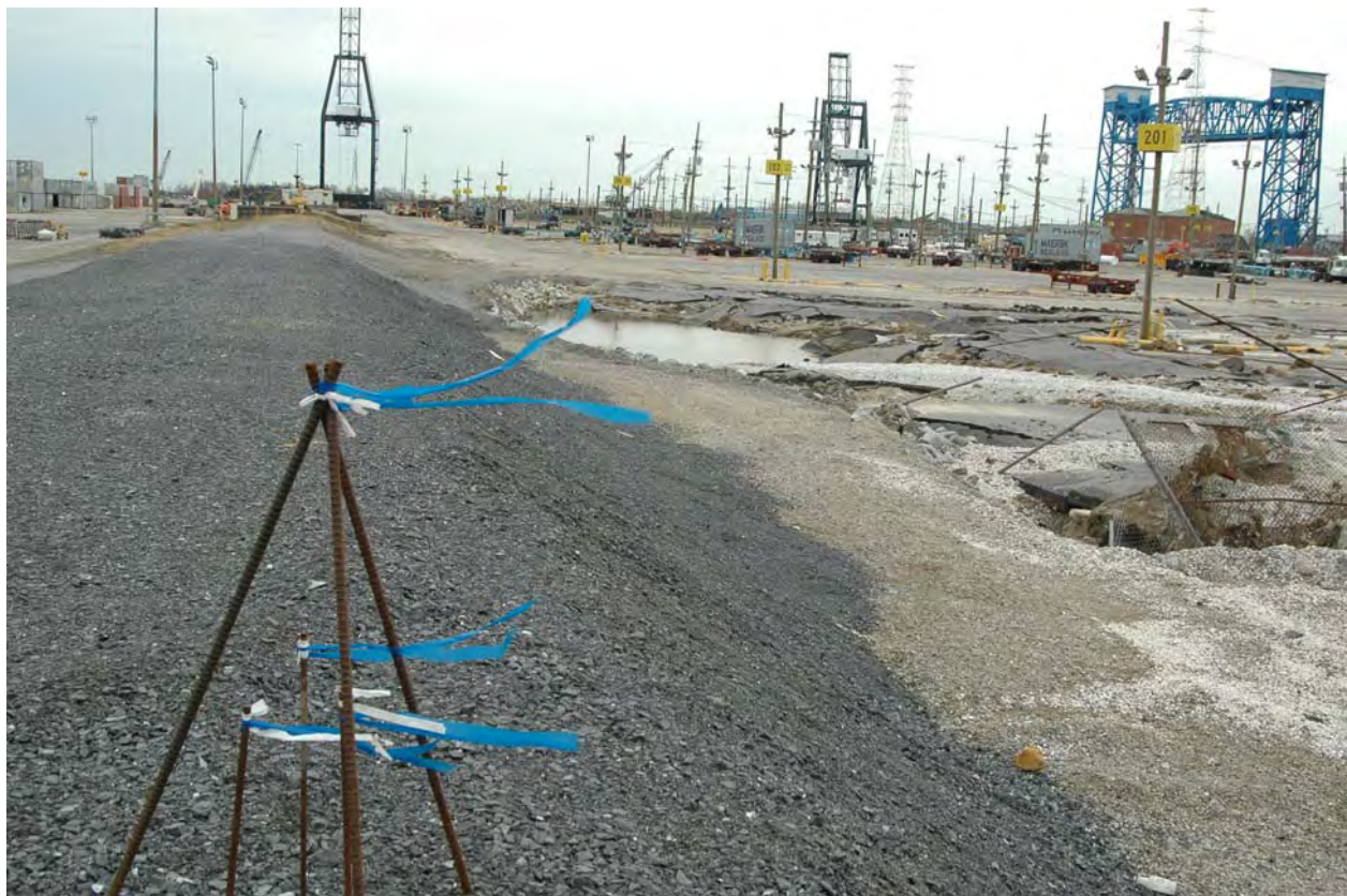
Figure 14-56. View West from France Rd. Ramp (approximate B/L Sta 212+00, C/L Sta 0+00). Remaining levee covered with fresh aggregate in preparation for new concrete wall construction
