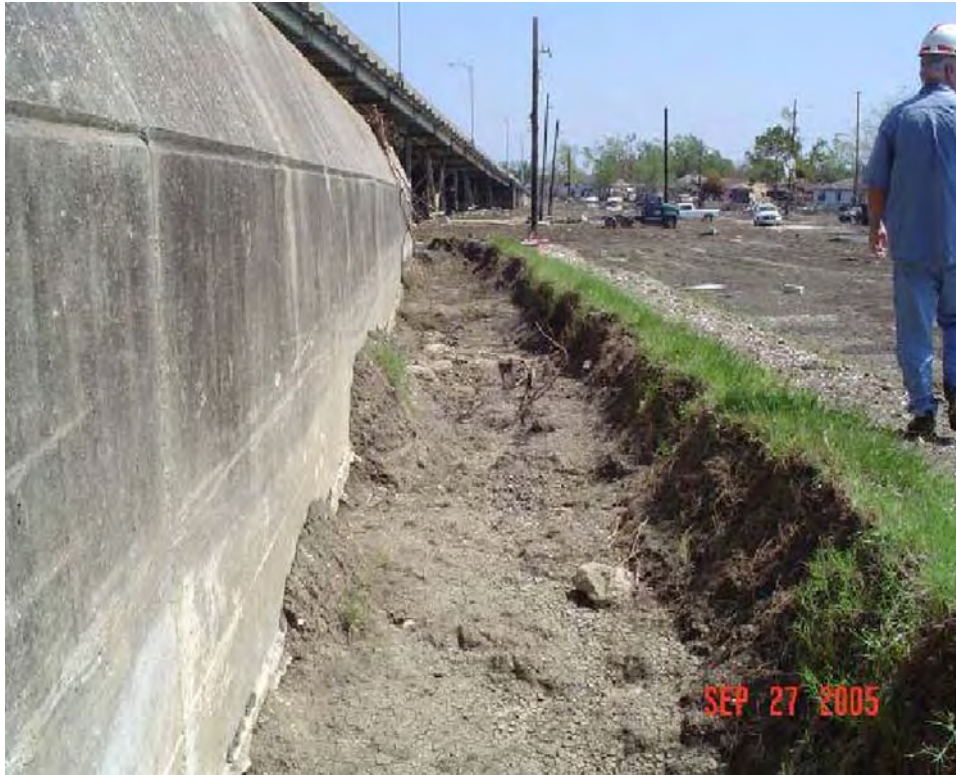
Figure 13-5. Scour Pattern "A" on East Side IHNC near N. Claiborne Ave. Bridge
