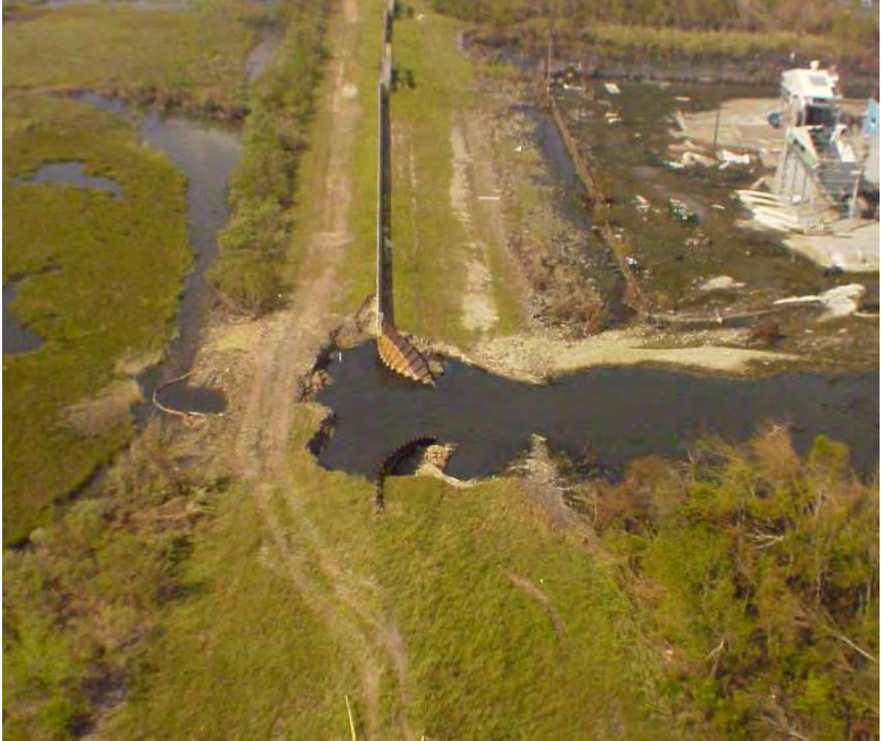
Figure 13-32. Air Products Sheetpile Breach
