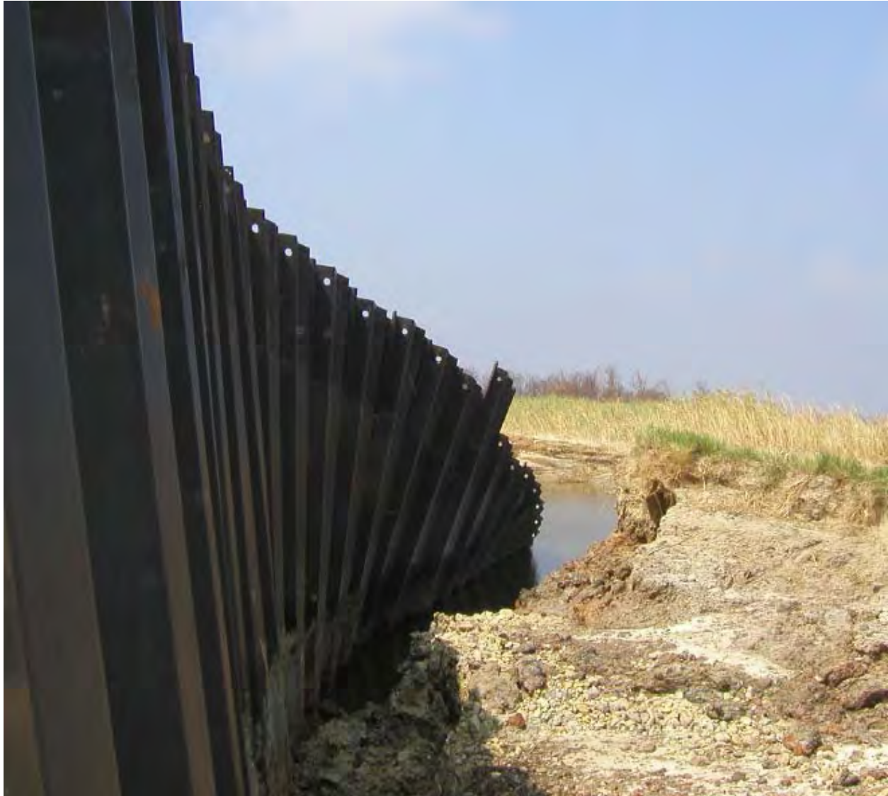
Figure 13-27. Closeup of Adjacent Breached Sheetpile with Backside Scour. Note the stratified layers in the soil profile representing existing hydraulic fill historically dredged from the MRGO
