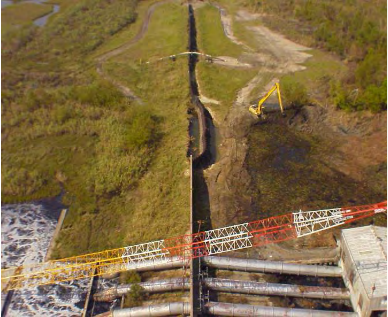
Figure 13-36. New Orleans East Basin, Pump Station 15 on the North Bank GIWW. Failed sheetpile between B/L Sta 874+40 and Sta 875+60 (N.O. East Back Levee). Pre-Katrina elevations ranged from 17.5 to 19.5 ft in this reach
