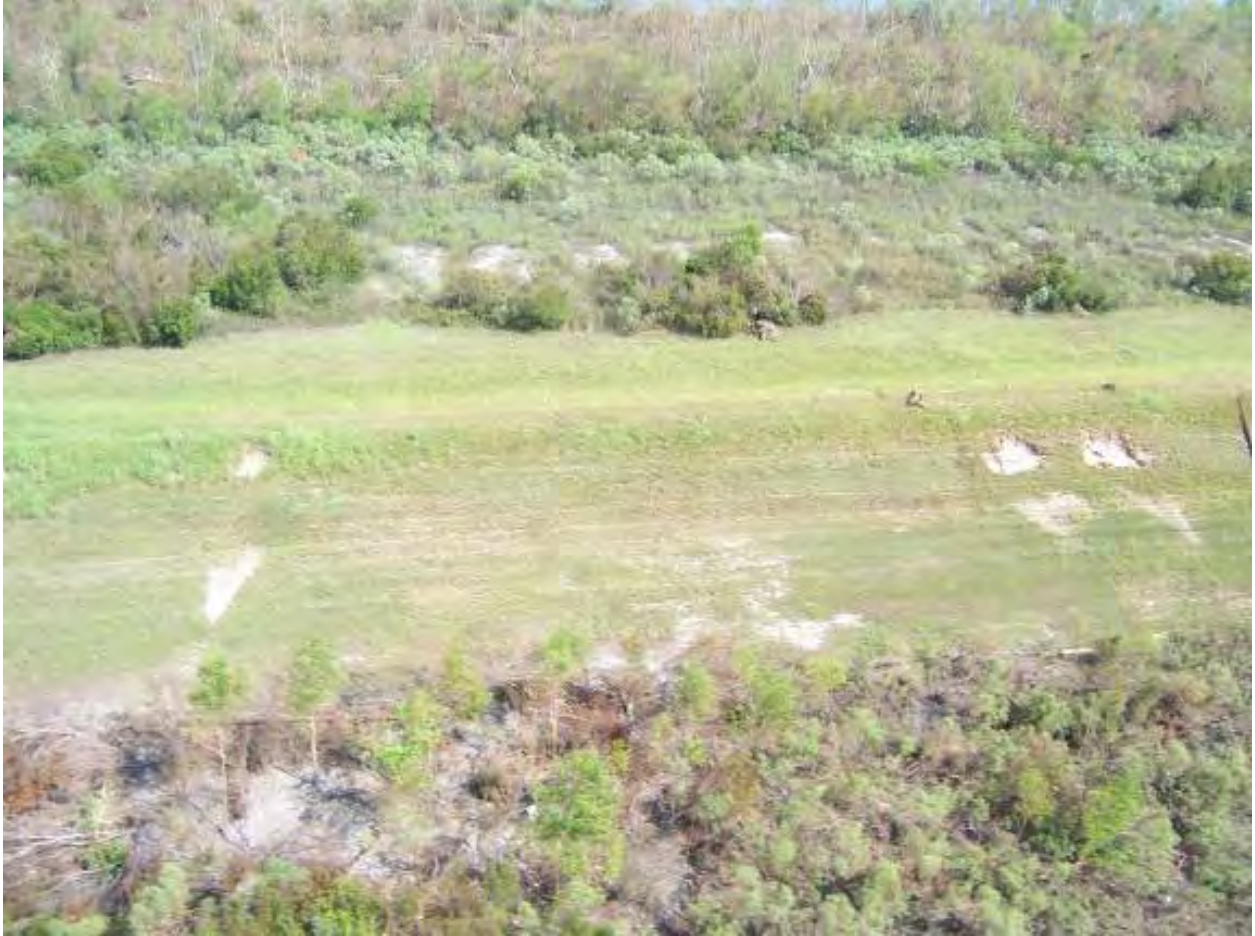
Figure 14-91. Localized Scour on the Levee South of the GIWW, Between IHNC and Paris Rd.
