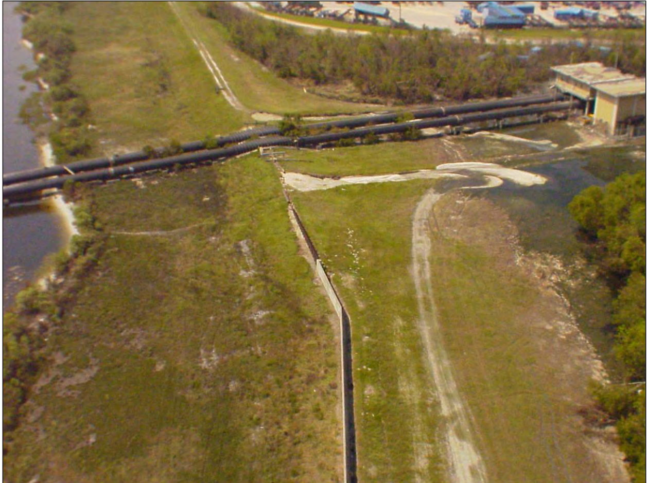
Figure 12-70. NOEX_Q. Amid Pump Station Landside Slope Erosion from Overtopping at Transition
