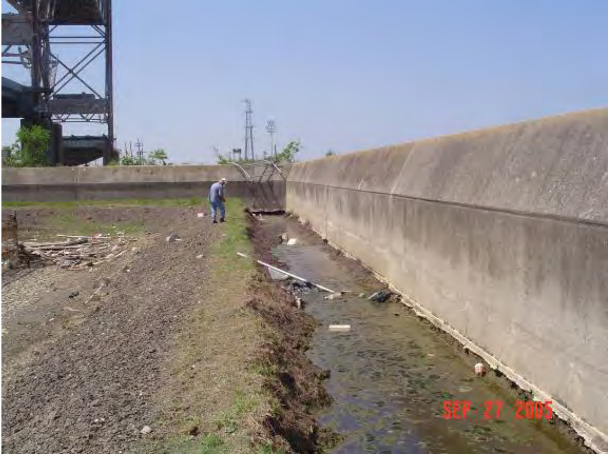
Figure 14-47. Approximate B/L Sta 7+00, View Toward Claiborne Ave. Bridge. Depth of scour was to the bottom of the I-wall concrete cap. Nearby soil boring 2U indicates the upper 5 ft was fat clay (CH) with sand / silt lenses
