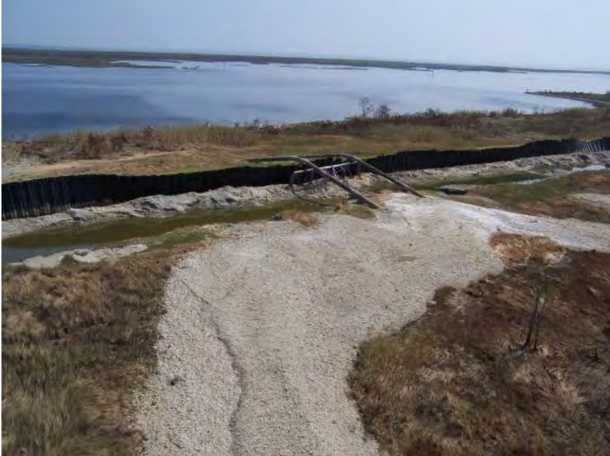
Figure 13-23. Pattern "A" Scour on the Backside of Exposed Sheetpile Wall Along the MRGO South Bank in St. Bernard Parish
