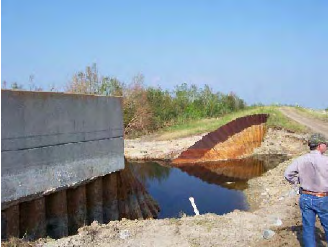
Figure 12-47. NOE3_G. West of Failure Looking East. Drawings from NOE3 Contract Solicitation Show Scour Depth And Outline
