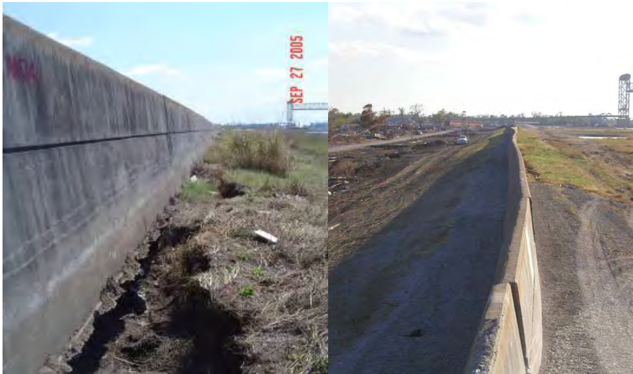
Figure 11-7. IHNC East Bank – North Breach – Wall Movement (View looking south)
