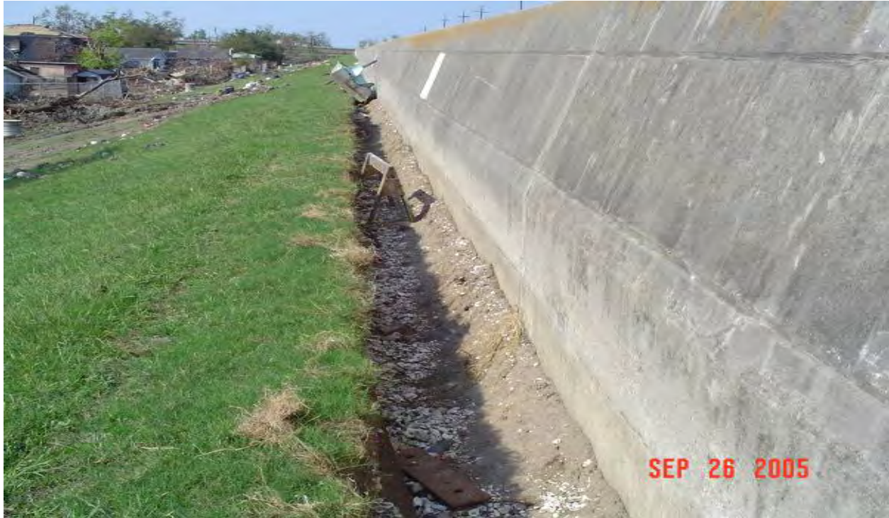
Figure 13-16. IHNC West Side Between Chef Menteur Hwy. and Hayne Blvd, Approx 8400 LF. Top of I-wall elevation is 14.75 ft(MSL), bottom of concrete is elevation 7 ft (MSL), and levee crown is elevation 8 ft (MSL). Borings in this reach (B/L Sta 31+06 to Sta 109+00, borings 1W to 14W) show the top 2 ft to 3 ft layer at crown elevation is composed of sandy and/or silty soil instead of fat clay
