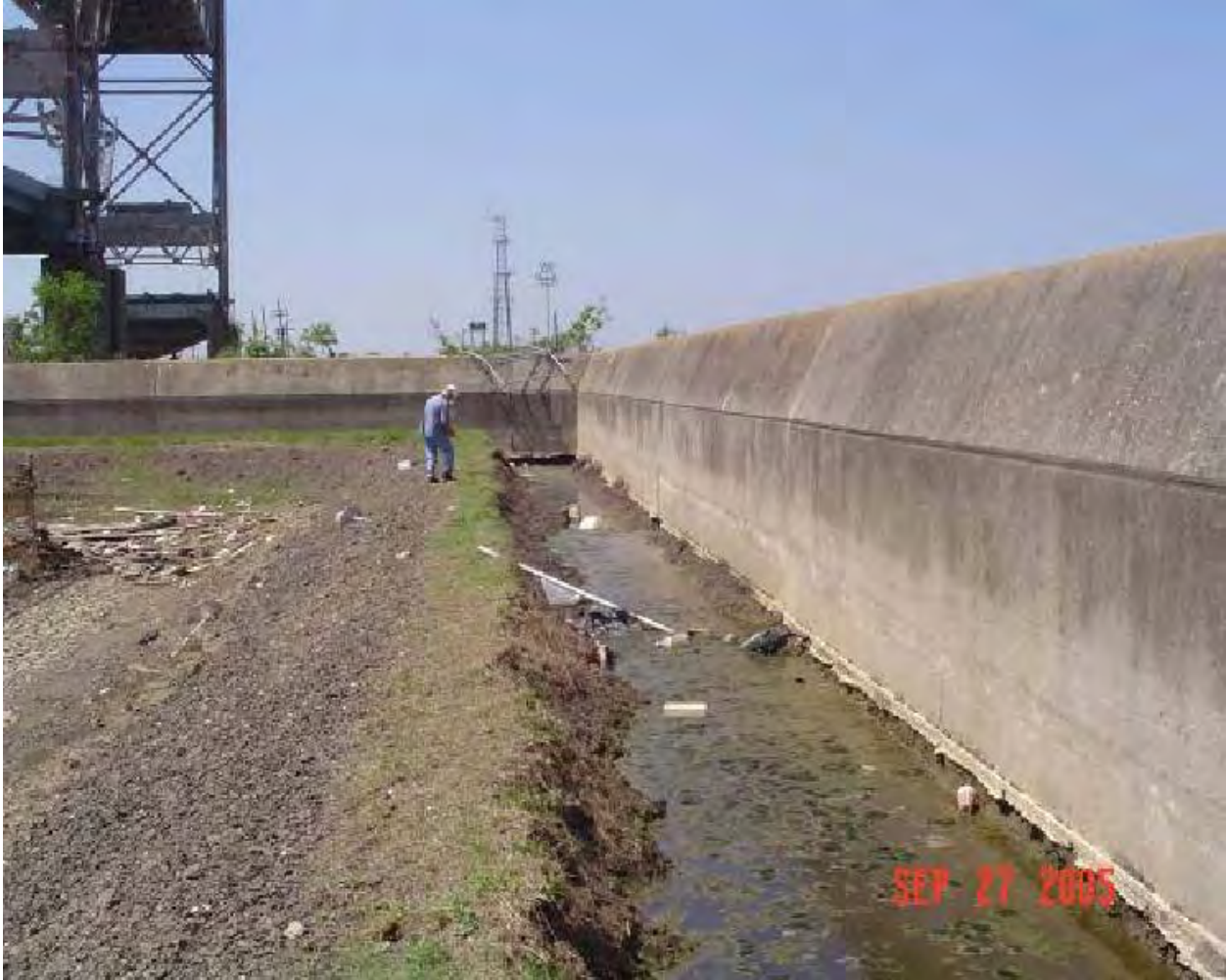
Figure 13-8. IHNC East, Approximate B/L Sta 7+00 (DM3 Chalmette Area Plan), North of the Claiborne Avenue Bridge. Depth of scour was to the bottom of the I-wall concrete cap. I-wall elevation was designed 15 ft above mean sea level (MSL), bottom of concrete was elevation 7 ft (MSL), and levee crown was elevation 9 ft (MSL). Actual wall height was reported to be 12.5 ft converted to local mean sea level (LMSL), and storm surge height was reported to be up to 15 ft. As an approximation of the overtopping water impact, a 2.5 ft crest of water cascaded from a 6-ft height onto the levee crown. Nearby soil boring 2U (Figure 13-9) indicates the upper 5 ft was fat clay (CH) with sand / silt lenses
