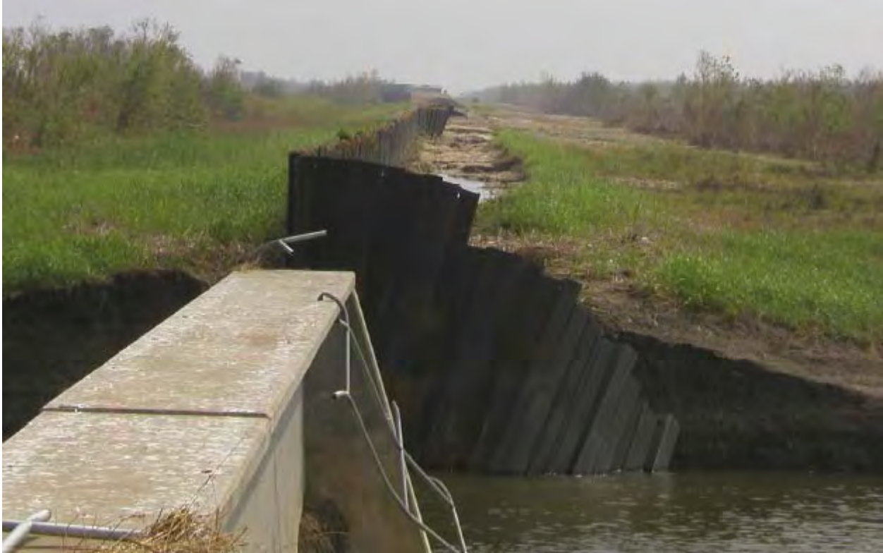
Figure 13-20. View Looking Southeast from the Bayou Bienvenue Control Structure Showing Backside Scour Beyond the Structure
