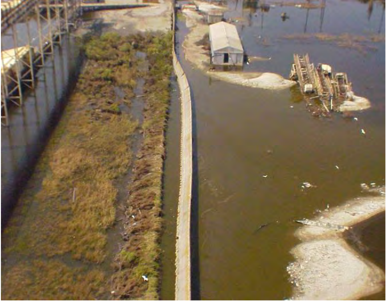
Figure 12-55. NOE4_B. Bulk Loading Terminal Facility I-Wall Failed by Rotation with Attendant Scour and Erosion (2000' near Elaine St. at GIWW), near Sta 271+55 B/L (Citrus Back Levee), Immediately Adjacent to the Tool Shed Metal Building
