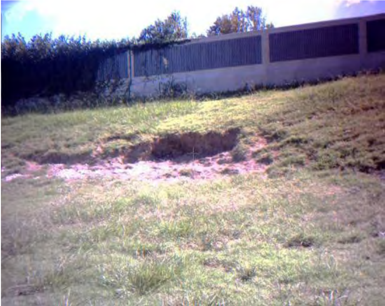
Figure 13-52. New Orleans East Bank Lake Pontchartrain Floodwall Scour, 20ft long x 10ft wide x 2ft deep. GPS coords N90 deg 05min 17.3 sec, W30deg 01 min 39.3 sec
