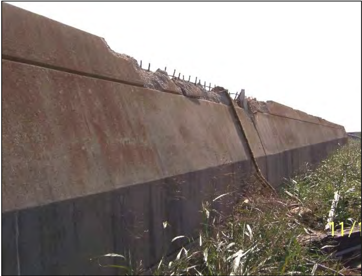
Figure 12-53. NOE9_C. I-Wall Damage Likely Due to Impact
