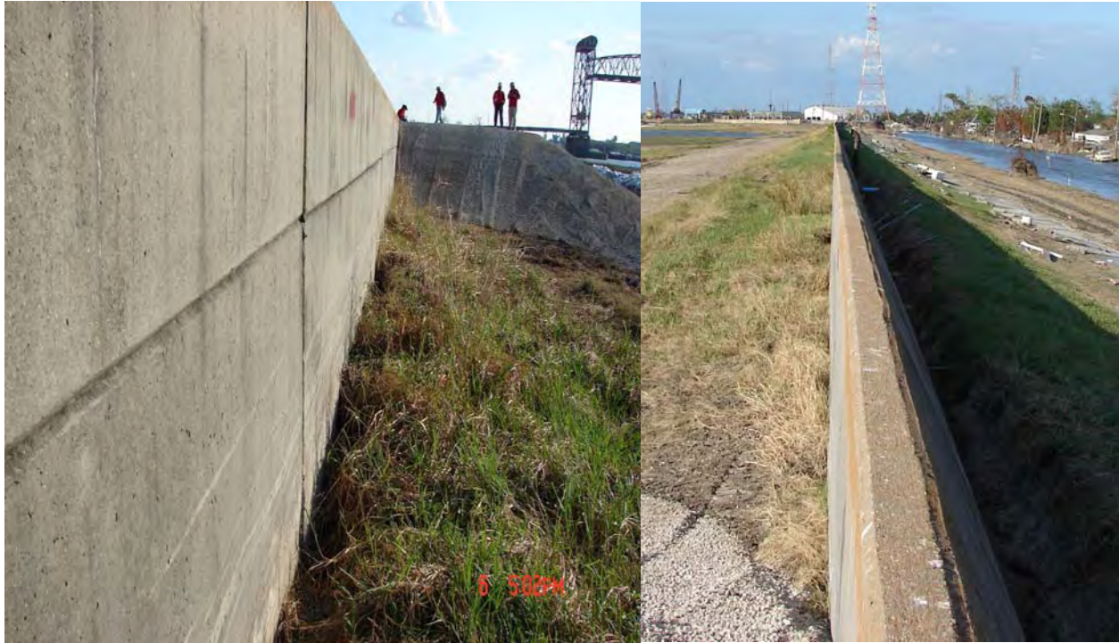
Figure 11-6. IHNC East Bank – South Breach – Wall Movement
