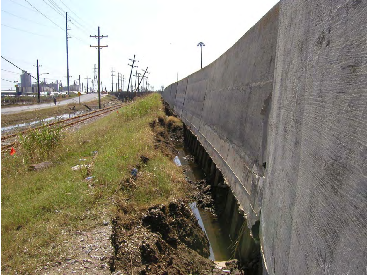
Figure 14-60. View South From Benefit St. Gate Toward France Rd Ramp. Approximate W/L Sta 5+56 (B/L Sta 205+44). Top of I-wall elevation 15 ft, levee crown 9 ft, bottom of concrete 7 ft, bottom of pre-existing Z-27 sheet pile (by Orleans Levee Board) at -10ft (MSL). From drawing file H-2-24111, plate IV-15. Nearest soil boring is 30W at B/L Sta 203+00
