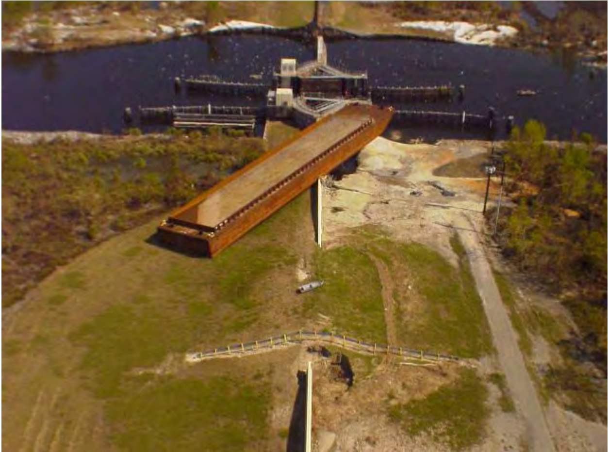
Figure 14-109. Post-Katrina. Note scour near guardrail shown in Figure 14-104
