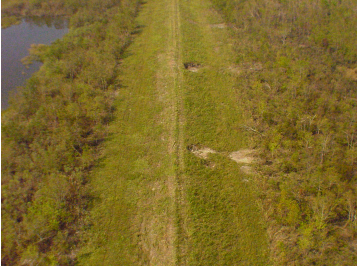
Figure 13-42. Backside Levee Erosion Pattern “B” on the Citrus Back Levee, N.O. East
