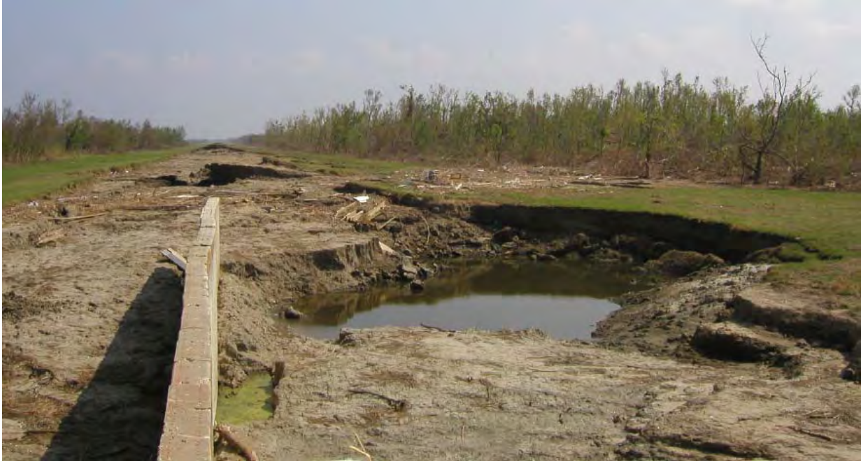
Figure 14-142. Closeup of East View, End of Concrete Wall, Showing Major Scour Holes and Complete Erosion of Levee
