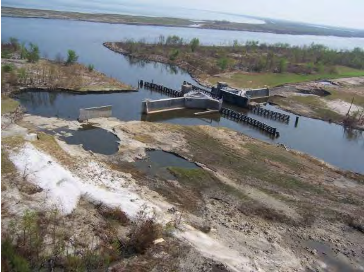
Figure 14-139. Bayou Dupre Control Structure, Post-Katrina. View toward MRGO. Note the missing levees on both sides of the structure
