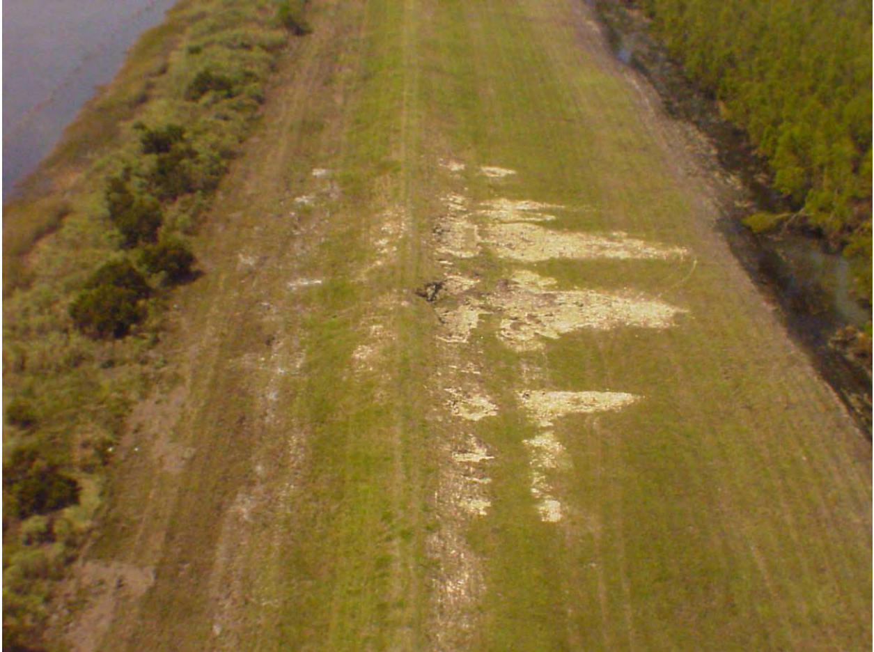
Figure 12-76. NOEX_W. 600' Reach of Levee with Landside Scouring
