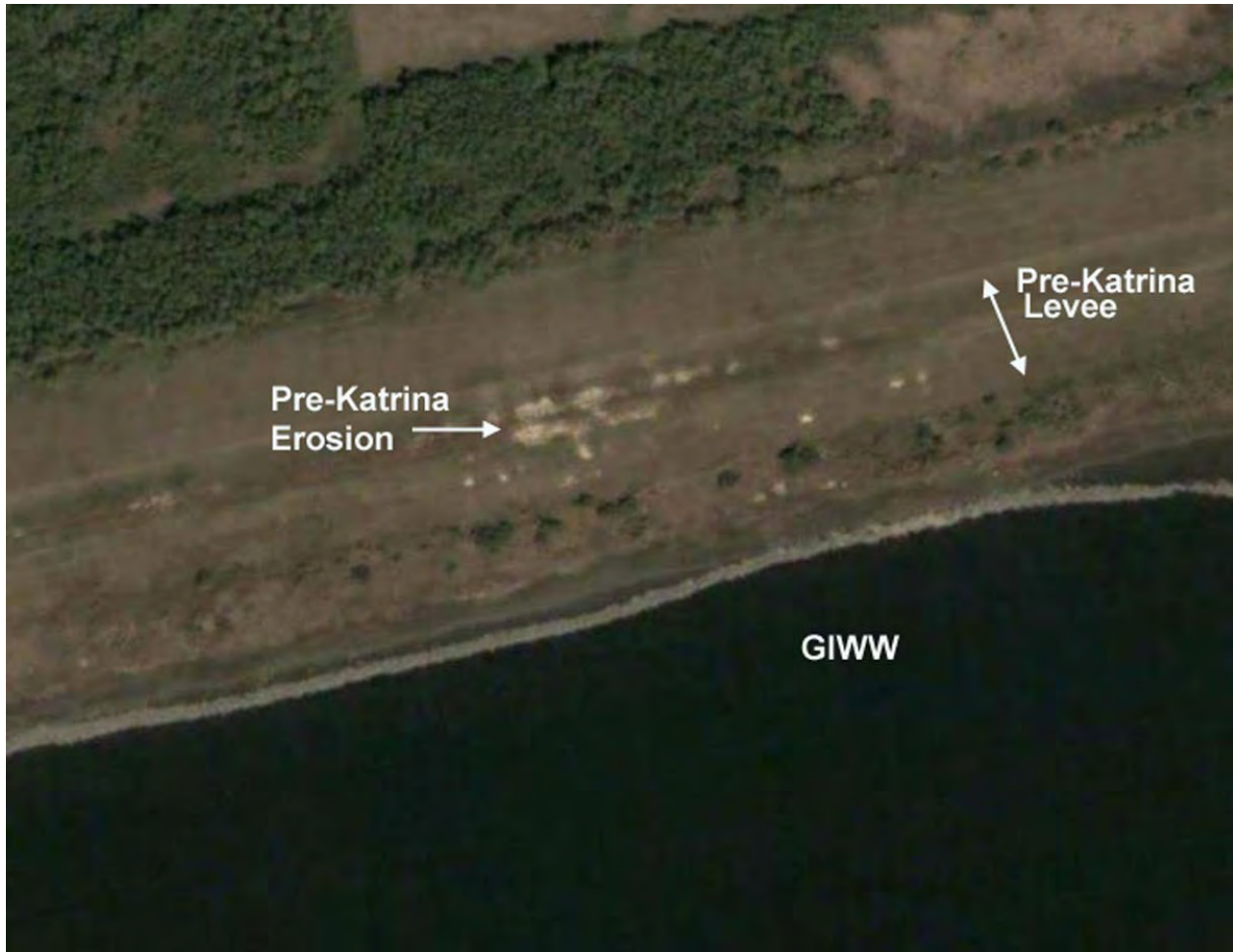
Figure 13-45. Possible Pre-Existing Surface Erosion on Levee Slopes Along the North Bank of the GIWW (Citrus Back Levee) at N 30deg 0 min 7 sec W 89deg 58min 31 sec. (pre-Katrina image from GoogleEarth website). Possible erosion is evidenced by vegetation distress and bare spots along the levee
