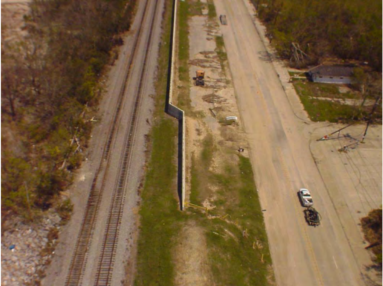
Figure 12-11. NOE7_C Floodwall Landside Scouring on Hayne Blvd. East of Downman Rd.
