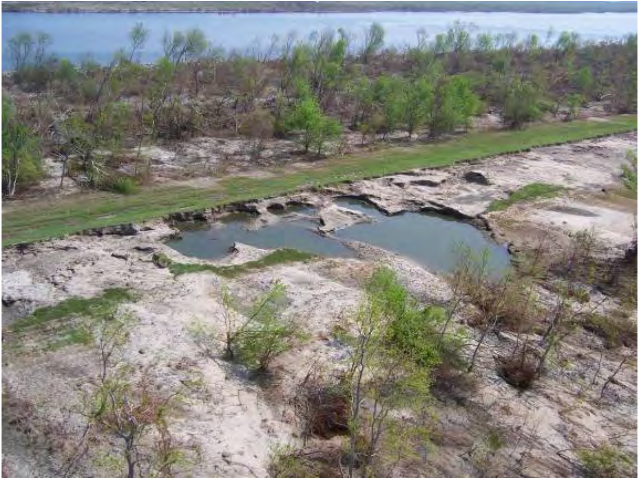
Figure 14-144. Major Scour on Levee Protected Side (Landside)
