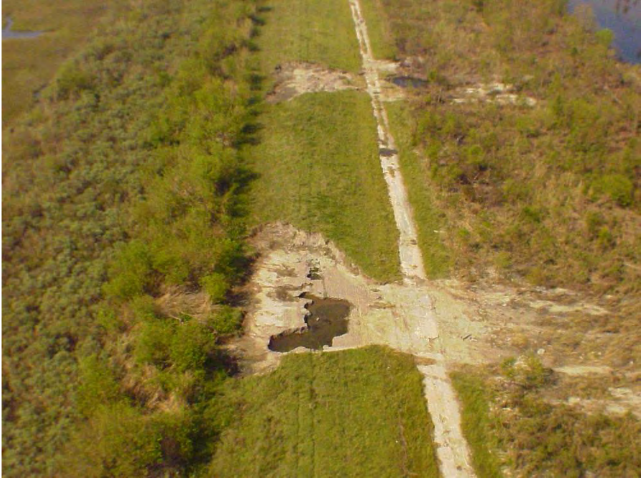
Figure 12-38. NOE1_E Partial Breach East of Pump Station 15
