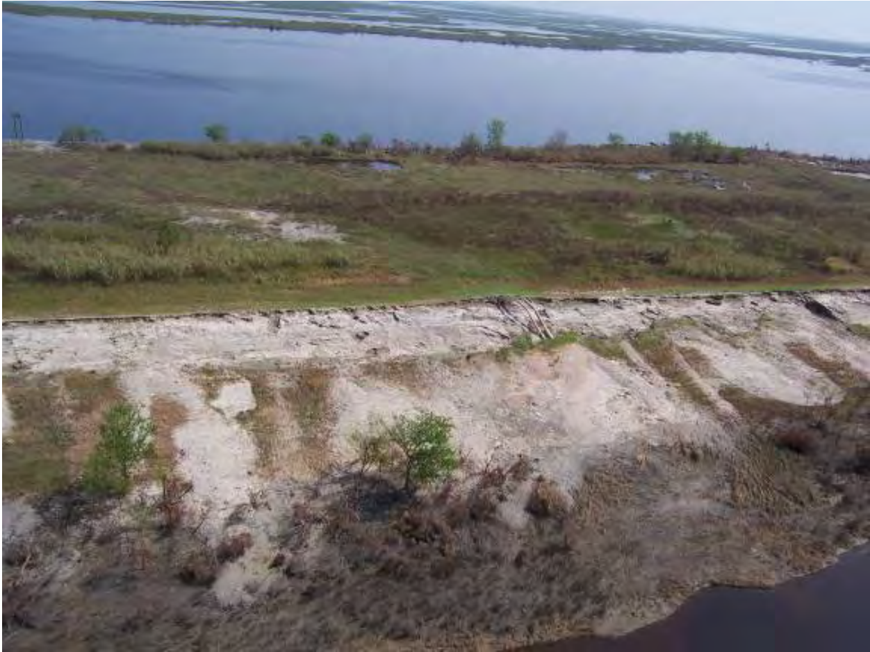
Figure 13-63. 19,000 ft. of Levee Between Bayou Bienvenue (Sta 383+00) and Bayou Dupre (Sta 704+00) Lost Approximately 12' of Levee Height From Original (design) Height 17.5 ft. Pre-Katrina elevation was approximately 12 ft, and storm surge along the MRGO was approximately 18 ft, causing an overtopping crest of up to 6 ft
