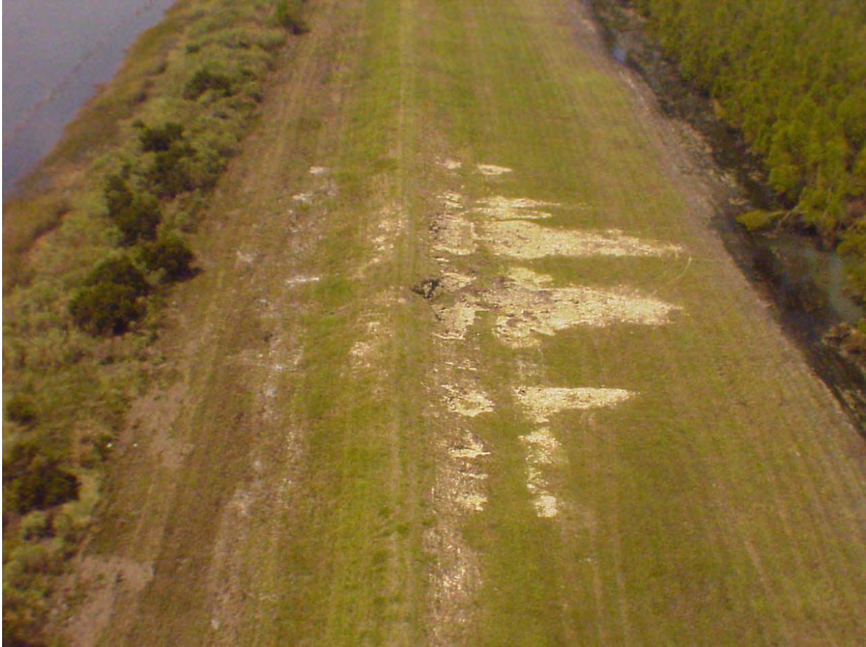
Figure 13-43. 600' Reach of Levee Along the North Bank of the GIWW (Citrus Back Levee, New Orleans East) Between Elaine Pump Station and Paris Road
