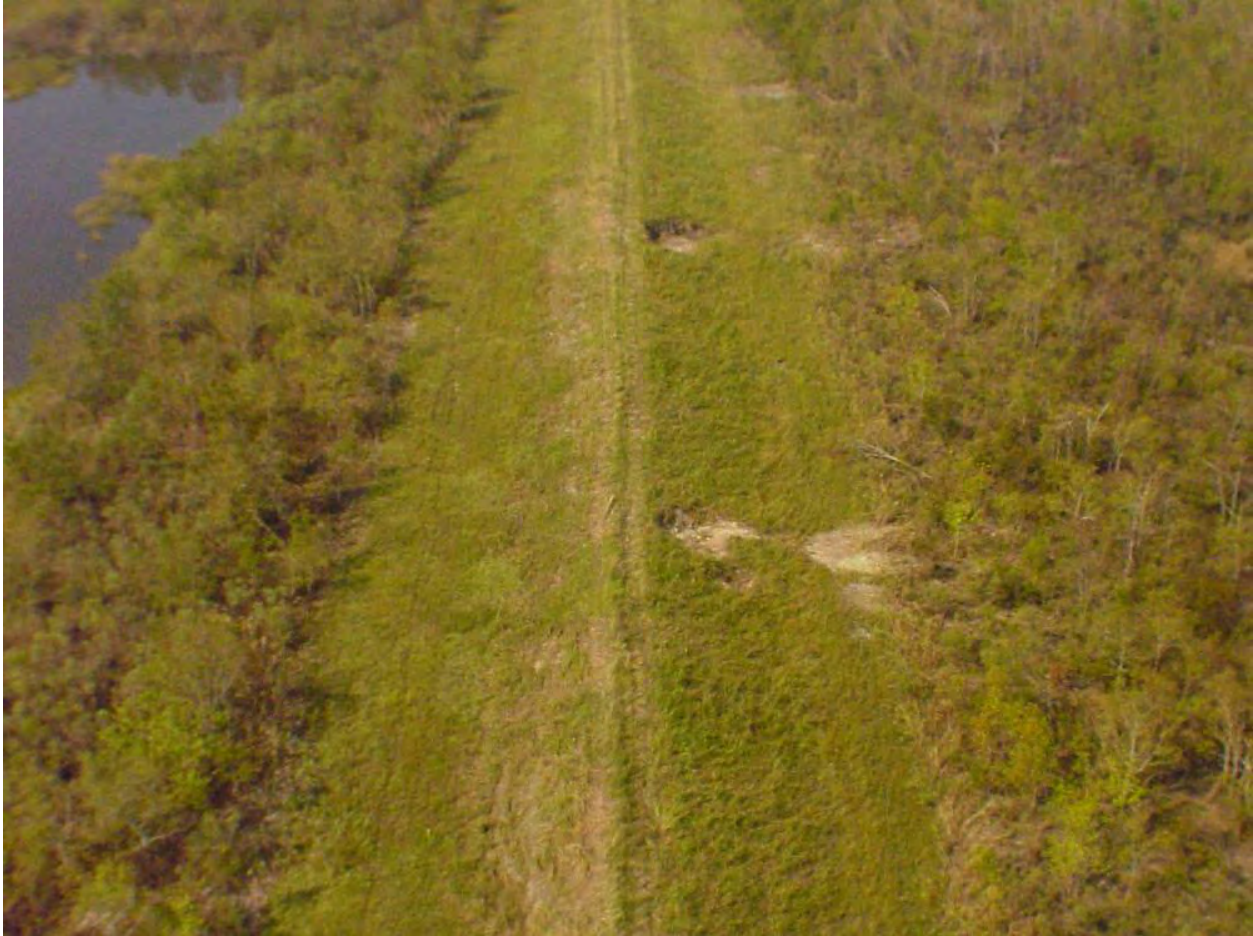
Figure 12-40. NOE1_G Localized Scour Typical of Several Locations
