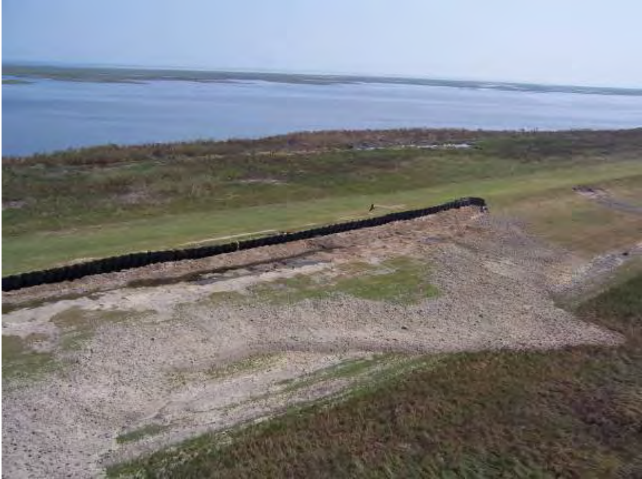
Figure 13-76. End of Sheetpile Wall at B/L Sta 980+58, Along the MRGO (St. Bernard Parish). Note that scour occurred along the sheetpile wall and minimally beyond the levee transition. Approximate sheetpile elevation was 17 ft and levee crown elevation was 13 ft. Beyond the transition, the levee crown elevation was approximately 17 ft. The approximate storm surge overtopping crest was 4 ft over the sheetpile and 1 ft over the transition levee
