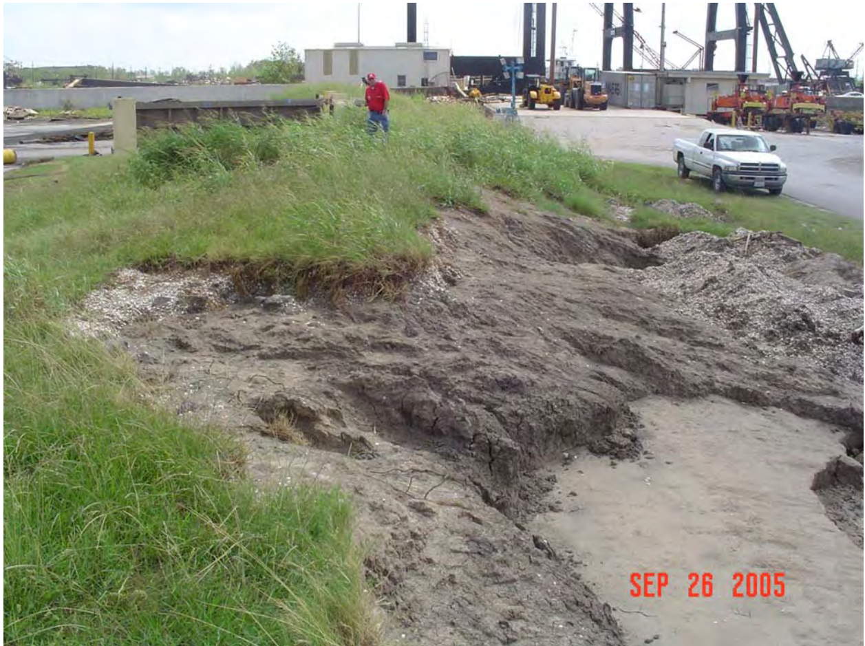
Figure 13-53. Eroded Levee Crown on the IHNC West Side at Container Facility
