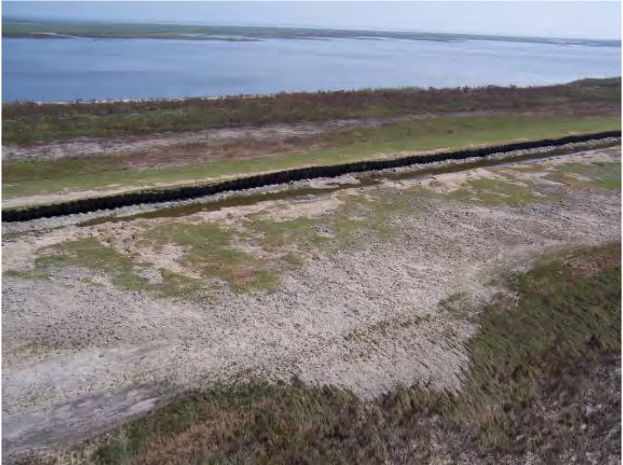
Figure 14-150. Scour on Protected Side of Sheetpile Wall
