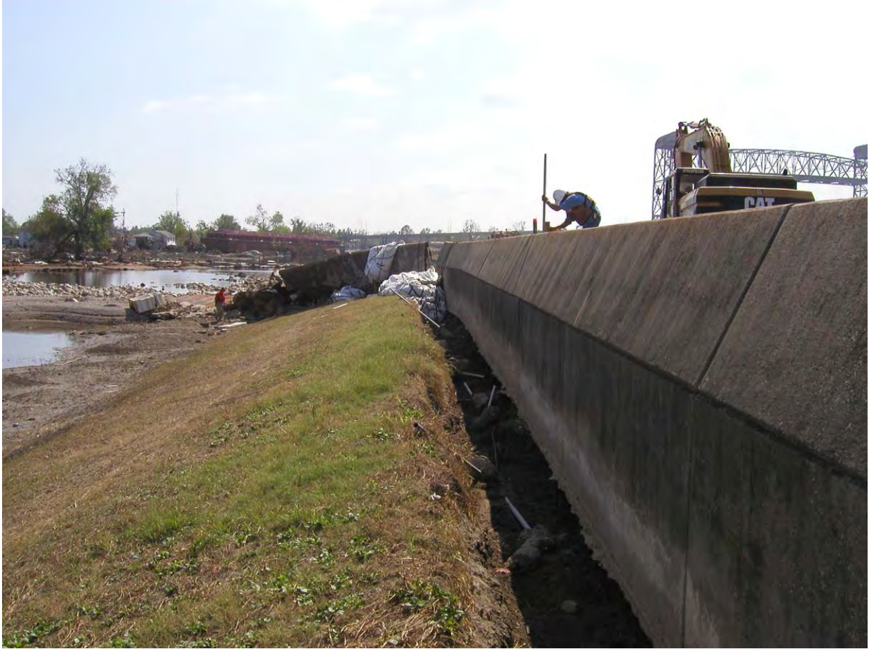
Figure 14-26. Northernmost Transition From Failed Wall to Intact Wall
