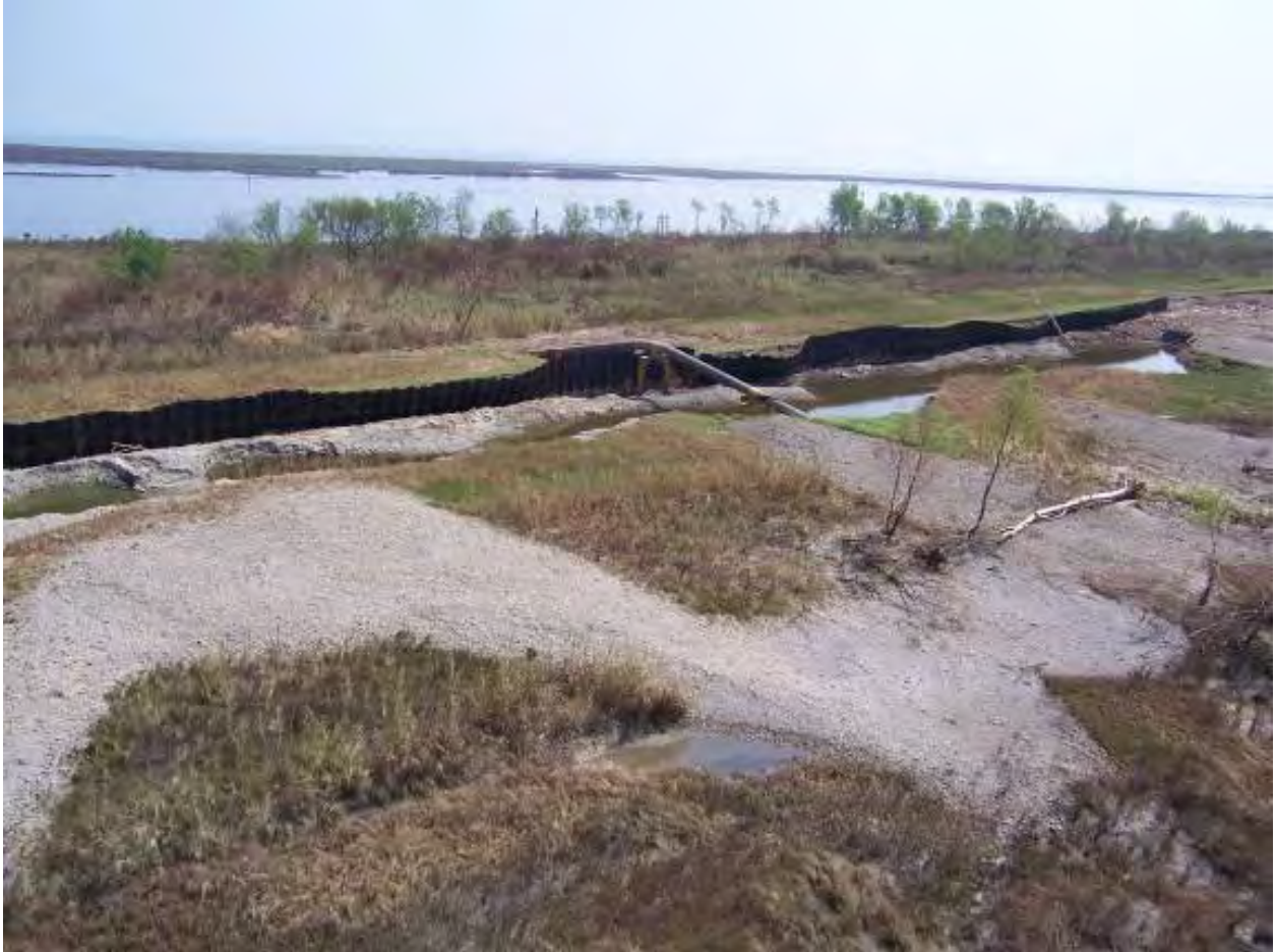
Figure 14-124. Additional Damaged Sheetpile at Utility Crossing, B/L Sta 600+00
