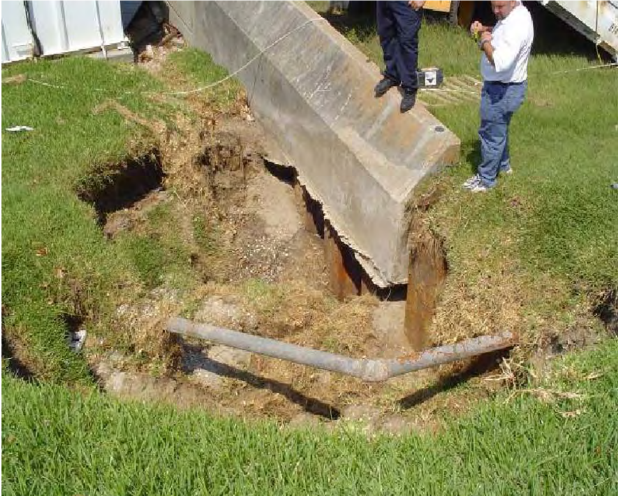
Figure 14-46. Scour at I-Wall / Levee Transition at IHNC Lock
