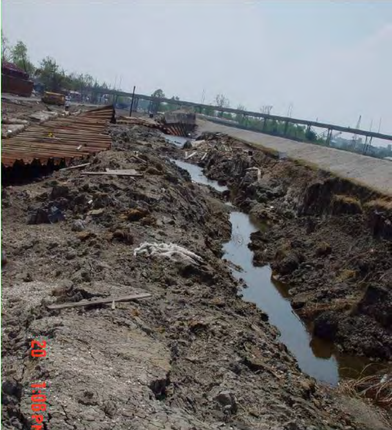
Figure 11-5. Scour and Erosion Leading to the Failure of the I-Wall on the IHNC Adjacent the South Breach (9th Ward)
