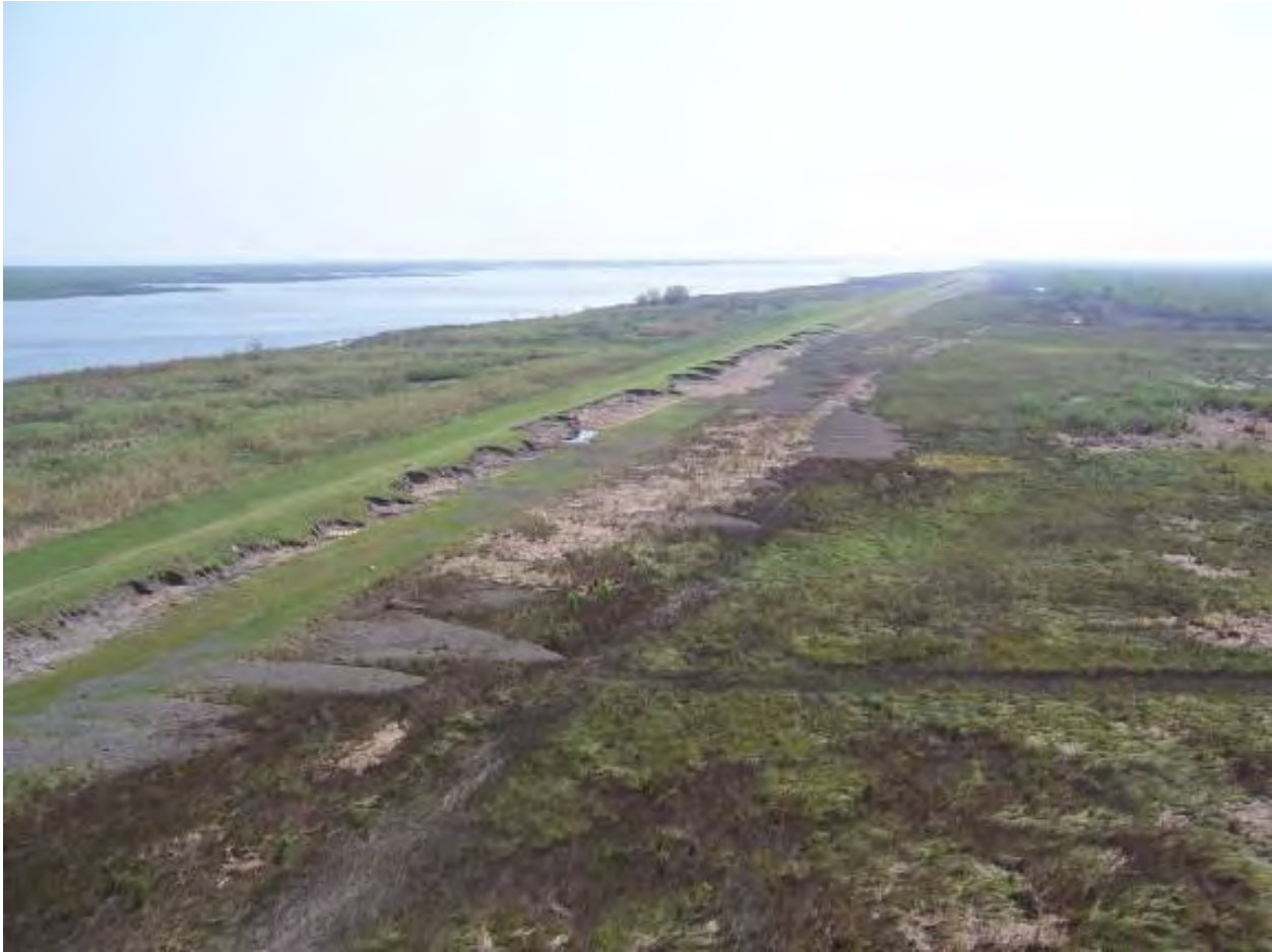
Figure 14-147. Major Scour on Protected Side of Levee
