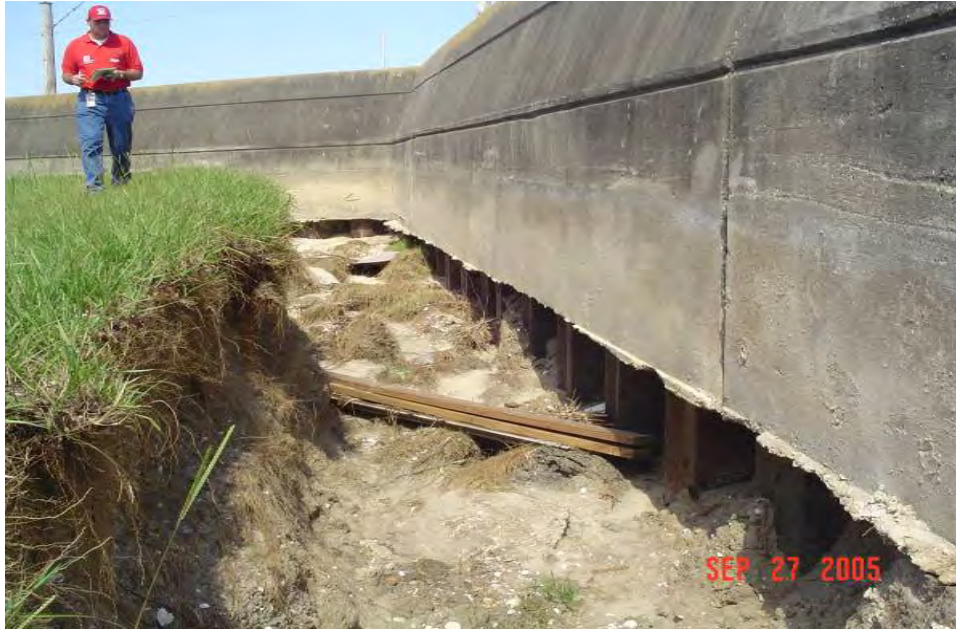
Figure 13-14. IHNC East, Approximate B/L Sta 101+00 (from drawing file H-2-24111, plate IV-23, DM2 Supp 8 IHNC Remaining Levees), North of Chef Menteur Hwy Bridge. Top of I-wall is elev 14.75, bottom of concrete is elev 7, and levee crown is elev 9. Nearest B/L boring is Sta 96+00 (No. 9EU), 500 feet distant. Approximate storm surge impact was a 2.5-ft water crest cascading over the 6-ft concrete wall. Note that the scour was deeper than the concrete base, indicating that the structural backfill and the original levee material eroded
