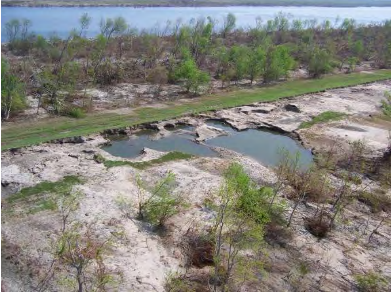
Figure 13-66. 8,000 ft. Section of the Levee Immediately Southeast of Bayou Dupre (St. Bernard Parish) That Was Severely Damaged and Not Only Lost Approximately 12 feet of Levee Height But Also Part of the Original Levee Foundation
