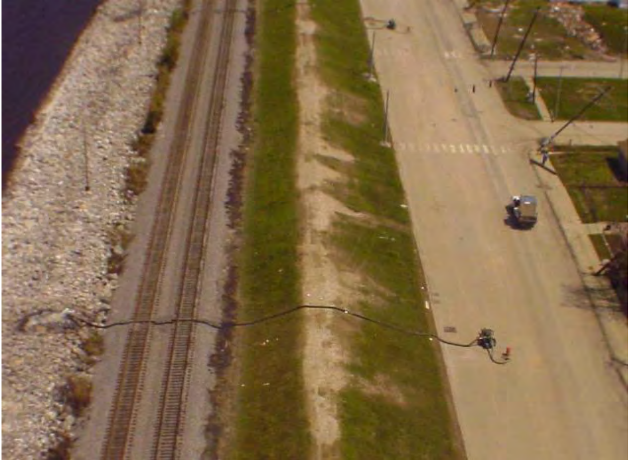
Figure 12-10. NOE7_B Typical Crown and Landside Scouring
