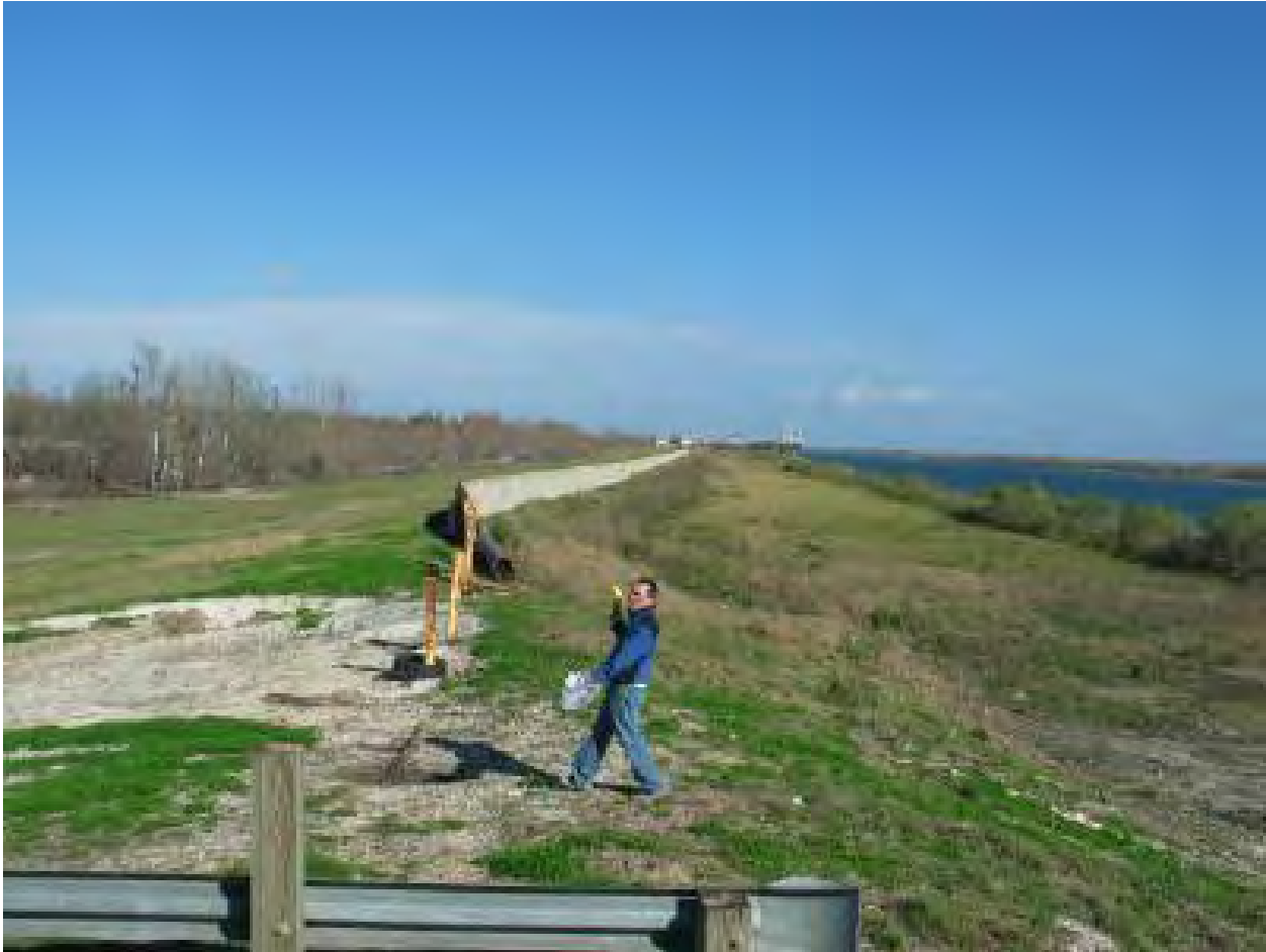
Figure 12-73. NOEX_T. Closeup of Scoured Road at Levee Crown, Amid Pump Station
