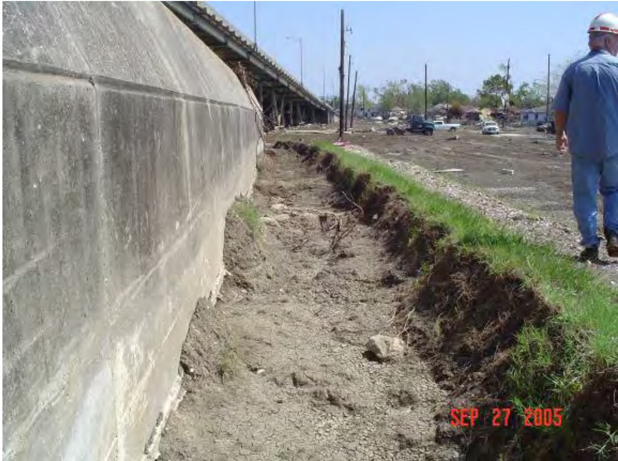
Figure 14-49. East Side IHNC Near N. Claiborne Ave, Approximate B/L Sta 11+00. I-wall elevation designed 15 ft (MSL), bottom of concrete elevation 7 ft (MSL), and levee crown elevation 9 ft (MSL). Nearest soil boring, No. 3, shows fat clay (CH) at surface
