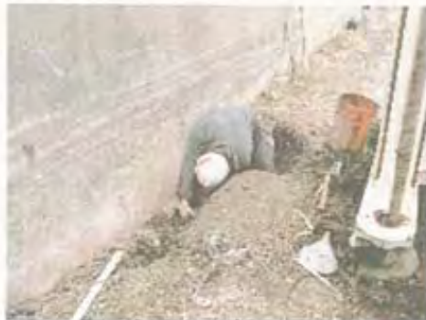
Photo 9 - IHNC 3-lb Impulse hammer impacts to sheet pile on canal side at Station 17+11
