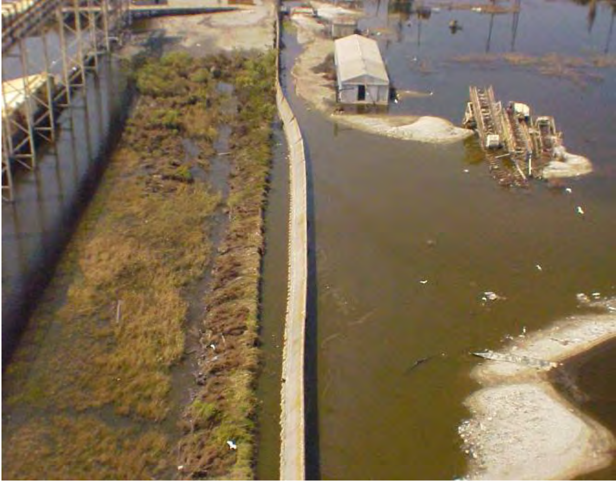
Figure 13-34. Bulk Loading Facility I-Wall Breach (2000' near Elaine St. at GIWW, near Sta 271+55 B/L, Citrus Back Levee, north bank GIWW). Scour depths were 6 to 10 ft on both floodside and protected side of the I-wall. Pre-existing wall elevation was approximately 15 ft (MSL), and levee elevation was approximately 9 ft (MSL), for an exposed wall height of approximately 6 ft. Storm surge ranged from elevation 15 to 17 ft
