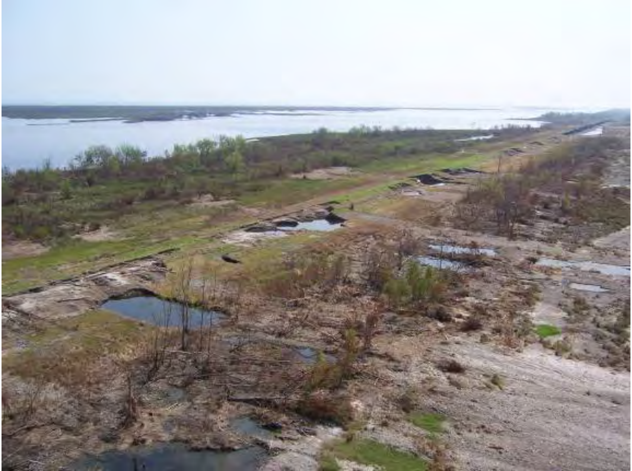
Figure 14-118. Partial Levee Eroded
