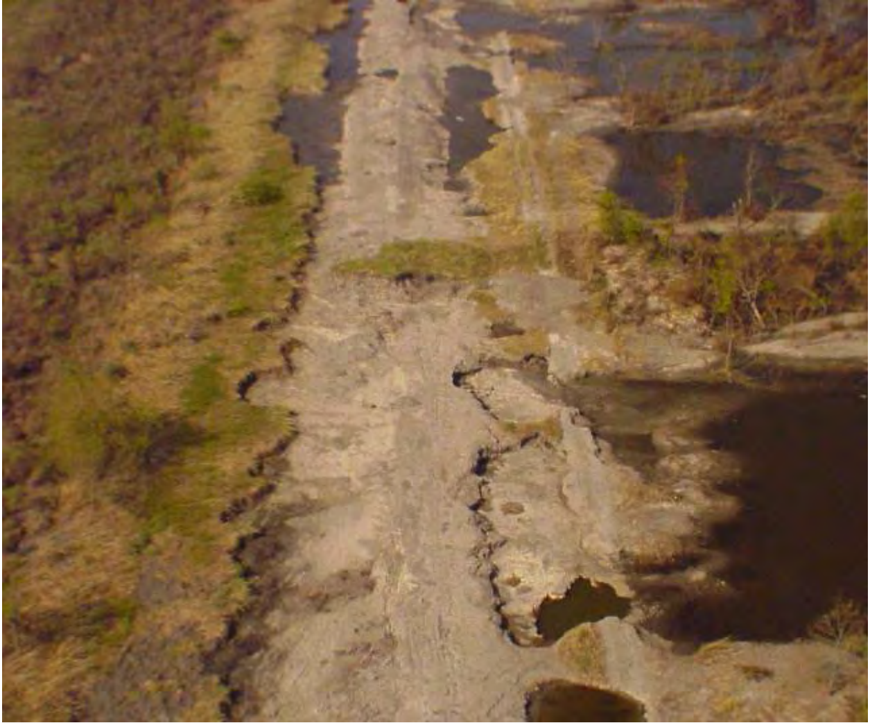
Figure 12-36. NOE1_C Complete Breach East of Pump Station 15
