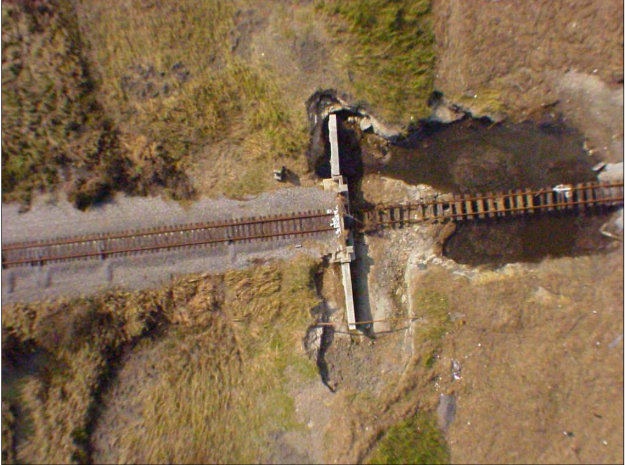
Figure 12-19. NOE5_C. View of Scour Around T-Wall
