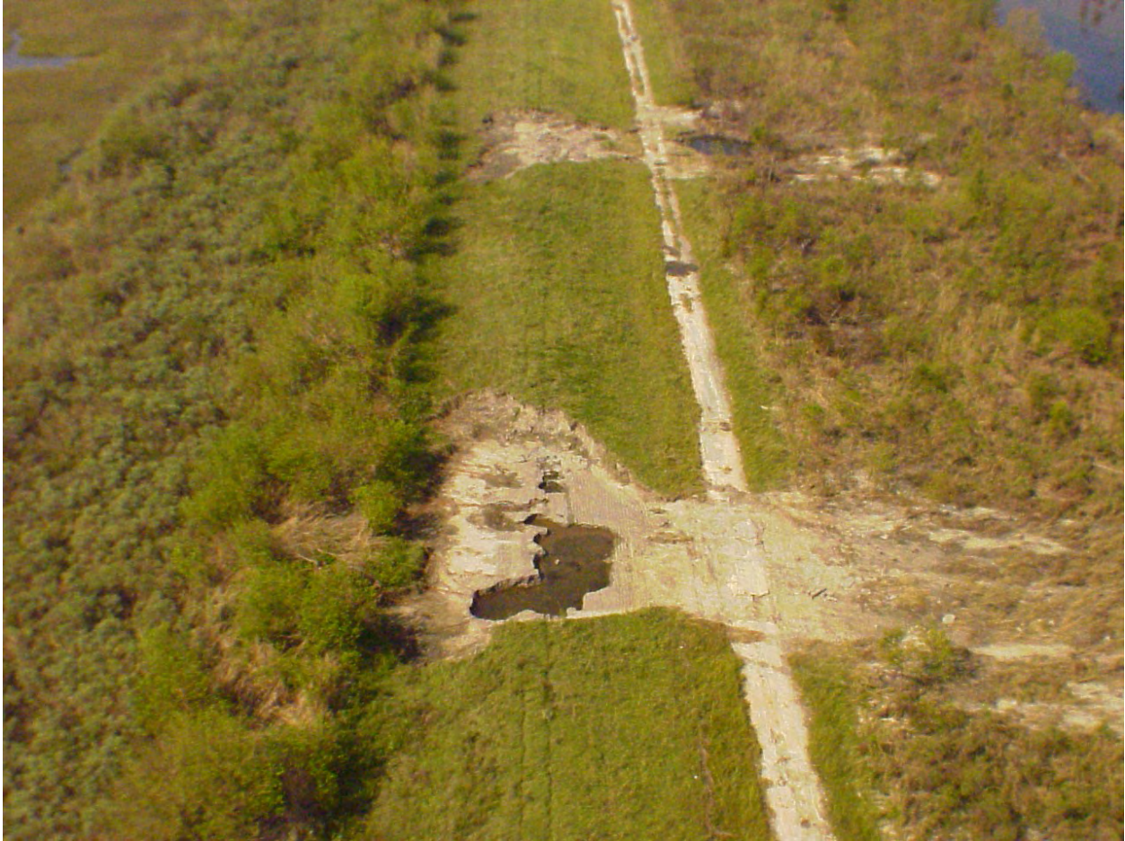
Figure 13-62. Partial Breach East of Pump Station 15
