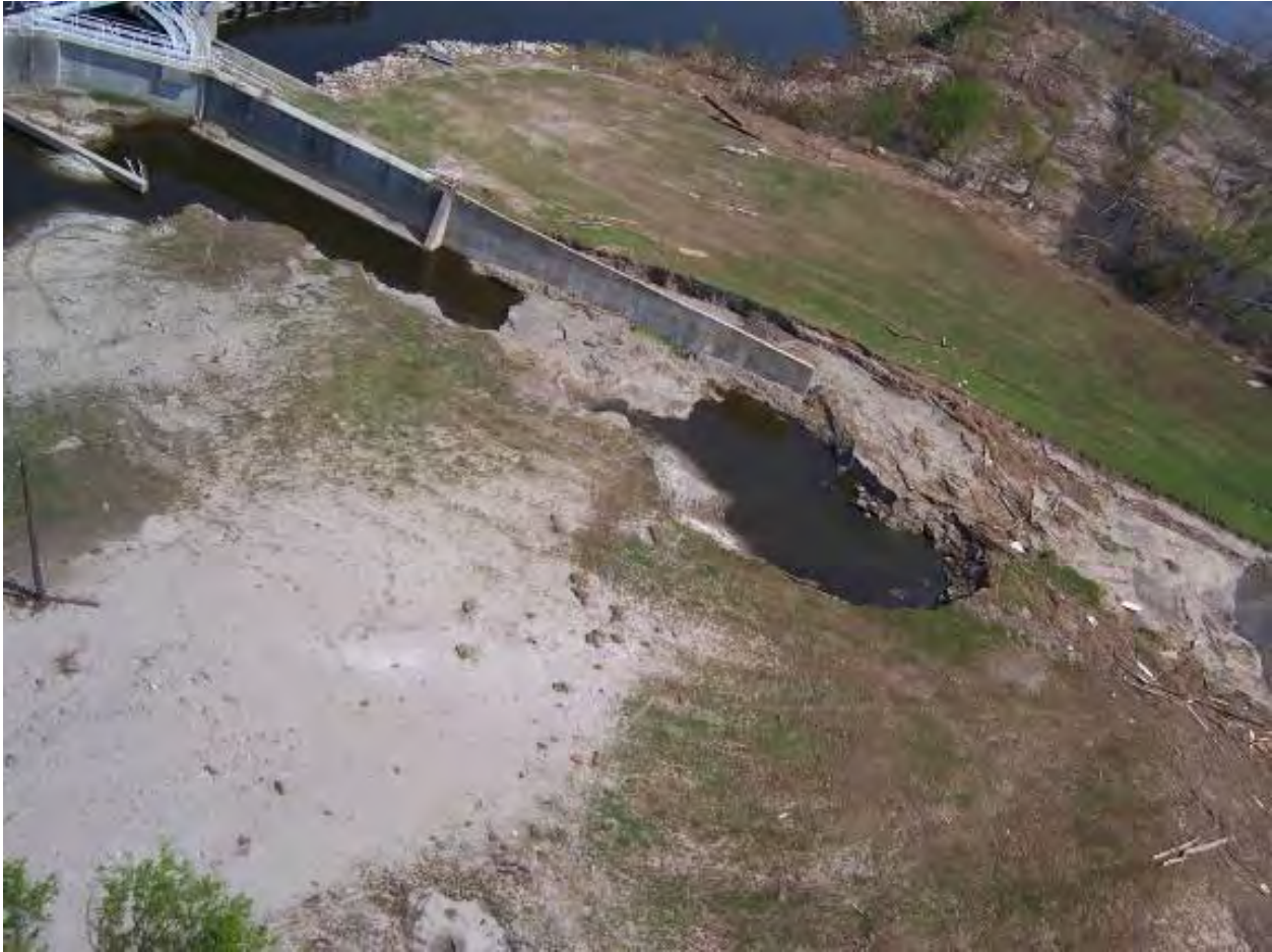
Figure 14-141. Severe Scour on East Side of Structure
