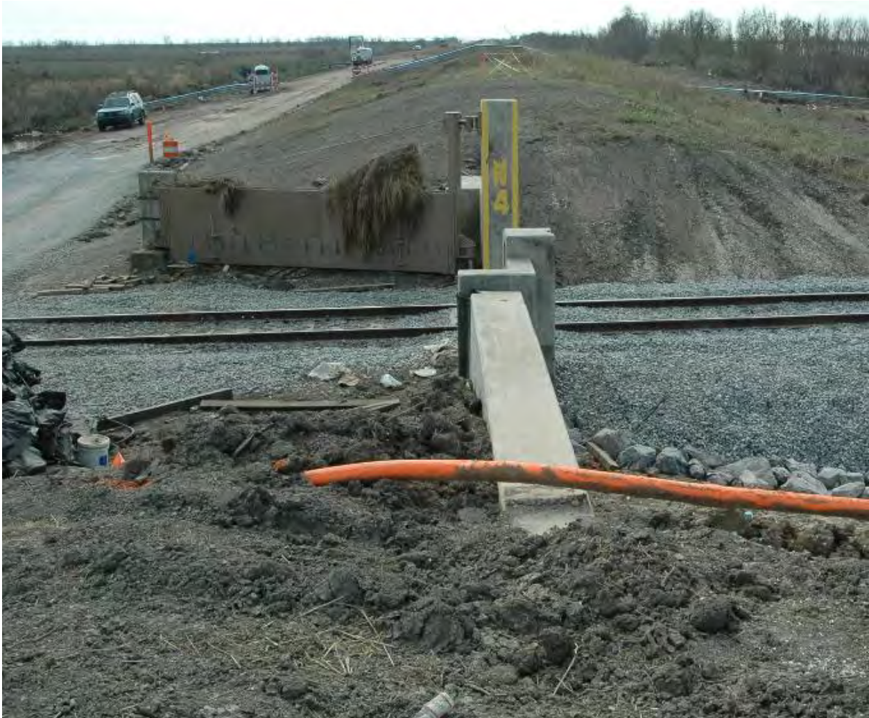
Figure 12-20. NOE5_C. Filled-In Scour Holes
