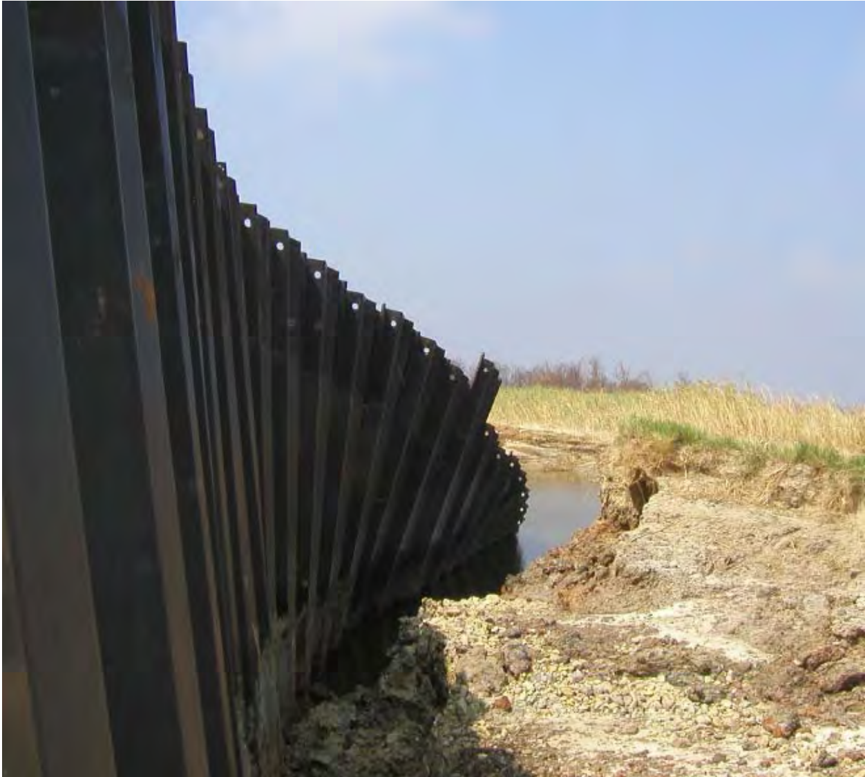
Figure 14-122. Closeup of Damaged Sheetpile and Scour. Note stratified layers in adjacent soil profile of existing hydraulic fill from the MRGO
