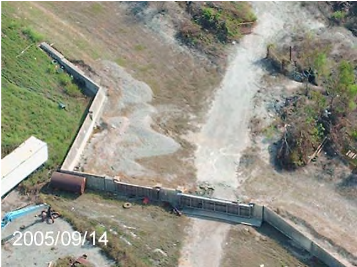
Figure 14-86. View of Scour Outside Gates S2 and S3. IHNC/GIWW and Southern Scrap sites are on the left side of photo
