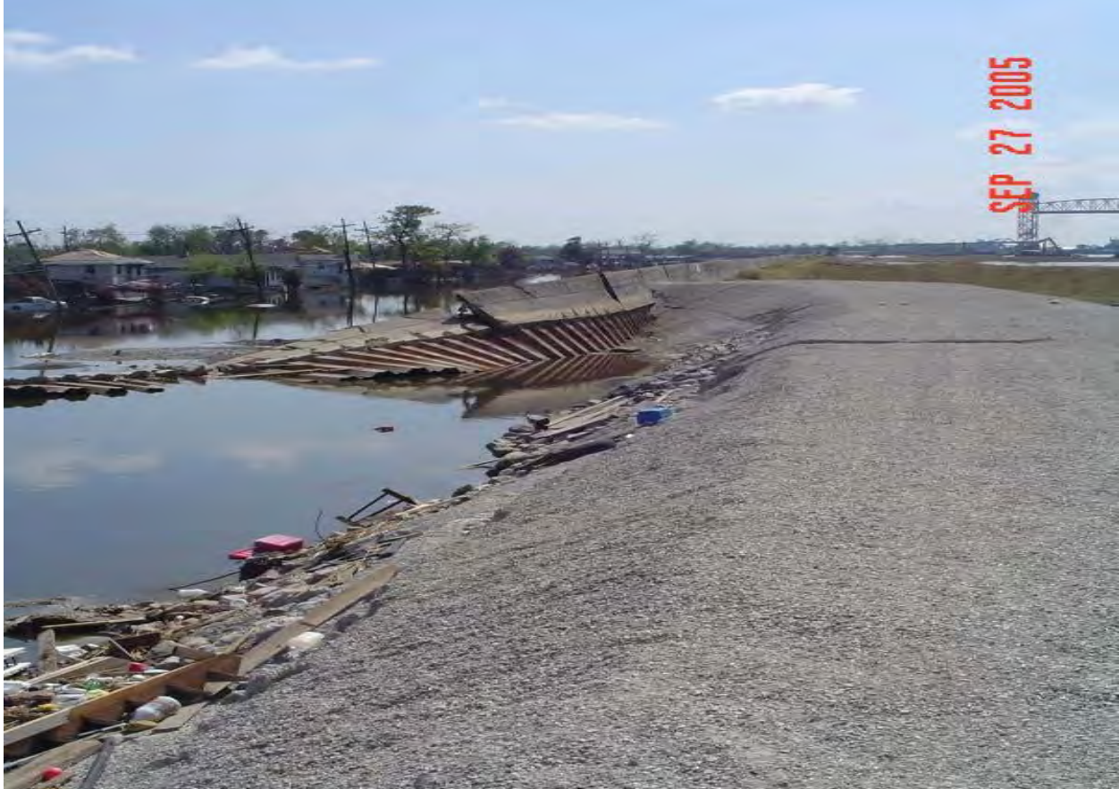
Figure 14-30. Southernmost I-Wall Failure Transition Between Florida Ave and Claiborne Ave.
