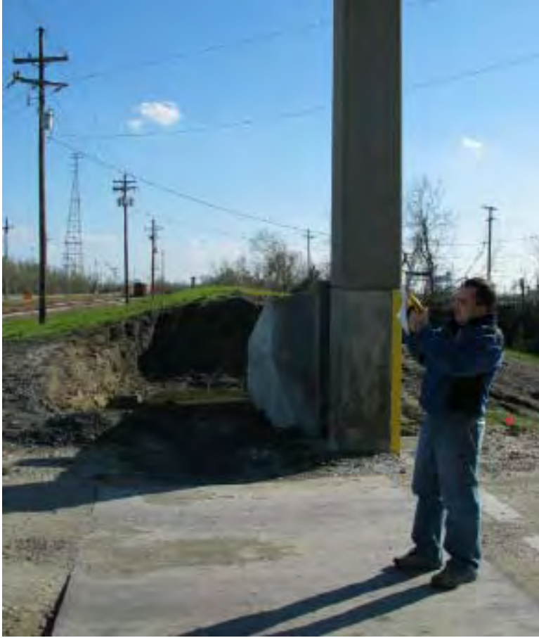
Figure 14-42. Gate E5 Looking South From Inside the Protected Area. Scour damage 7' (w) x 7' (d) around adjacent flood wall. Top of wall at gate is Elev. 13.2 +/-
