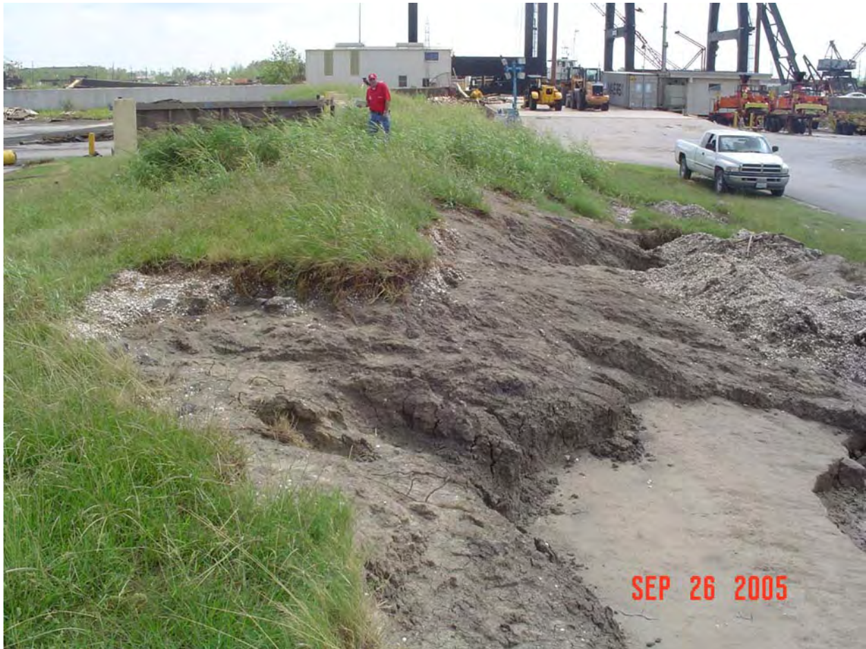
Figure 14-53. Overtopped Levee Section With Scour. View west from approximate CL Sta 14+00, B/L Sta 222+00
