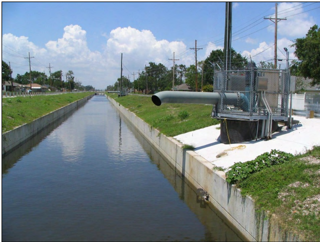
Photo 6. N. Cumberland Interior Pump at Interior Canal #4, W. Napoleon Ave.
