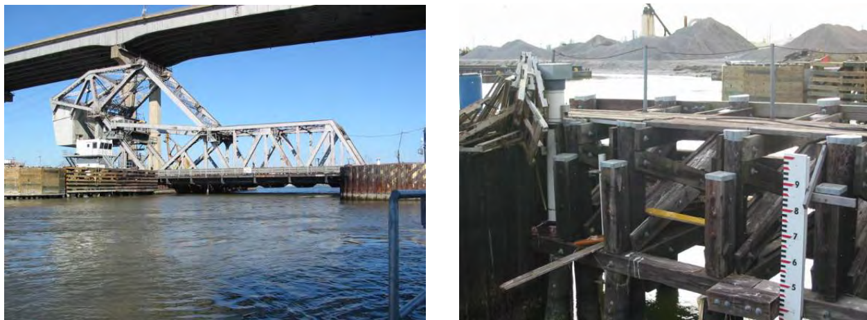
Figure 64. (Left) IHNC Almonaster Bridge—low chord elevation 3.51 ft NAVD88 (2004.65). (Right) Leveling to USGS recording gage and Orleans Levee District staff gage on I-10 bridge over IHNC
