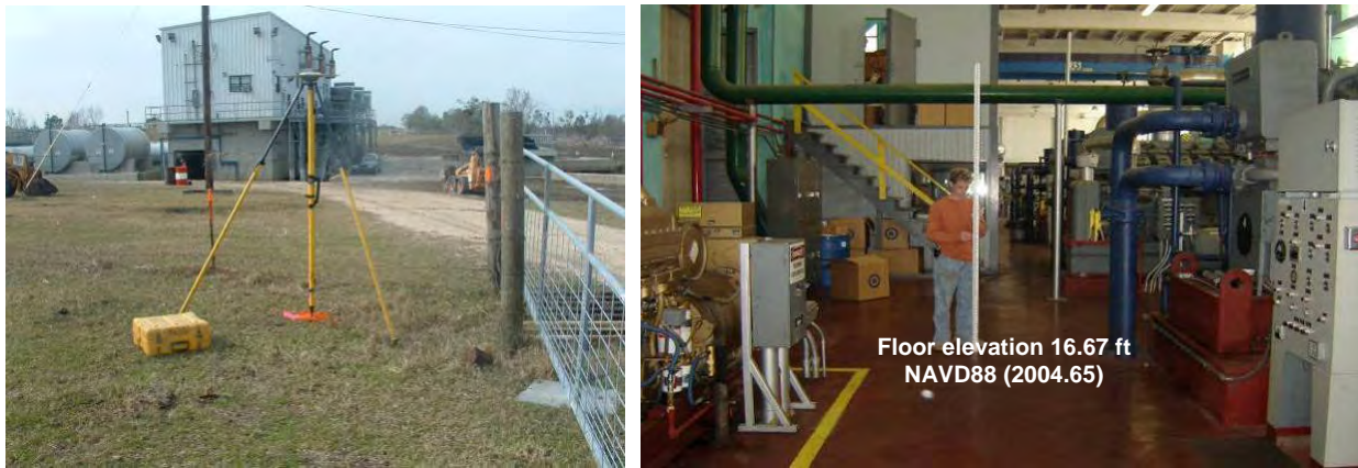
Figure 63. (Left) Static GPS survey to establish elevation on a benchmark outside a St. Bernard Parish pump station. (Right) Leveling first floor elevation inside Jefferson Parish Pump Station No. 3
