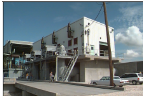
Post-Hurricane Katrina - View from the Inlet Canal
