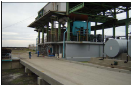
Post-Hurricane Katrina – View from the Inlet Canal
