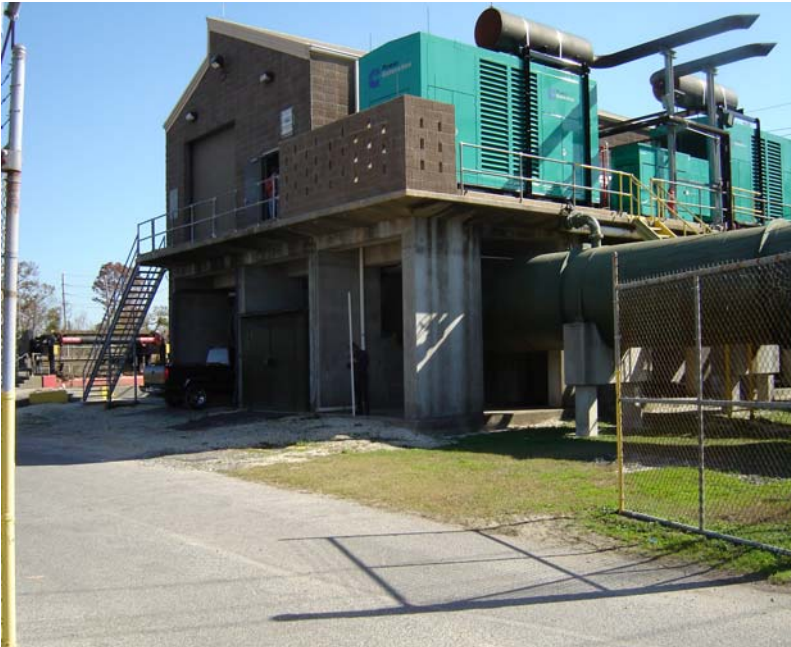
Parish Line Pump Station
