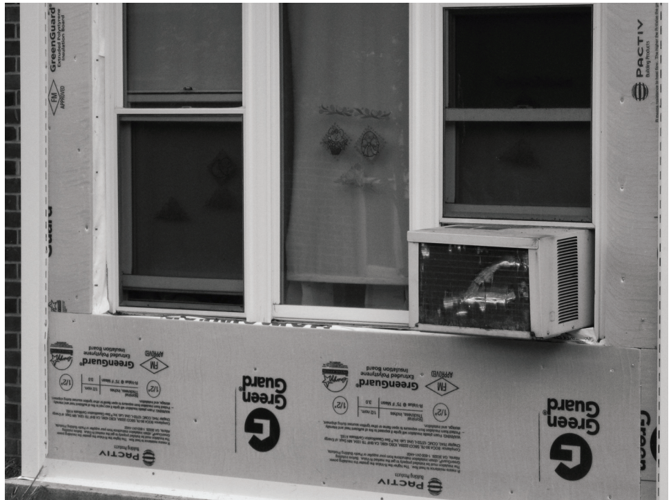
Figure 11: Siding in the process of completion using Rahway Housing Authority's Recovery Act funds
