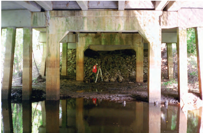
Figure 14. Composite bent at structure 262050103200 on U.S. Route 501, crossing the Waccamaw River in Horry County, South Carolina (from Benedict, 2003). (Photograph by the U.S. Geological Survey, South Carolina Water Science Center, June 13, 2000)
