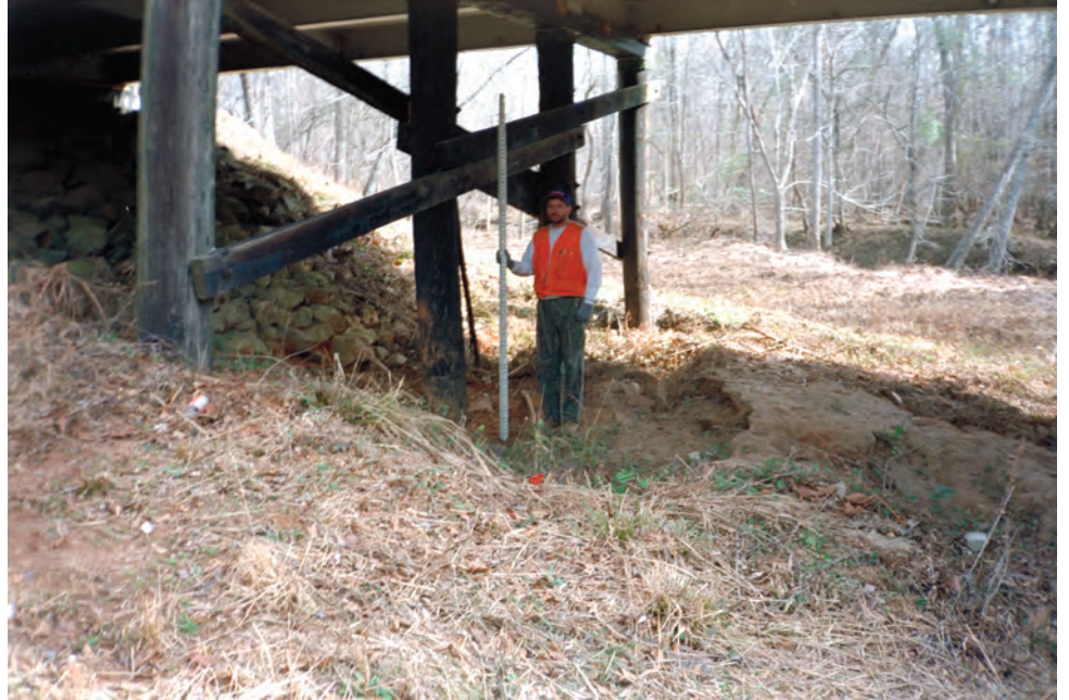
Figure 17. Timber pile bent at structure 194023000500 on S.C. Route 230, crossing Horne Creek in Edgefield County, South Carolina (from Benedict, 2003). (Photograph by the U.S. Geological Survey, South Carolina Water Science Center, February 6, 1997)
