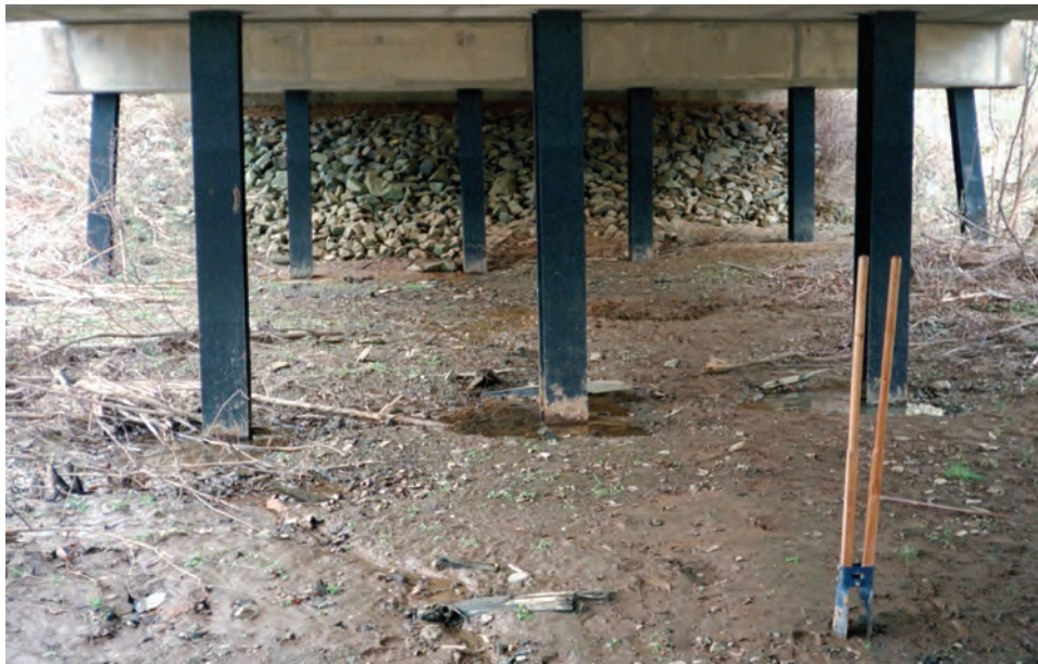
Figure 18. Steel H-pile bent at structure 467072100100 on Road S-721, crossing Taylors Creek in York County, South Carolina (from Benedict, 2003). (Photograph by the U.S. Geological Survey, South Carolina Water Science Center, January 29, 1997)
