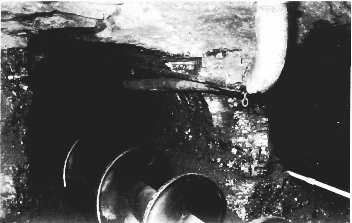
Figure 2.—Inert gas stub pipe used to direct inert exhaust into the hole. Note small-diameter pipe used for collar measurements.
