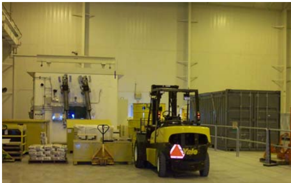
The challenging WMF facility – hot cell, overhead crane, and under floor storage)
