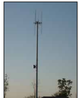
Figure 8 - Antenna Tower and Antennas.
