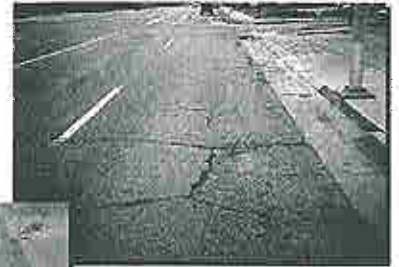
Deteriorating Pavement (e.g., potholes, cracks)
