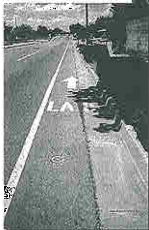
Poor Condition of Pavement Markings
