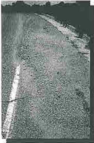
Glass, Gravel or Sand in Roadway
