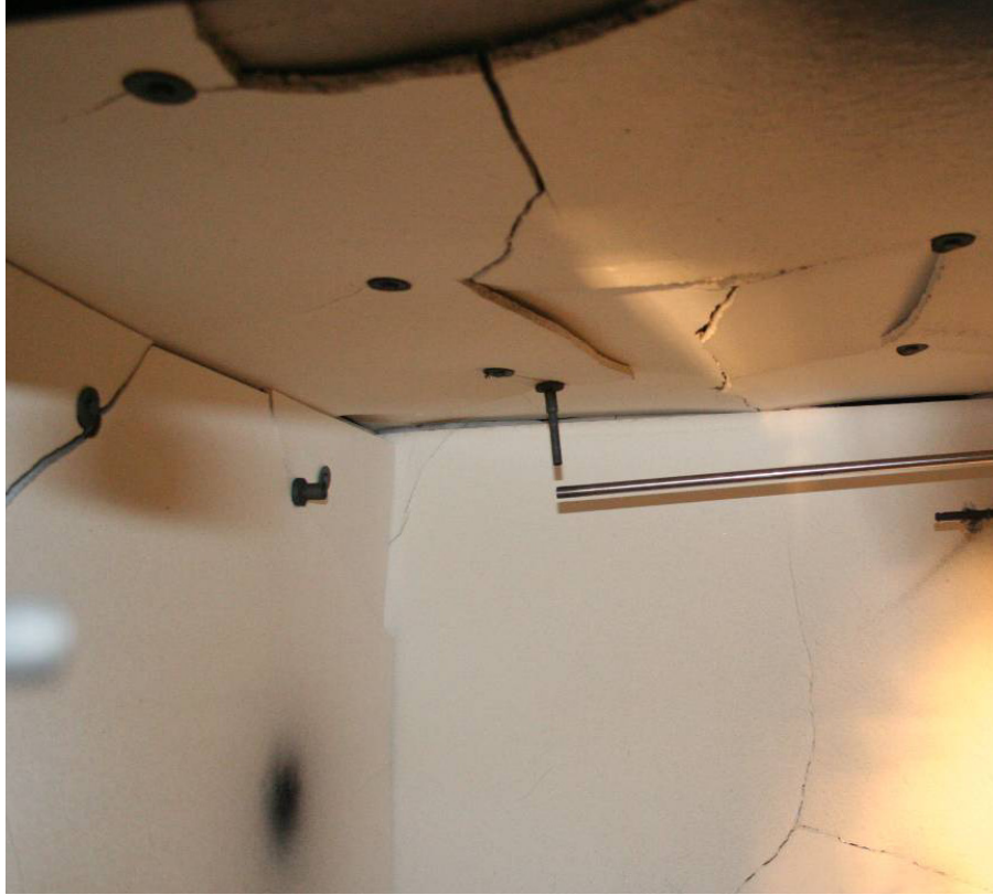
Figure 66. Photo inside enclosure after test #6 showing Marinite I condition. Large chunks of ceiling fell to the floor during this test.
