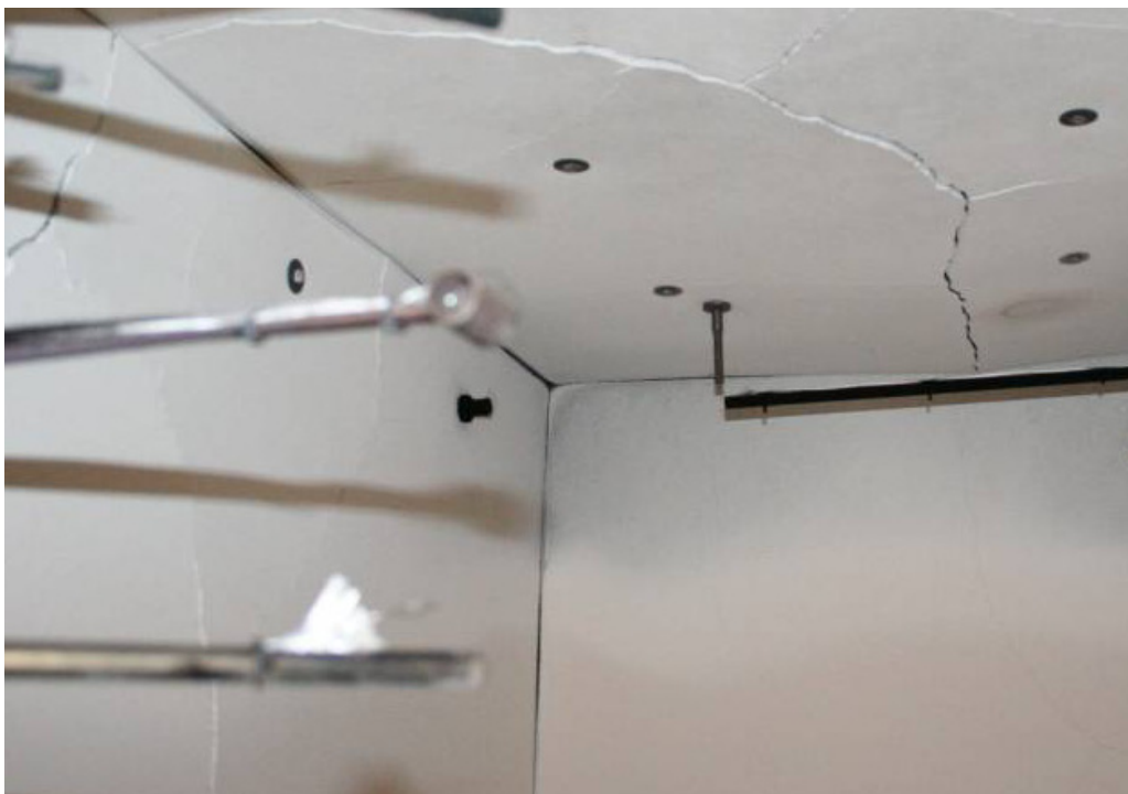
Figure 65. Photo of rear gas sample location and Marinite I construction after test #2 with natural gas.
