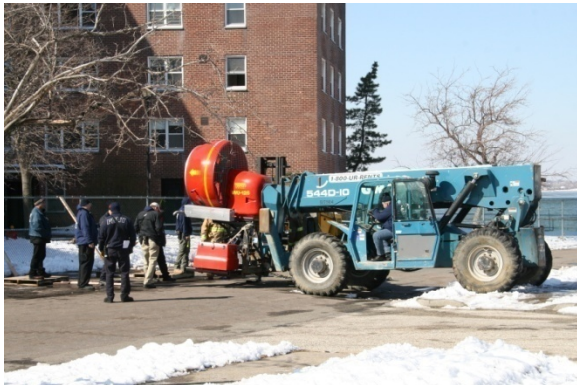
Figure 1.3-1. MVU on Lift
