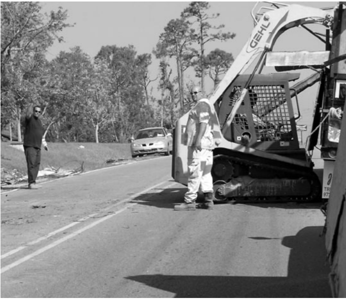
Figure 5: Work Zones with Equipment Not Protected from Traffic by Safety Cones
