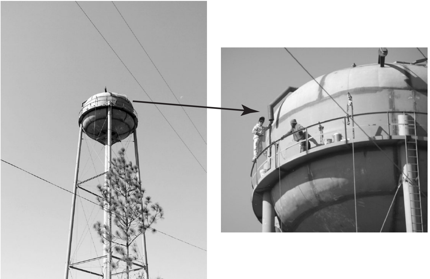
Figure 6: Workers on a Water Tower without Fall Protection Such As Guard Rails or Safety Harnesses
