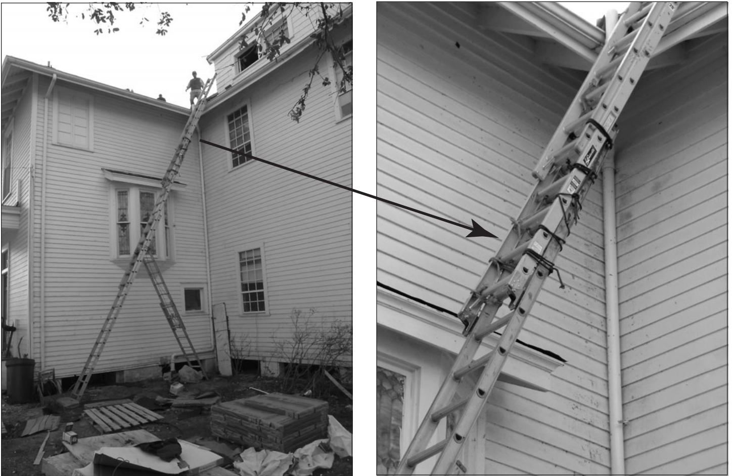
Figure 7: Workers on a Roof without Safety Harnesses and with Poorly Secured Ladders
