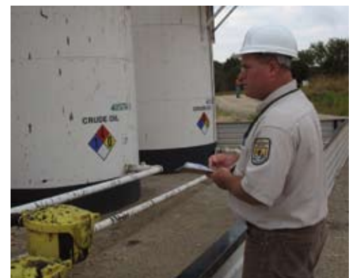
Fire Effects Monitor Craig Hoffpauir examines tank battery equipment during a site visit at last year’s oil and gas course held at Hagerman National Wildlife Refuge Complex in Texas. (USFWS)
