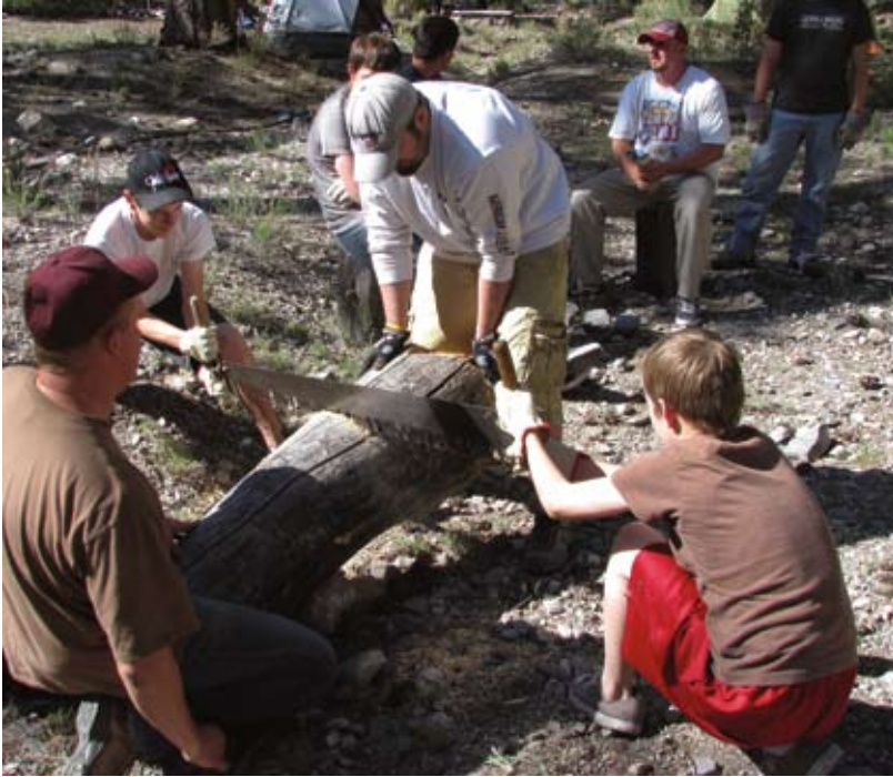
Boy Scouts help repair a remote log cabin at Desert National Wildlife Refuge in Nevada. (USFWS)
