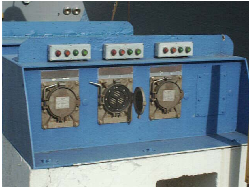
Figure 13-7. 480 Volt Pier Electrical Outlet Assembly Without Cable Connections
