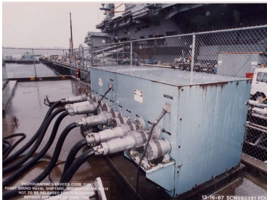
\2\ Figure 13-8. 4.16 kV Pier Electrical Outlet Assembly and Outlets – Existing Installations /2/
