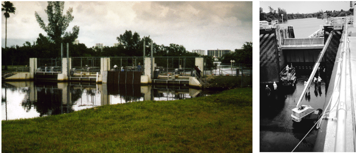
Figure 14. Water control structure retrofitted with pressure sensitive technology (left). Retrofitting of St. Lucie Lock with acoustic sensors (right) to protect manatees from being crushed as the gates close. ( Photographs by FWS and B. Brooks )
