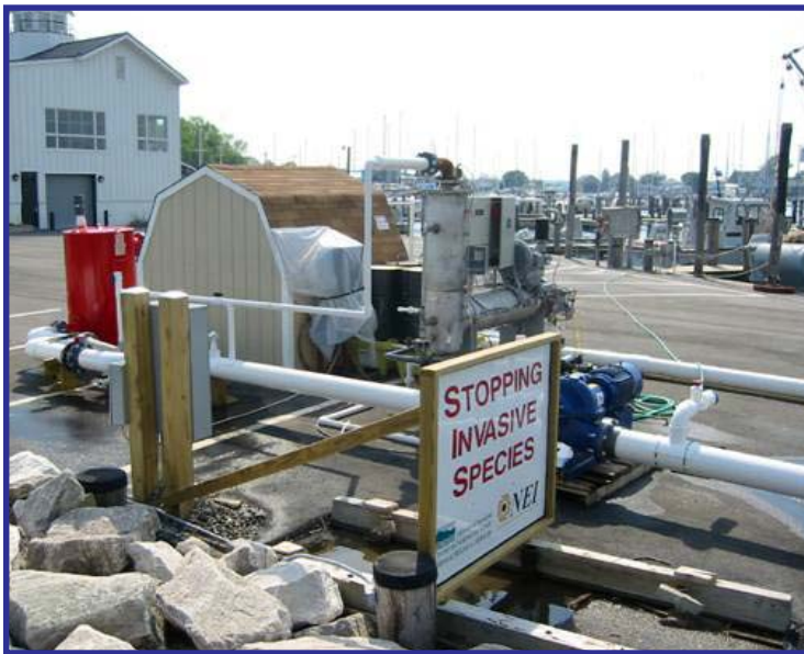
Pilot-Scale VOS System at the Chesapeake Biological Laboratory
