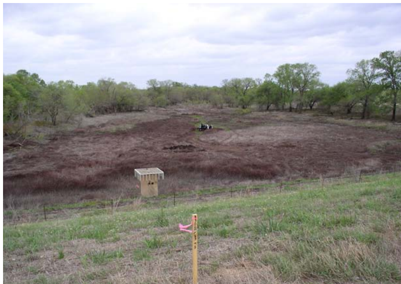
The flood pool of Calaveras Creek Dam No. 6, although dry now, provides flood protection downstream. Rehabilitation to meet current safety standards will require the following: raising the top of the dam, adding an additional principal spillway, adding an impact basin and modifying auxiliary spillways.
