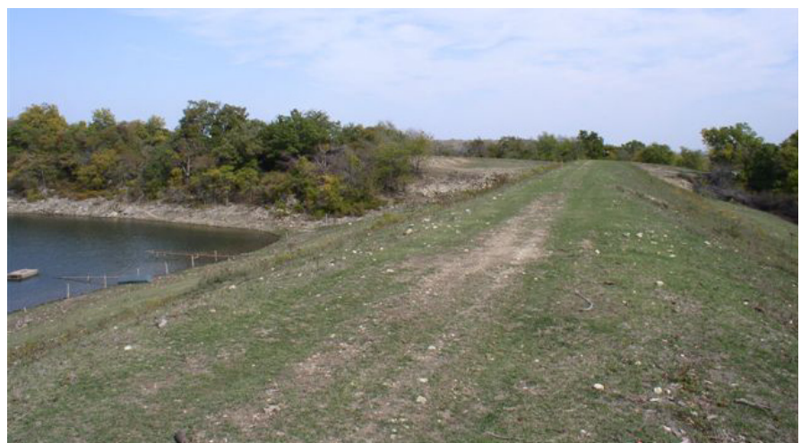
Upper Clear Boggy Watershed Dam No. 35 traps sediment that would otherwise end up in Dam No. 34, located downstream.
