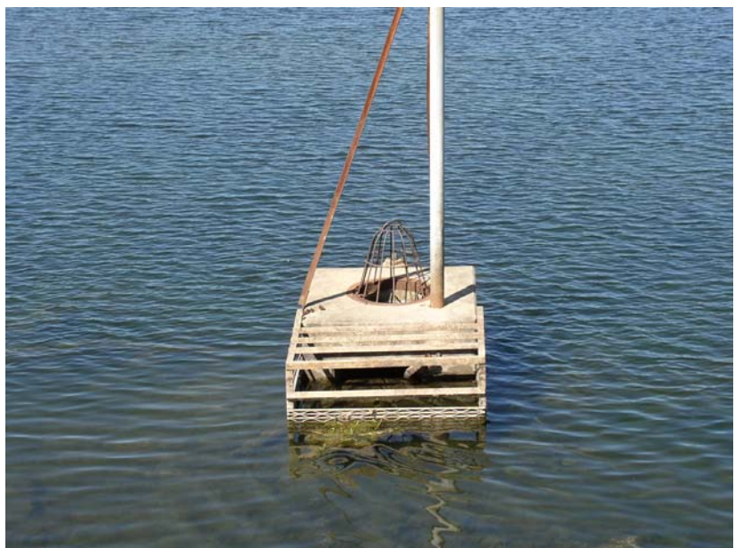
The existing principal spillway inlet on Upper Clear Boggy Watershed Dam No. 34.
