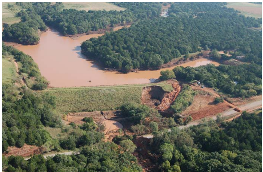
Damage to Sugar Creek Watershed Dam No. L-44 as a result of 8.3+ inches of rain in a 6-hour period in August 2007.
