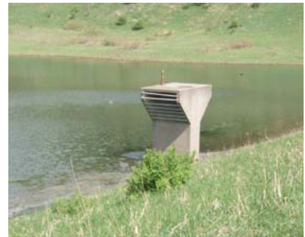
Two stage riser and flood pool after rehabilitation; this will protect 150 downstream residents.
