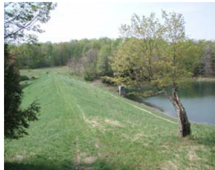
Earthen dam to be raised to meet modern safety criteria at Conewango site 6.
