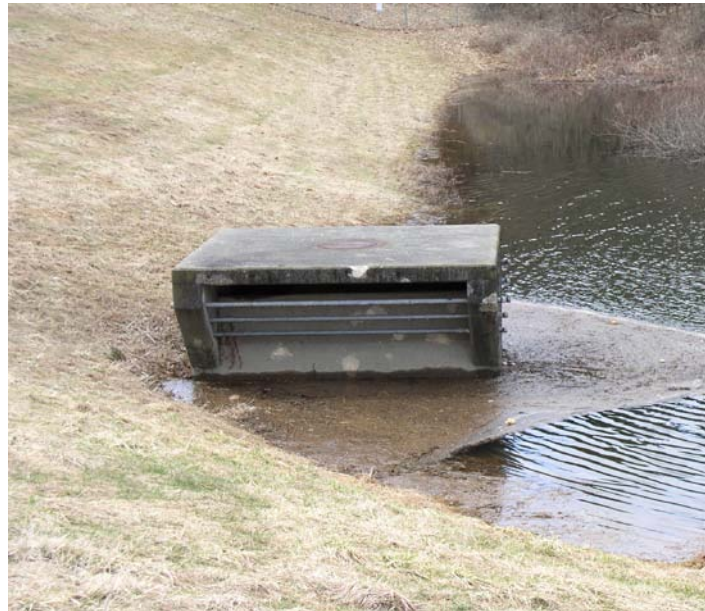
The water control structure at the Hop Brook dam.
